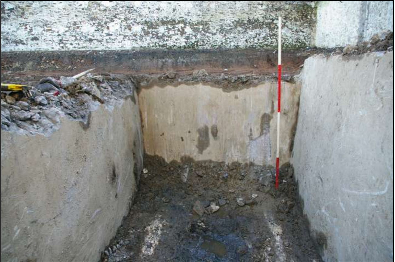
Figure 11: Internal shot of the concrete structure; viewed from the west (2m scale).
