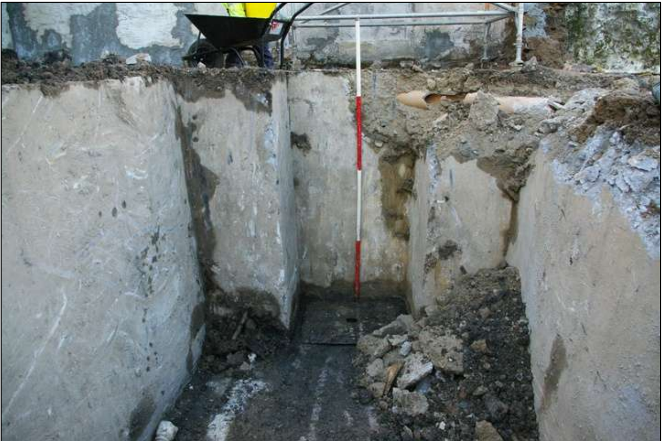
Figure 12: Internal shot of the concrete structure; viewed from the east (2m scale).
