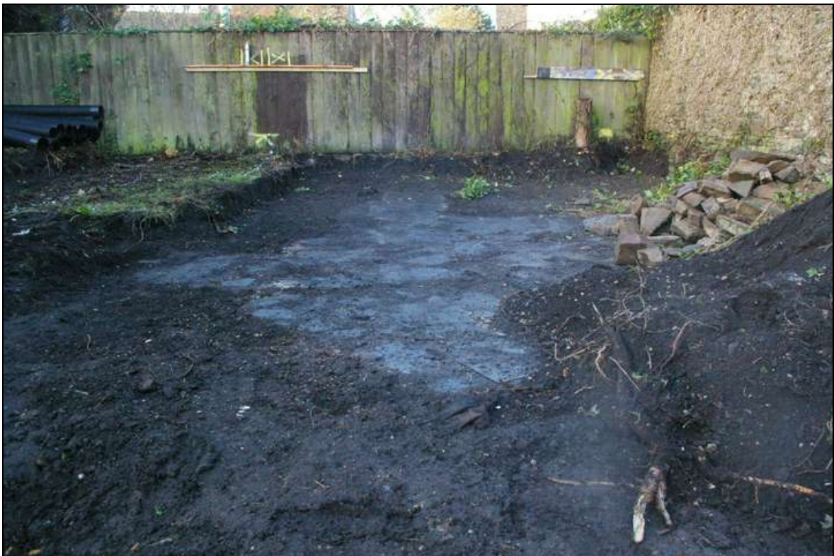
Rear garden of 13 High Street, Torrington, post topsoil strip; looking north (no scale).
