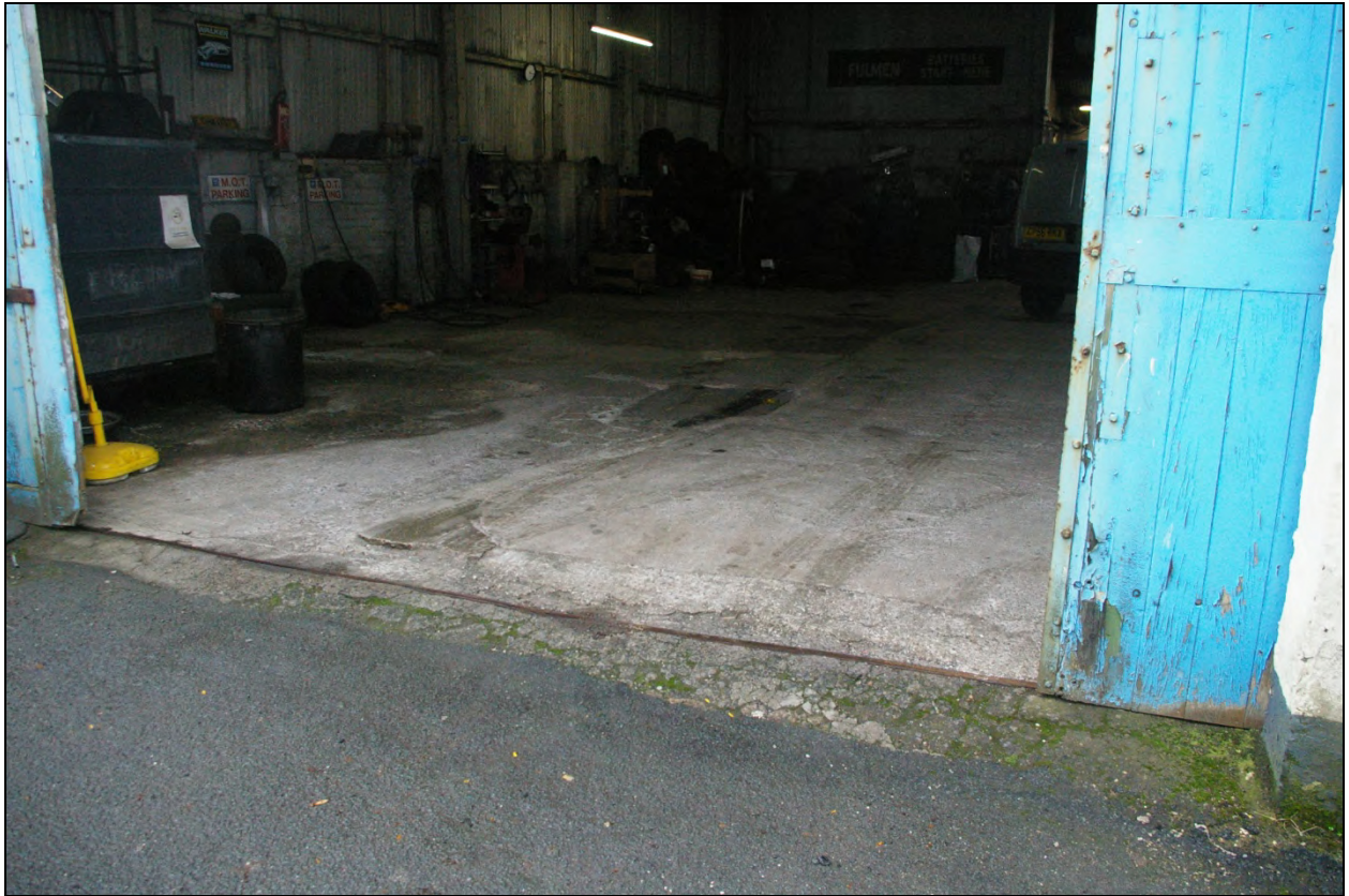
View showing the raised concrete floor level, within the site, in comparison to the levels along Park Row; from the east, north-east.
