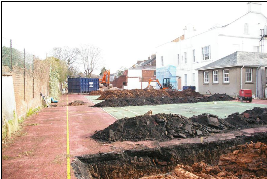
Site shot, west half of site, viewed from the west (no scale)
