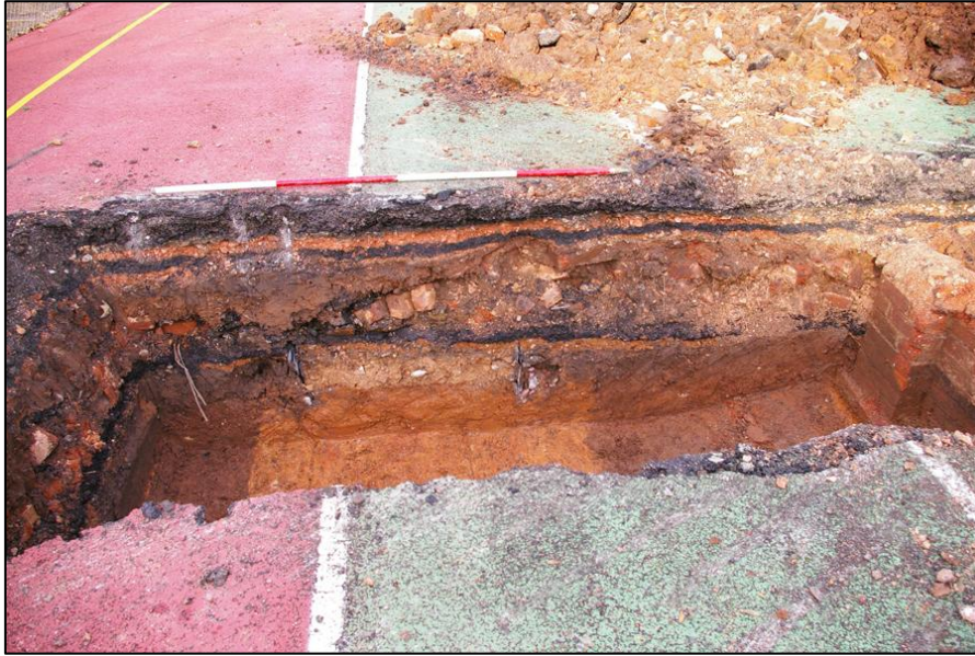
South facing section, west end of Trench 3, viewed from the south (2m scale).
