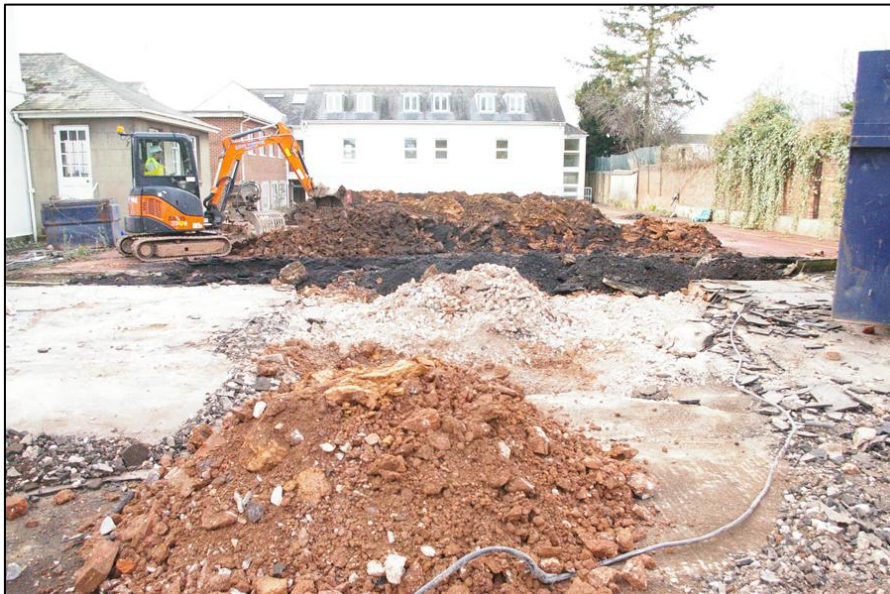
Site shot, west half of site, viewed from the east (no scale)
