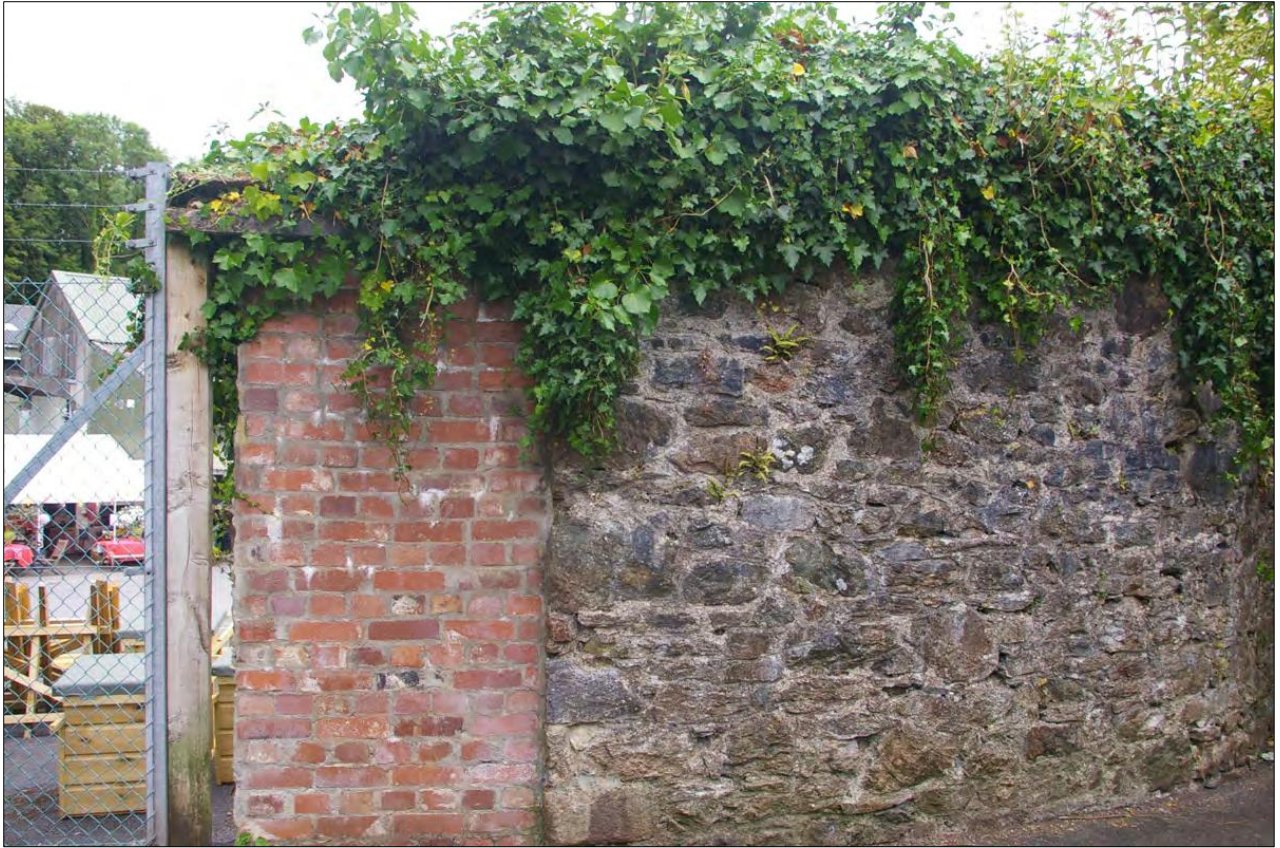
The blocked opening, now demolished on its northern side; from the north-west.
