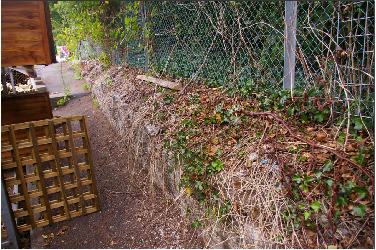
View along the surviving section of stone wall in the north-west corner of the site; from north.
