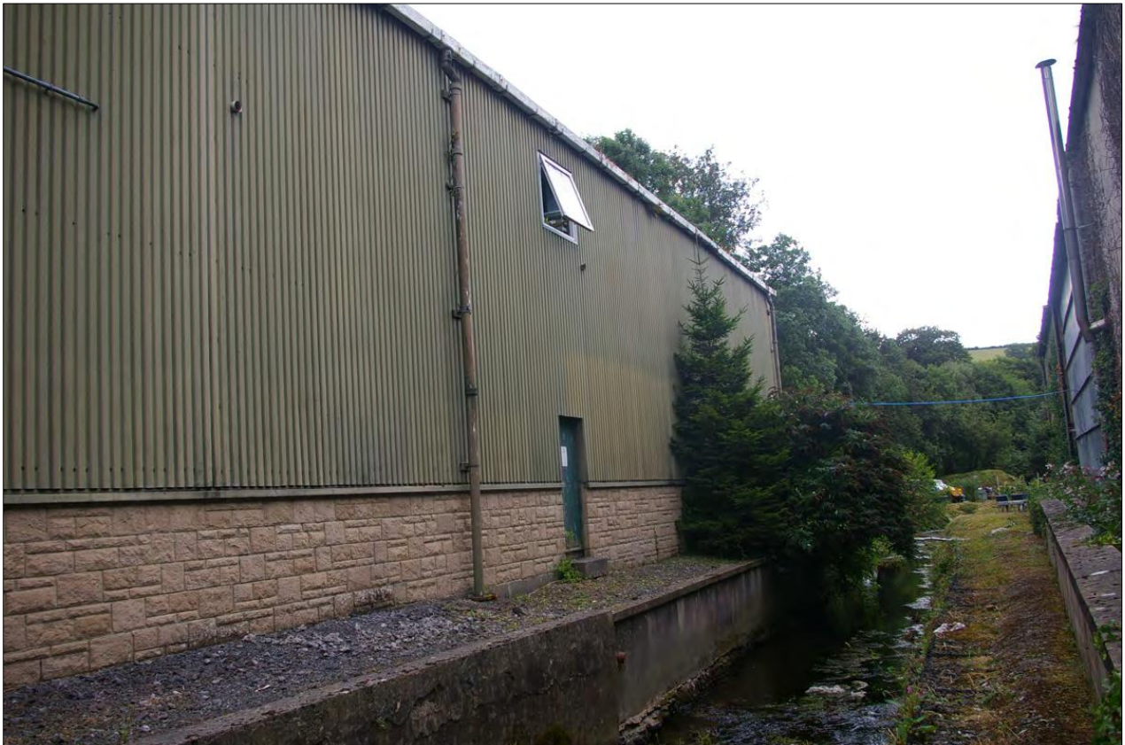
View along the back of the building on the east side of the river bank; from the north-west.
