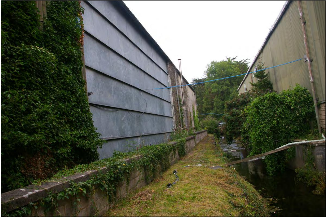
View along the back of the northern part of the main range of buildings; from the south-east.
