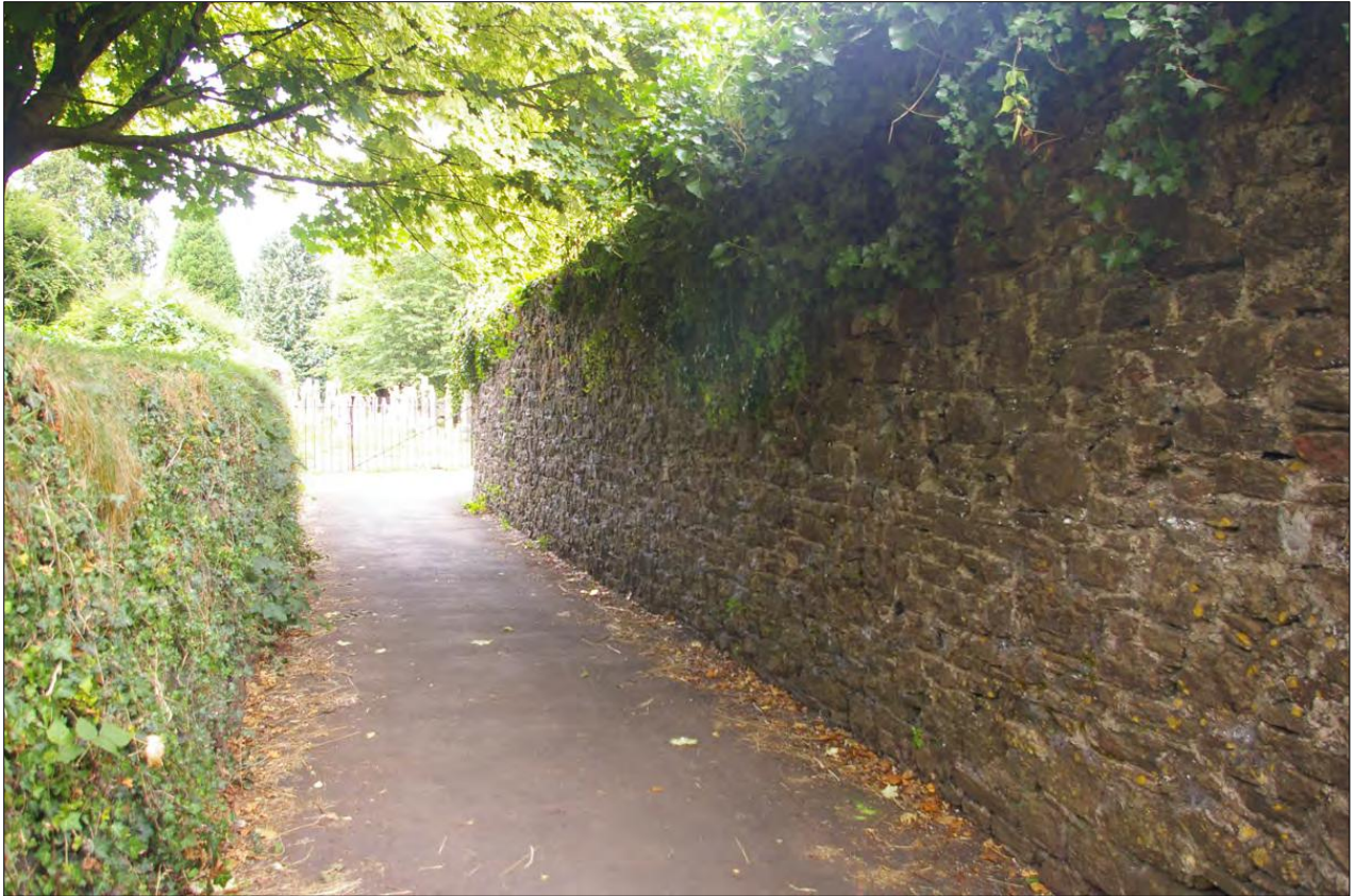
View along the section of stone wall on the western boundary; from the south-west.
