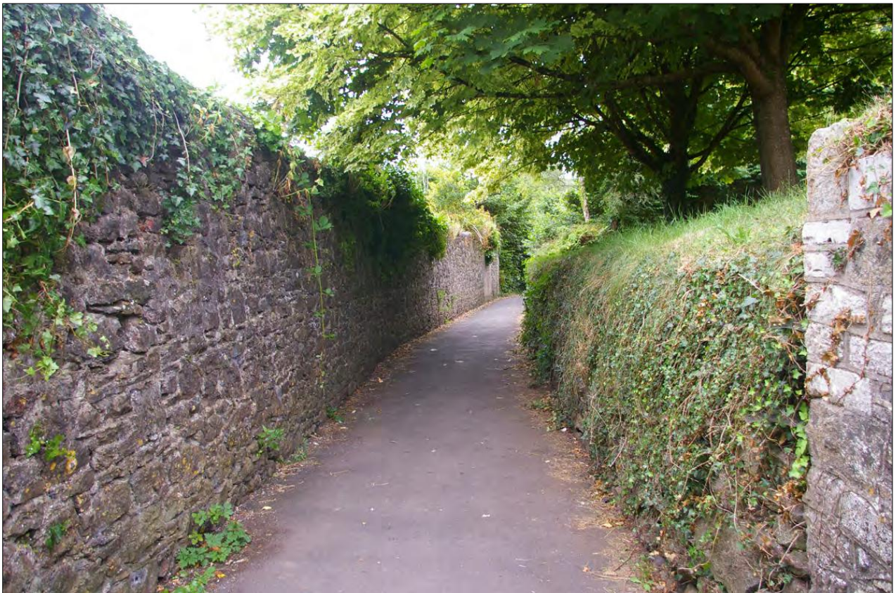
The length of the stone wall, on the western boundary; from the north.
