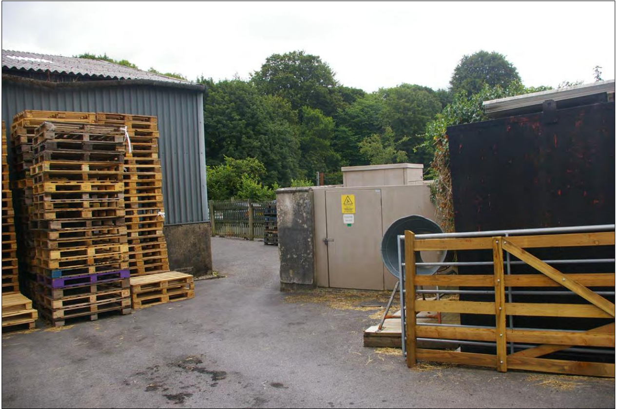
View down to the southern boundary, showing the sub-station; from the north-west.
