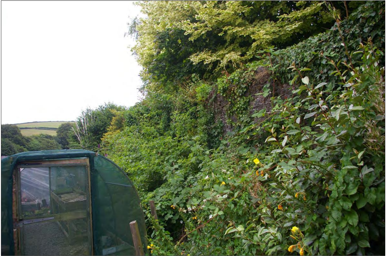
View of the inner face of the section of stone wall along the western boundary; from the north-east.
