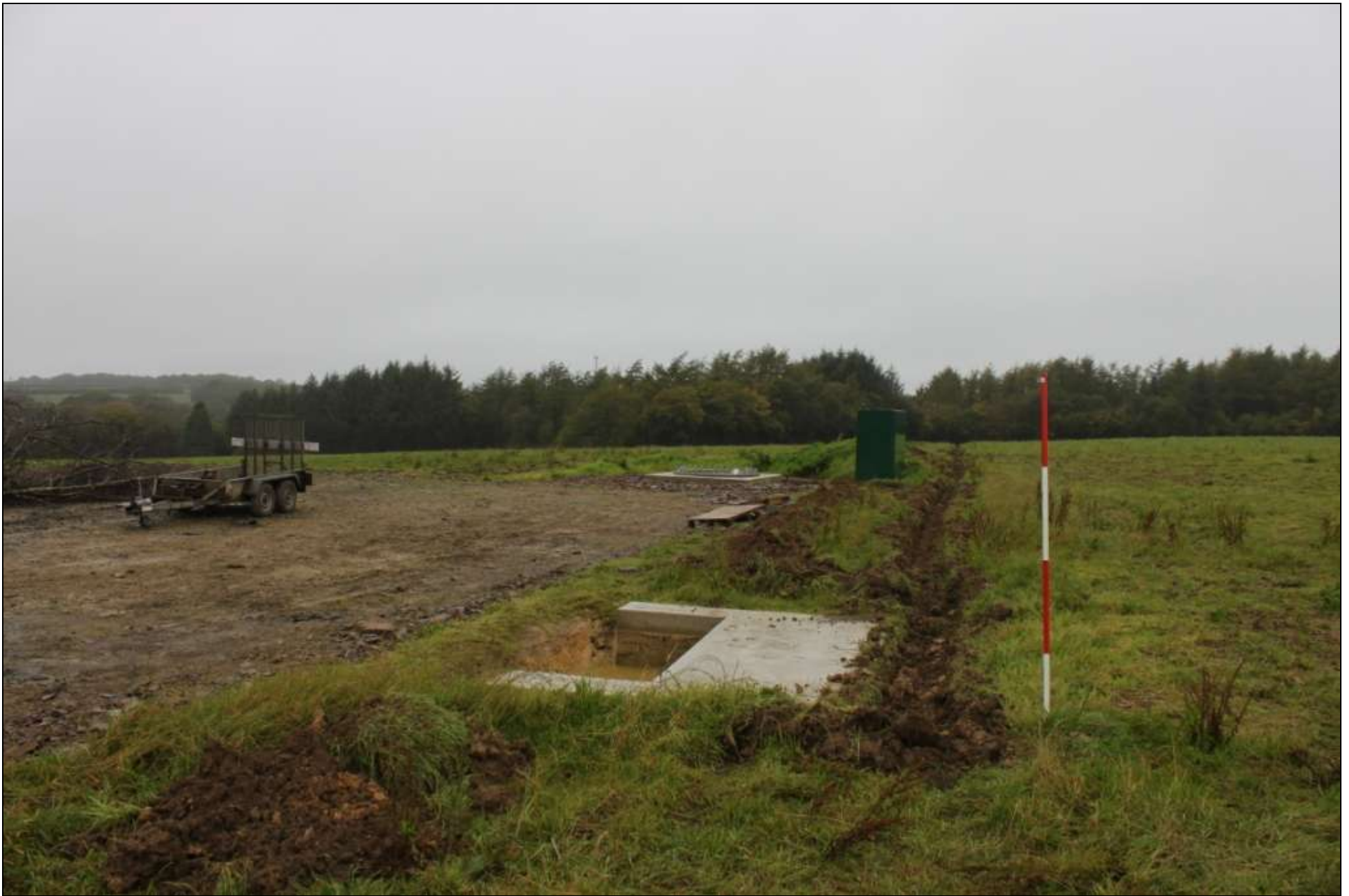
Figure 3: Shot of the cable trench in Field 3, the turbine base and transformer are visible in the centre of the photo, viewed from the south-east (2m scale).
