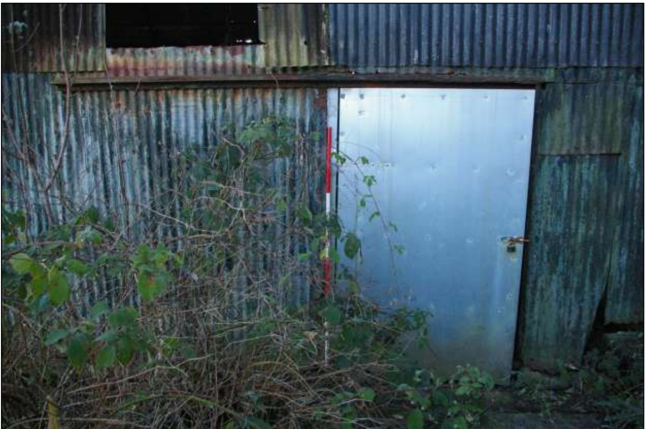
Figure 29: Detail of the door and rails in the north elevation; viewed from the north (scale 2m).
