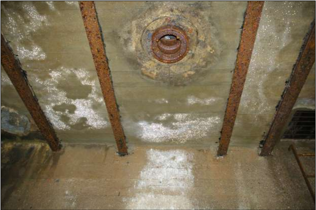
Figure 88: The iron collar for the vertical shaft of the turbine, in the ceiling of the chamber; viewed from the east (no scale).
