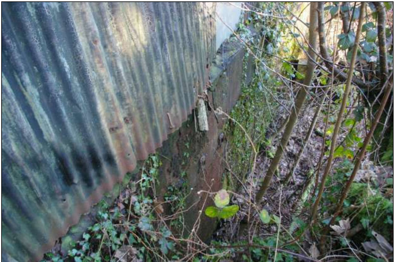
Figure 72: The base of the south elevation of B1 where the ground level steps down; note the DOULTON brackets in the wall. Viewed from above and to the south-west (no scale).
