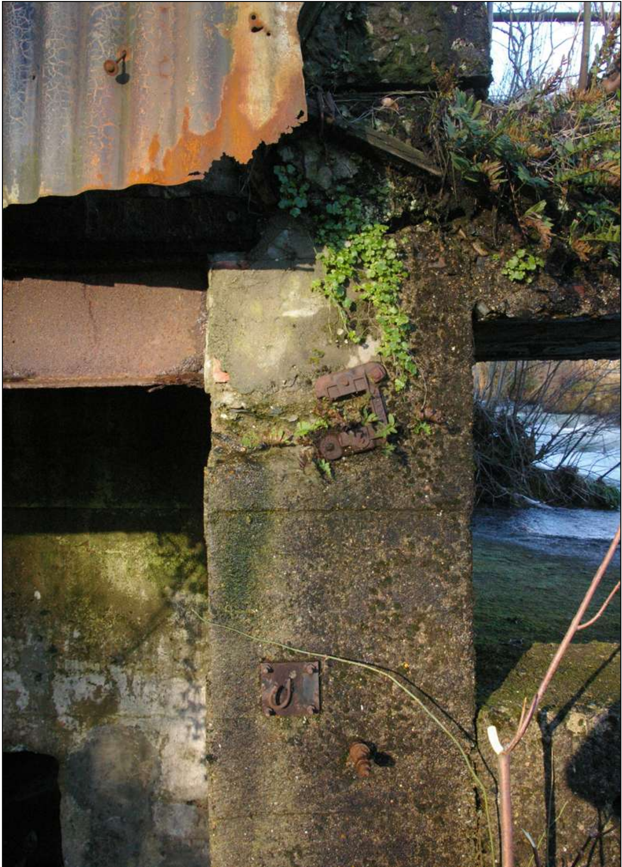
Figure 70: The south face of the east wall of the turbine chamber, showing the later iron fittings and inserted iron girder; viewed from the south (no scale).
