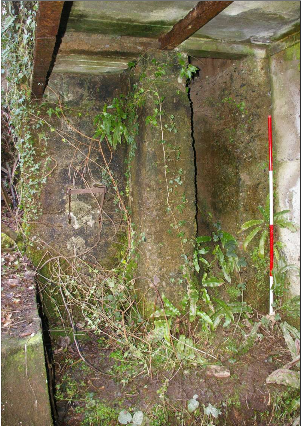
Figure 80: The west wall of the turbine chamber, showing the potentially earlier mass concrete plinth; viewed from the south-east (scale 2m).
