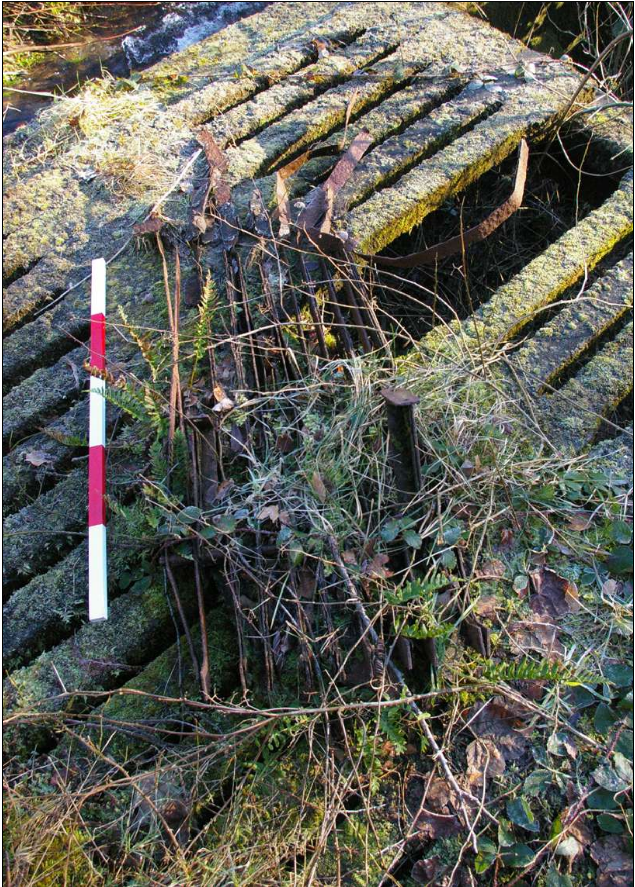
Figure 103: Detail of one of the filter screens at the site.
