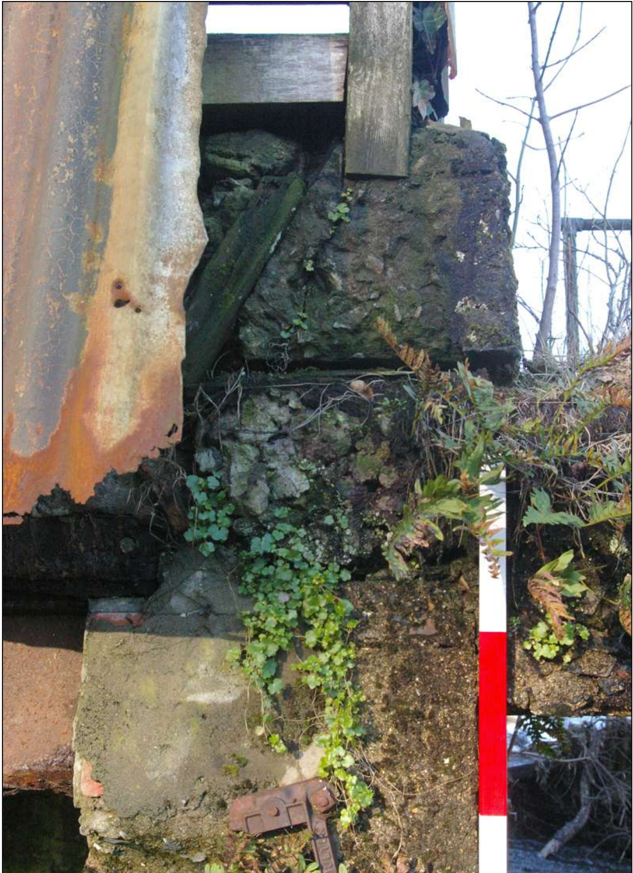
Figure 75: Detail of the south-east angle of B2, showing the raises in the concrete; viewed from the south (scale 1m).
