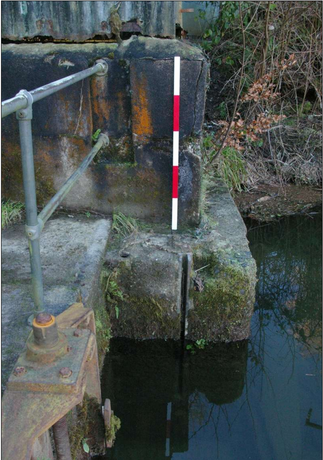
Figure 33: North-east angle of B1, showing the former sluice gate slot; viewed from the east (scale 1m).
