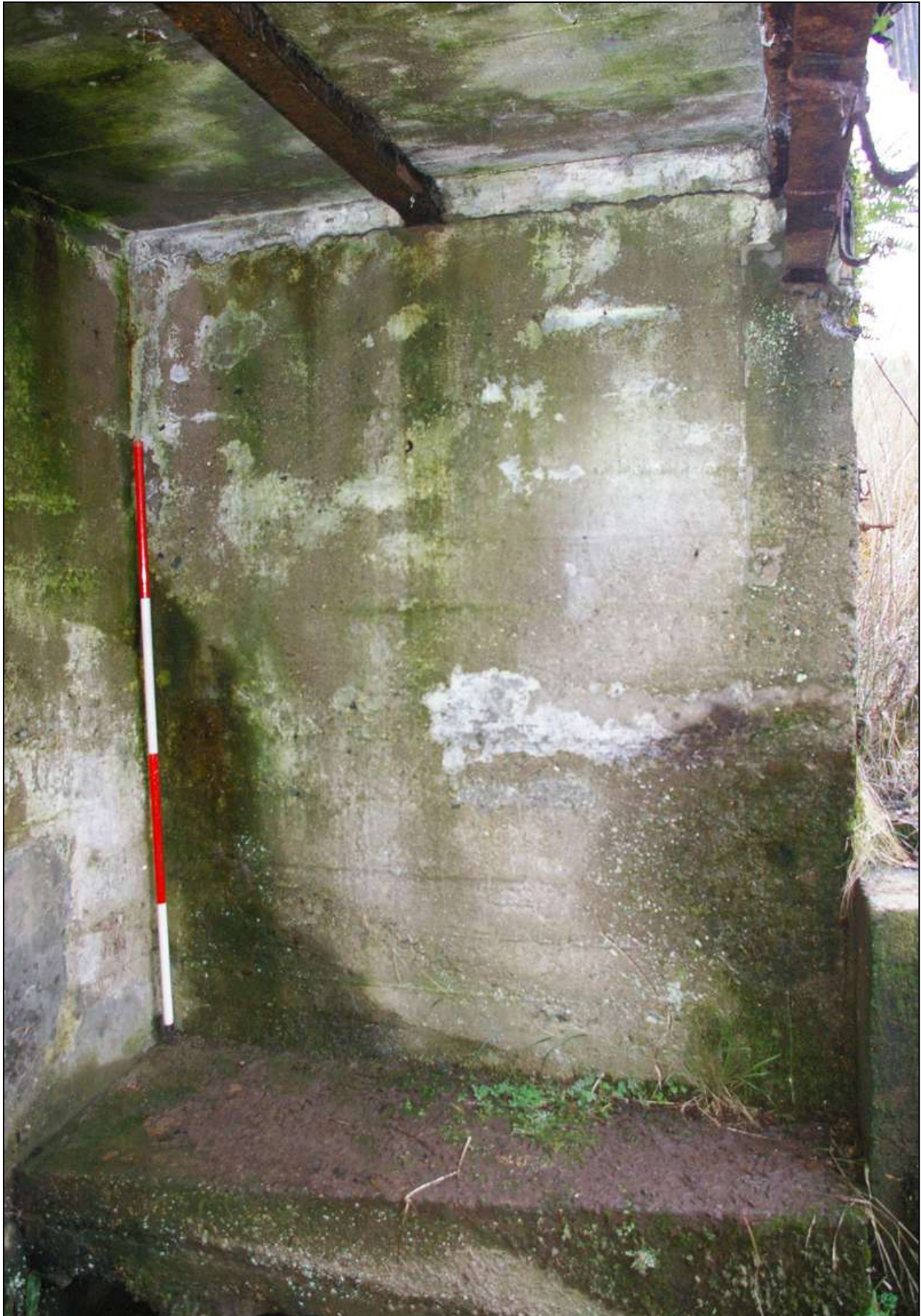
Figure 82: The east wall of the turbine chamber, viewed from the south-west (scale 2m).
