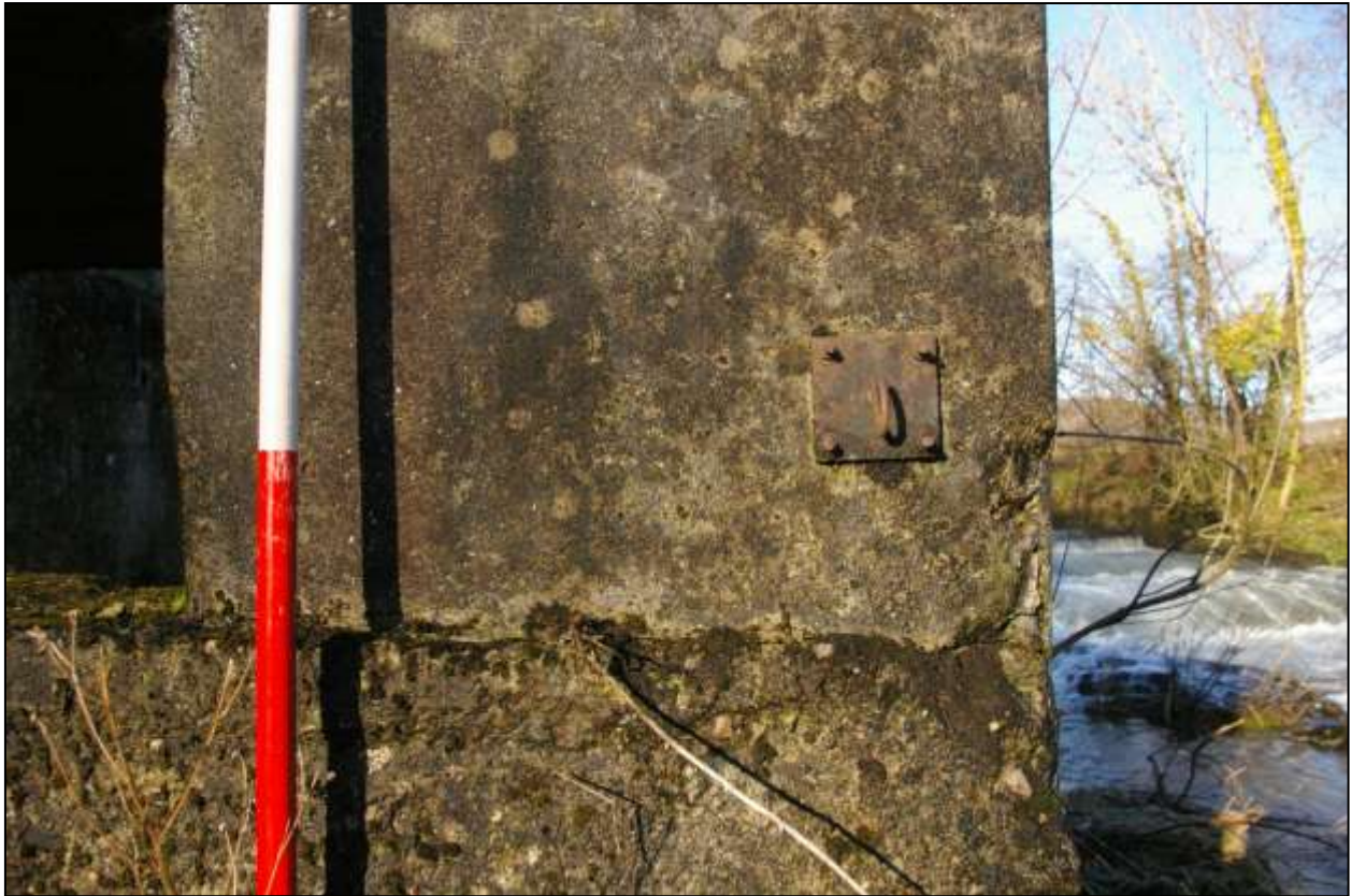
Figure 67: As above, detail of a hook and plate on the southern pillar; viewed from the south (scale 2m).
