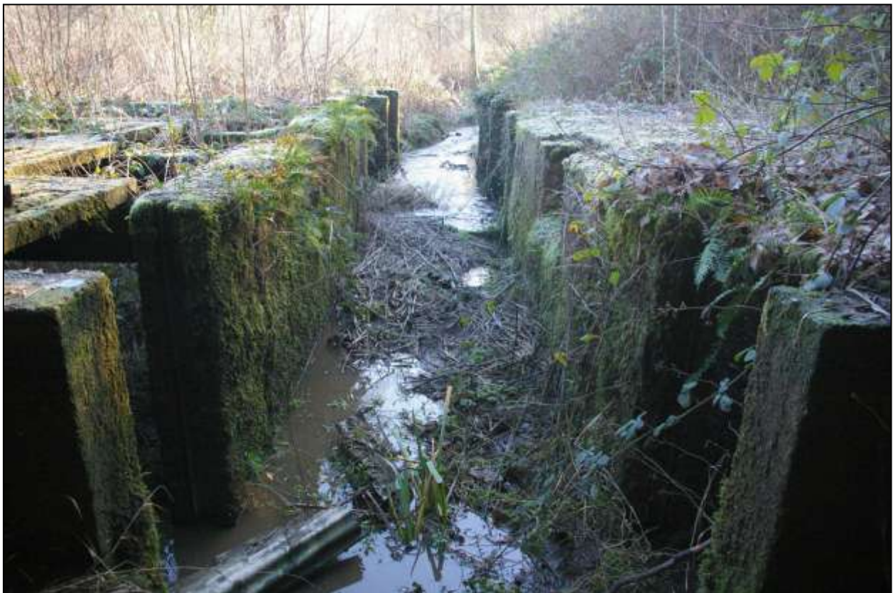
Figure 93: View along the fish tanks from the entrance to the turbine chamber; viewed from the north (no scale).
