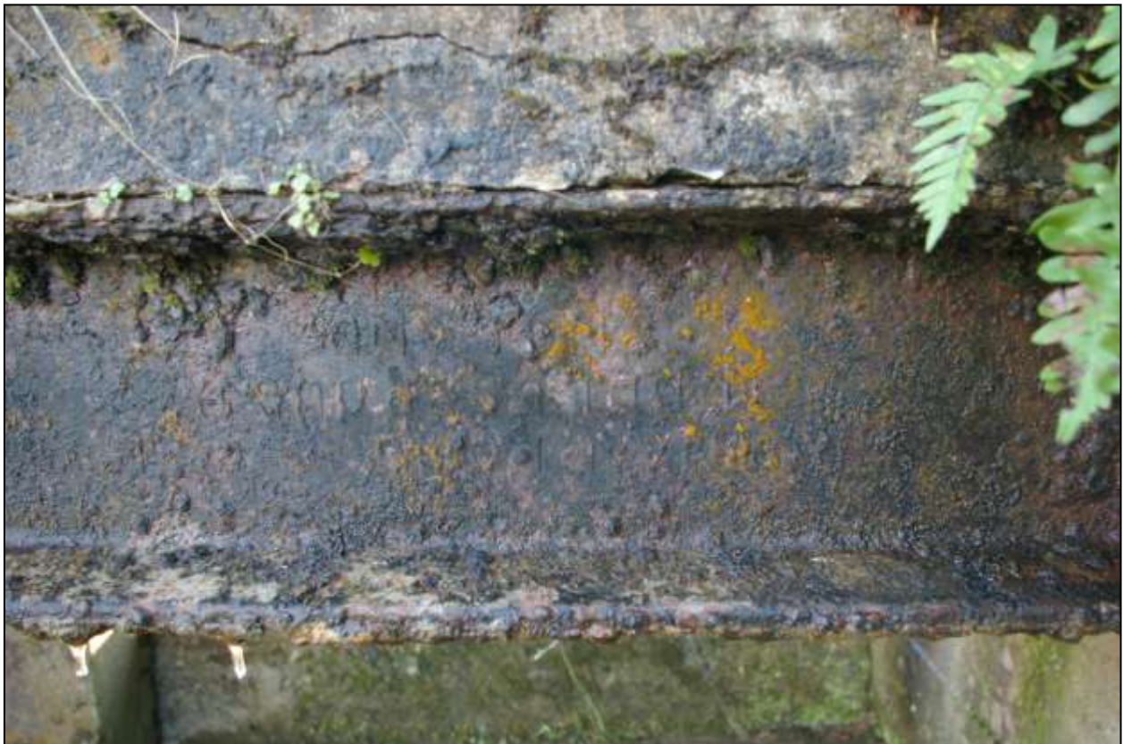
Figure 57: As above, detail of the name on the girder [...HAN IO... MIDDLESBOROUGH ENGLAND] (no scale).
