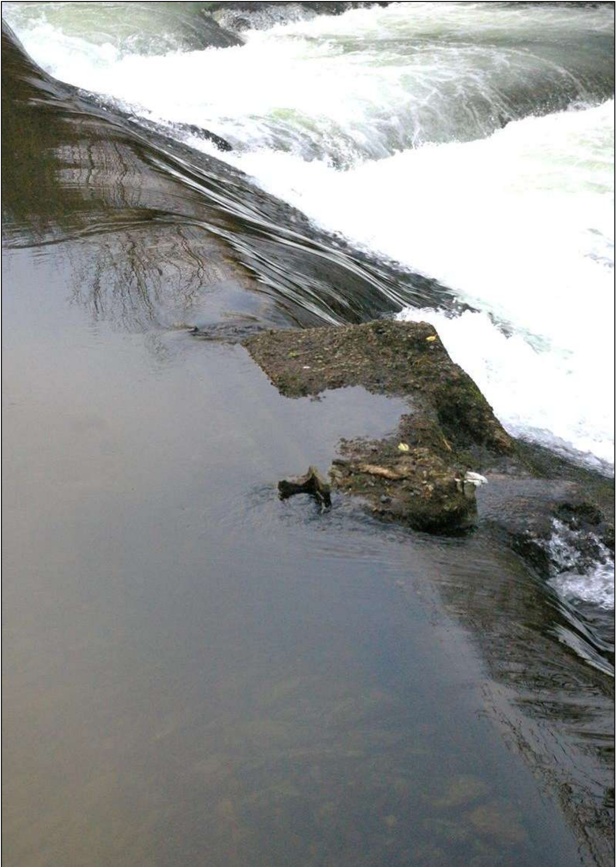
Figure 40: Detail of the weir, showing the possible broken stubs of iron fittings and a possible sluice gate; viewed from the south (no scale).
