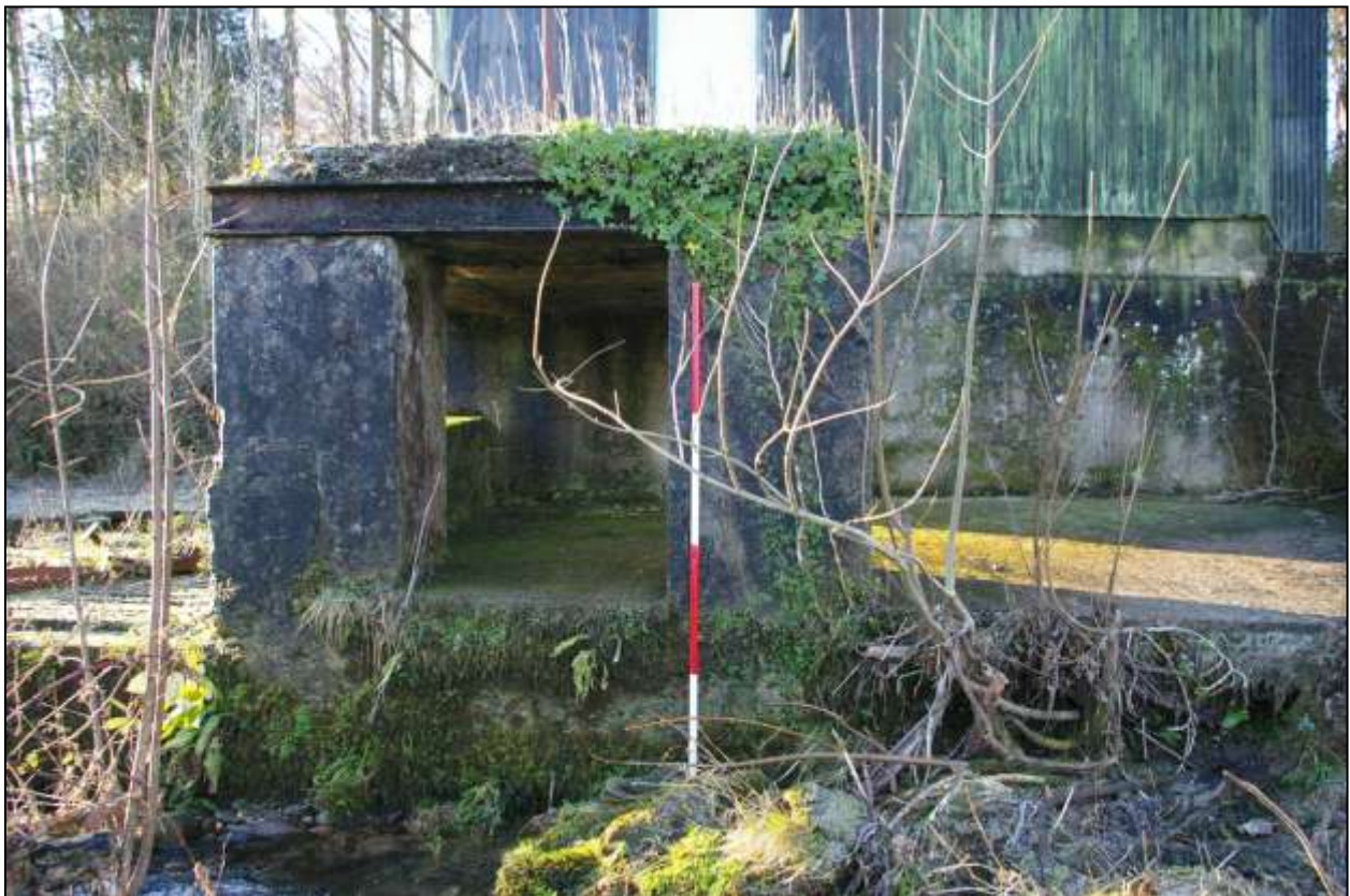
Figure 59: The east elevation of the platform, viewed from the east (scale 2m).
