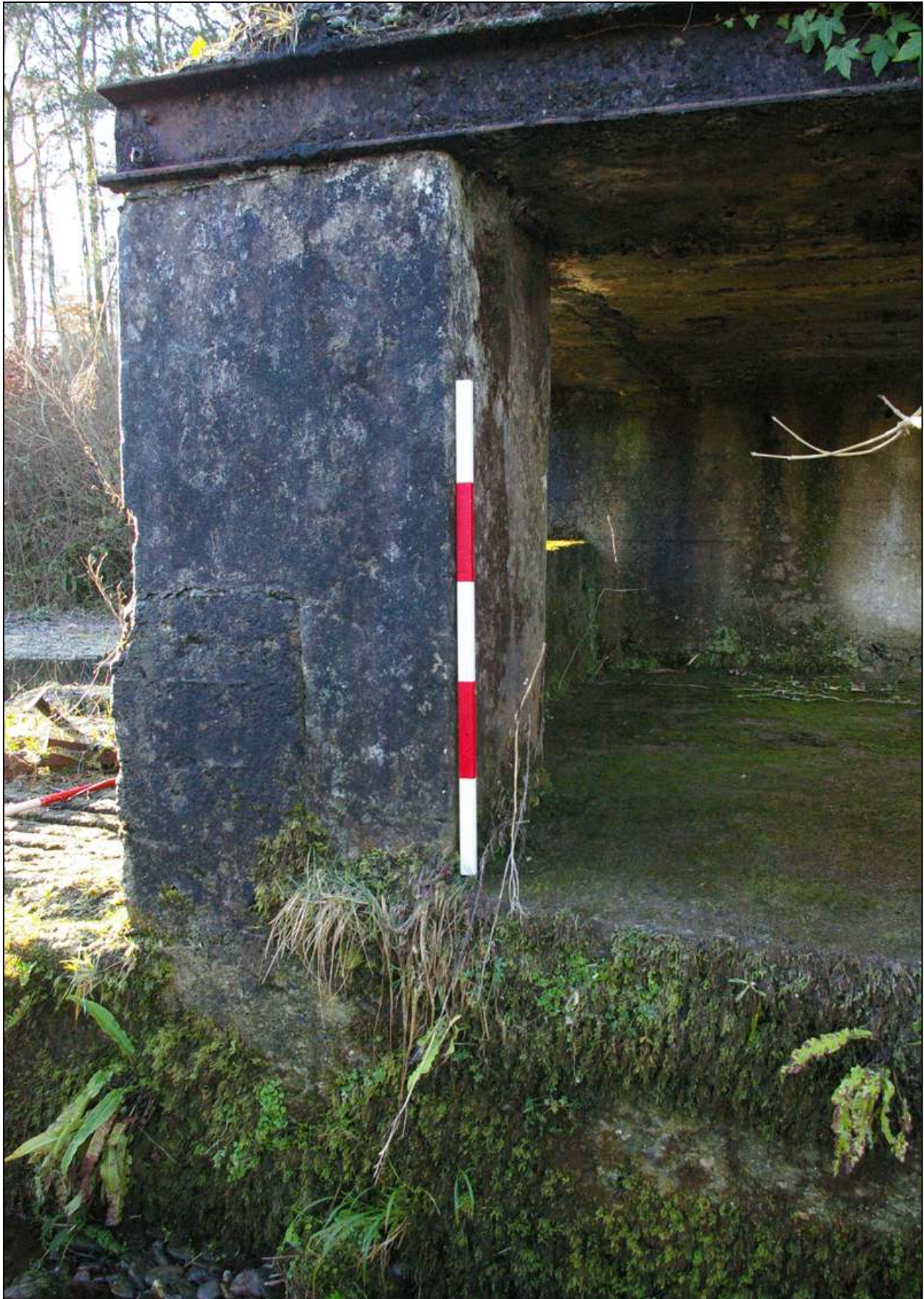
Figure 60: Detail of the east face of the south pillar, showing it built over and around the southern wall of the spillway; viewed from the east (scale 2m).
