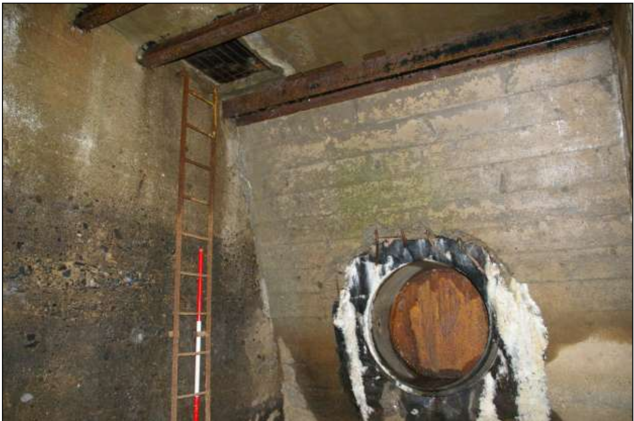
Figure 86: The ladder against the west wall, leading to a blocked hatch; viewed from the south-east (scale 2m).
