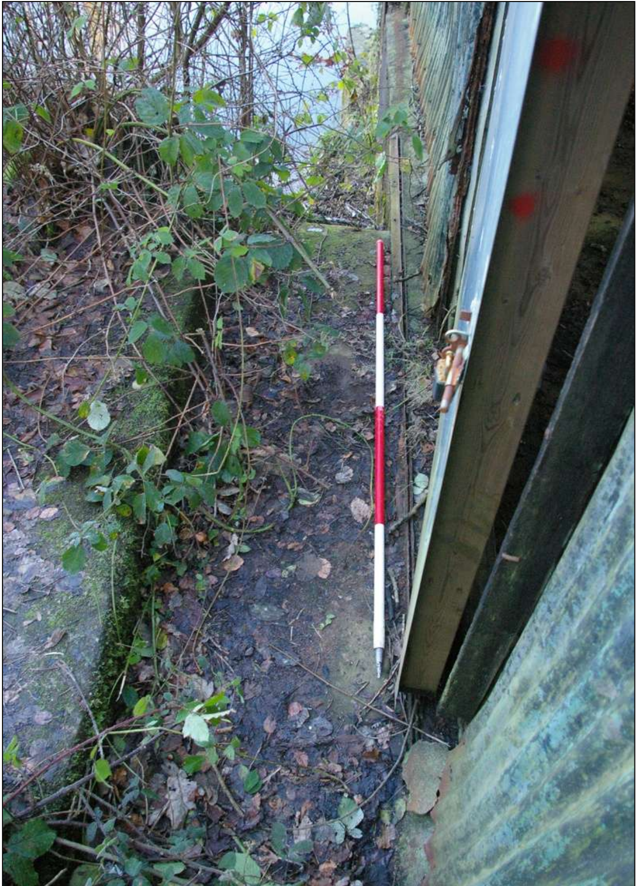
Figure 30: Detail of the lower door rail; viewed from the west (scale 2m).
