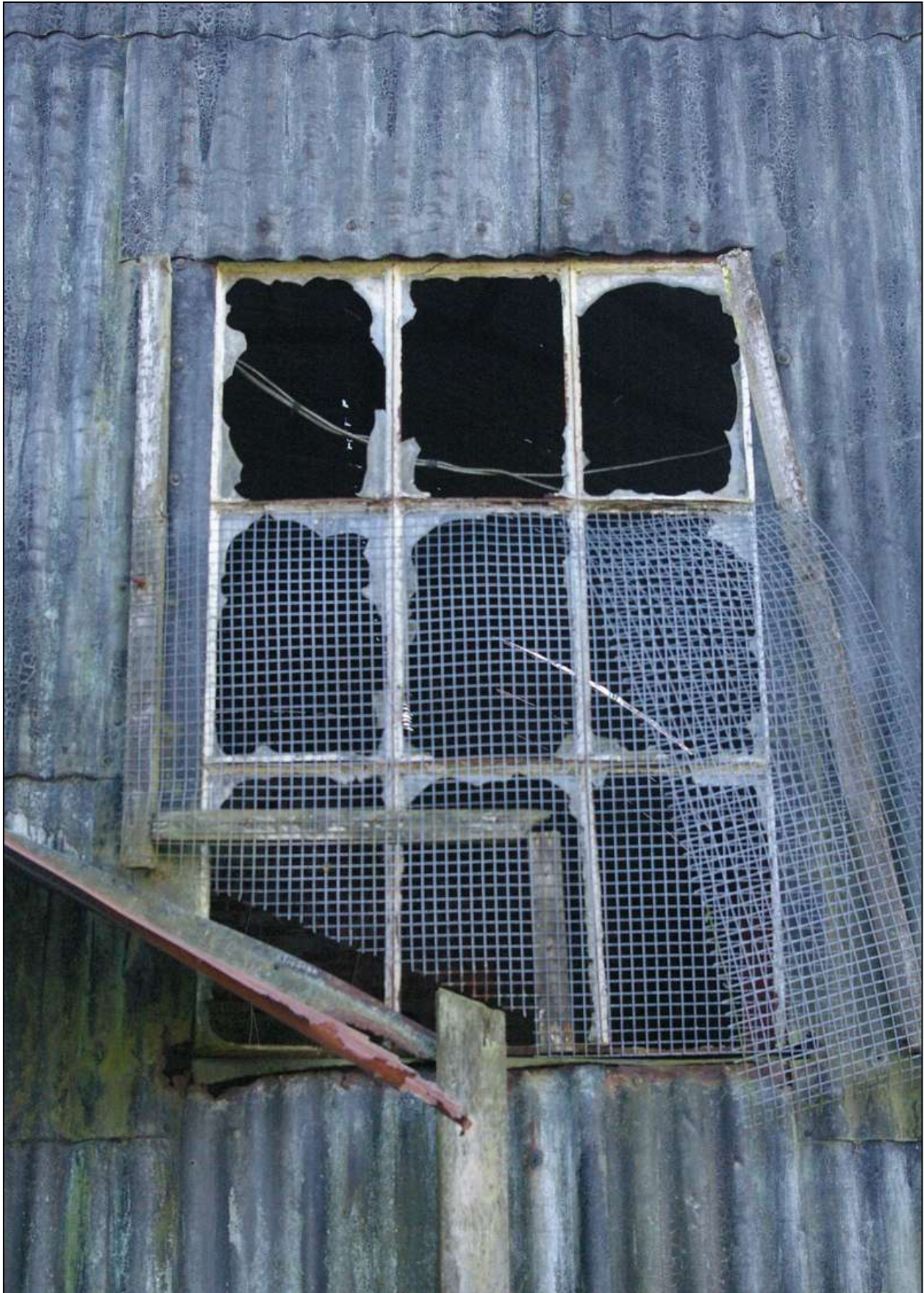
Figure 44: Detail of the window in the east elevation; viewed from the east (no scale).
