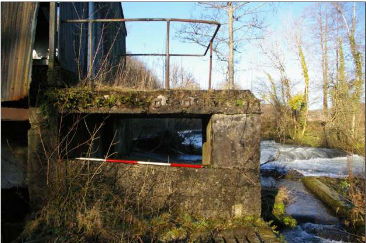
Figure 64: The south elevation of the platform, viewed from the south (scale 2m).
