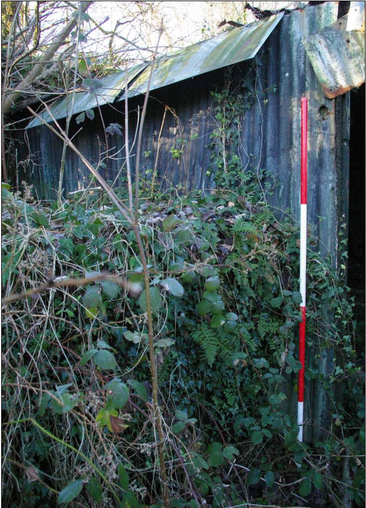
Figure 76: The west end of the south elevation of B1, showing the location of the concrete tank here; viewed from the south-east (scale 2m).
