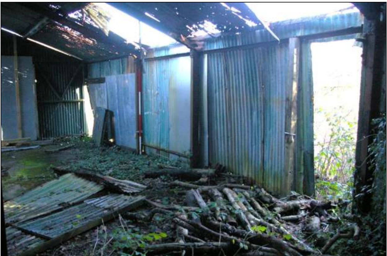
Figure 121: The south wall of B1 and B2; viewed from the north-west (scale 2m).
