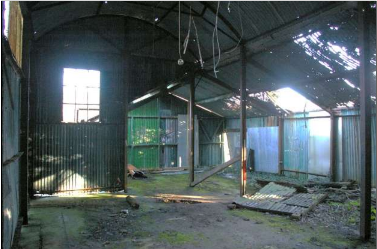
Figure 128: The interior of B1 and B2, viewed from the north-west (scale 2m).
