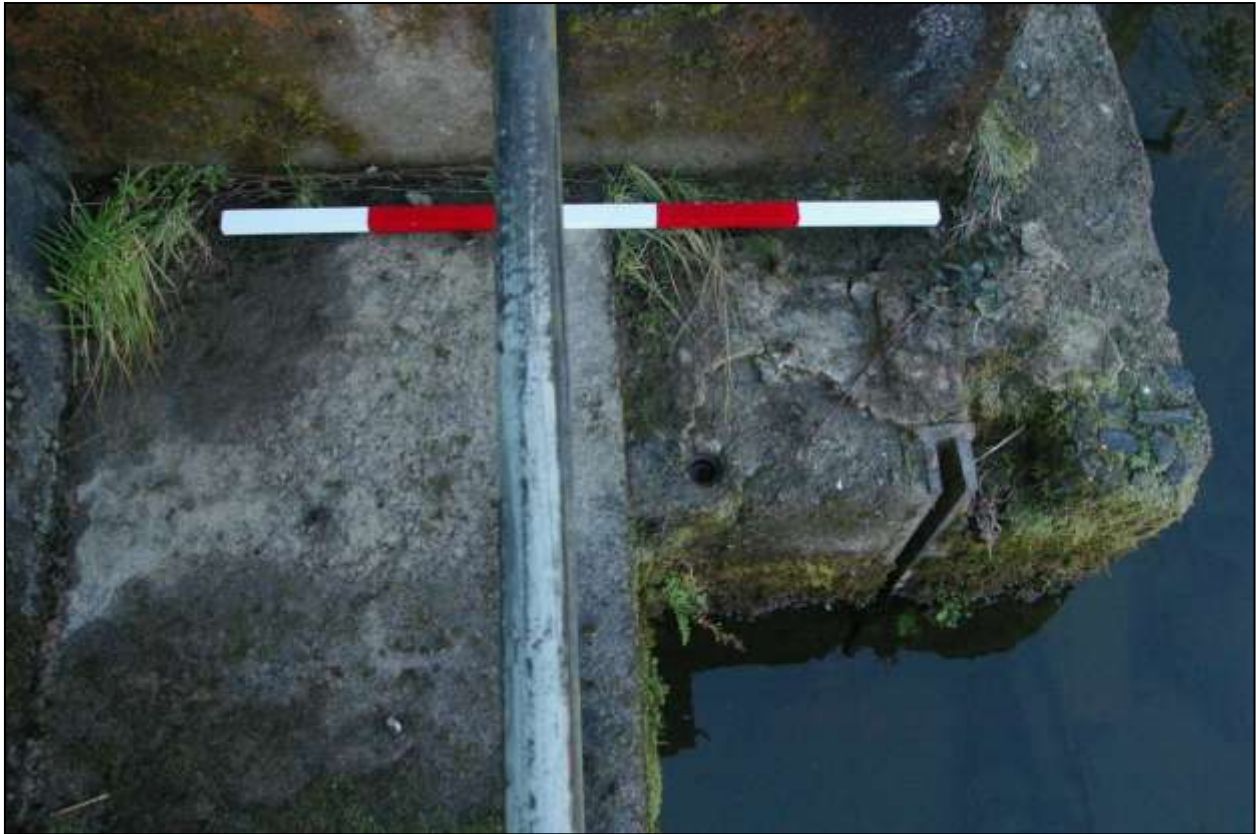
Figure 34: As above, from above, showing the sluice gate and associated pintles; viewed from the east (scale 1m).
