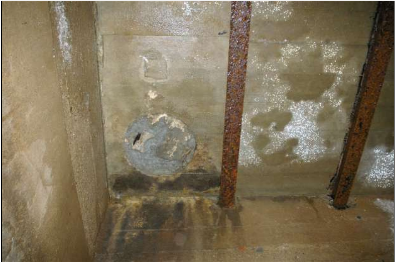
Figure 90: The blocked opening in the ceiling above the rotor control; viewed from the east (no scale).
