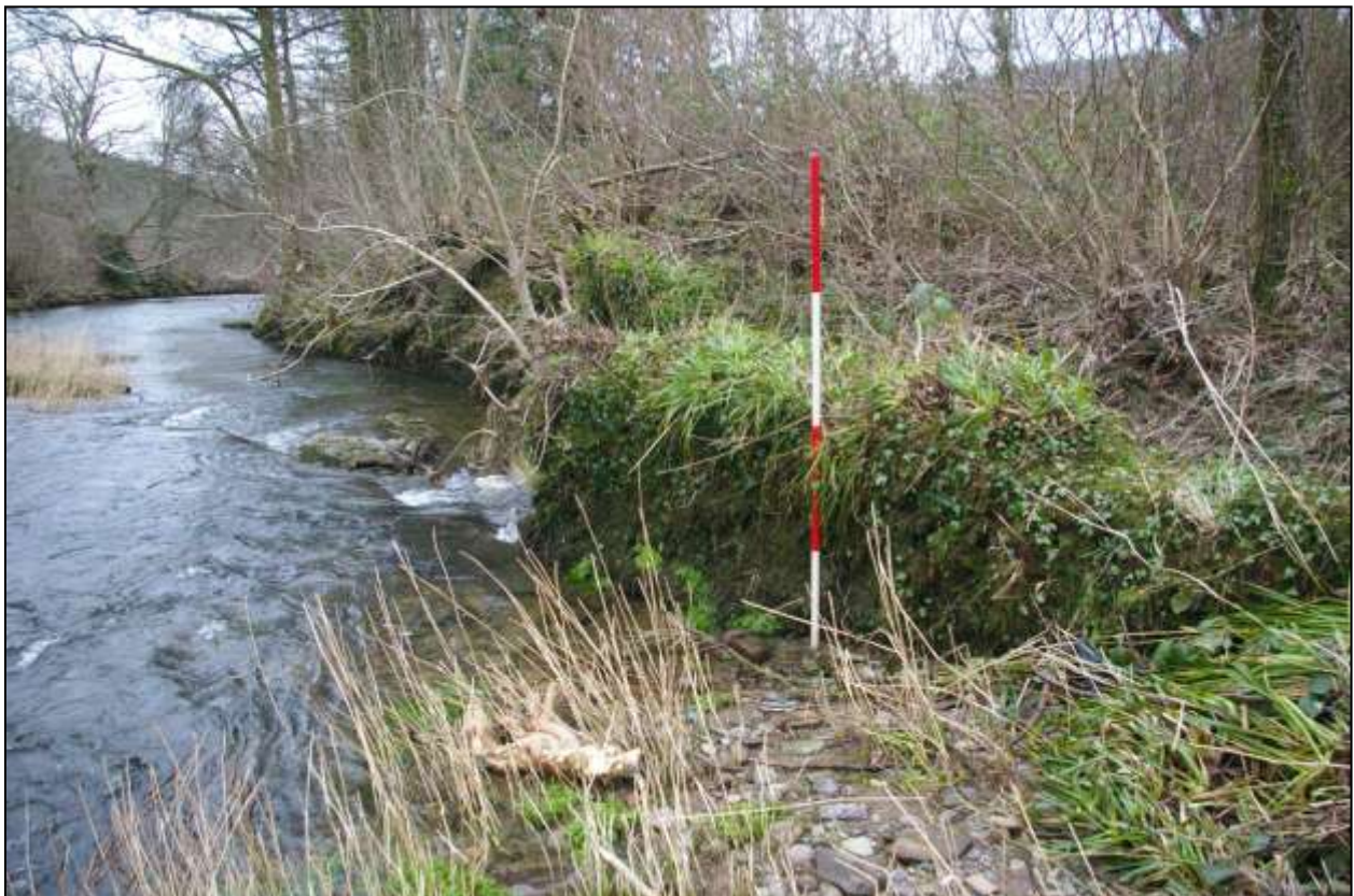
Figure 107: Masonry wall at the end of Leat 3, viewed from the north-east (scale 2m).
