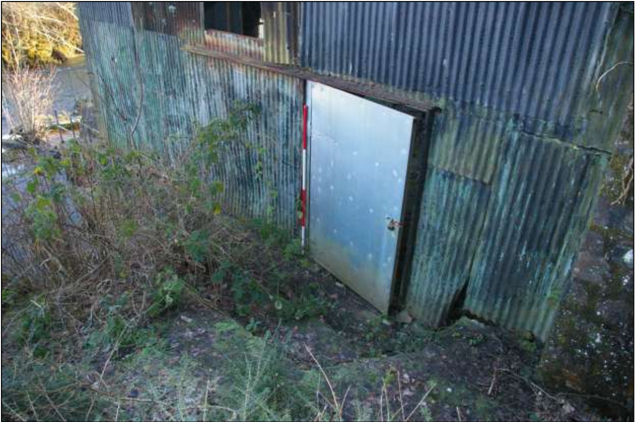
Figure 28: As above, detail of the new door and external steps (scale 2m).
