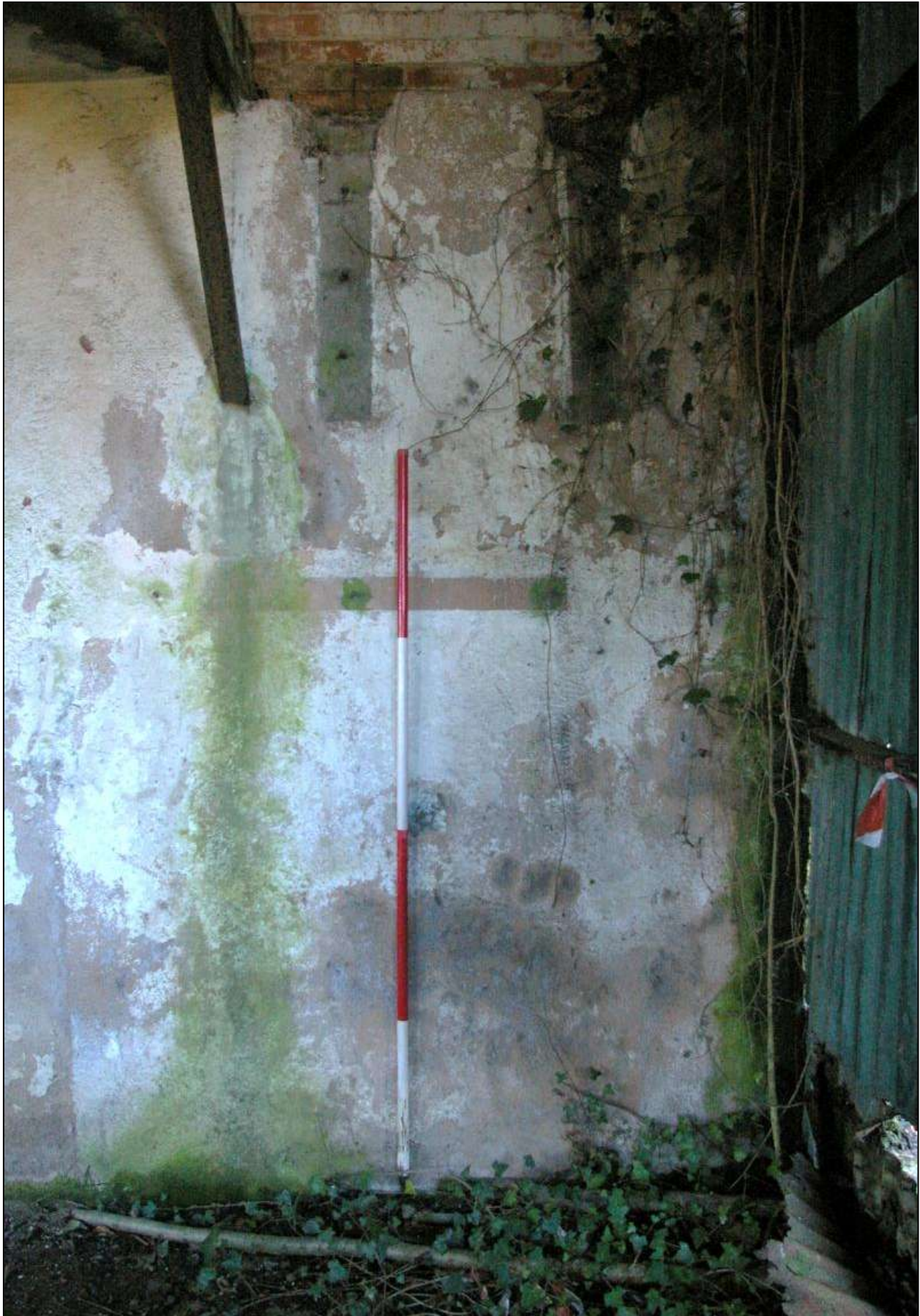
Figure 117: Scars on the west wall of B1, viewed from the east (scale 2m).
