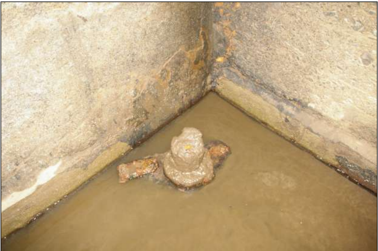
Figure 89: The stub of the rotor control in the south-west corner; viewed from the north-east (no scale).
