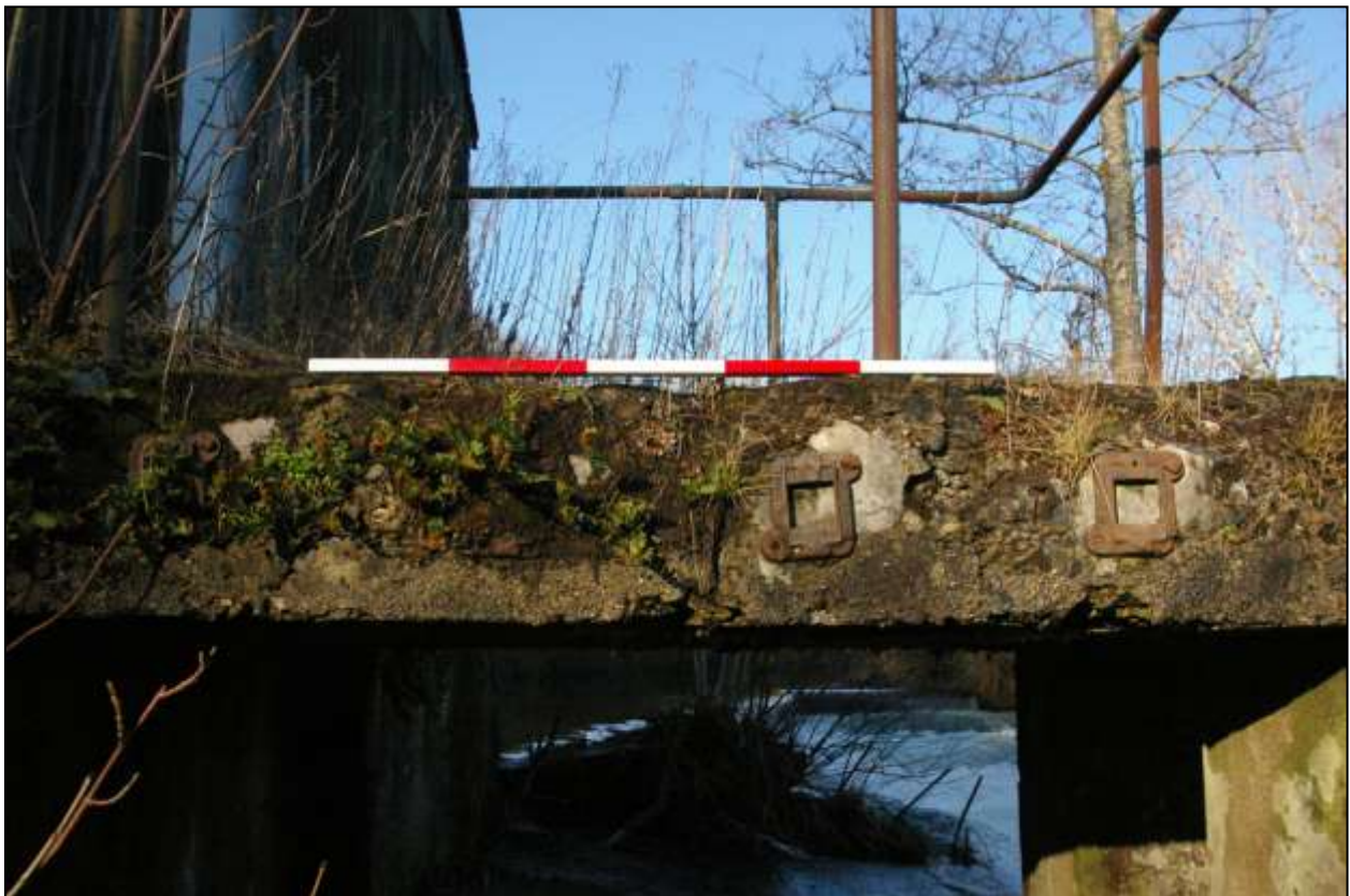
Figure 68: Detail of the platform, showing the DOULTON brackets; viewed from the south (scale 1m).
