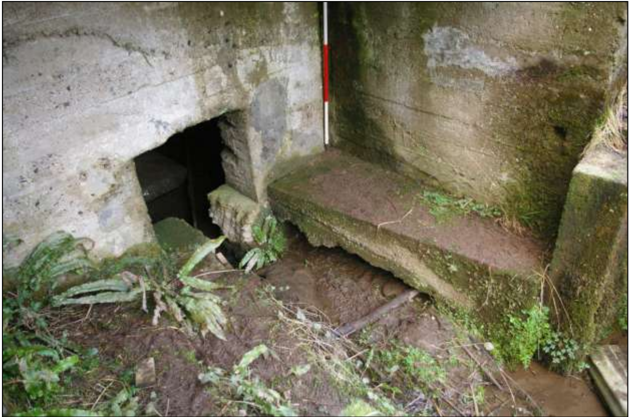
Figure 83: The floor of the outer part of the turbine chamber, showing the former spillway; viewed from the south-west (scale 2m).
