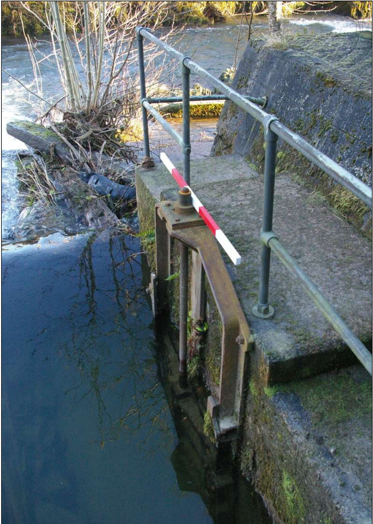
Figure 31: Detail of the FARRER sluice gate at the eastern end of the north elevation; viewed from the north-west (scale 1m).
