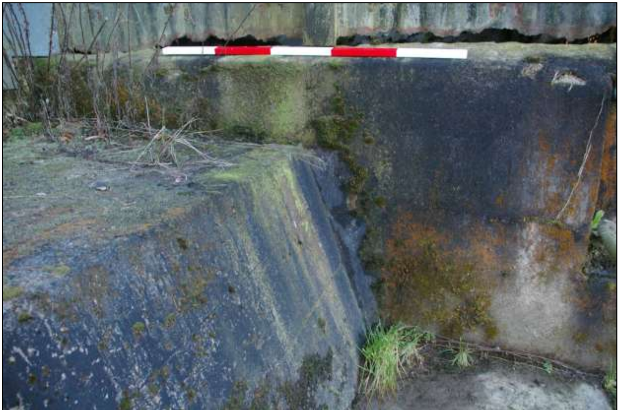
Figure 42: Base of the east elevation of B1, showing rebuilt sloping concrete front; viewed from the east (scale 1m).
