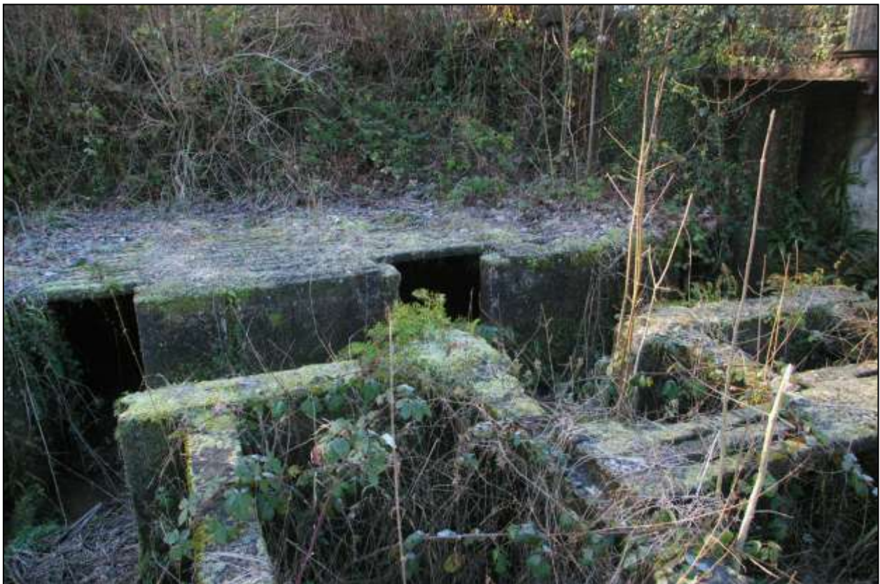
Figure 95: The fish tanks adjacent to the south elevation of Building #2, viewed from the east (no scale).
