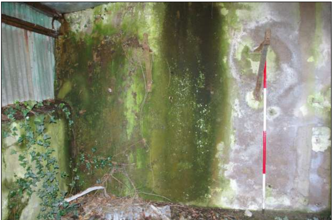
Figure 119: The south end of the west wall; viewed from the east (scale 2m).
