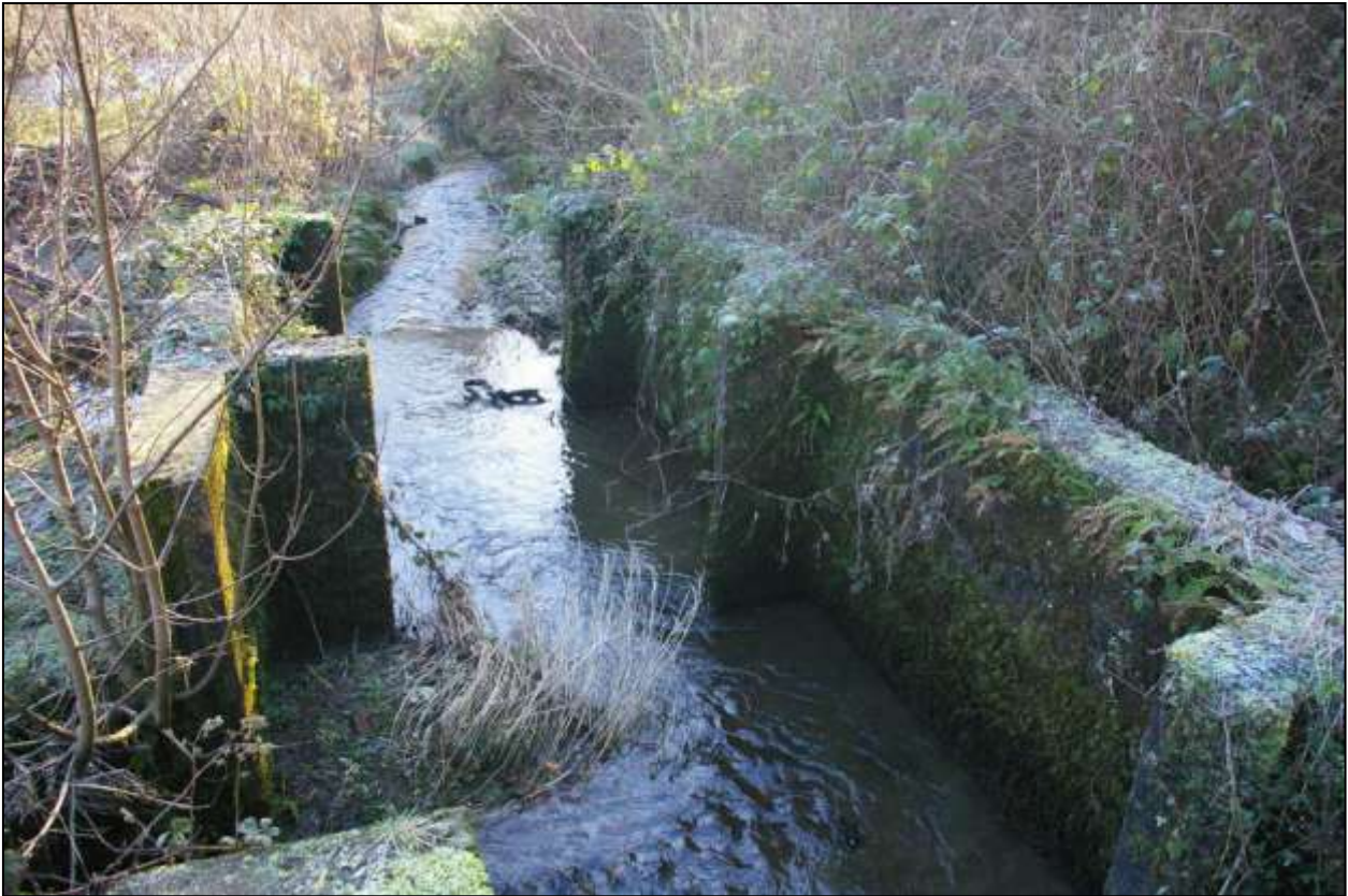
Figure 98: View of the control chambers to the south of the fish tanks; viewed from the NNE (no scale).
