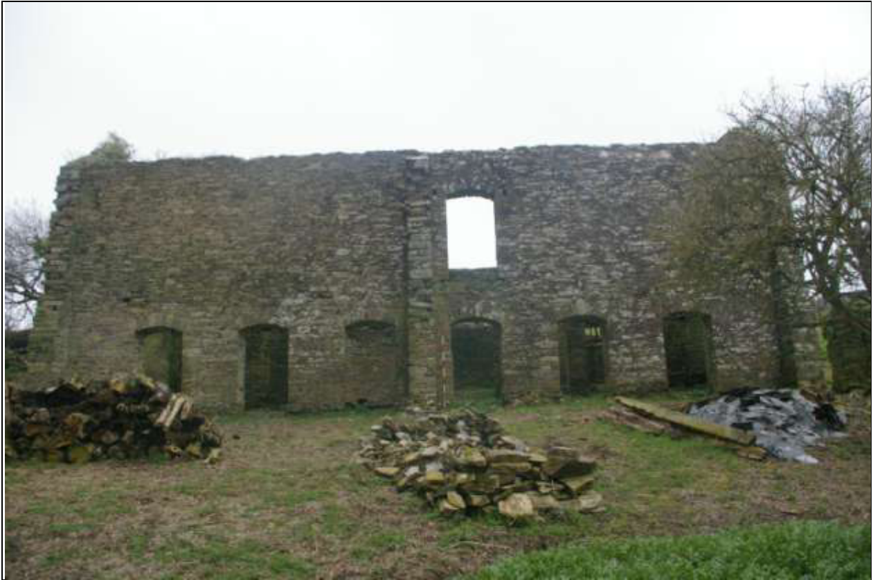
The south elevation, viewed from the foldyard to the south (2m scale).
