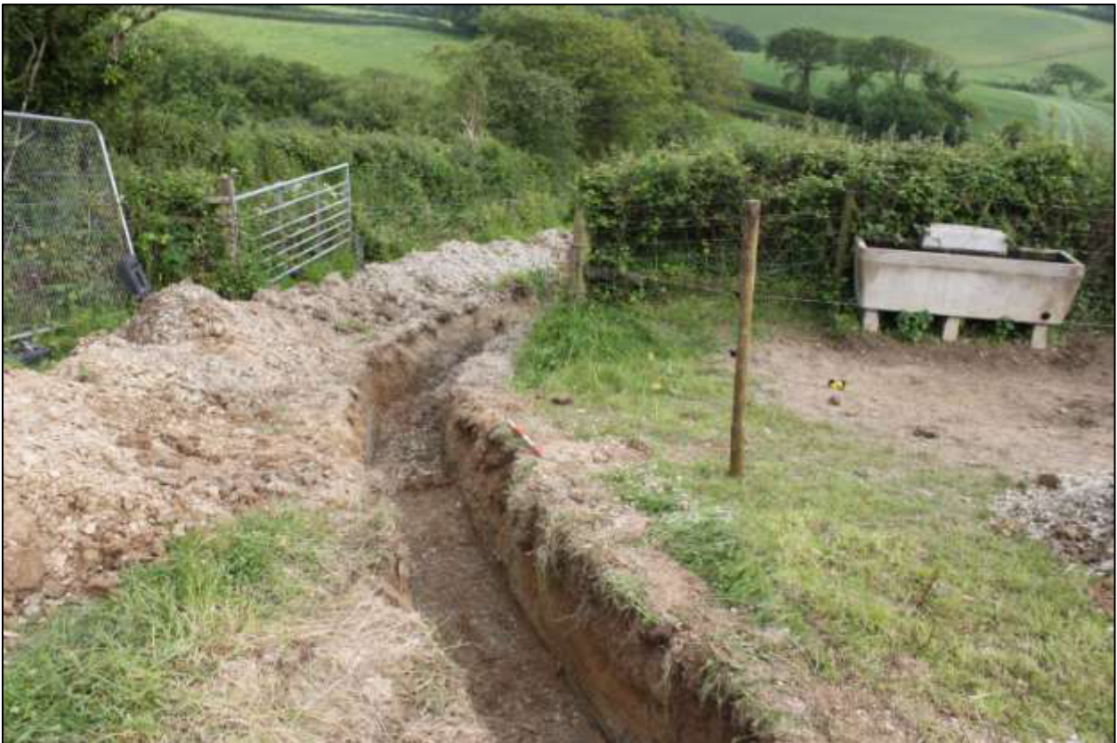
Service trench as it passes through gateway between Fields 3 and 4, viewed from the north (1m scale).
