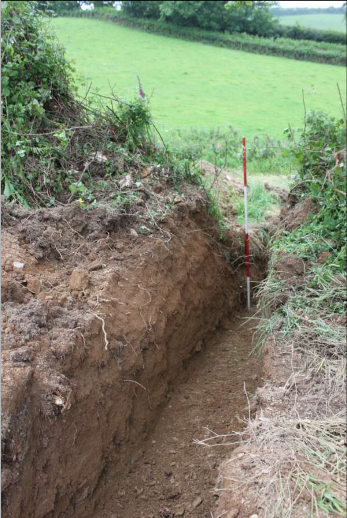
Shot of service trench through hedgebank between fields 2 and 3, viewed from the south-south-east (2m scale).
