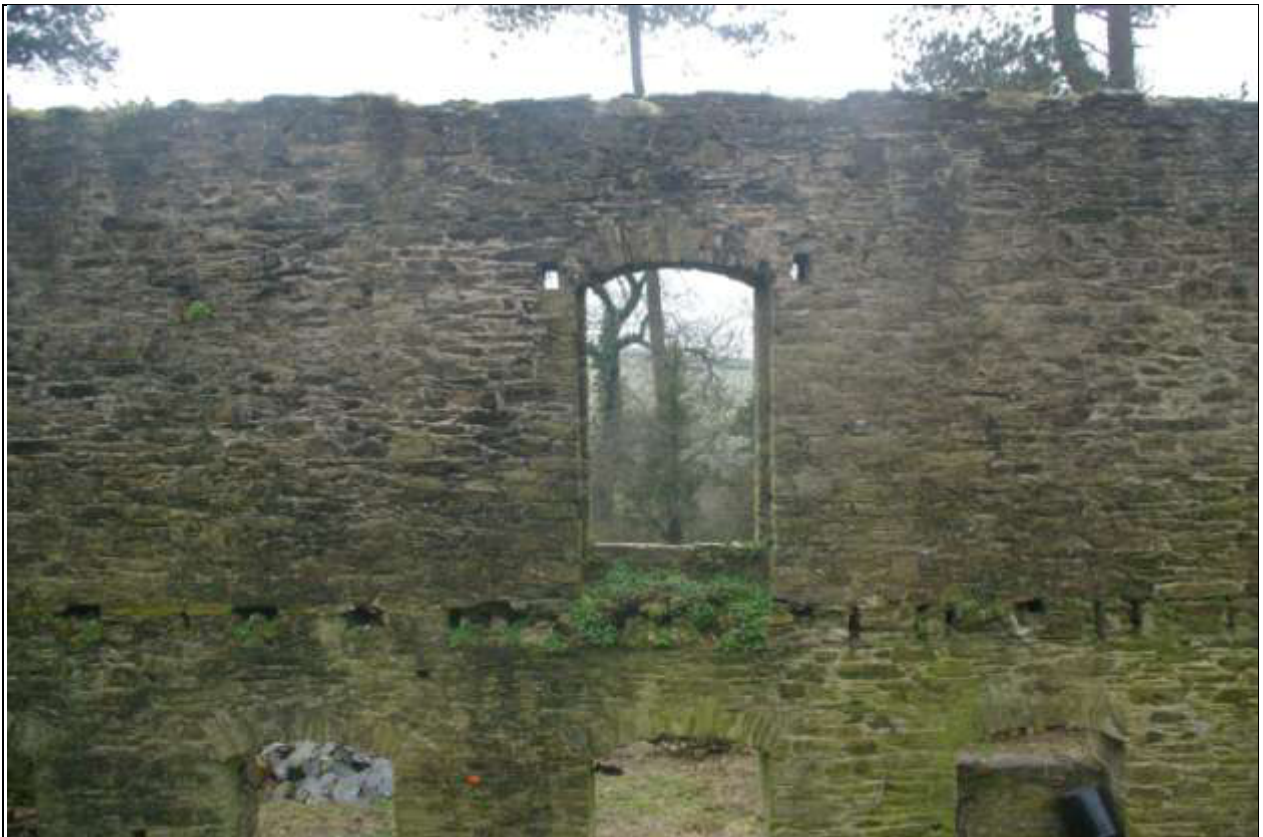
The loading door at the first floor in the south elevation; viewed from the north.
