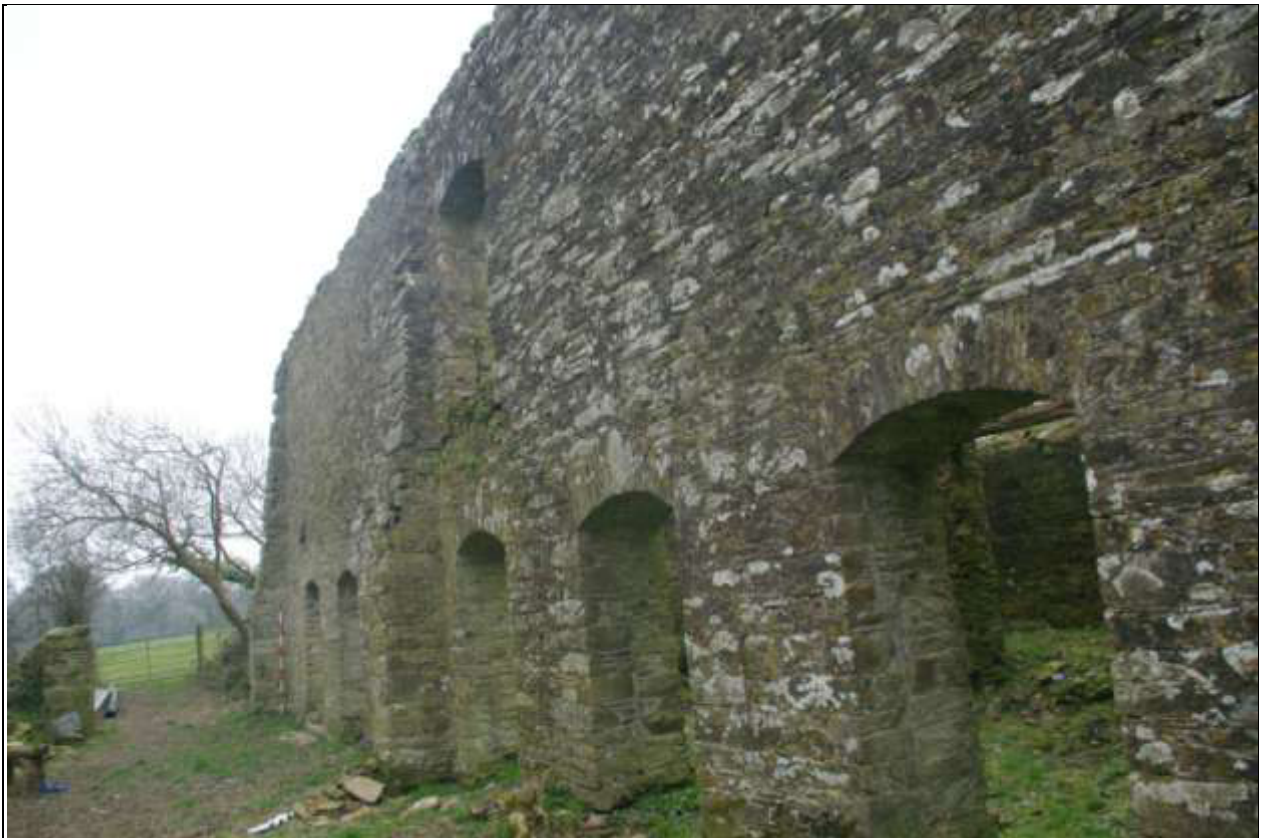
Shot along the south elevation, showing the buttresses; viewed from the east-south-east (2m scale).
