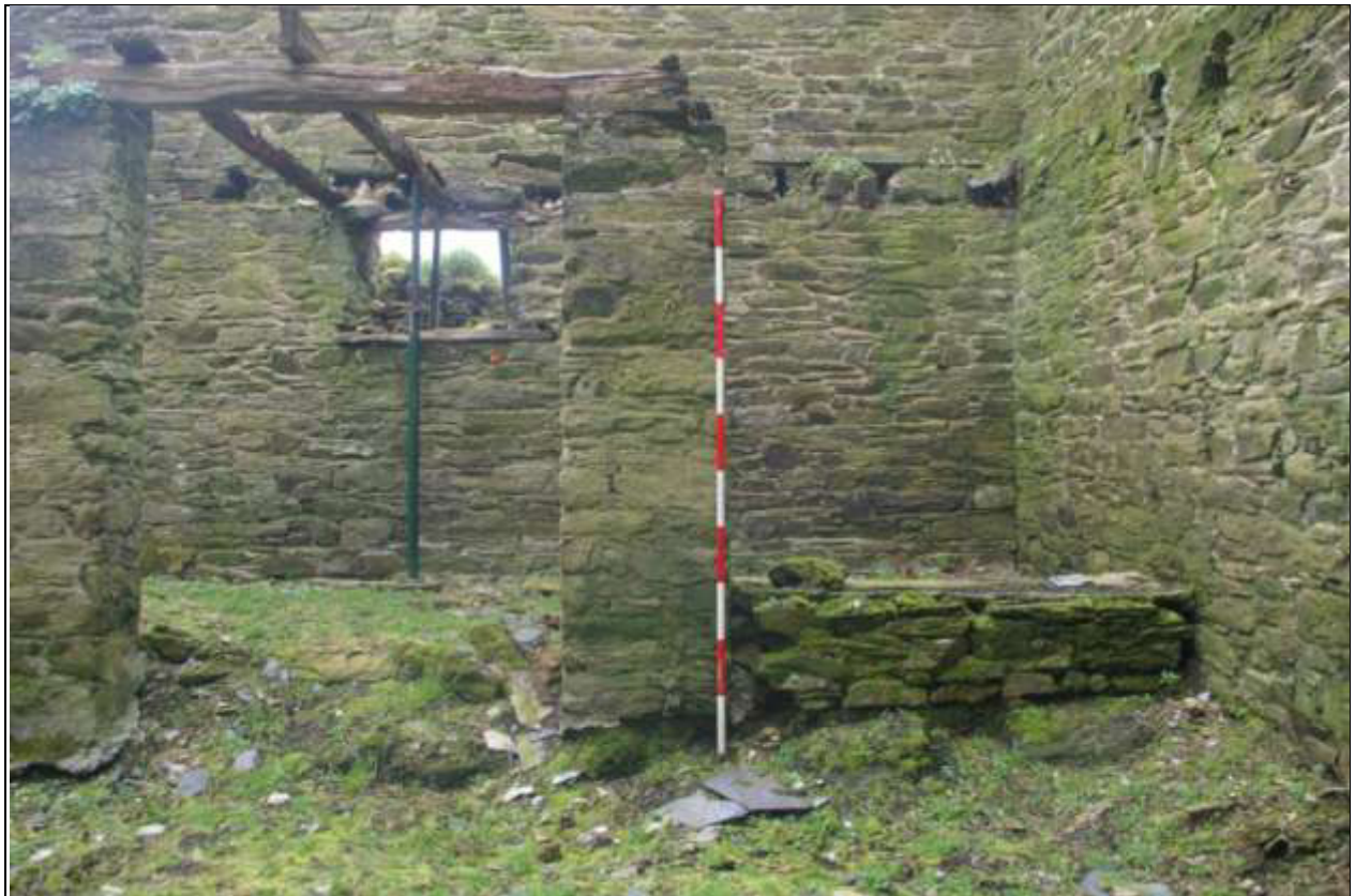
The pillars and stone-built trough to the east end; viewed from the south (2m scale).
