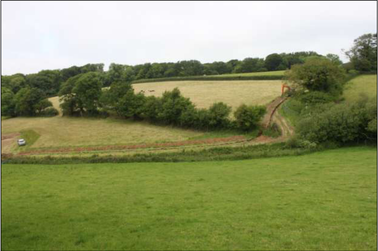
Shot of the service trench mid-excavation through Fields 2 and 3, viewed from the east.
