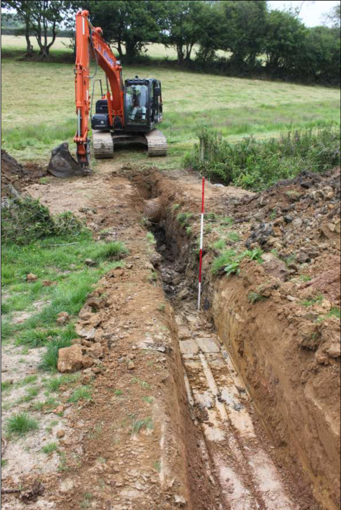
Shot of service trench as it crossed the recently piped watercourse separating Fields 1 and 2, viewed from the south-east (2m scale).
