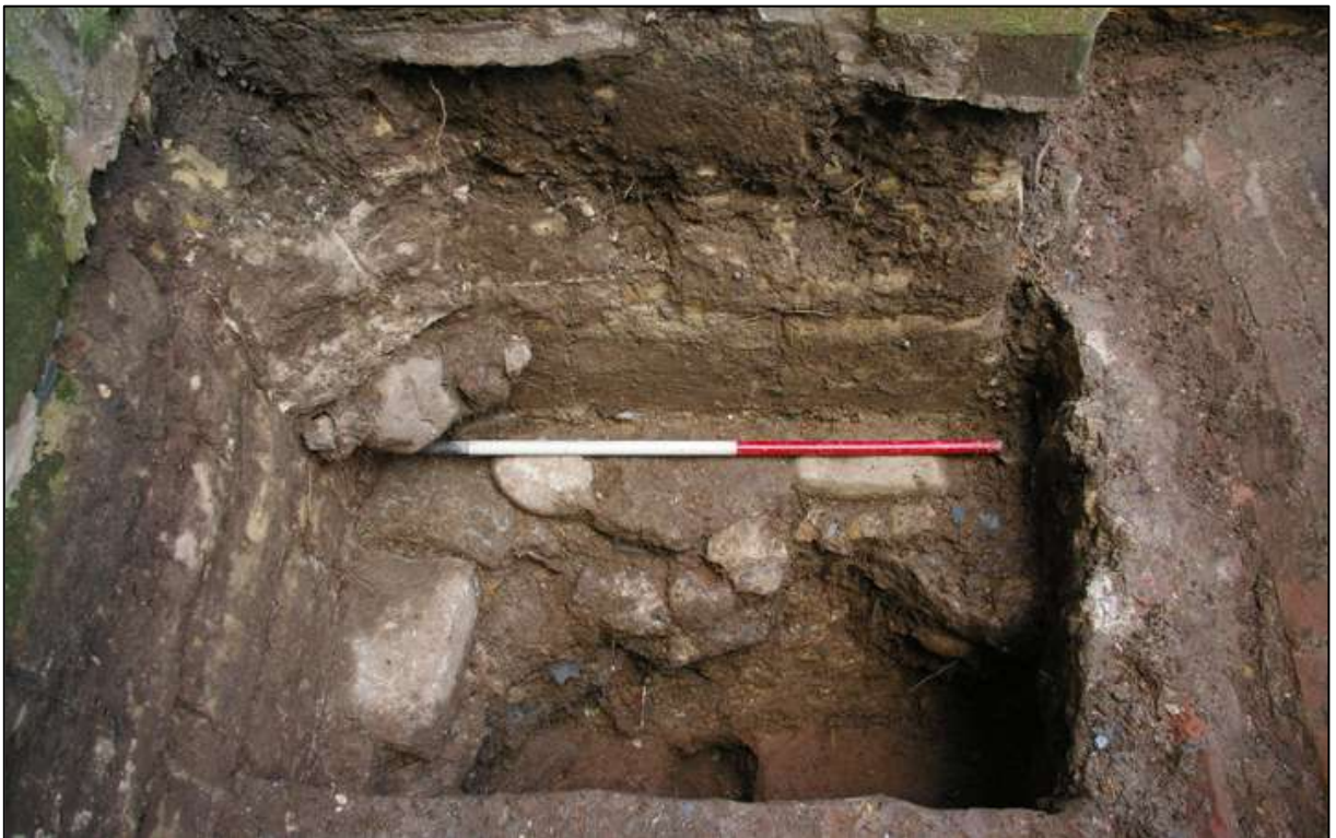
Figure 5: Foundations of north-western buttress to the tower; viewed from the east (1m scale).
