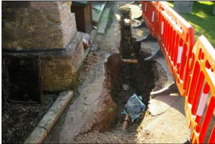
Location of existing man-hole and brick rubble in drainage trench; viewed from the east (no scale).
