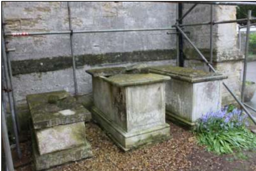
Chest tombs on north side of tower, pre-removal viewed; from the north-east (no scale).
