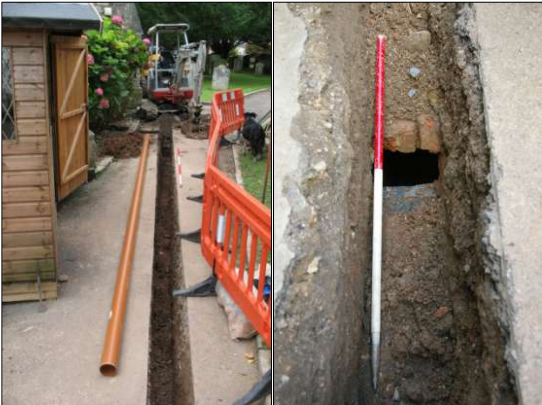
(Left): Drainage trench (east end) along north side of church; viewed from the east (2m scale). (Right): Brick-built tomb in drainage trench/footpath left in situ; viewed from the east (1m scale).
