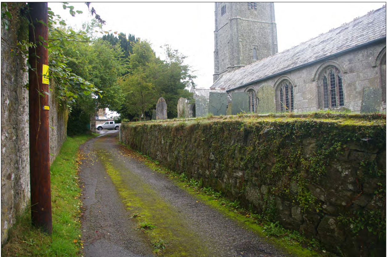
The wall of the churchyard, to the south and the walls to Withiel House; from the east-south-east.
