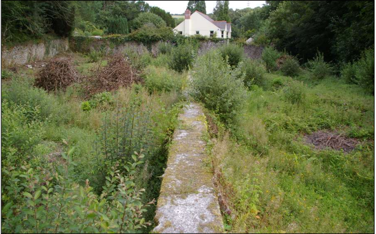
Figure 12: Shot of settling tanks; viewed from the south (no scale).
