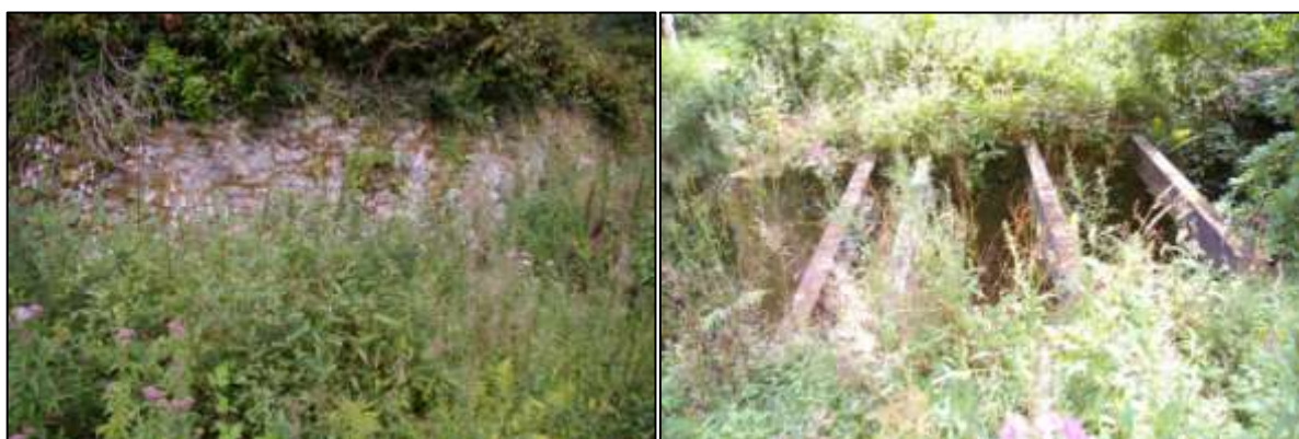
Figure 18: Western retaining wall in south half of site; viewed from the east (no scale).
