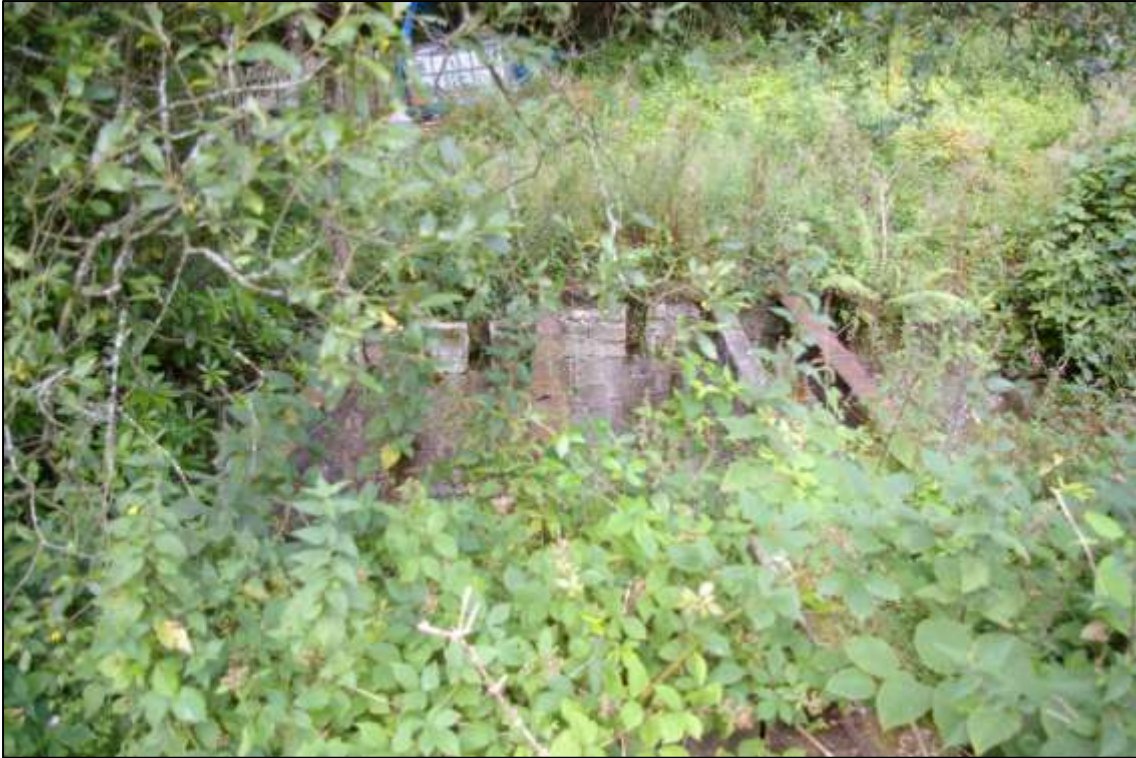
Iron girder and concrete block setting of derelict bridge; viewed from the east (no scale).
