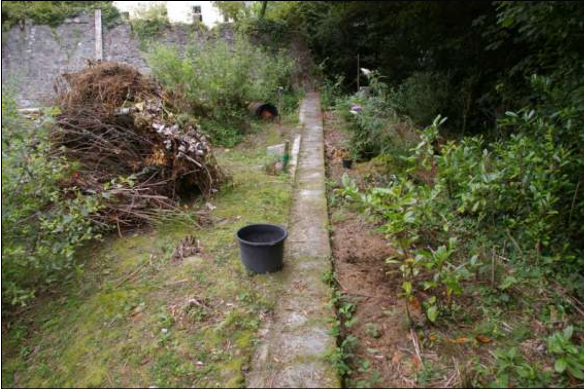
Eastern wall of eastern settling tank; viewed from the south (no scale).
