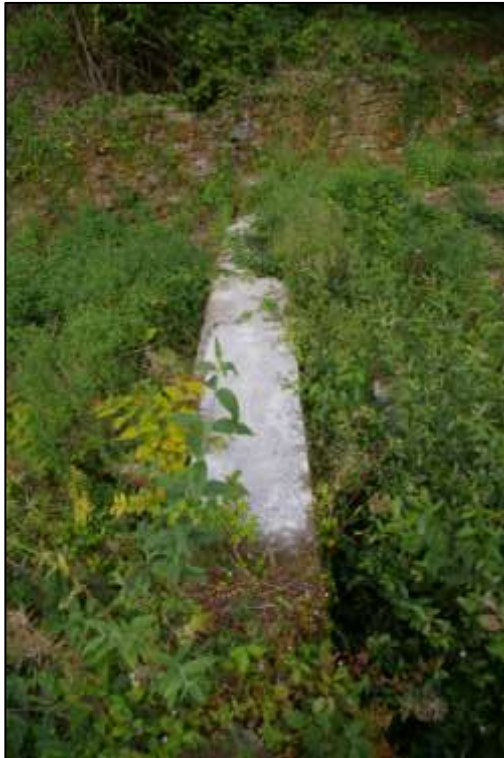
South wall of western settling tank; viewed from the east (no scale).
