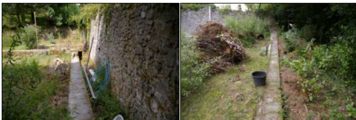
Figure 10: North boundary wall and north settling tanks wall; viewed from the east (no scale).
