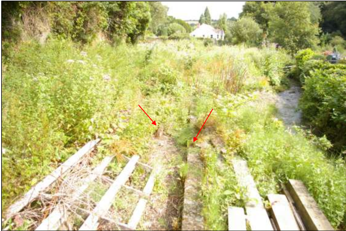
Concrete drag visible in centre (indicated) with debris on either side; viewed from the south (no scale).
