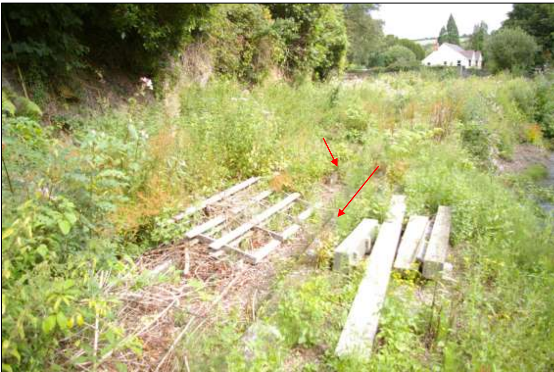
Concrete drag visible in centre (indicated) with debris on either side; viewed from the south (no scale).
