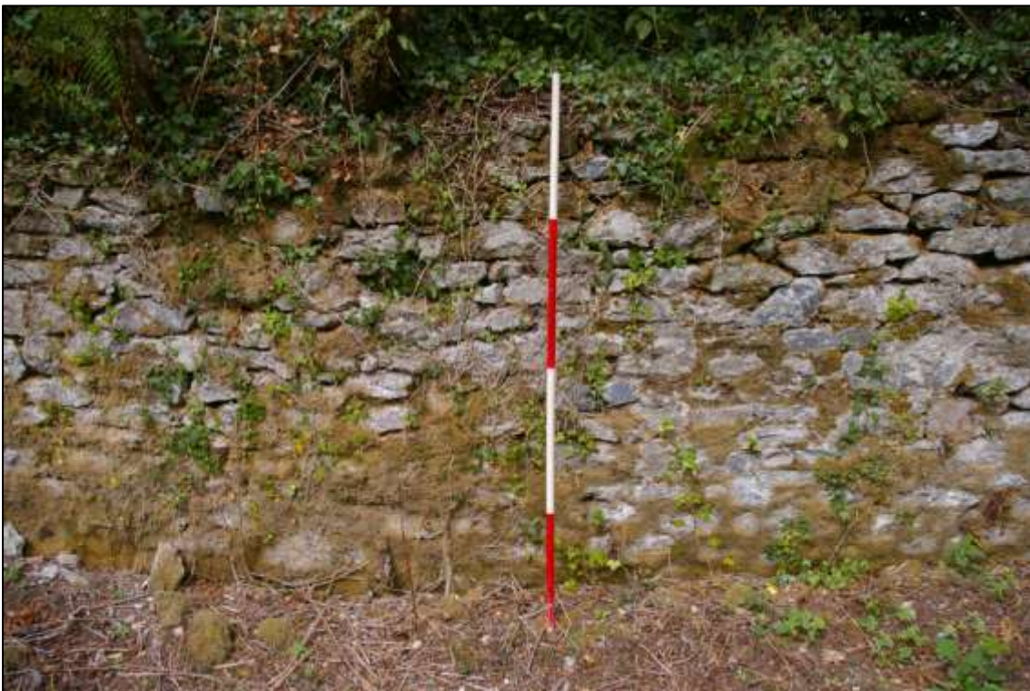
Retaining wall/western wall of western settling tank; viewed from the east (2m scale).
