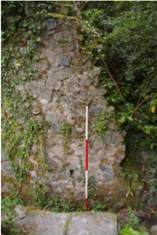
East end of northern boundary wall; viewed from the south (2m scale).
