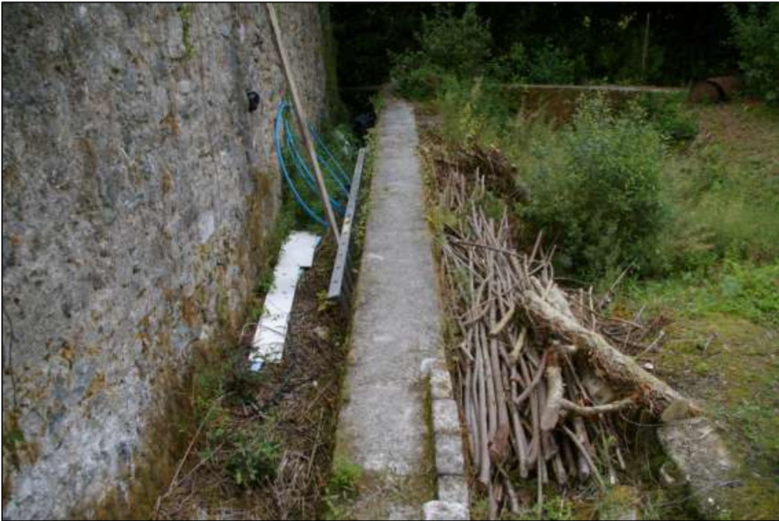
North wall of eastern settling tank; viewed from the west (no scale).
