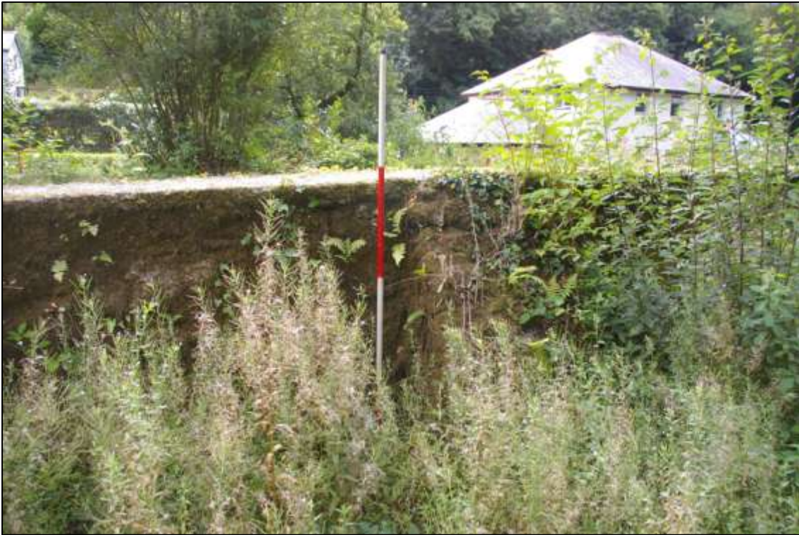
Brick buttress in western settling tank against dividing wall; viewed from the north-west (2m scale).
