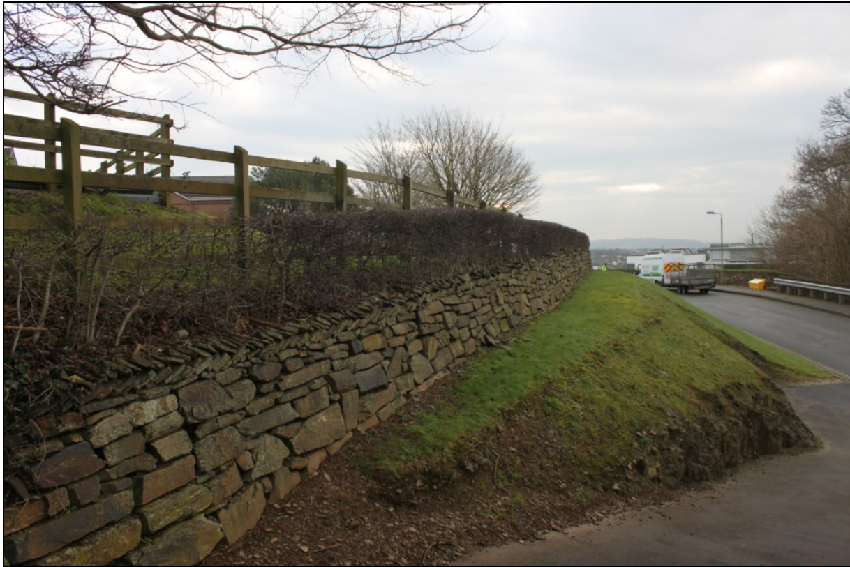
The new wall to the south of the proposed drainage access, viewed from the west (no scale).
