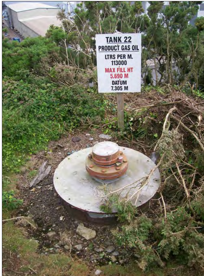
Dip-well or gas-release valve above tank 22; viewed from the south.
