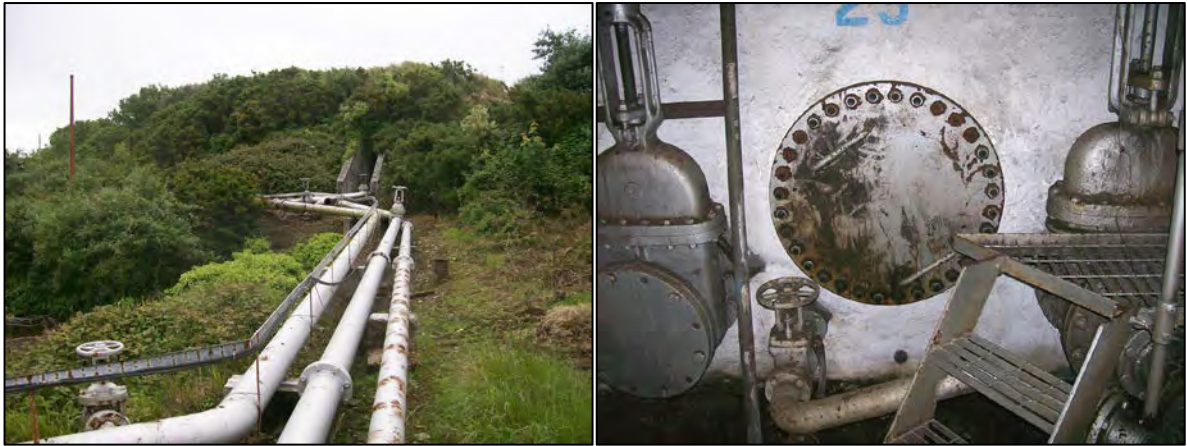
Figure 14: View along the pipework before it enters the east tank; viewed from the north-west. Figure 15: Inside the east tank; viewed from the north-west.
