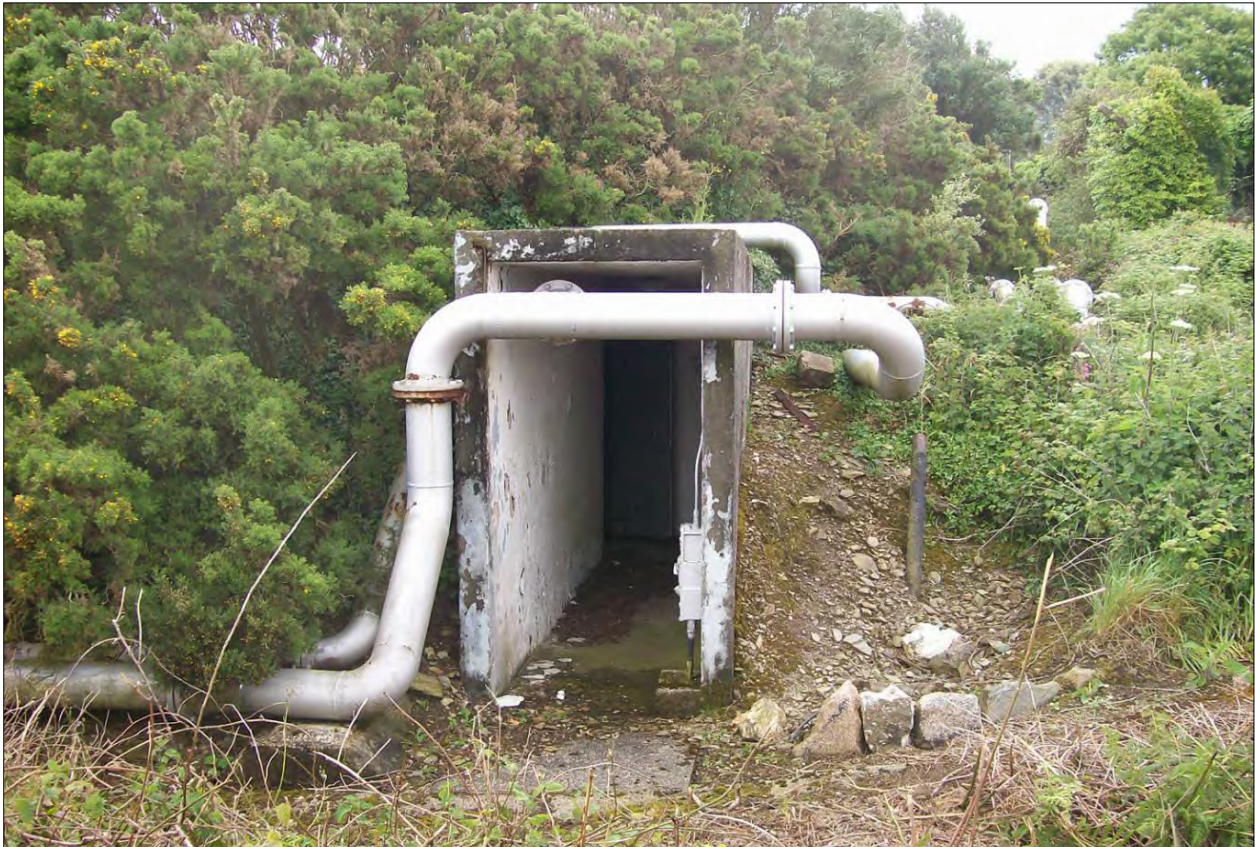
Entrance to the tank at western end of the depot; viewed from the west.
