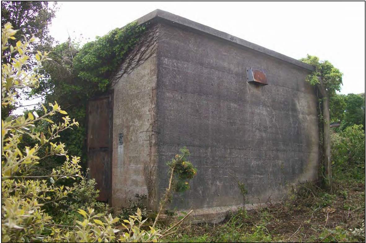
Figure 27: Ancillary structure at the western end of the fuel depot; viewed from the west.
