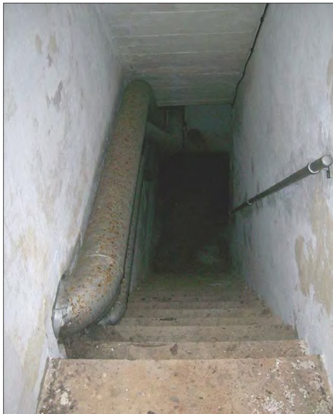
Stairwell down to the central bunker, south-west of the administrative building; viewed from north-east.
