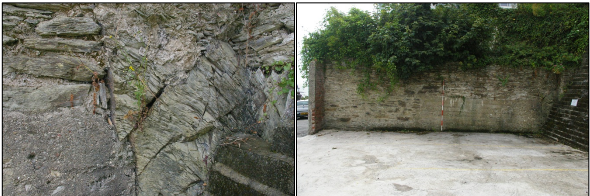
Figure 12: Detail of natural bedrock into which the site has been terraced; viewed from the east
