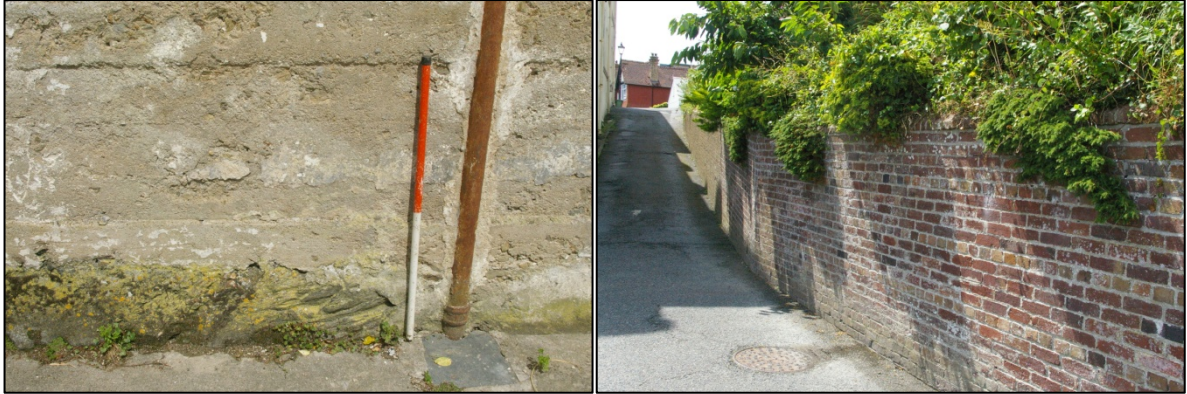
Figure 25: View of drainage channel along eastern site boundary; viewed from the west (1m scale)
