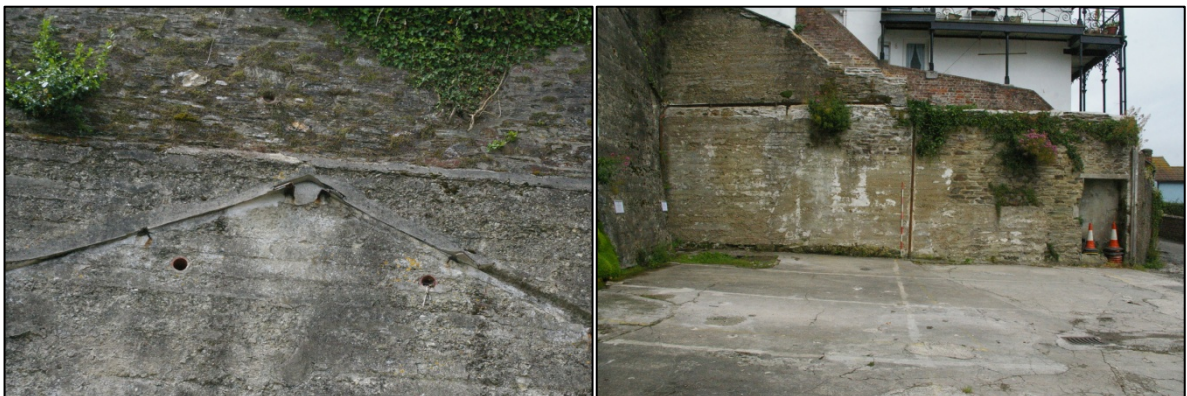
Figure 18: Detail of roof line cut into northern site boundary; viewed from the south
