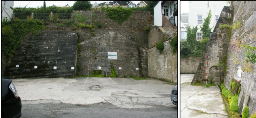
Figure 14: View of the northern boundary showing partially rendered lower part; from the south (2m scale)
