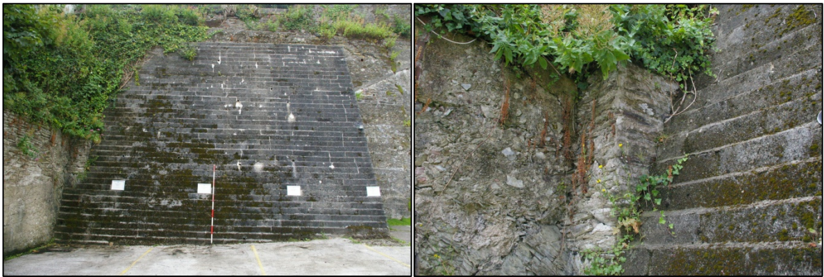
Figure 16: View of the buttress at the western end of northern boundary; viewed from the south (2m scale)
