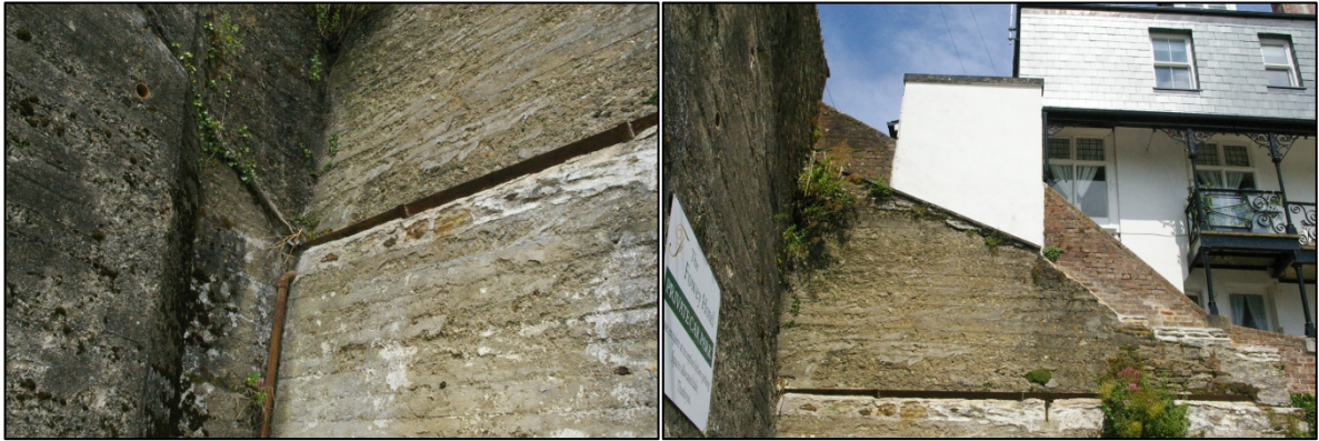
Figure 20: Detail of guttering of former structure, running along eastern wall; viewed from the south-west Figure 21: View of eastern boundary wall showing adjacent property boundary; viewed from the west
