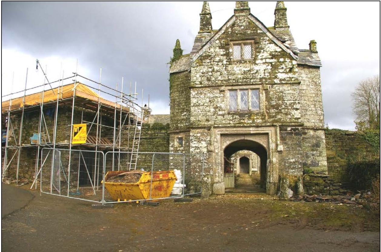
View between Bradstone Manor beyond and the gatehouse, showing the close relationship of the buildings, which the turbine cannot interrupt; from the west, south-west.
