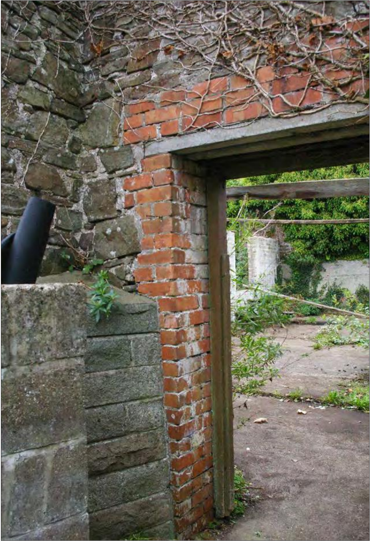
The forced opening the stone wall between Areas 3 & 4, from Area 4, showing the brickwork, concrete block patching and concrete slab lintels; from the south-west.
