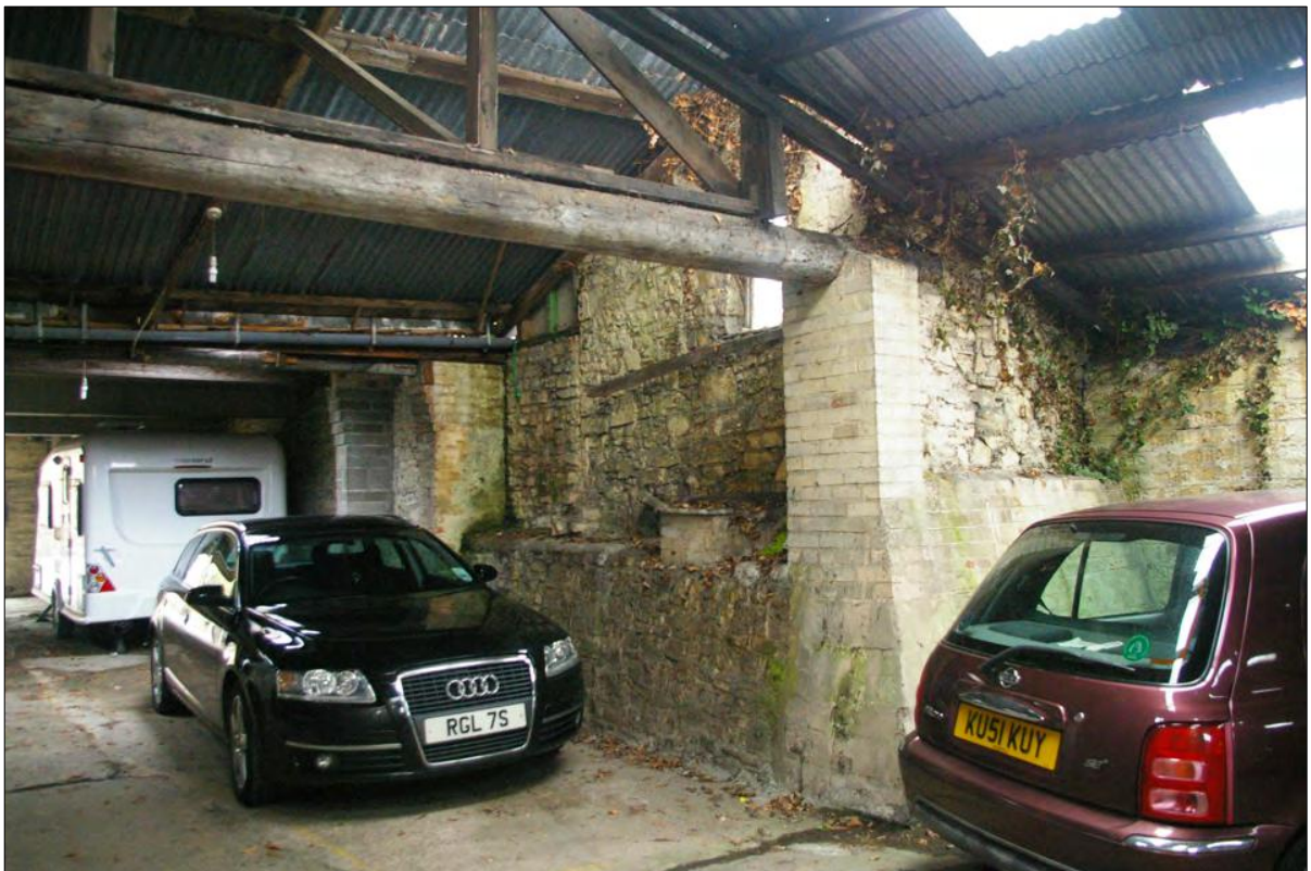
Figure 15: The various phases of stone work visible in the north wall of Area 6, party walls with Area 4; viewed from the south-east.
