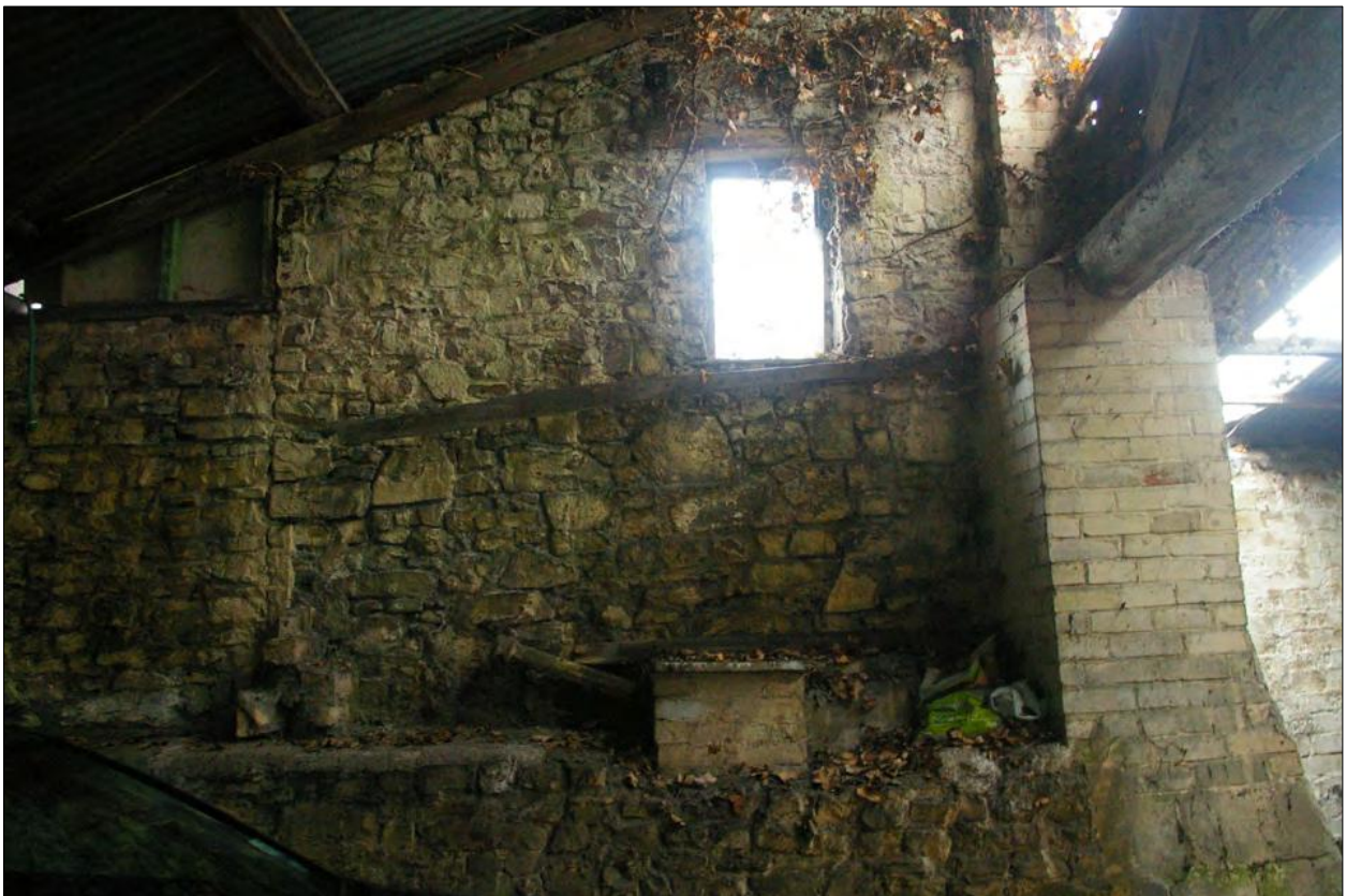
Detailed view of the party wall, of various phases of stonework between Areas 6 & 4; from the south.
