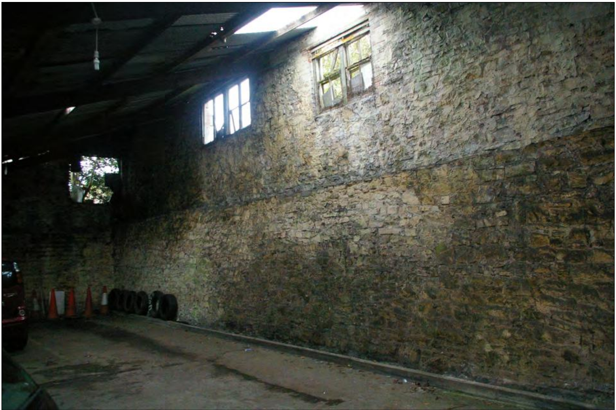
The eastern end of the south wall in Area 6, showing the large buttress to the base; from the north-west.
