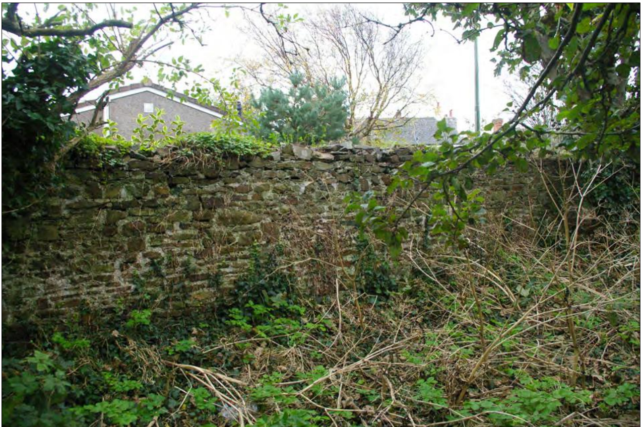
View of the central section of the south wall of Area 1; from the north-north-east.
