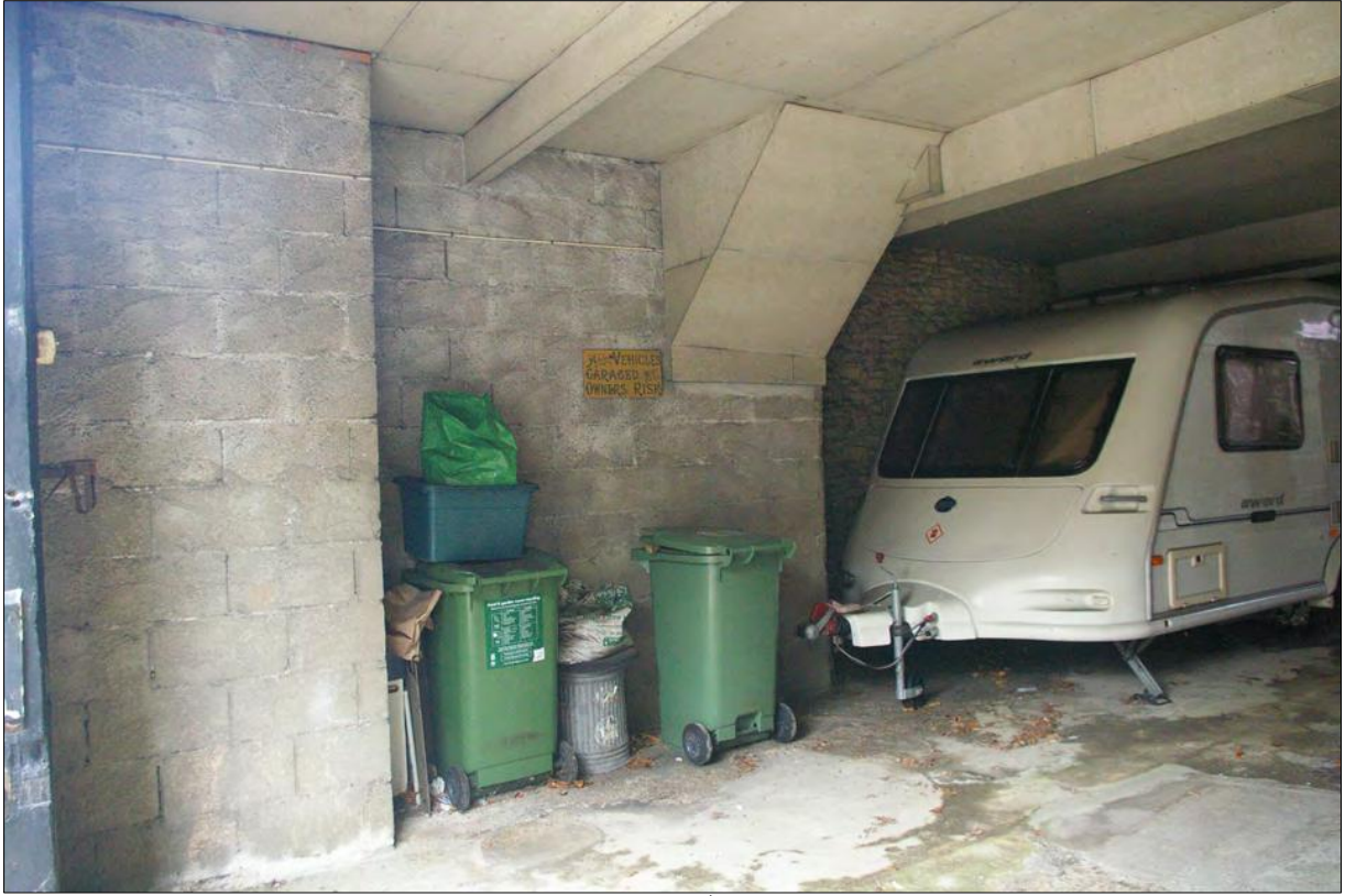
The concrete block walls which support the stairs to the 20 th century first floor structure; from the south-west.
