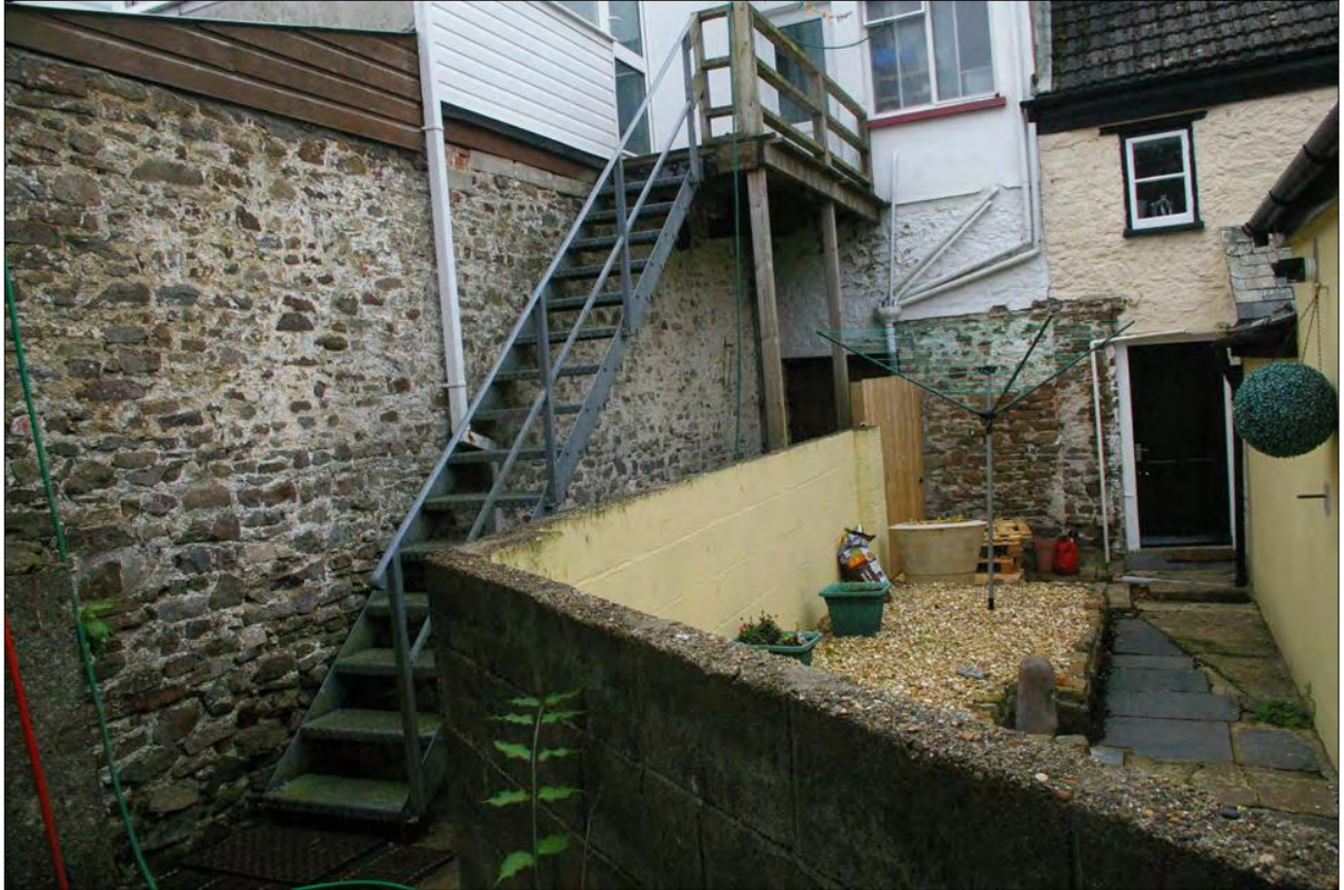
Figure 13: View of Area 4, from the doorway between Area 4 and Area 3, showing the boundary plot wall; viewed from the east-north-east.
