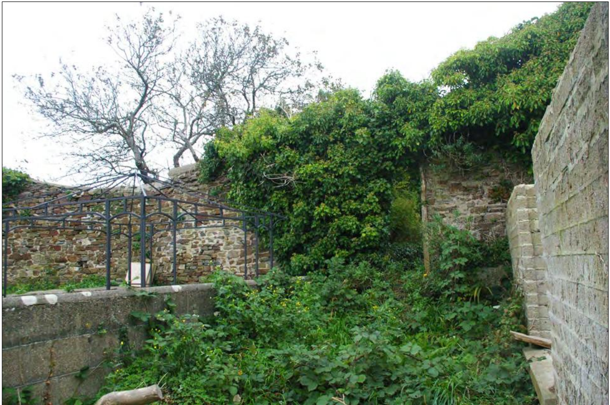
Figure 11: The overgrown Area 2, looking to the doorway leading to Area 1; viewed from the south-west.
