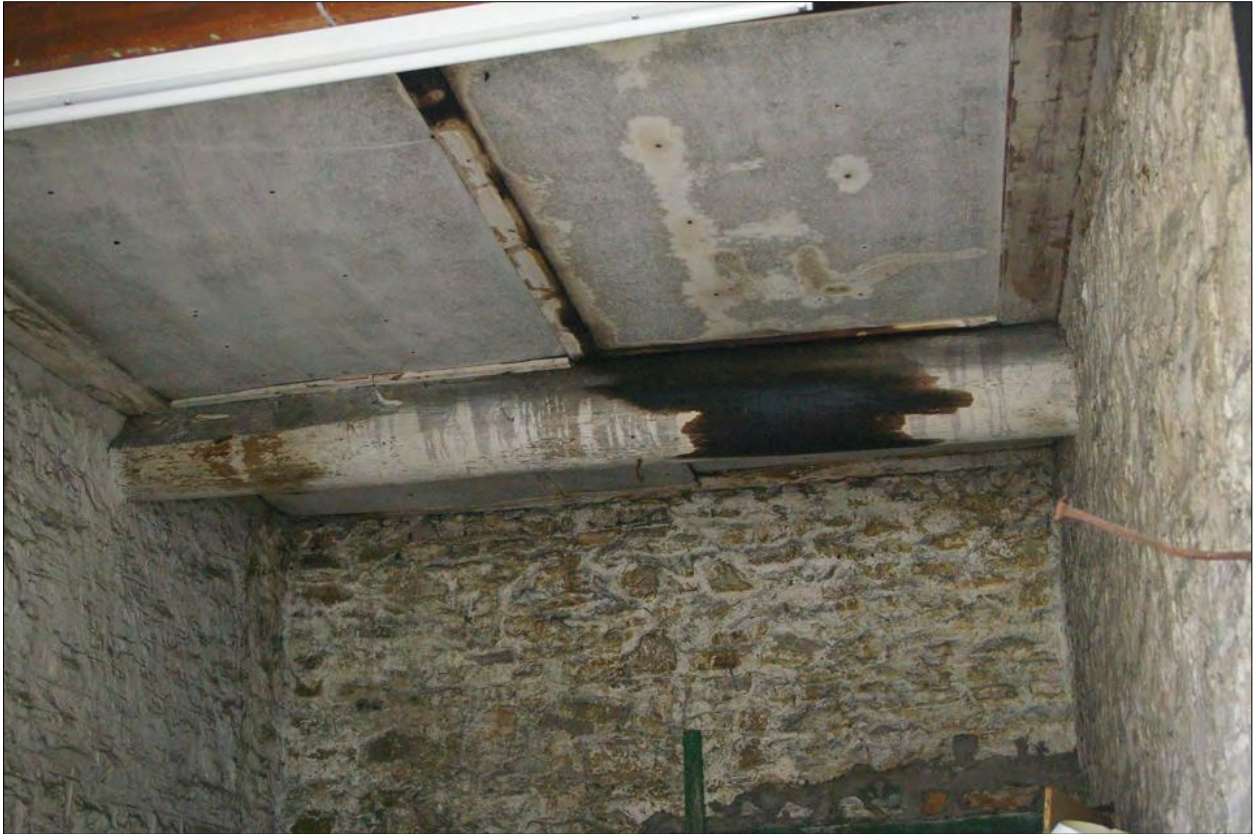
The modern boarded ceiling of Area 5 and the large former boat's mast beam; from the west, south-west.
