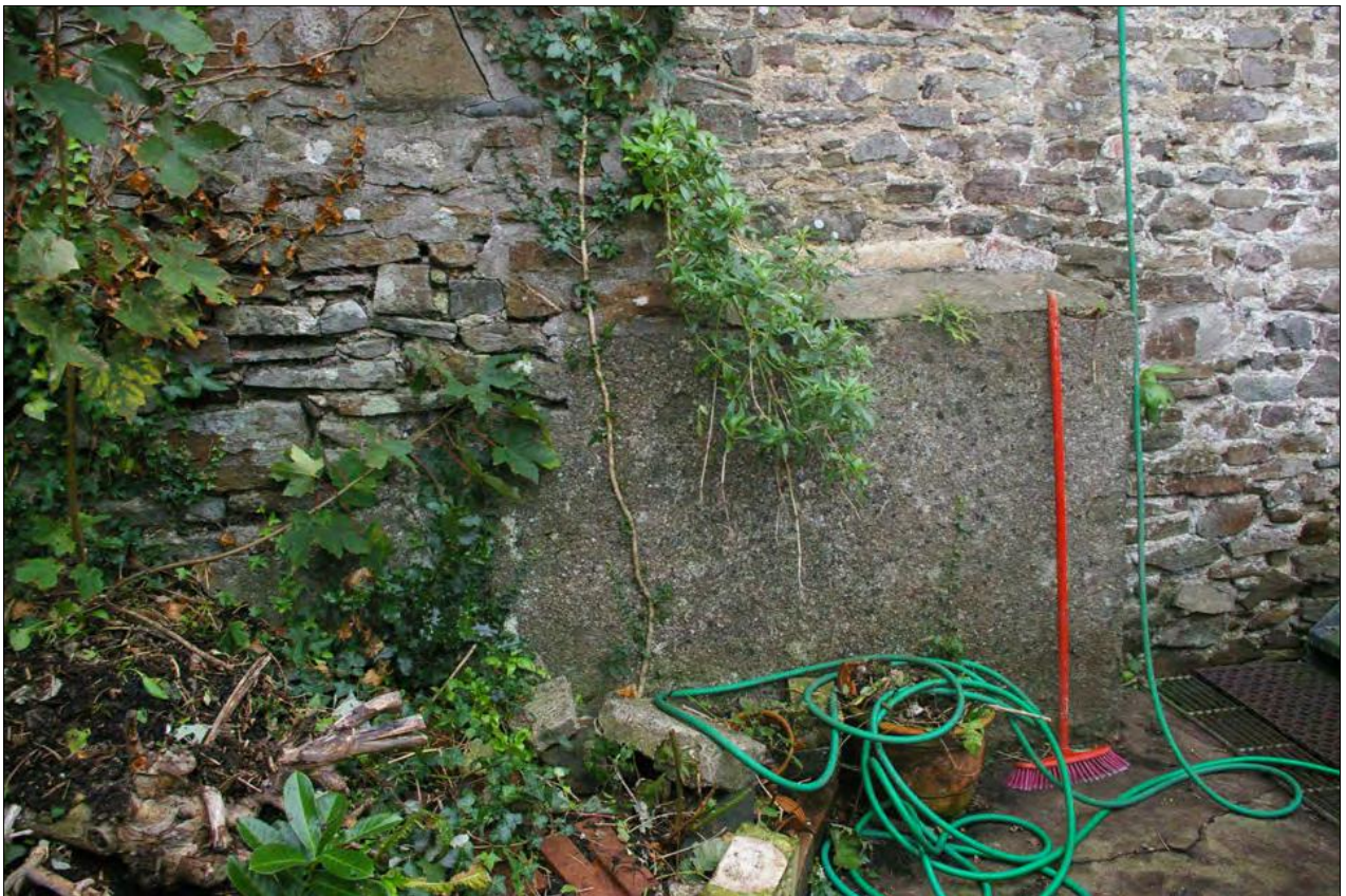
The rendered and buttressed stone areas in the south-east corner of Area 4; from the north-east.
