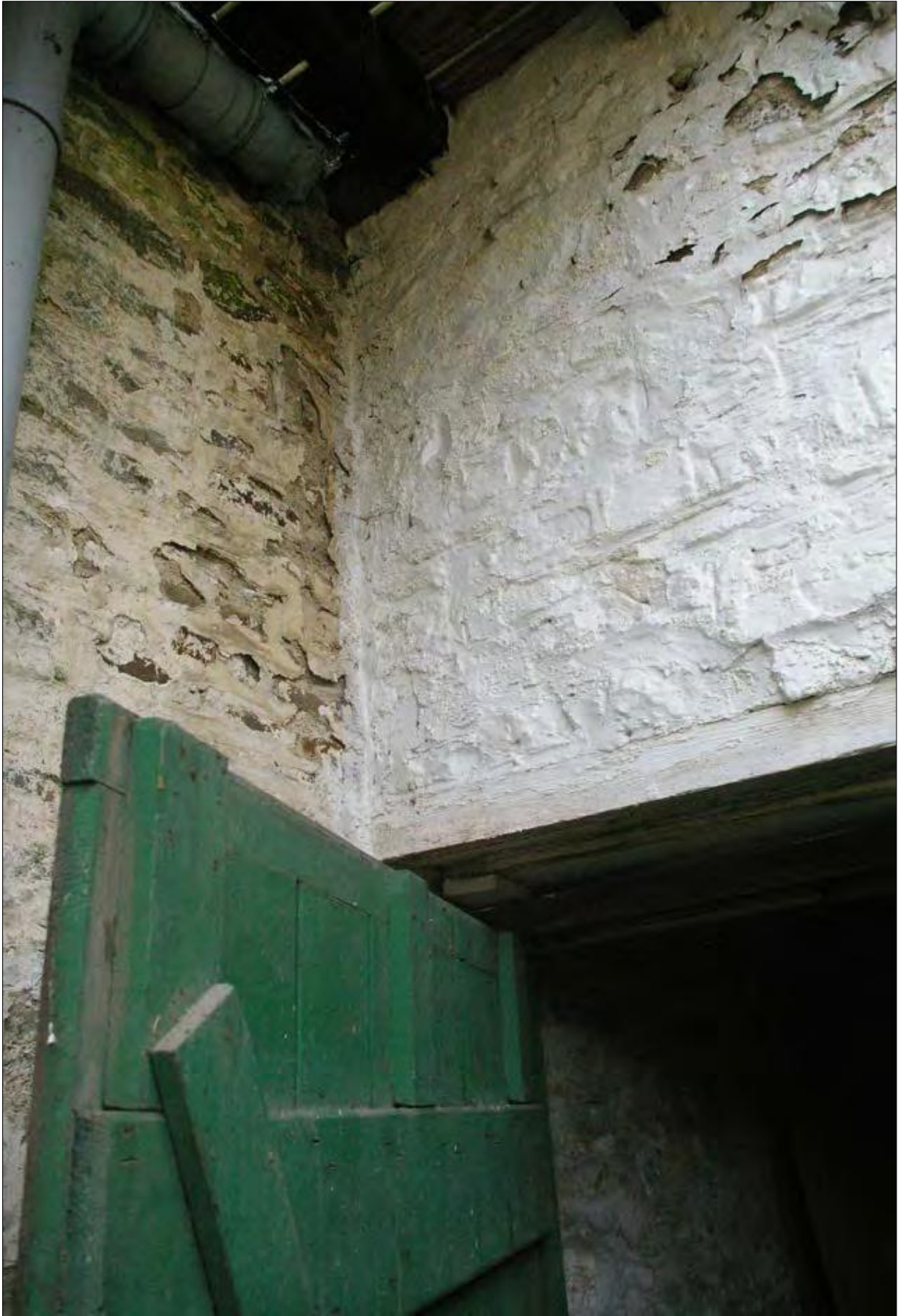
Detailed view of the south-west corner of Area 4, where the east wall of Area 5 meets the boundary plot wall; from the north-east.
