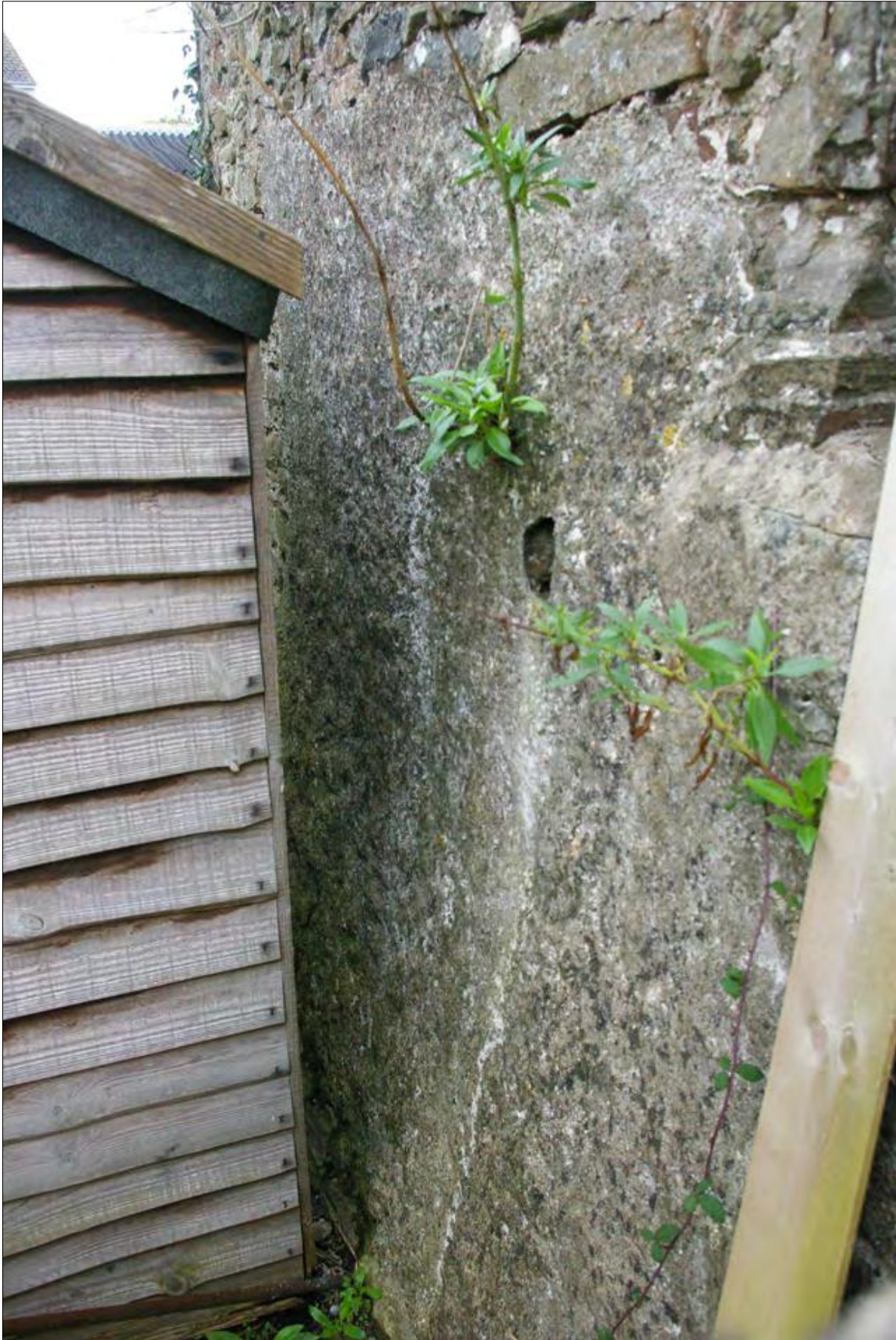
The lower part of the stone wall between Areas 3 & 4, rendered to the base, within Area 4; from the south.
