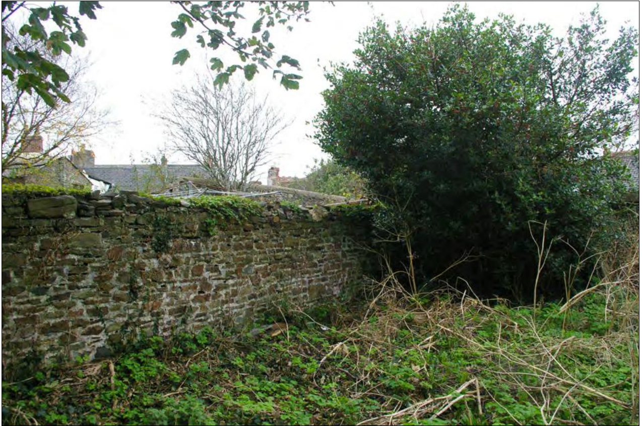
View of the south-west corner of Area 1, where the south wall meets the structure built over Area 6; from the north-east.
