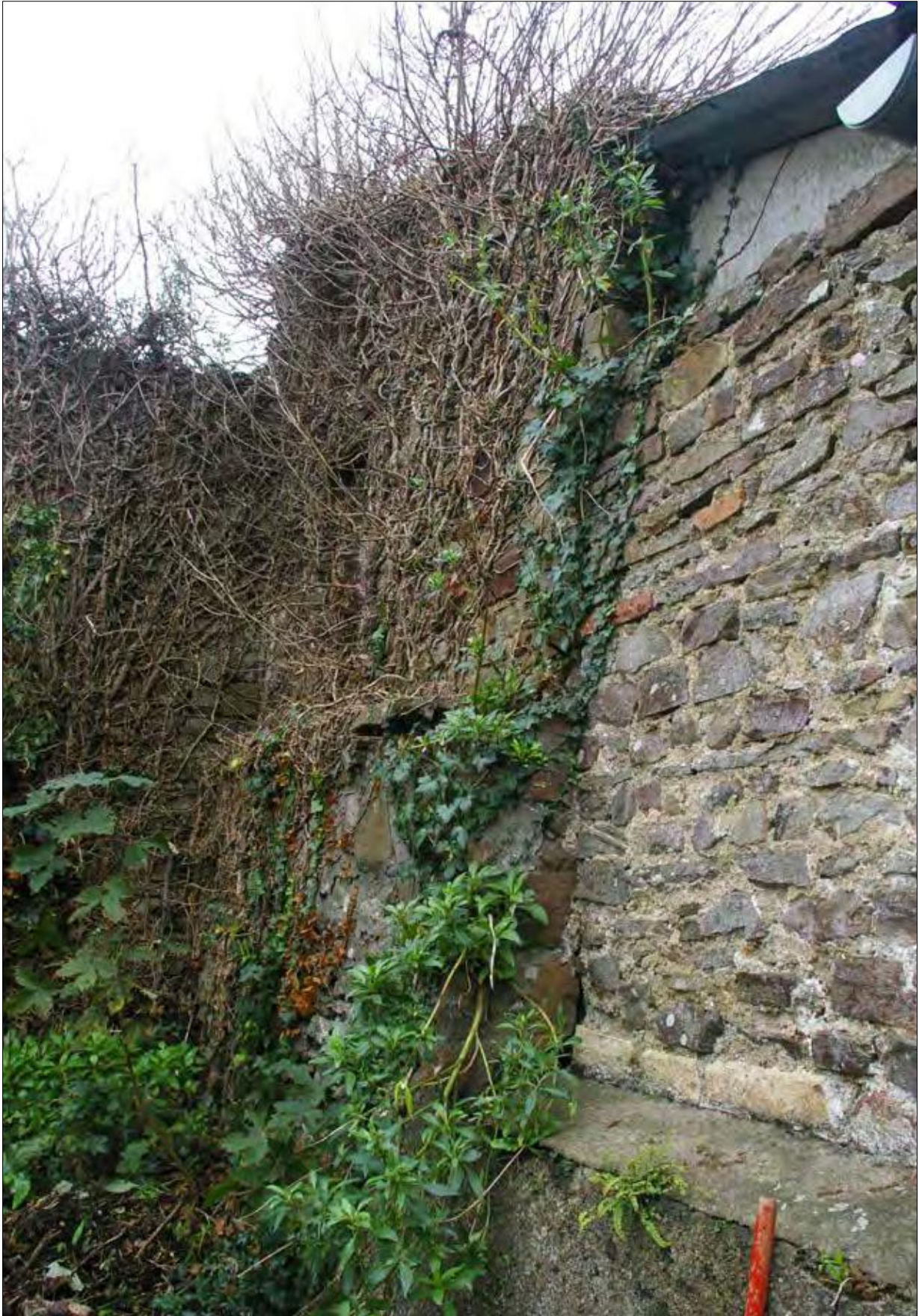
The former gable end of a building and other phases of stonework, seen to the south-east corner of Area 4; from the west-north-west.
