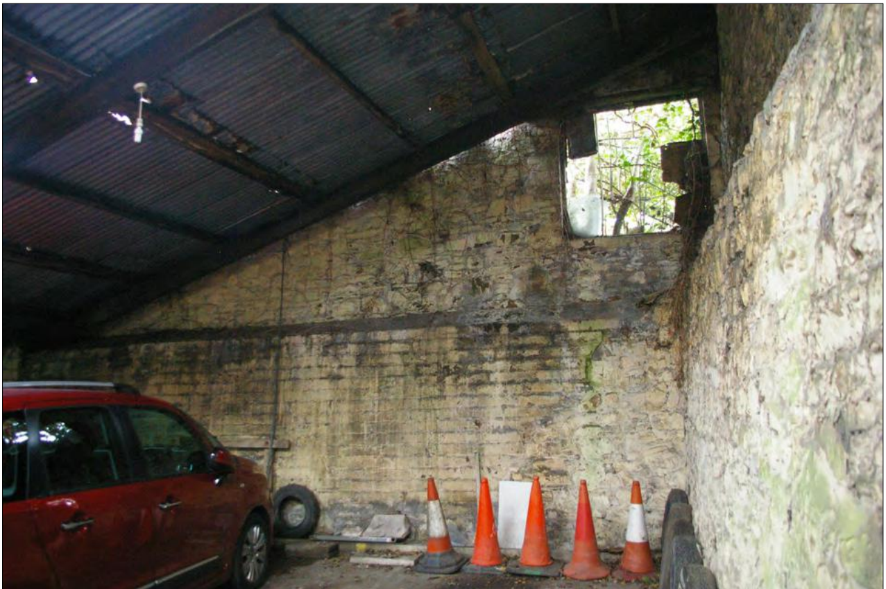
The east wall of Area 6, the party wall with Area 1, of stone but buttressed to the base in concrete blocks; from the west-south-west.
