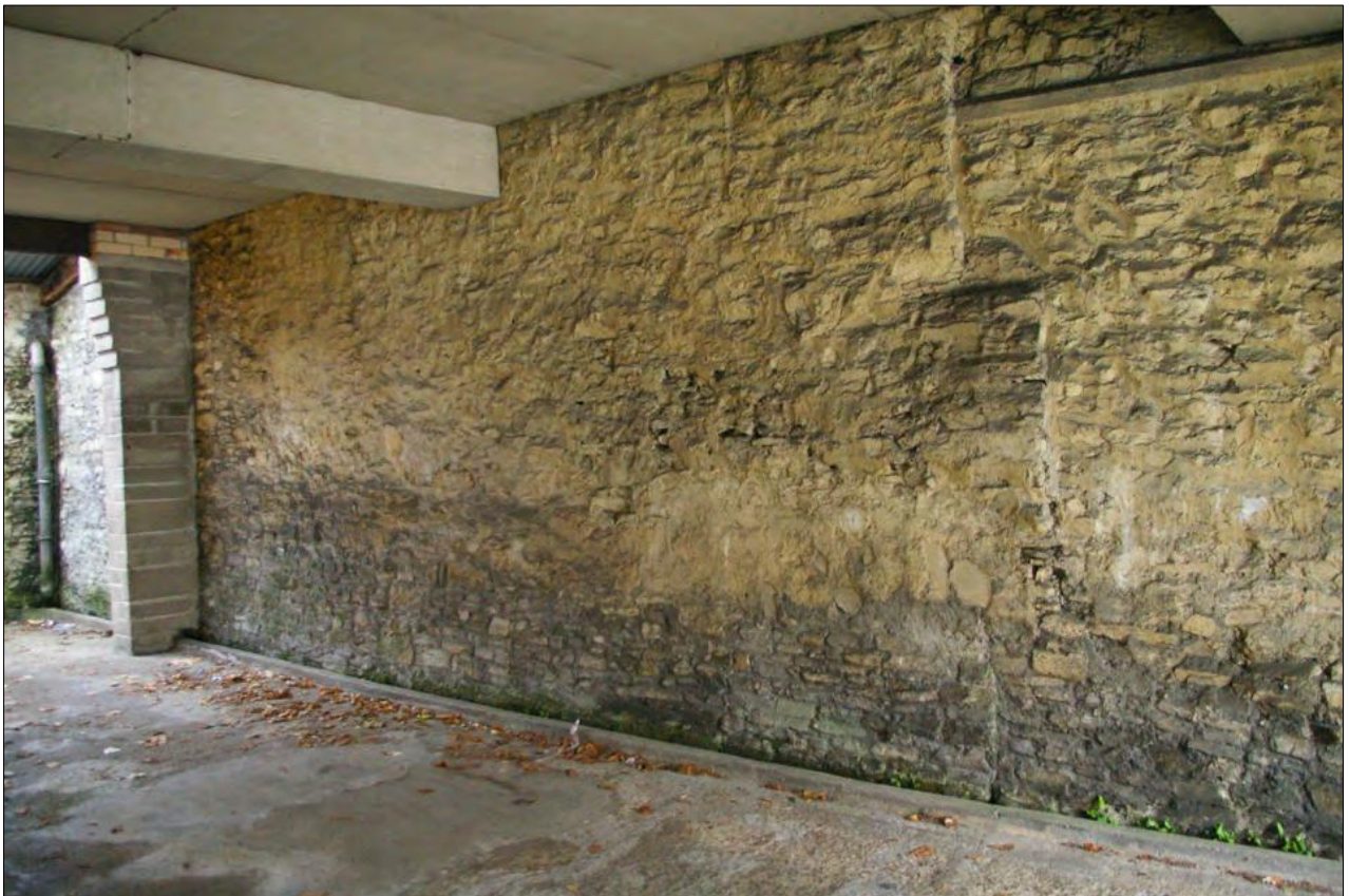
The western end of the south wall in Area 6, showing disturbance and several phases of possible rebuilding; from the north-west.
