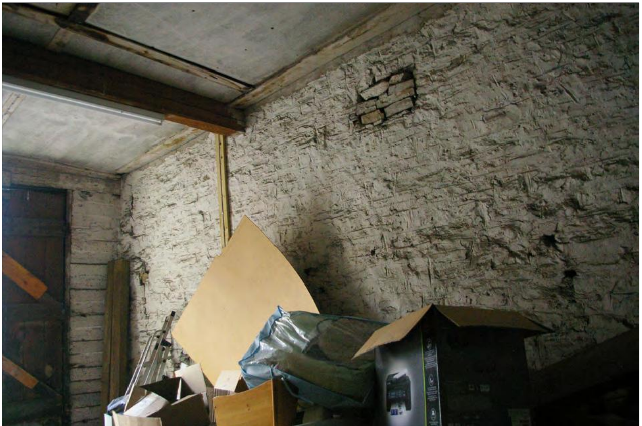
View of the north wall in Area 5, the shared part wall with the adjoining Listed Building; from the south-east.
