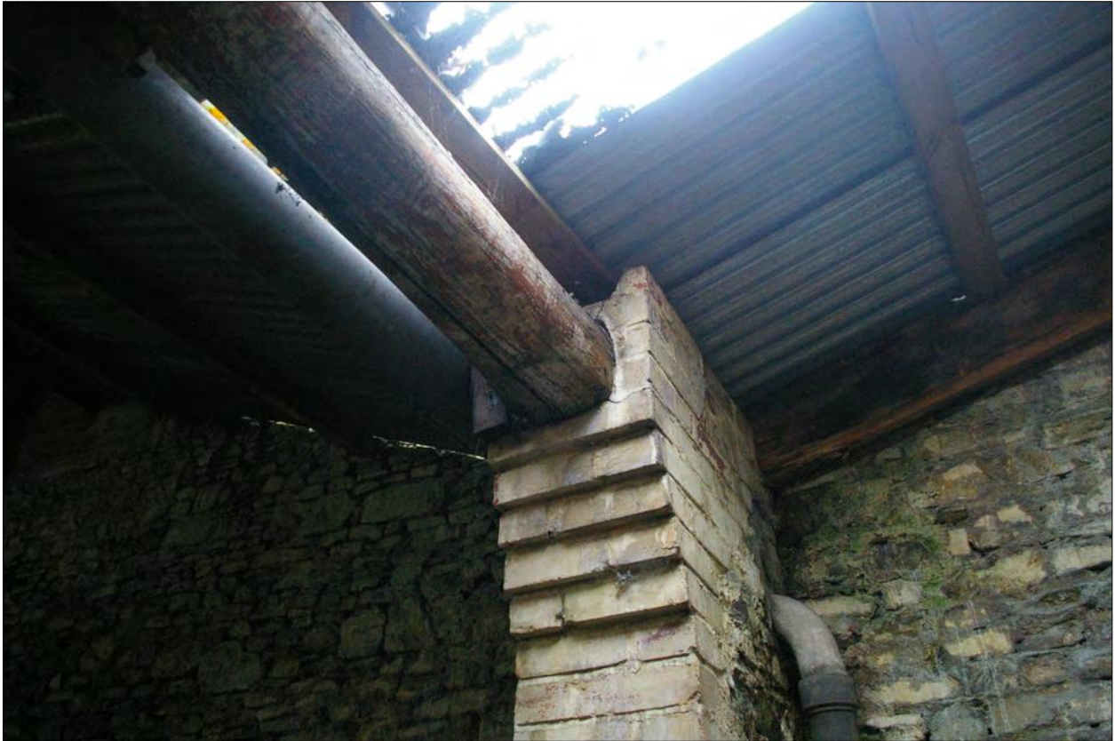
One of the brick pillars supporting the roof in Area 6, with a cut down boat mast used as a supporting beam; from the north-west.
