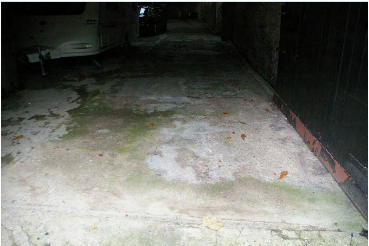
The concrete floor of Area 6, to the western end, showing the position of the underground fuel tank; from the west.
