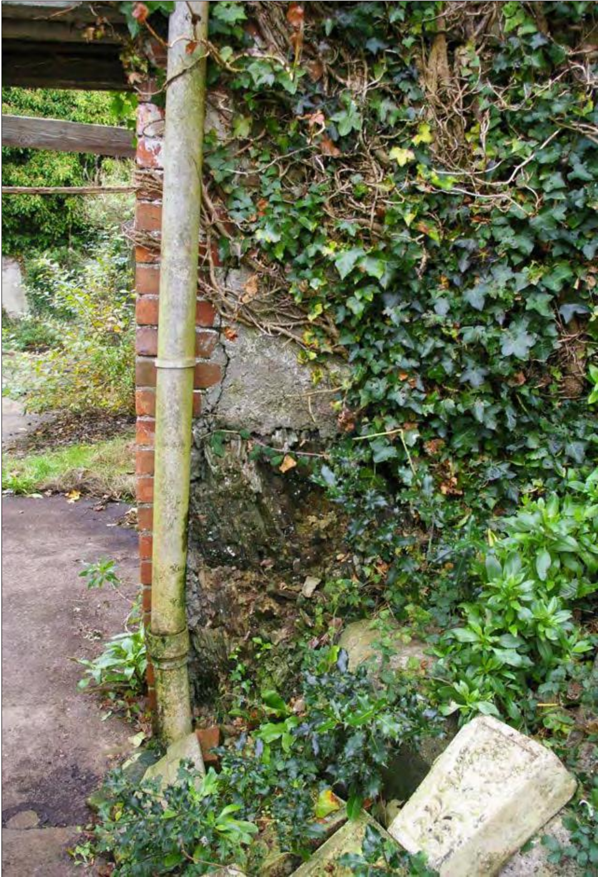
The doorway to Area 3, in the stone wall between Areas 3 & 4, showing the wall built on a rock outcrop; from the west.
