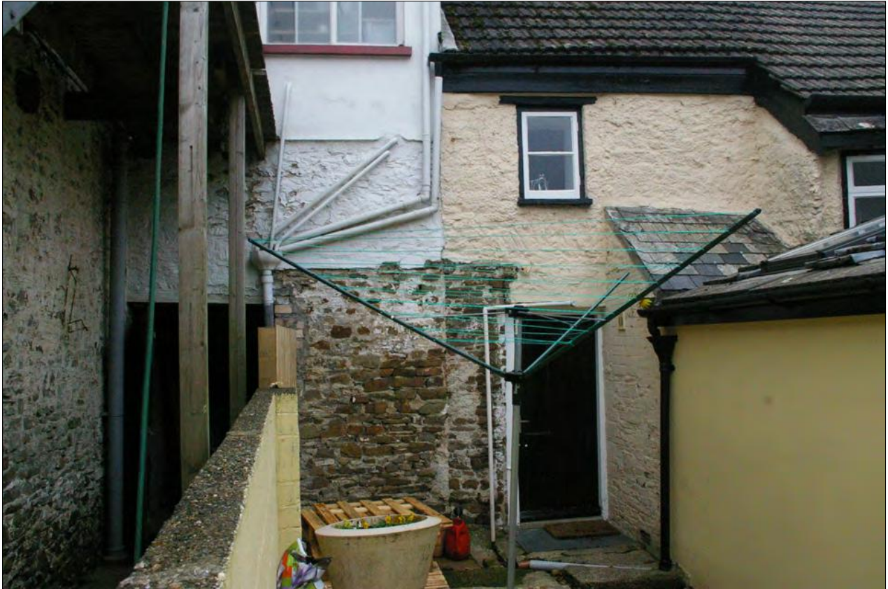
The rear of No.20 and Nos.18-19 Fore Street, showing the east wall of Area 5 and how it abuts the earlier building to the north; from the east.
