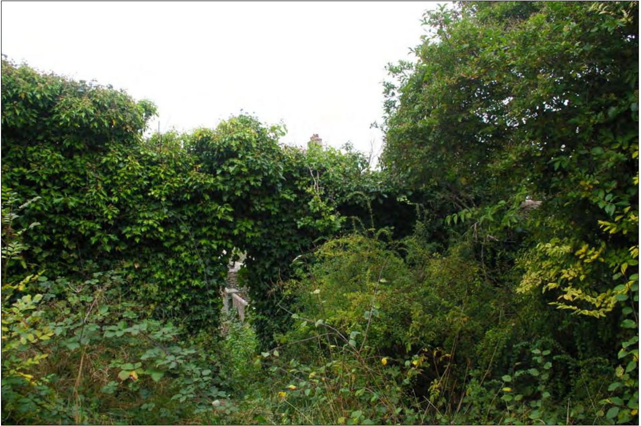
View of the ivy clad wall to the west of Area 1, with door to Area 2; from the east-south-east.
