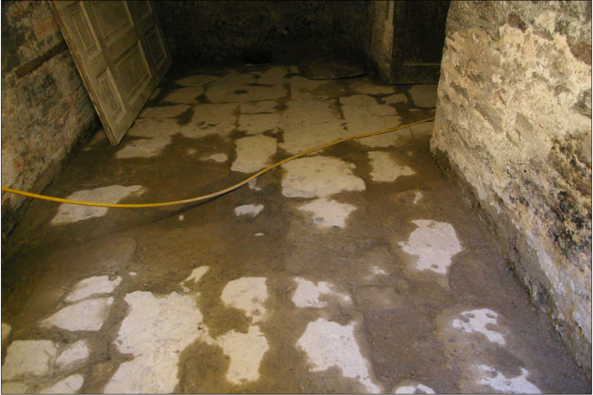
The stone slab floor in the lobby of Area 1; from the west.
