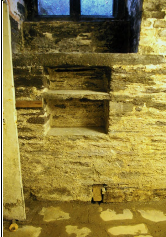
The keeping place in the south wall under the first window; from the north.
