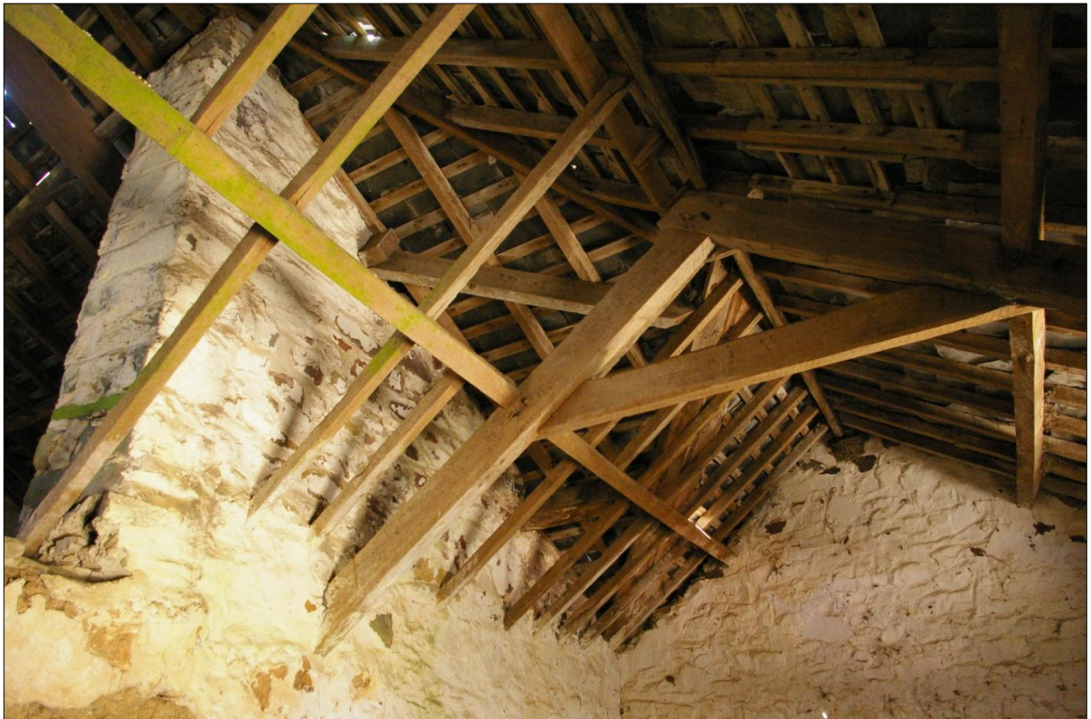
Figure 15: Detail of the roof structure within B7, showing the earlier double-pitch roof replaced with a single-pitch cat-slide roof; viewed from the east-north-east.
