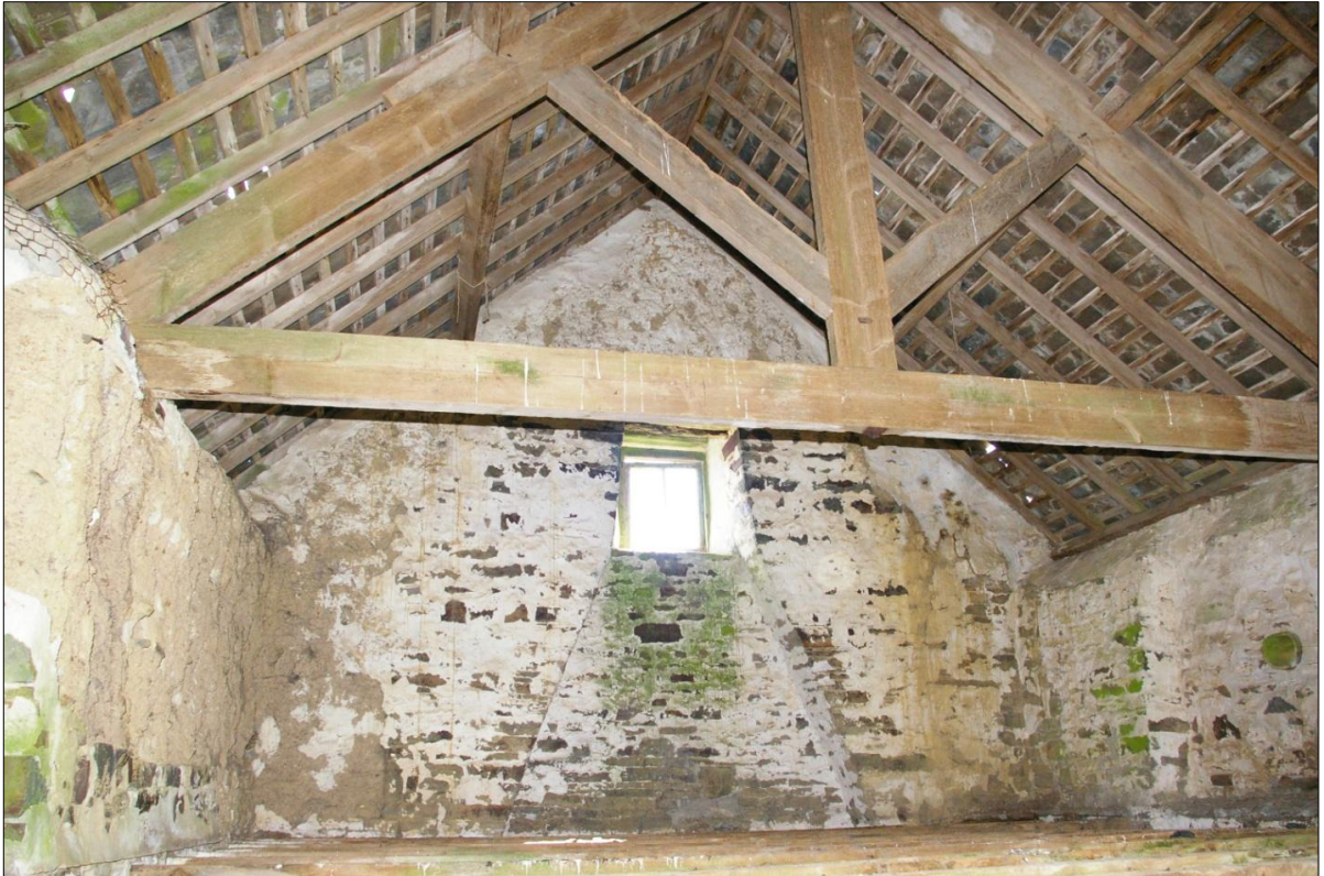
Figure 12: Detail of the east, interior wall of B1 showing the upper portion of the stack; viewed from the north-west.
