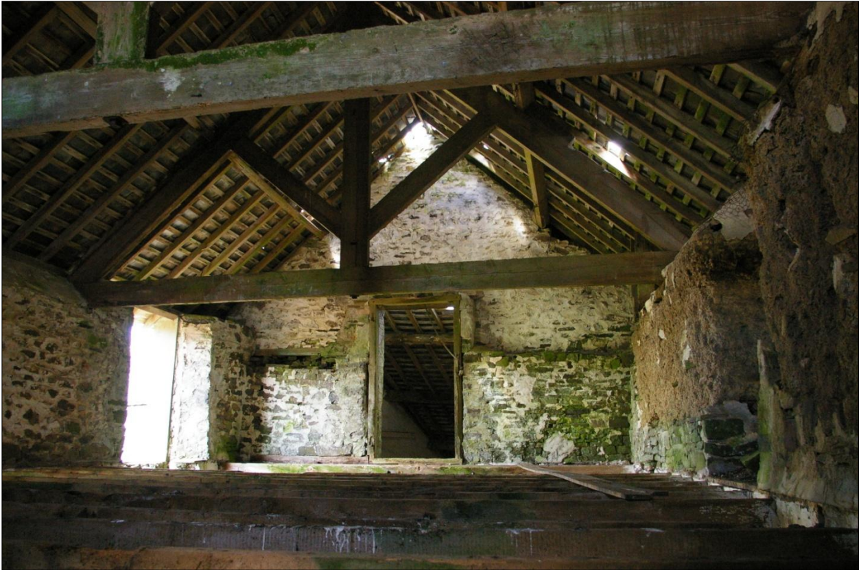
View of the west wall of Building 1, internal face, showing the first floor level; viewed from the east-north-east.
