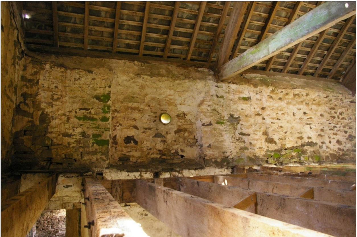
The south wall of Building 1, internal face, at first floor level showing the blocked window; viewed from the north-east.
