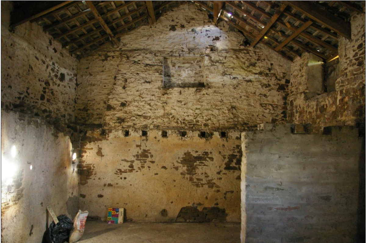
Figure 13: The north wall of B2, showing the remains of a stack and a window forced into that stack; viewed from the south.
