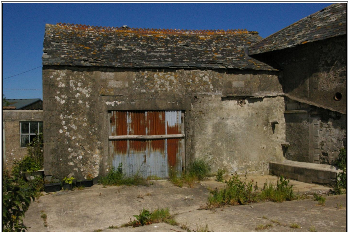
Figure 16: East wall of B2 showing remnants of roof structure to B12; viewed from the south-east.
