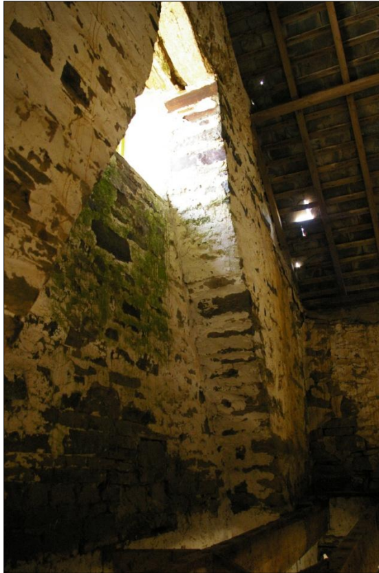
The east gable of Building 1, internal face, showing the potential chimney stack with window forced into the top, at first floor level; viewed from the north-west.
