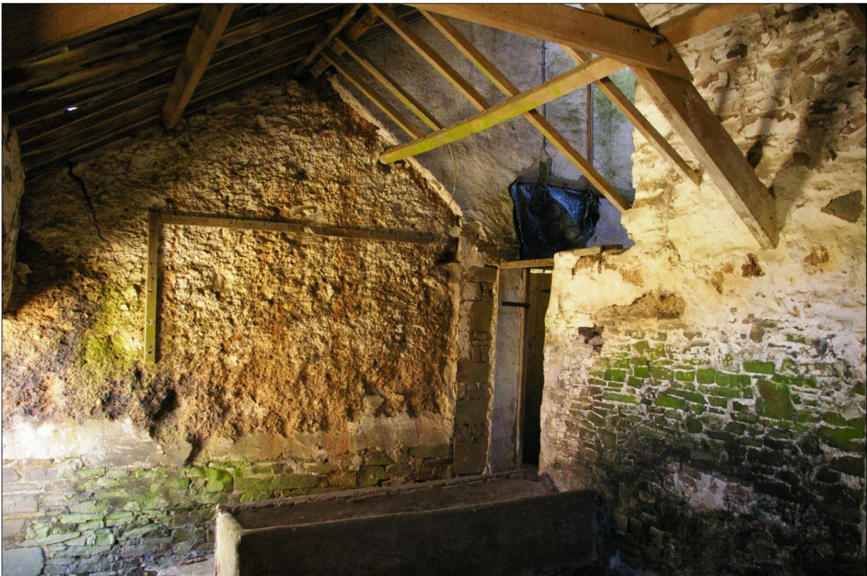
The east and south walls of Building 7, internal faces, showing the forced doorway into Building 8 and the relationship to Building 1; viewed from the north-west.
