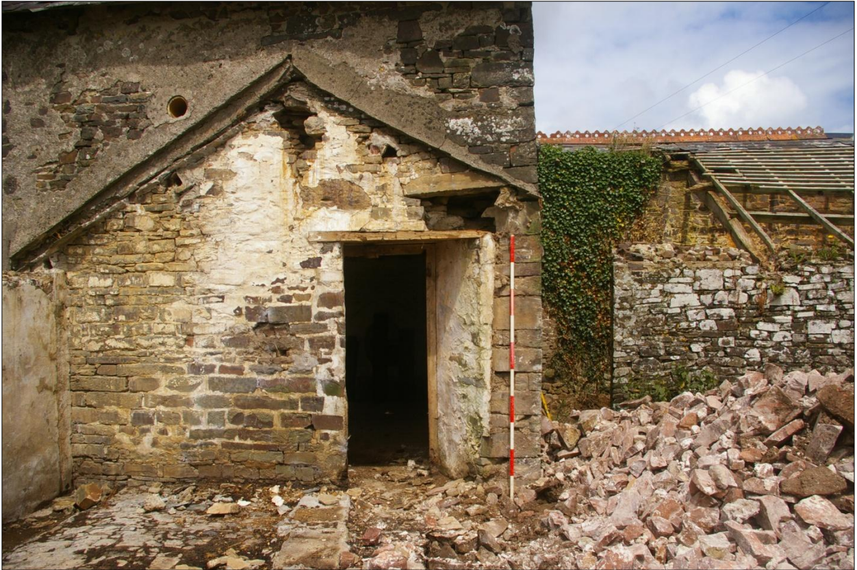
View of the south-east corner of B1 after the demolition of the east wall of B4, Area #3, showing the dressed stones of B1 and that B4 abutted and was not keyed in; viewed from the south (2m scale).
