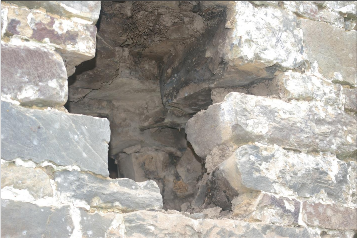
Detail of the wall construction of the east gable of B1; viewed from the south-east.
