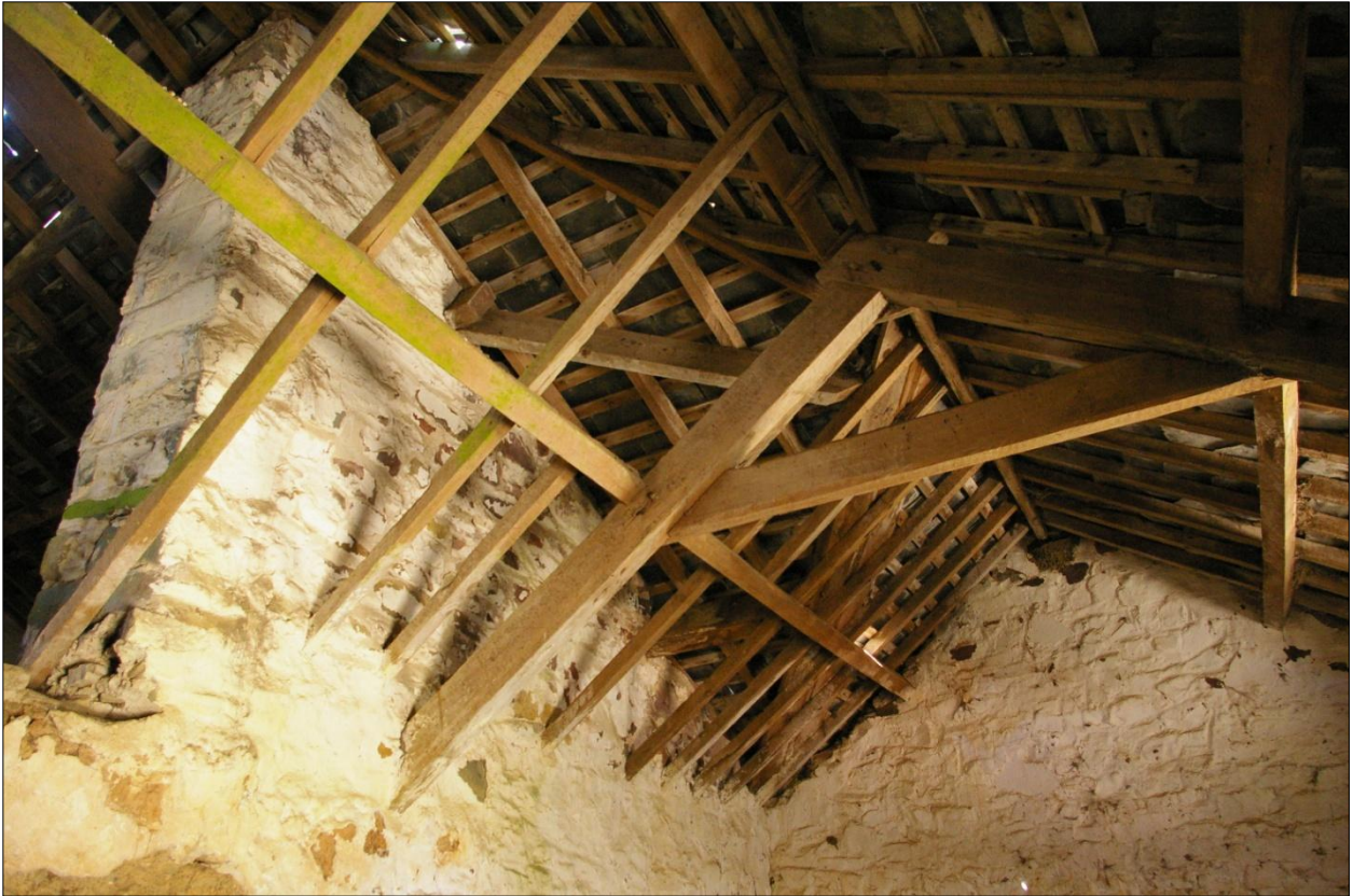
The pegged and bolted A-frame roof within Building 7, which survives within the modern roofing, which runs over the top; viewed from the north-east.
