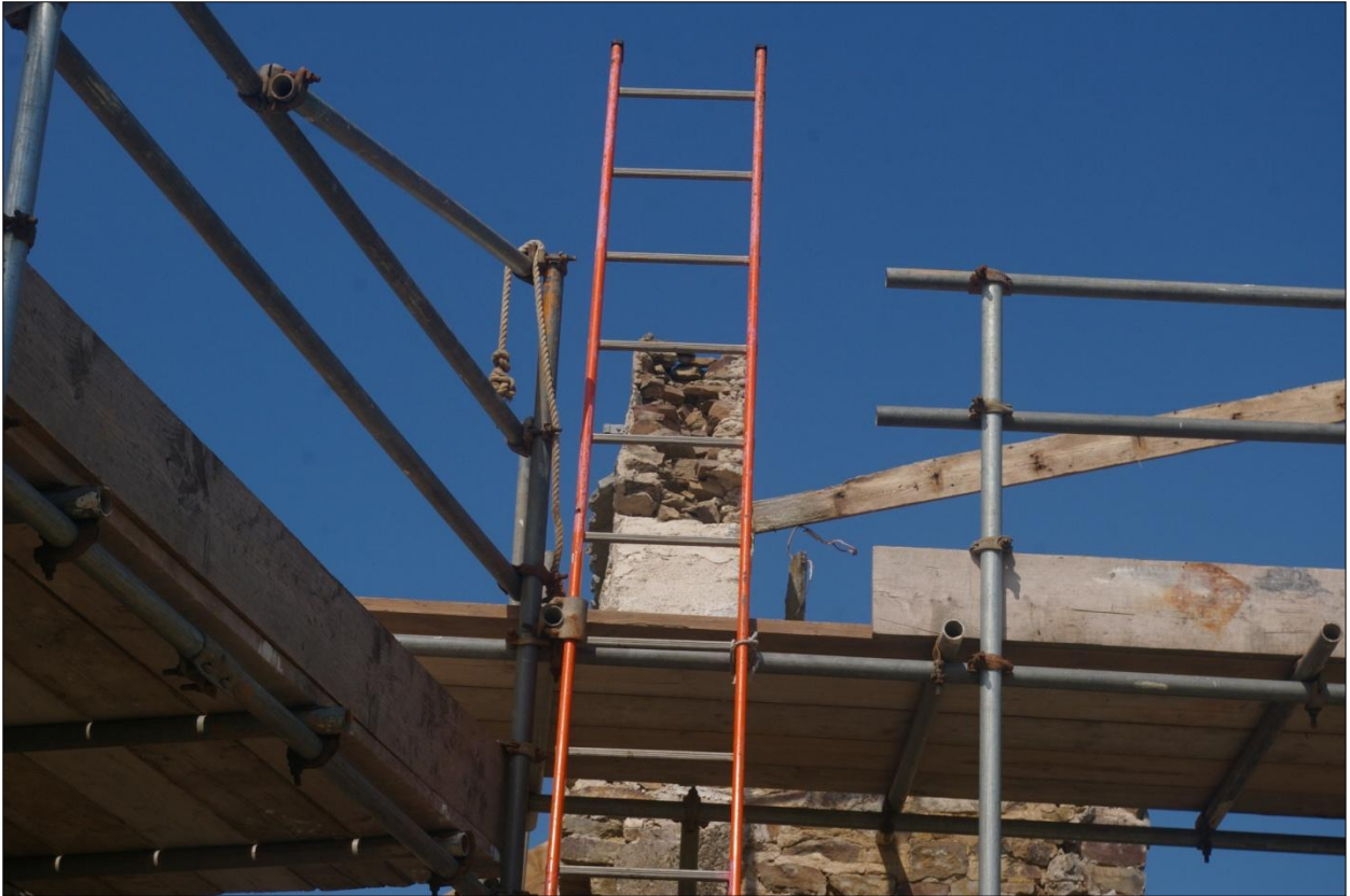
Detail of construction of west gable end of building 1; viewed from the south.
