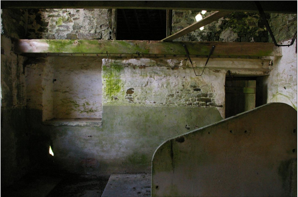
The west wall of Building 1, internal face, showing the blocked window at ground floor level; viewed from the east.
