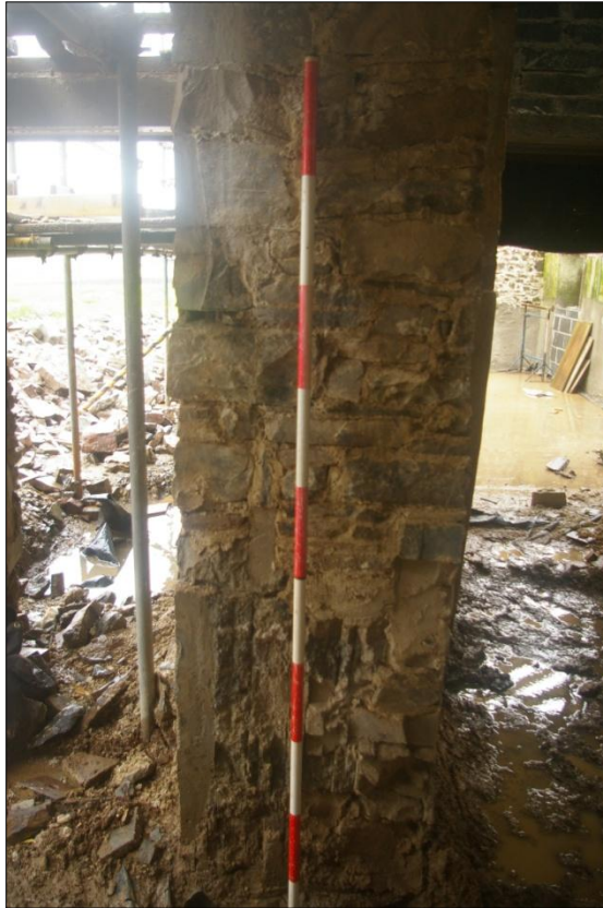
Recent forced opening through east wall of B1 showing recent wall repairs, Area #5; viewed from the north (2m scale).
