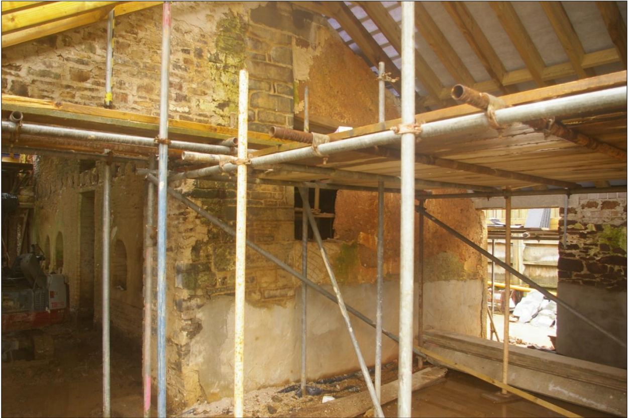
View of east wall of building B1, external face, Area #5; viewed from the south-east (no scale).
