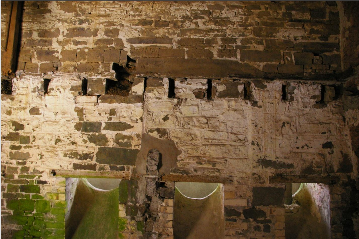
The south wall of Building 3, internal face, showing detail of the joist sockets forced into the external north wall of Building 1, to carry the loft within Building 3; viewed from the north.
