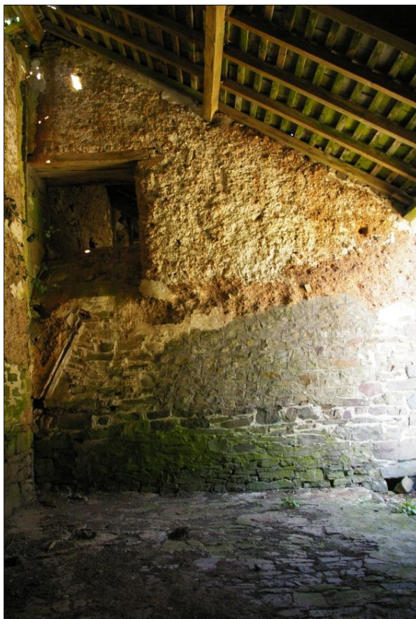
Figure 10: East interior face of B3 showing combination of stone and cob build; viewed from the west.
