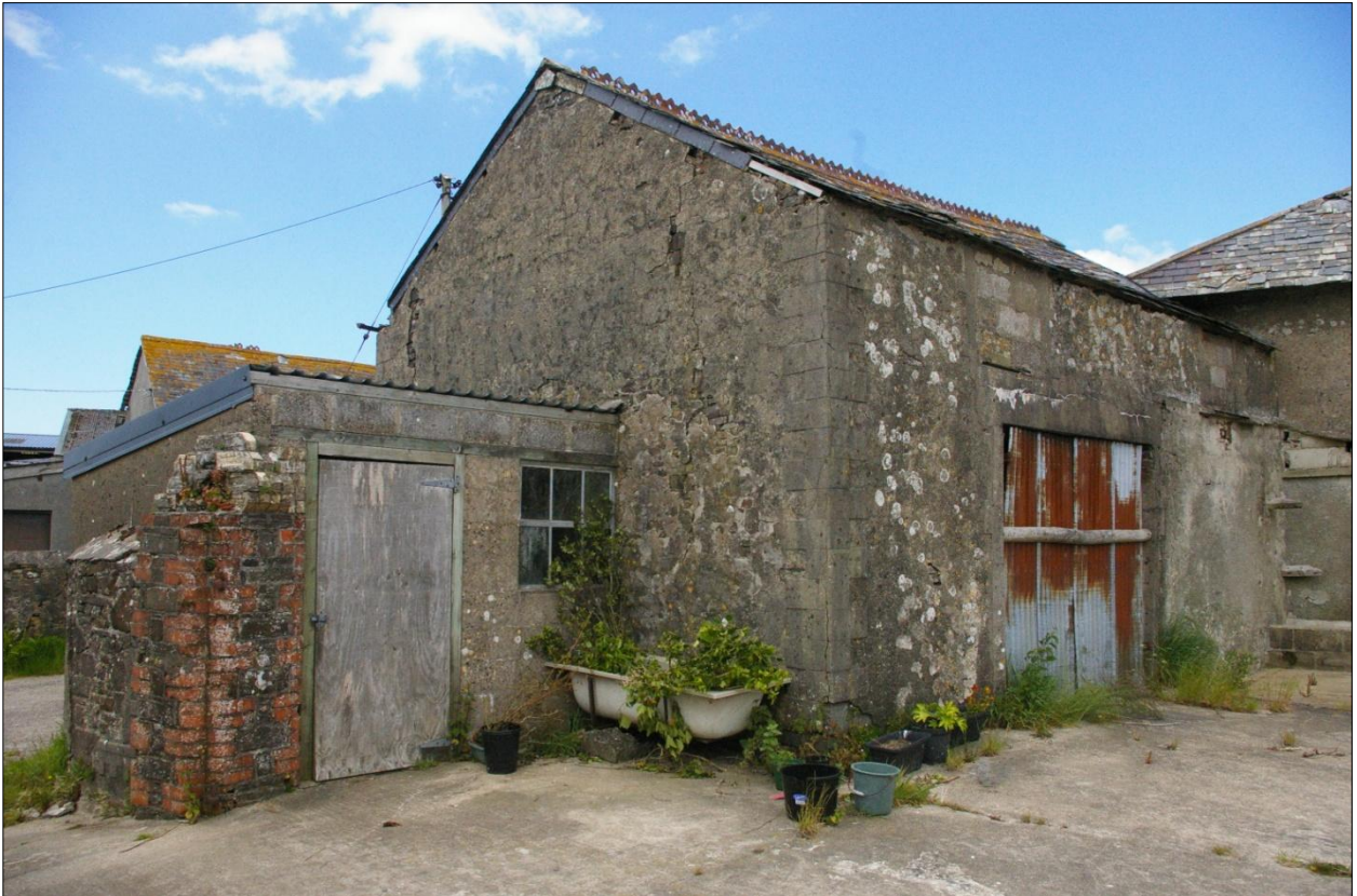
The east and south walls of Building 2, showing Building 9 abutting the south wall; viewed from the south-east.
