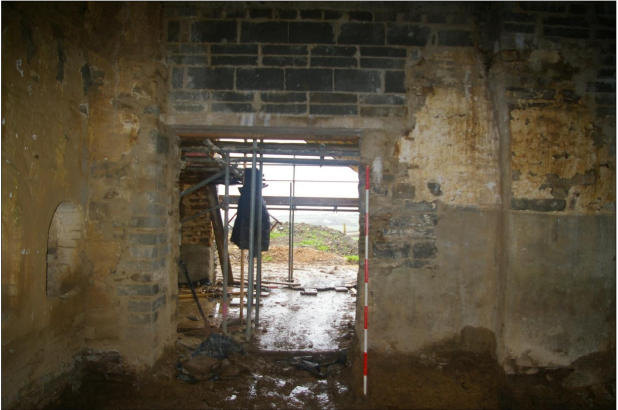
East wall of building B1, internal face after recent forced opening, Area #5; viewed from the west (2m scale).
