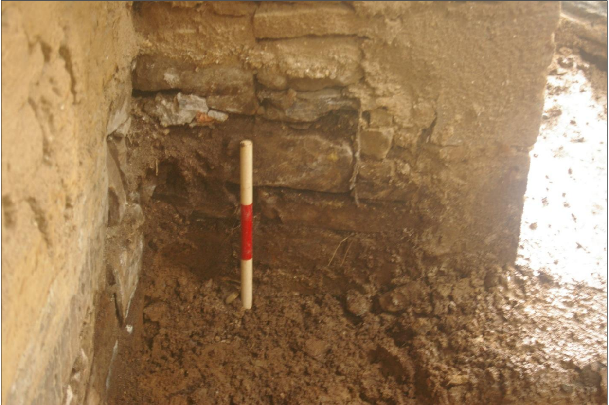
Detail of lower wall foundation of east wall, building B1, north end, Area #5; viewed from the west (0.3m scale).
