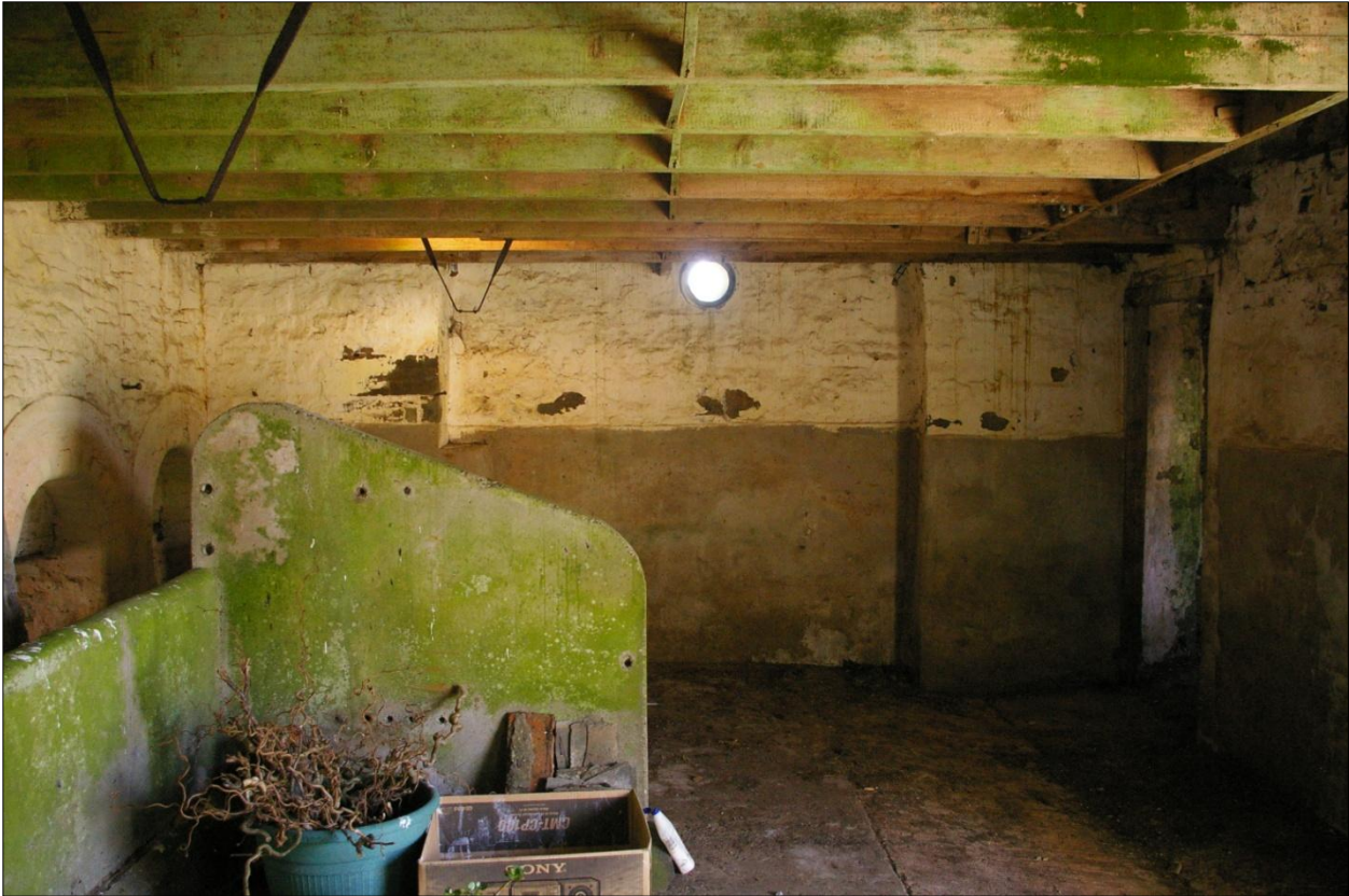
The east wall of Building 1, internal face, showing the potential chimney stack at ground floor level; viewed from the west.
