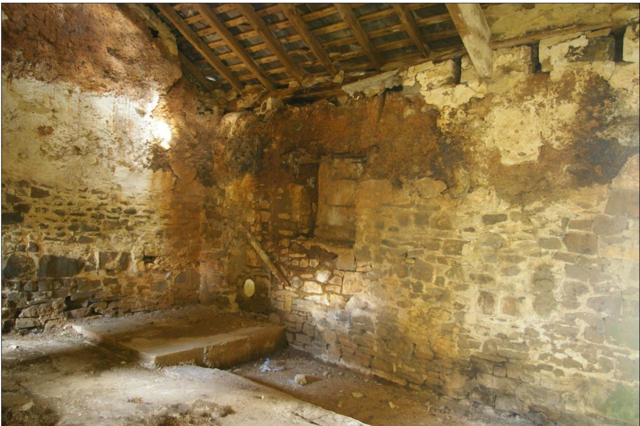
The north and west walls of Building 3, internal face; viewed from the south-east.
