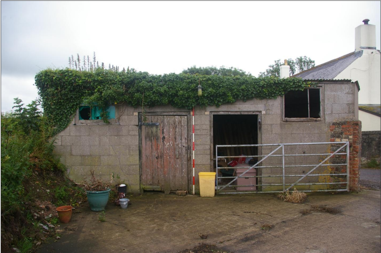
The north wall of Buildings 10 and 11; viewed from the north (2m scale).
