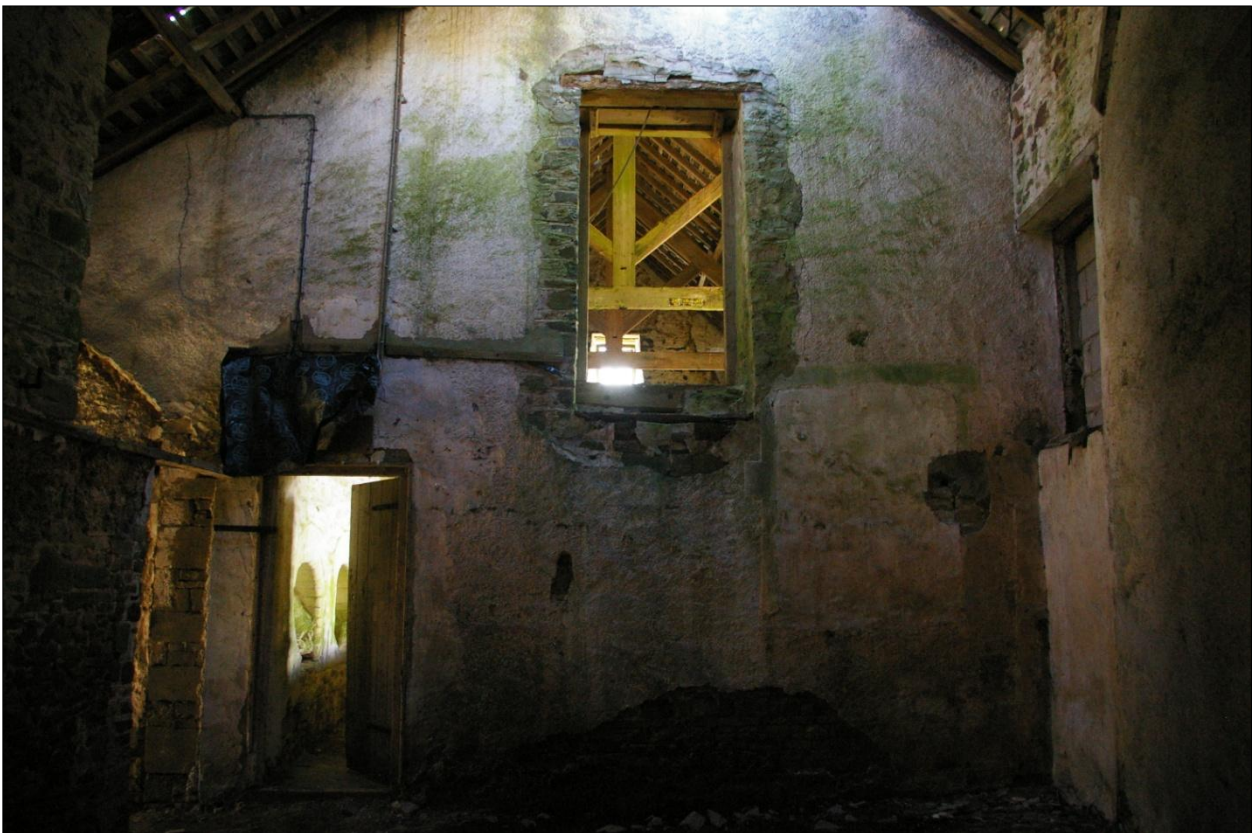
The east wall of Building 8, internal face, showing the external west wall of Building 1, from within Building 8; viewed from the west.
