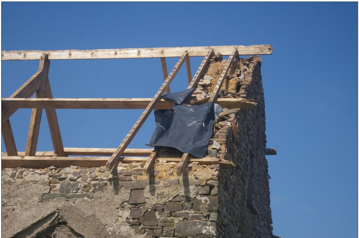
Detail of construction of east gable end of building 1; viewed from the south-east.
