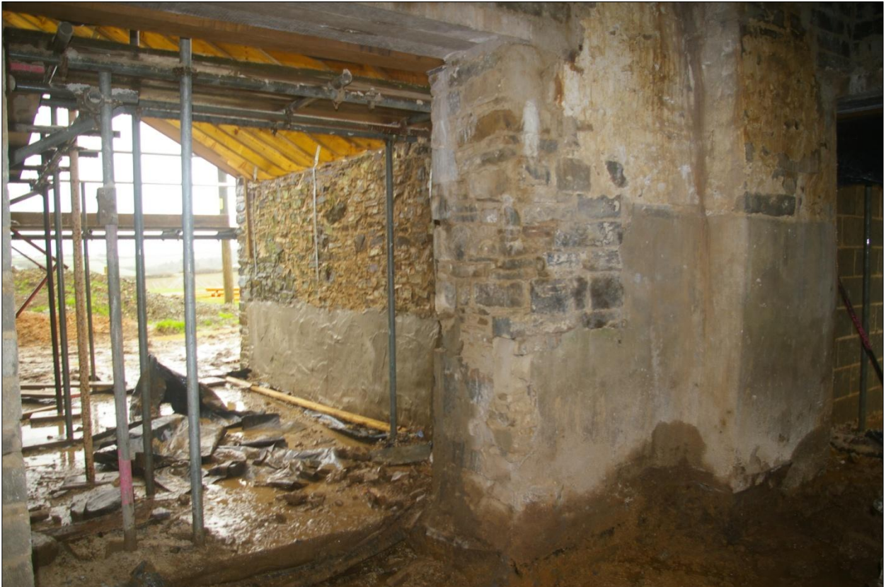
Detail of east wall of building B1, south end, Area #5; viewed from the north-west (no scale).
