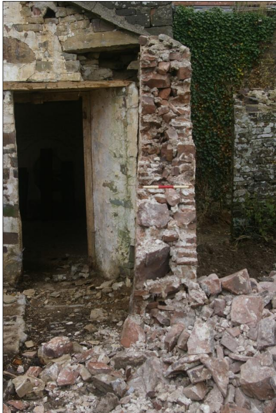
Detail of the construction of the east wall of B4, Area #3; viewed from the south (0.3m scale).
