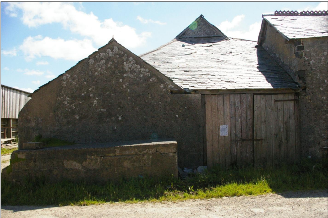
The west wall of Building 7, showing the west wall of infill Building 8; viewed from the west.
