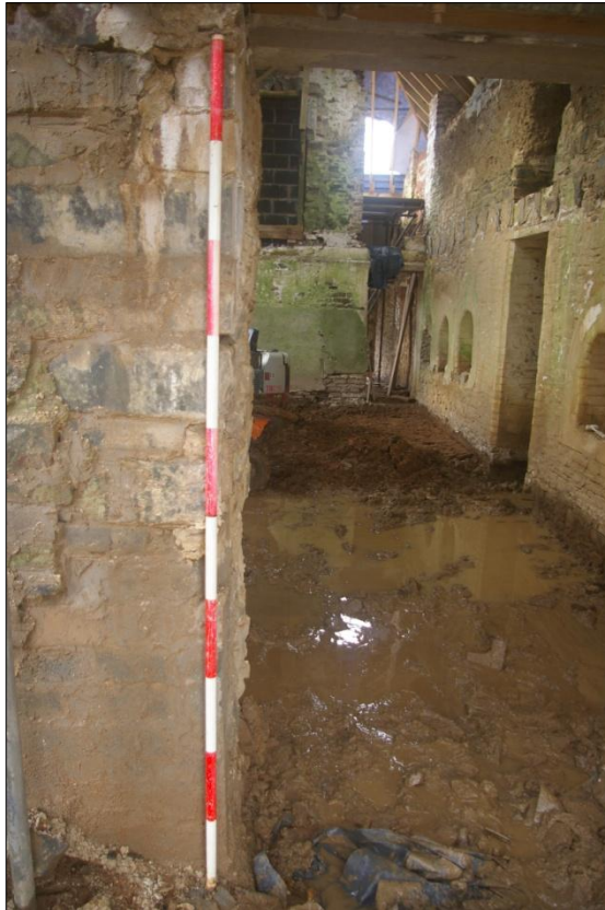
Detail of east wall of building B1, external face, south end of recent forced opening, Area #5; viewed from the east (2m scales).
