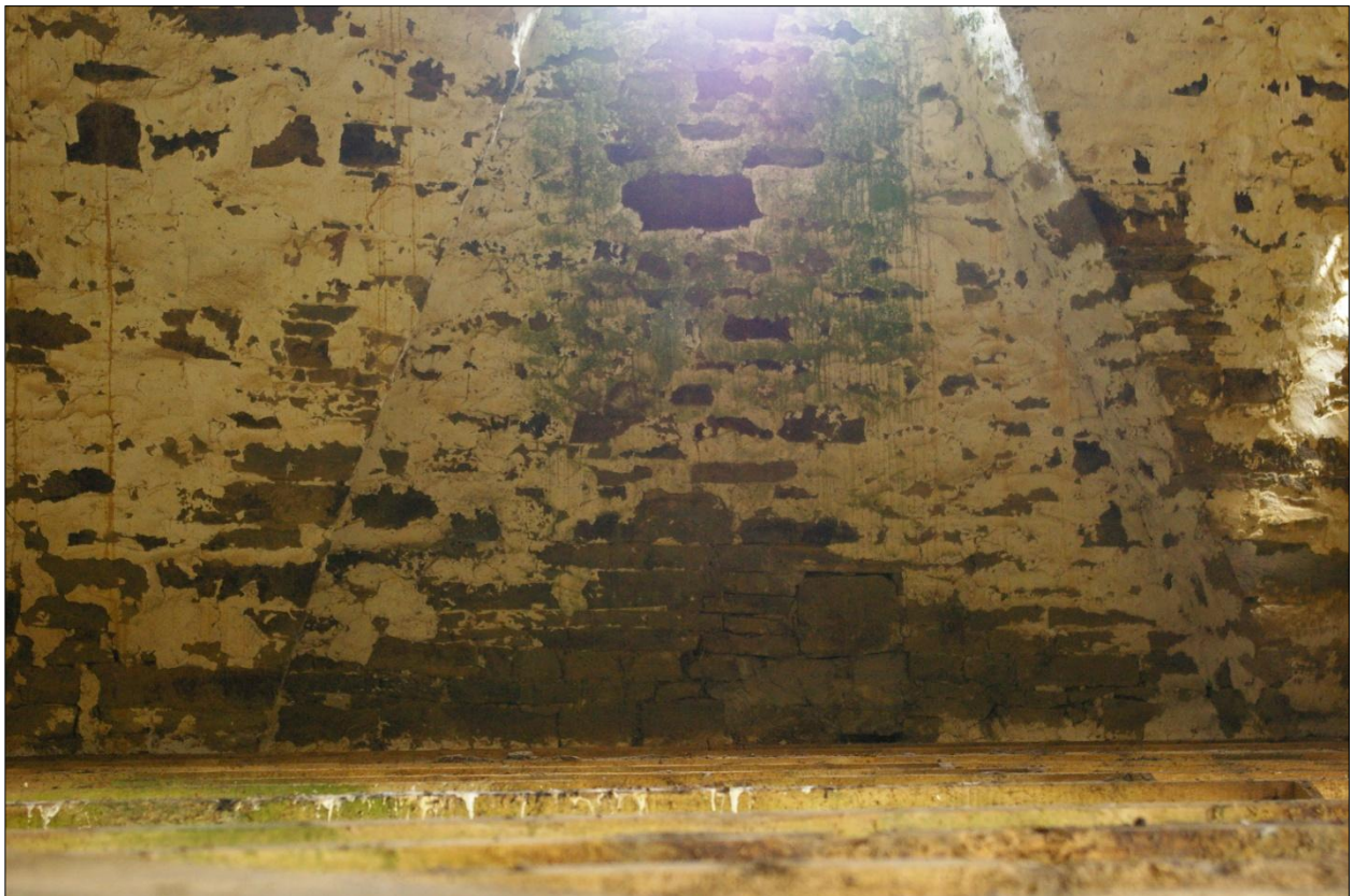
The east gable wall of Building 1, internal face, at first floor level, showing detail of the possible chimney stack structure, viewed from the north-west.
