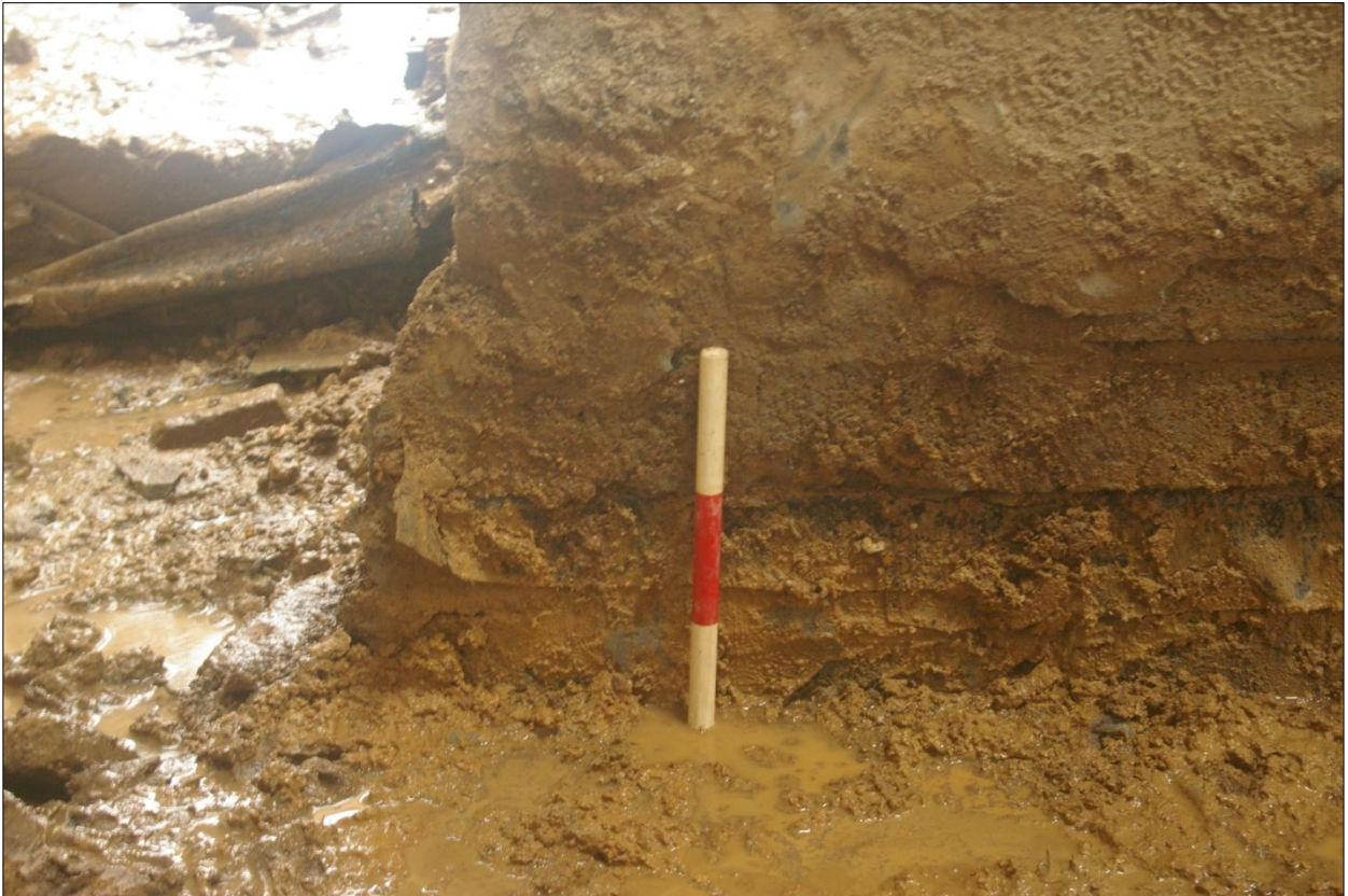
Detail of lower wall foundation of east wall, building B1, south end, Area #5; viewed from the west (0.3m scale).
