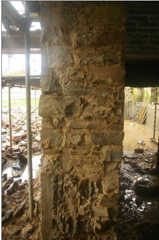
Detail of east wall of building B1 forced opening, south end, Area #5; viewed from the north (no scale).
