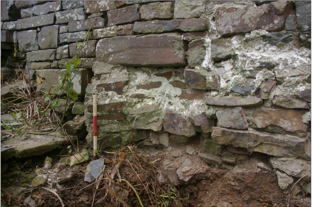
Detail of the blocking within the east gable of B1, possibly relating to the removal of an oven, Area #2; viewed from the north-east (0.3m scale).
