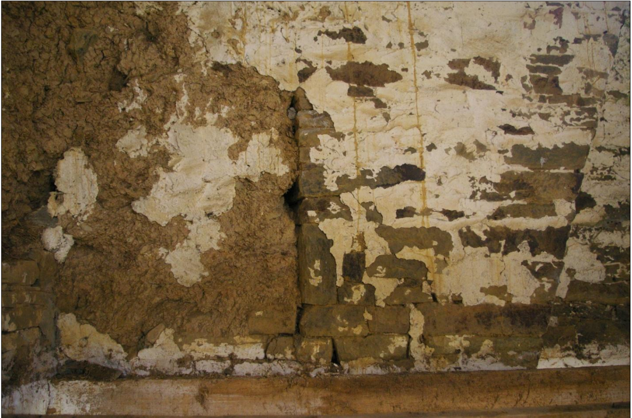
The east gable wall of Building 1, internal face, at first floor level, showing detail of the blocked window embrasure; viewed from the west
