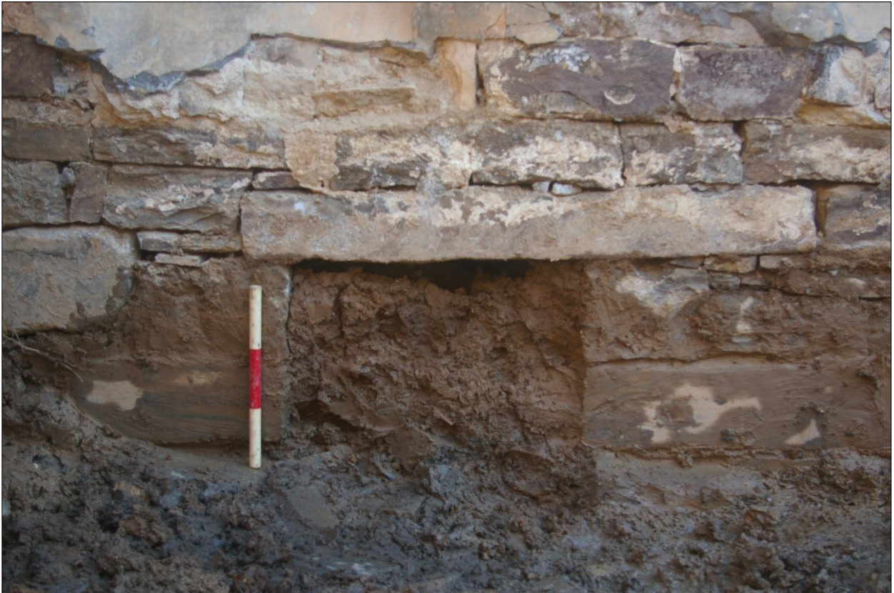
North elevation of building 1, external view during excavation of Area #4, showing forced opening below ground level; viewed from the north (0.3m scale).
