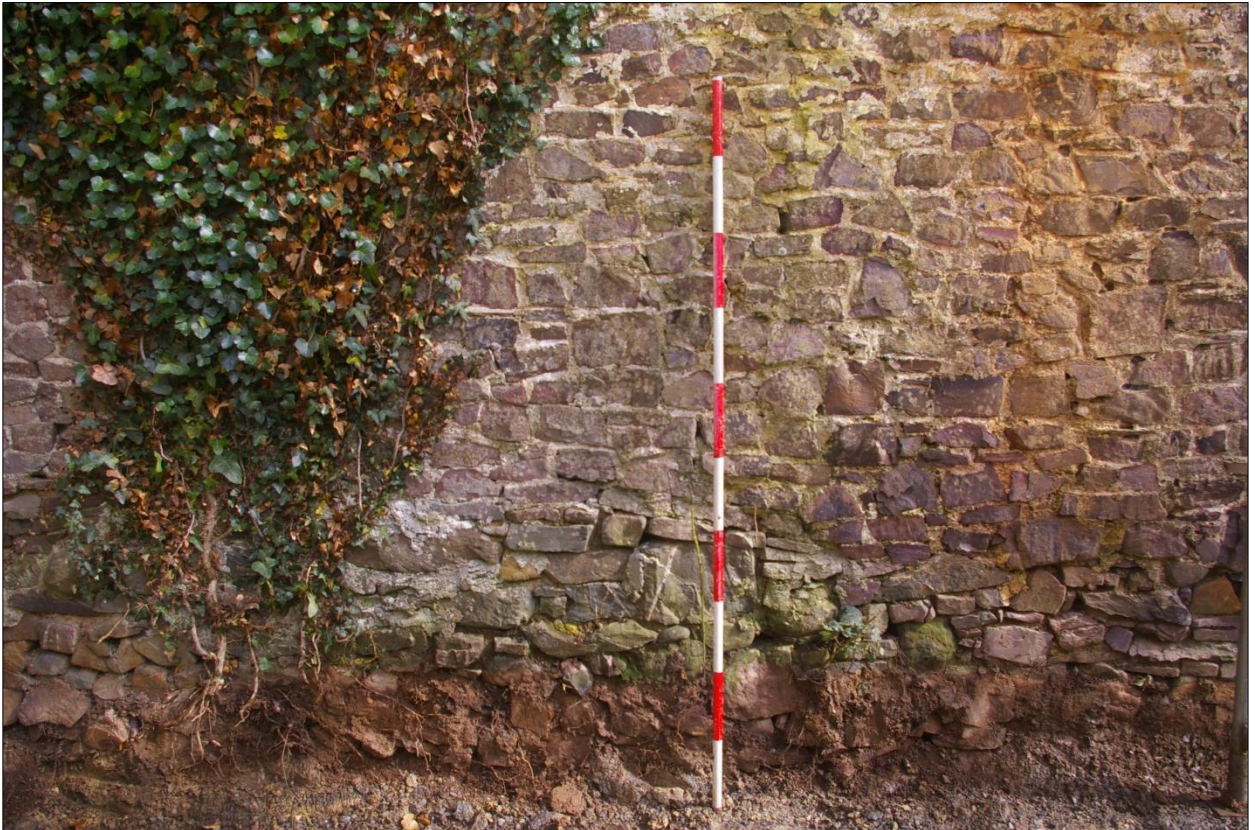
The south wall of Building 5, showing detail of the wall construction; viewed from the south.
