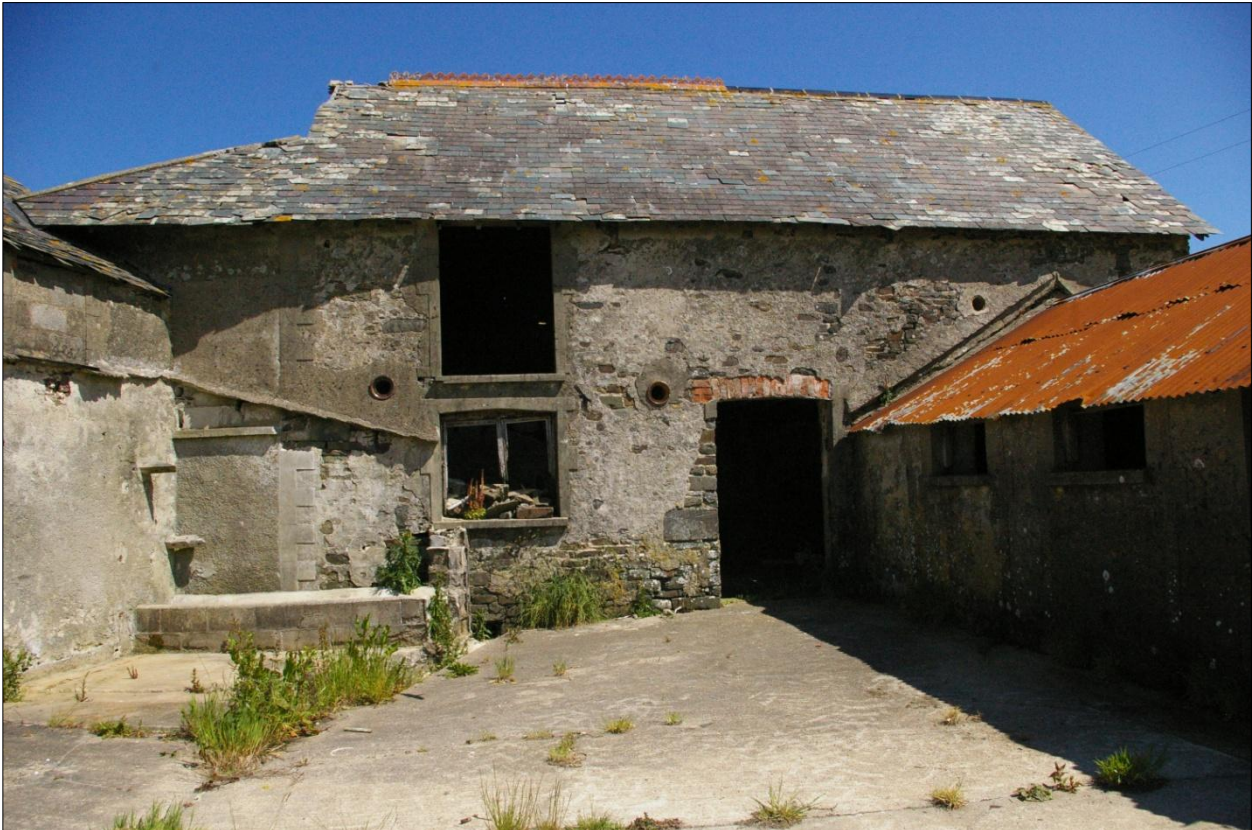
The south elevation of Building 1, within the yard; viewed from the south.
