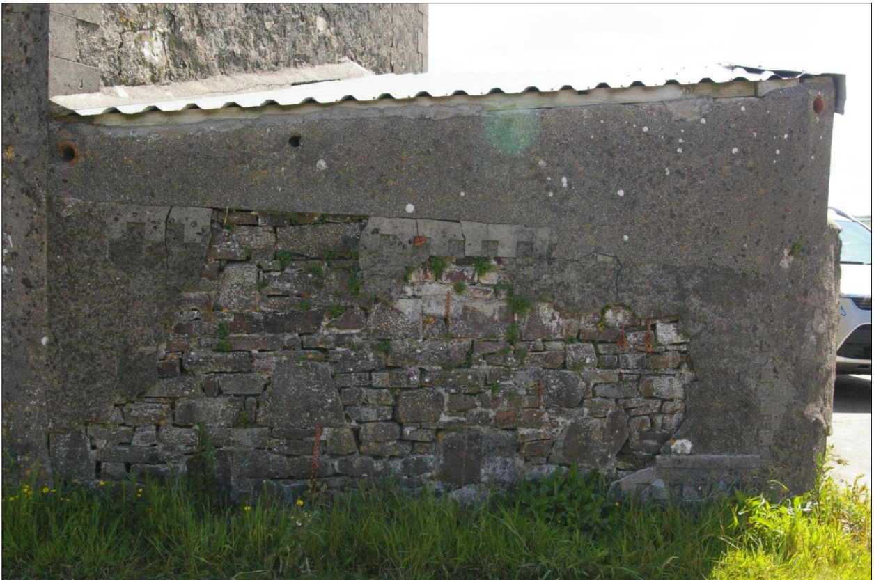
The west wall of Building 9, incorporating the west yard wall and north gatepost, in the south-west corner of the yard; viewed from the west.
