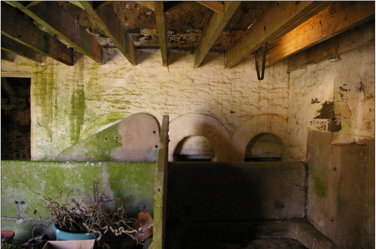
The north wall of Building 1, internal face, east end; viewed from the south.
