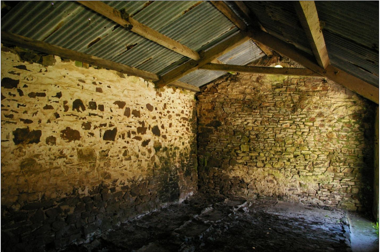
The south and east walls of Building 4, internal faces; viewed from the north-west.
