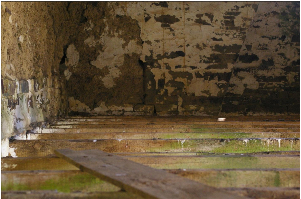
The east gable wall of Building 1, internal face, at first floor level, showing detail of the chamfered reveal/edge visible to the north of the chimney stack in the east wall of Building 1; viewed from the west.
