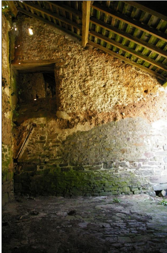
The east wall of Building 3, external face, from within Building 5; viewed from the north-west.
