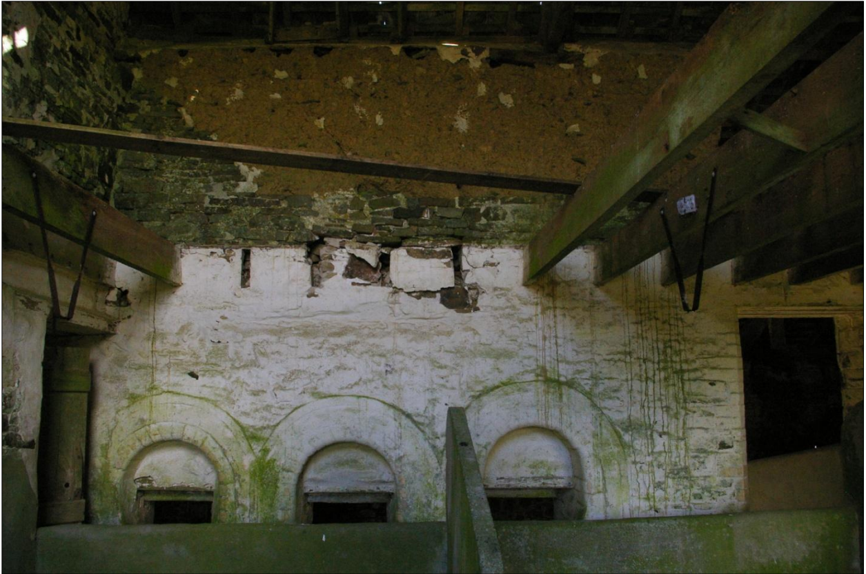
The north wall of Building 1, internal face, west end; viewed from the south.
