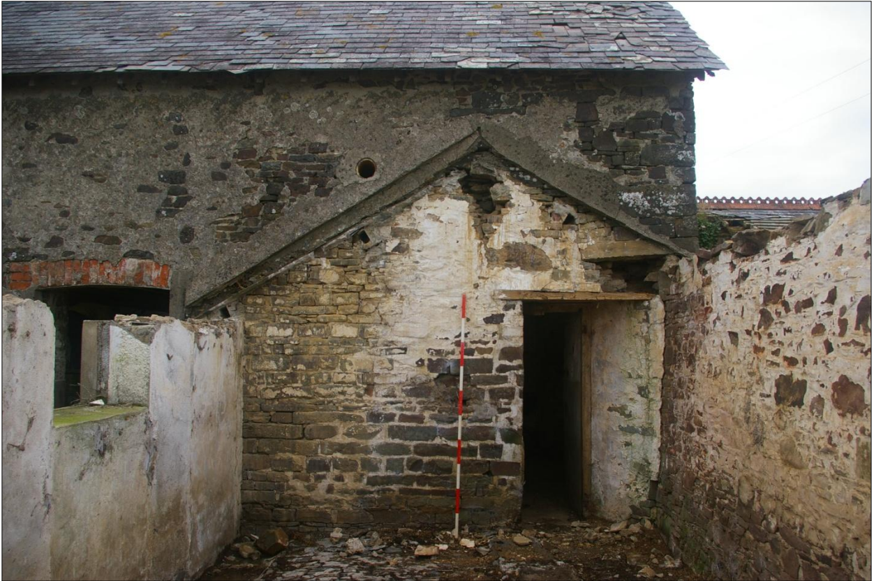
The north wall of Building 4, internal face, the external face of the south wall of Building 1; viewed from the south (2m scale).
