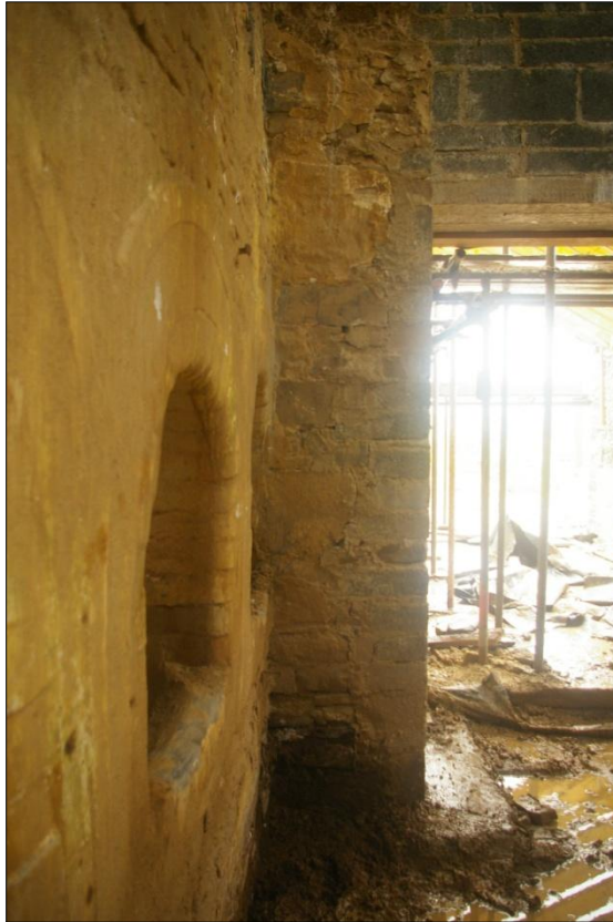
Detail of east wall of building B1, north end, Area #5; viewed from the west (no scale).
