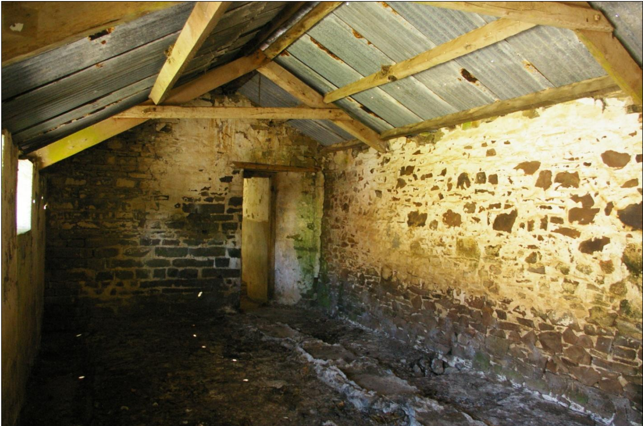
The north and east walls of Building 4, internal faces, showing the south wall of Building 1, external face from within Building 4; viewed from the south-west.
