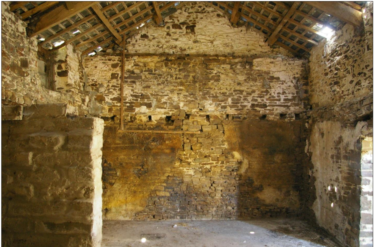
The south wall of Building 2, internal face, with blocked window at ground floor level; viewed from the north.
