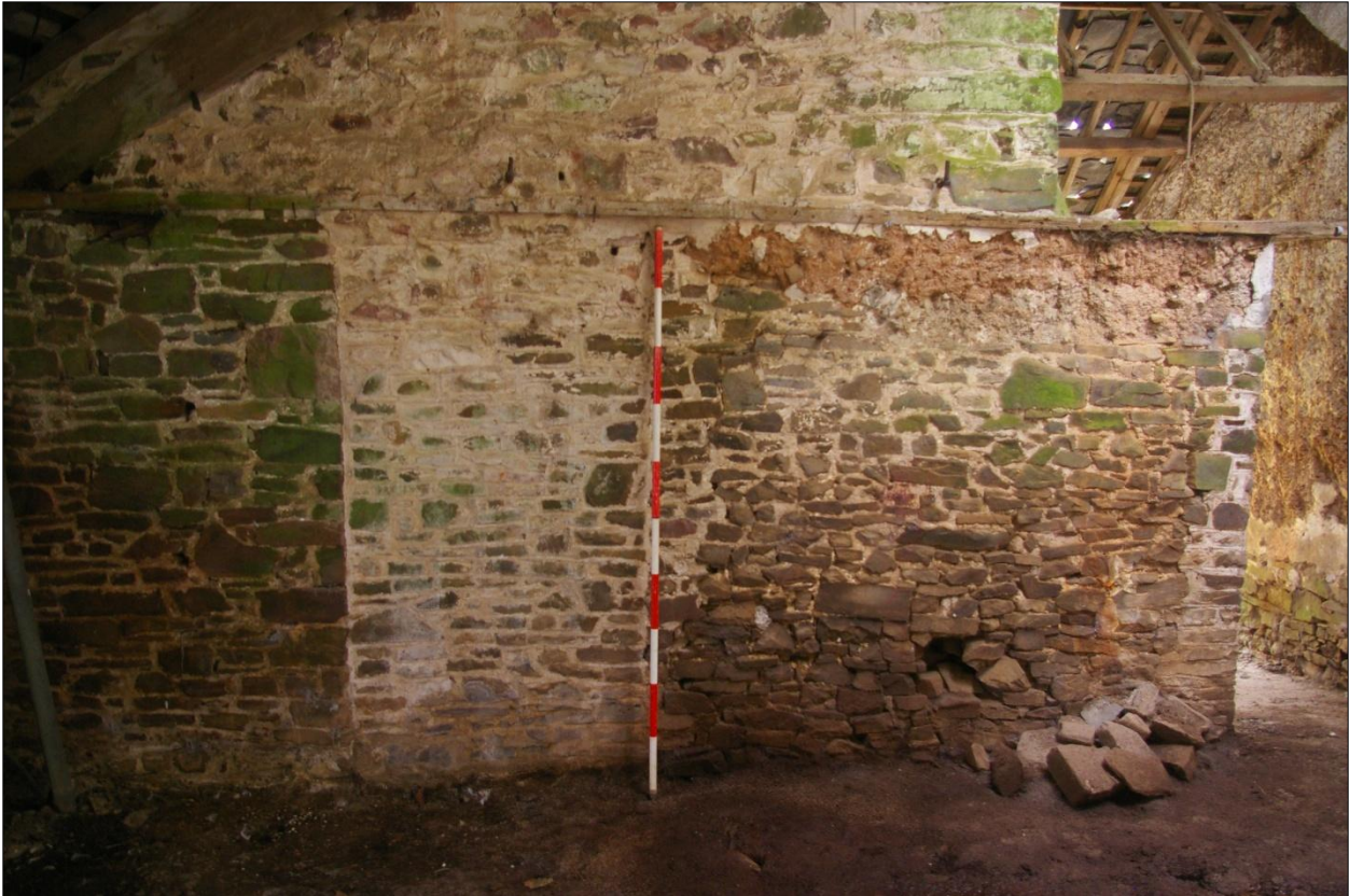
The south wall of Building 7, external face, from within Building 8, showing detail of the blocked doorway; viewed from the south (2m scale).
