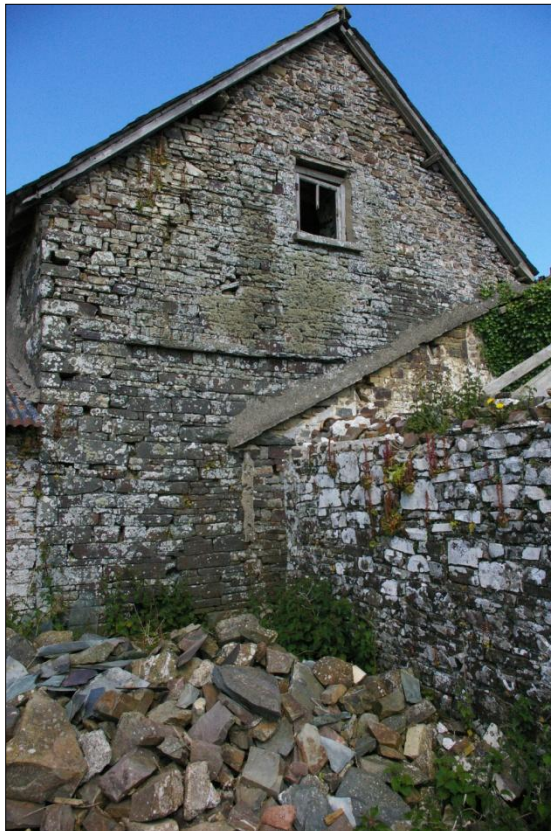
The east gable wall of Building 1, showing the drip-moulding to the south side of the wall; viewed from the south-east.
