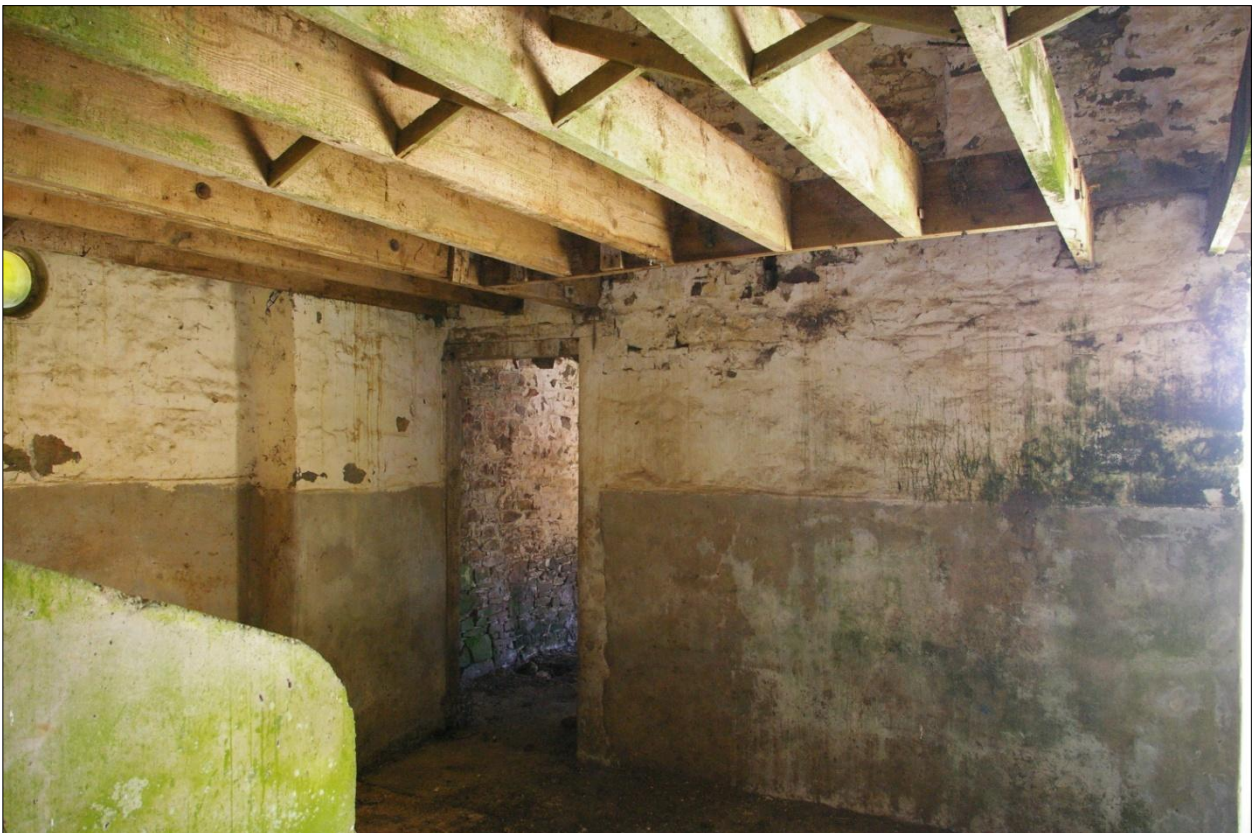
The south wall of Building 1, internal face, showing the forced opening doorway leading to Building 4, at the east end; viewed from the north-west.
