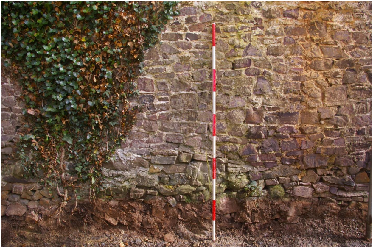
Detail of the footings to the south wall of B5, Area #2; viewed from the south (2m scale).
