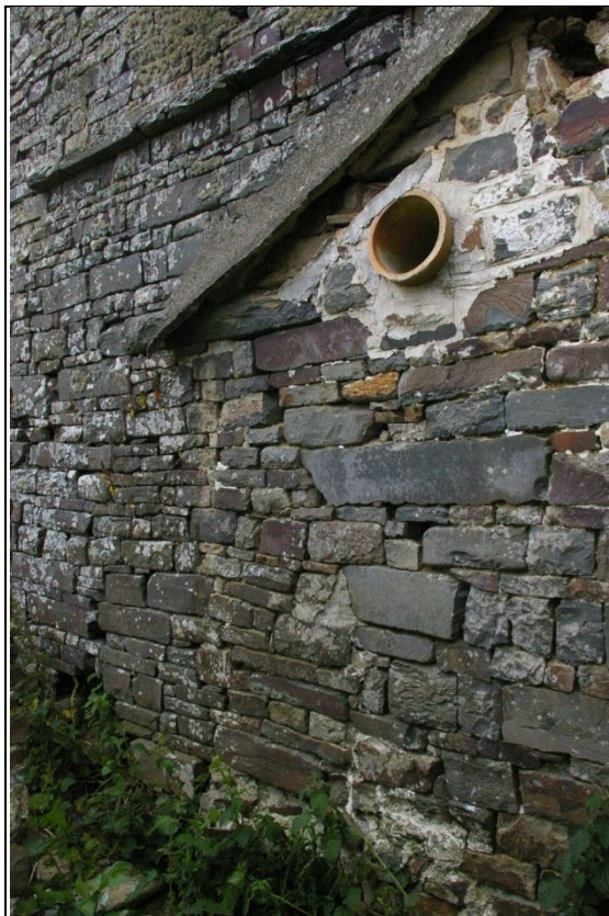
Figure 11: Detail of east wall of B1, showing the blocking of a former oven to the south of the chimney stack; viewed from the north-east.
