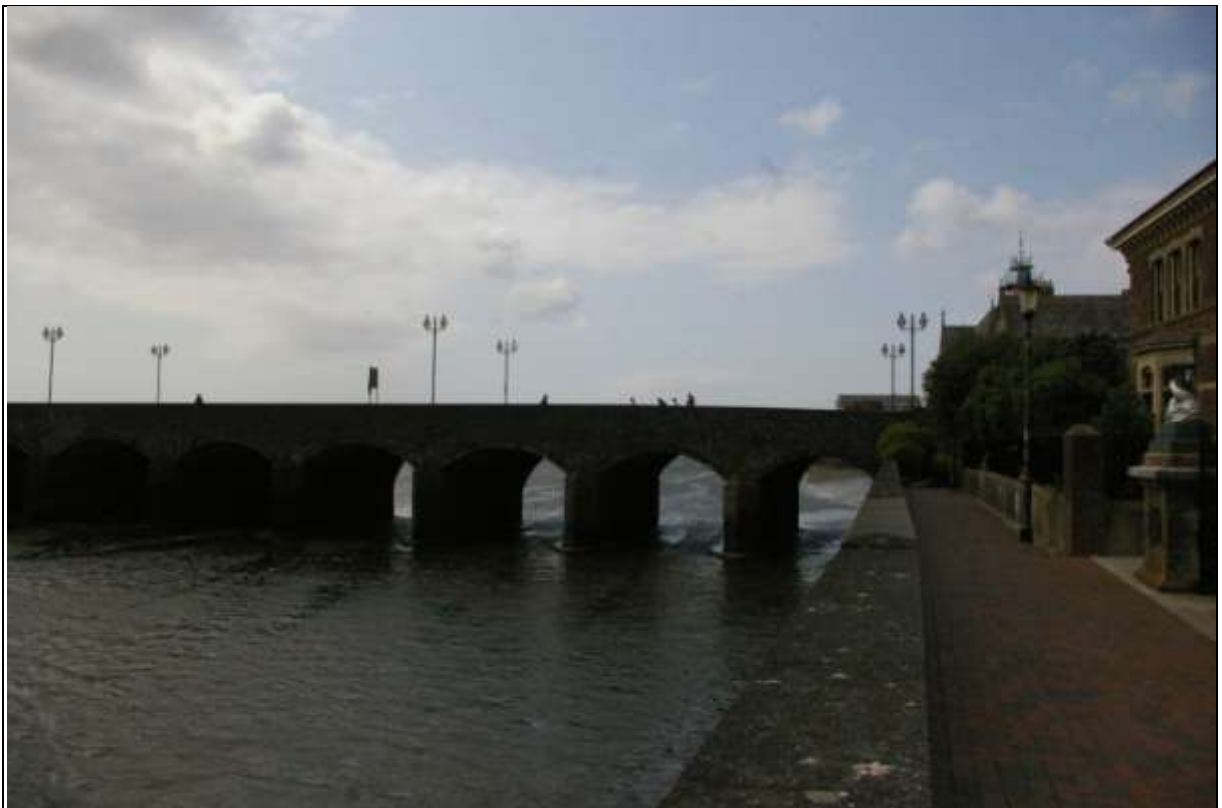
View of the Longbridge in Barnstaple, spanning the Taw River; from the east, south-east.
