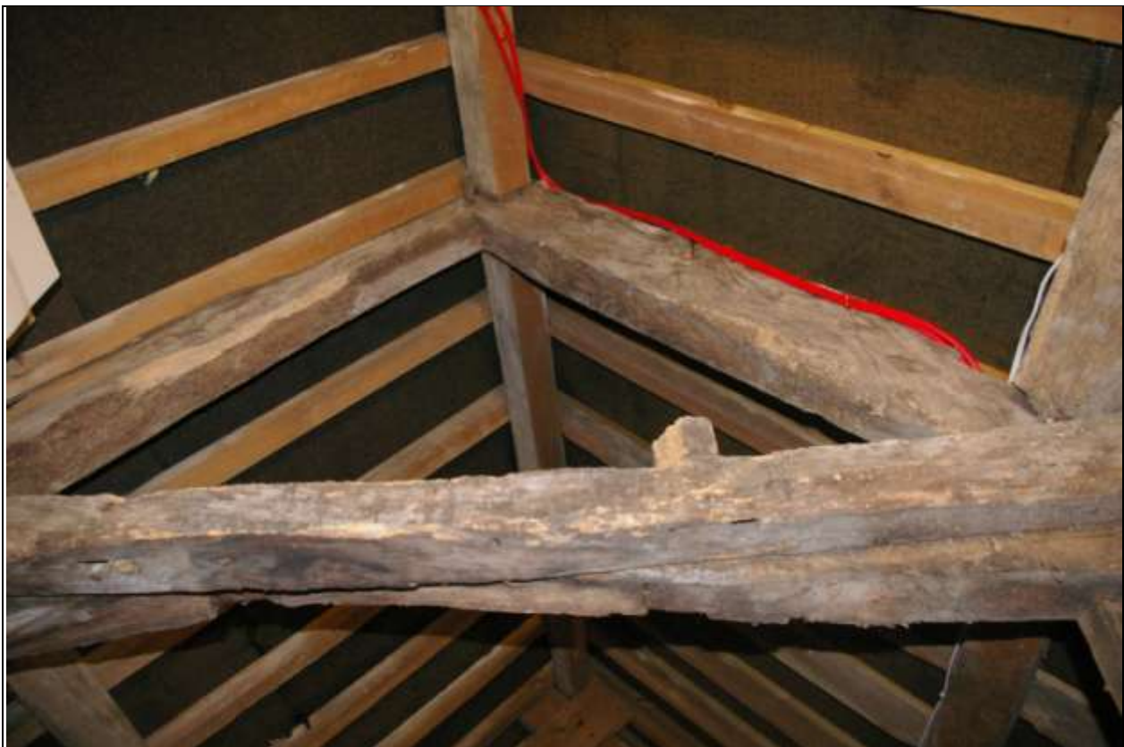
View of part of one of the surviving A-frame two-part truss blades pegged at the top. A collar with spiked joints is braced across the A-frame, with a later additional rough-cut and irregular beam for strength; the collar has sockets for a partition. One original large square-set purlin socketed into the south truss blade. Viewed from the west.
