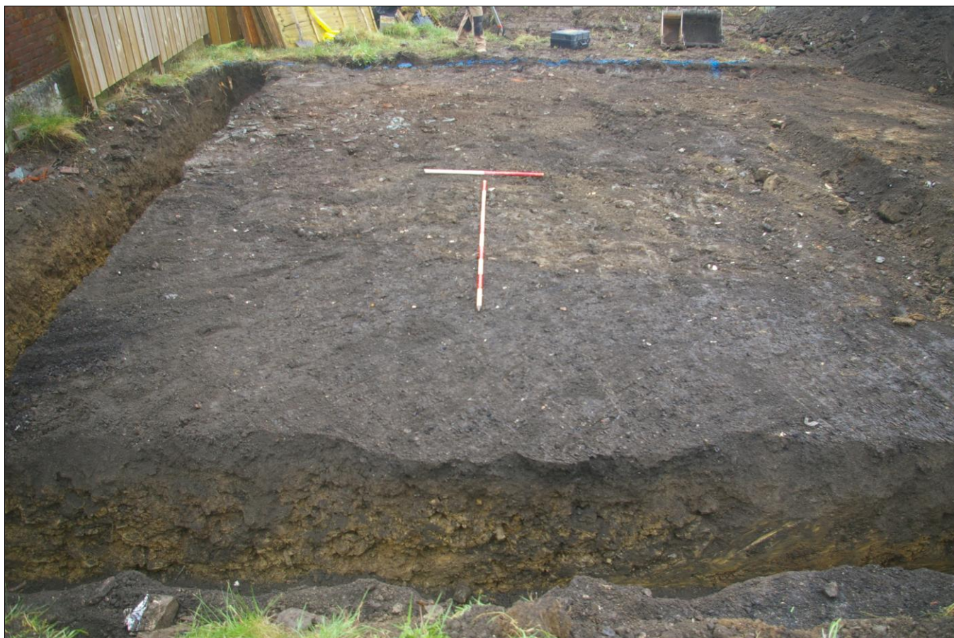
Figure 3: View of the site following secondary site strip; viewed from the west (1m and 2m scales).
