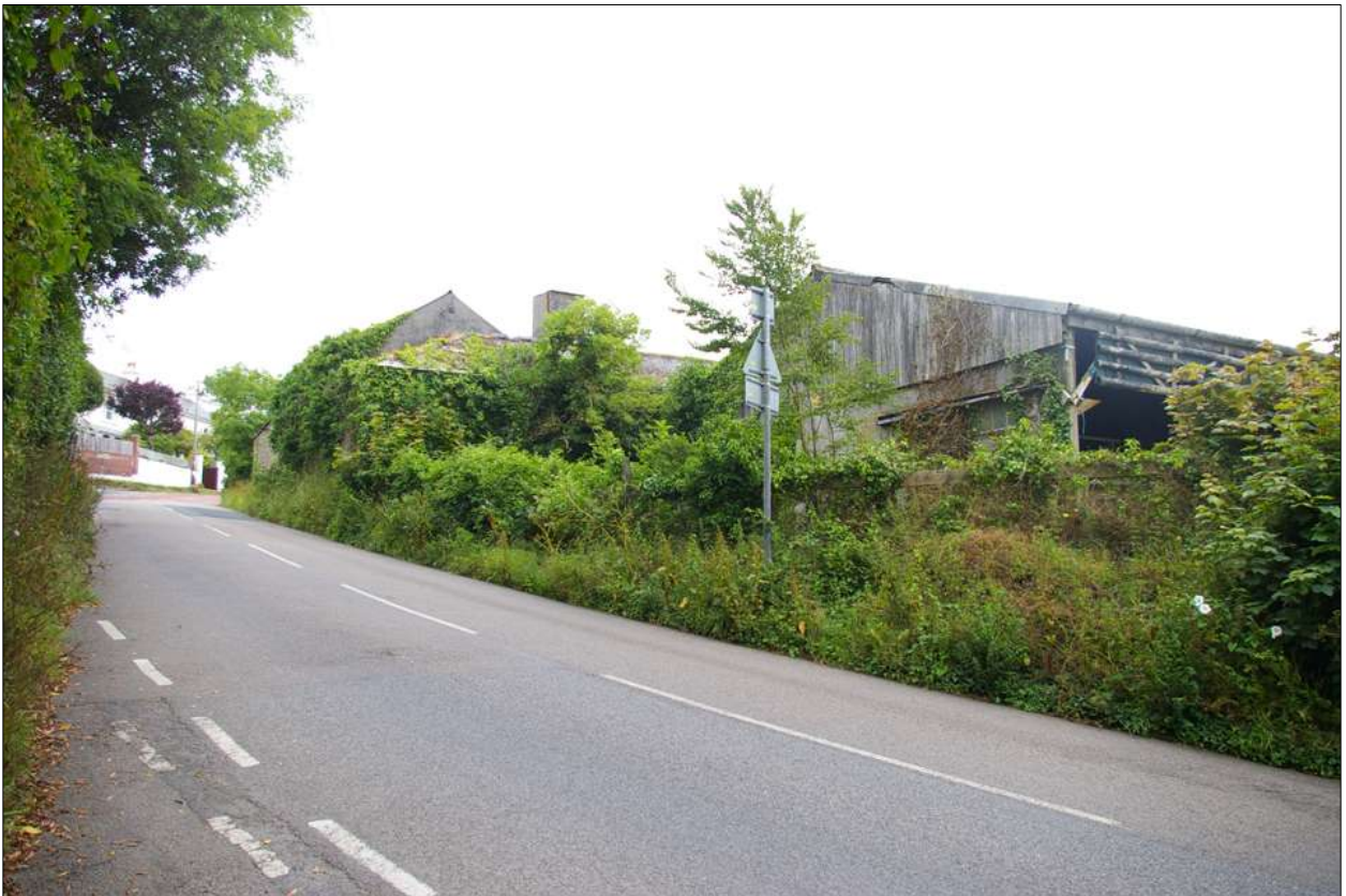
View to B2, B3 and B8 from Tregew Road; viewed from the south-west.
