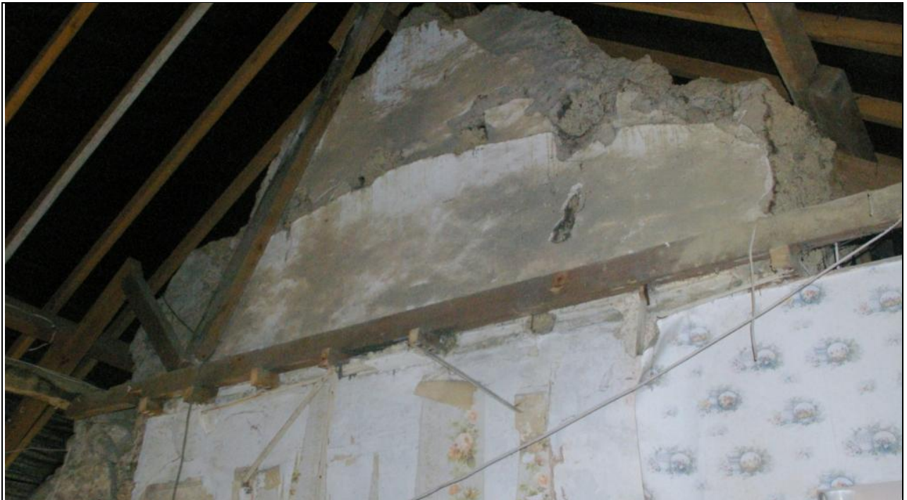
The scar from the former barrel vault in the upper north wall of the former open hall; from the south-east.
