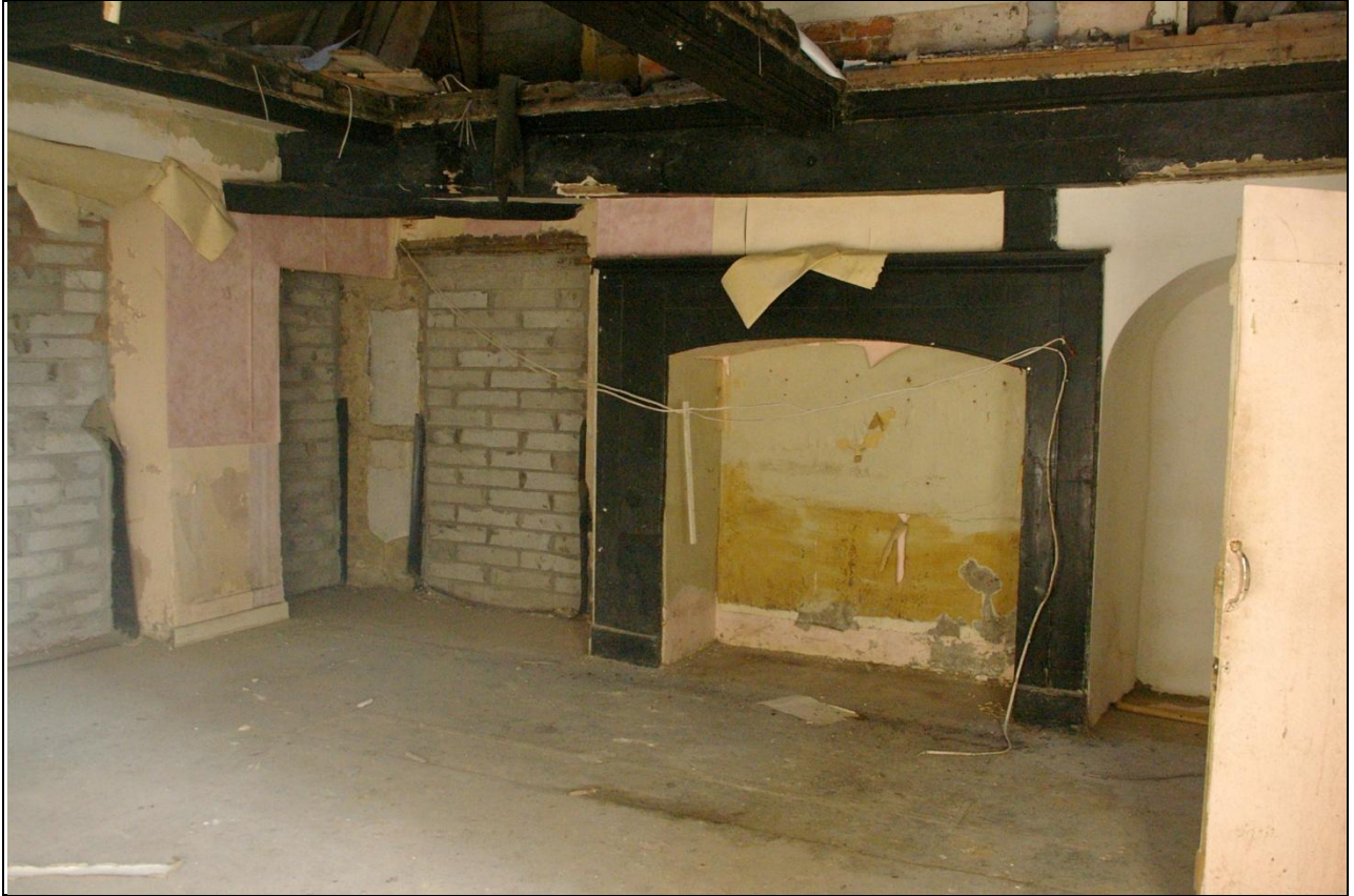
The 18 th century kitchen fireplace in the former open hall, on the ground floor, in the service range; from the north-west.
