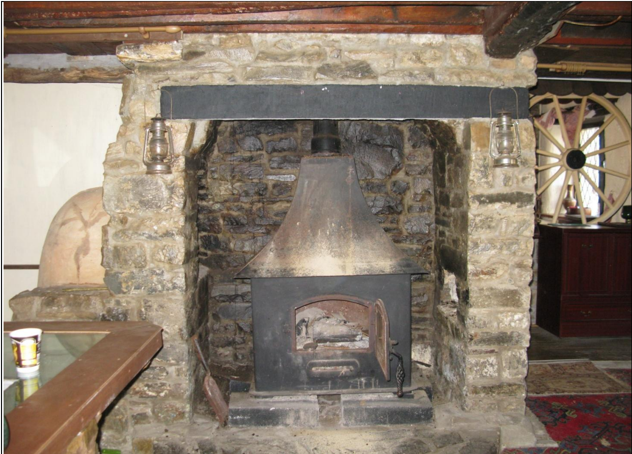
Fireplace in west gable end stack in the Farmers Arms, with replaced concrete lintel; from the east.
