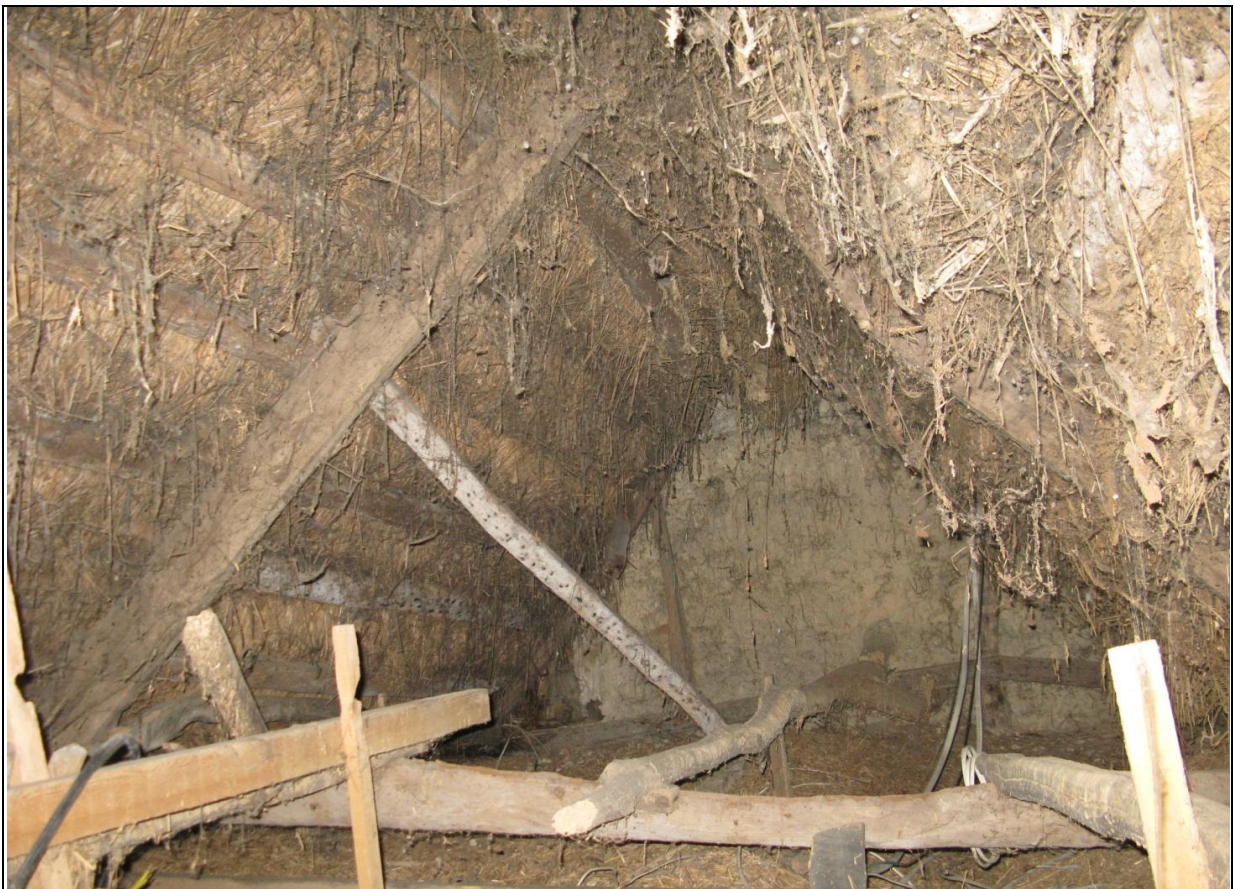
The thatch roof with A-frame trusses and multiple purlins; from the south-west.
