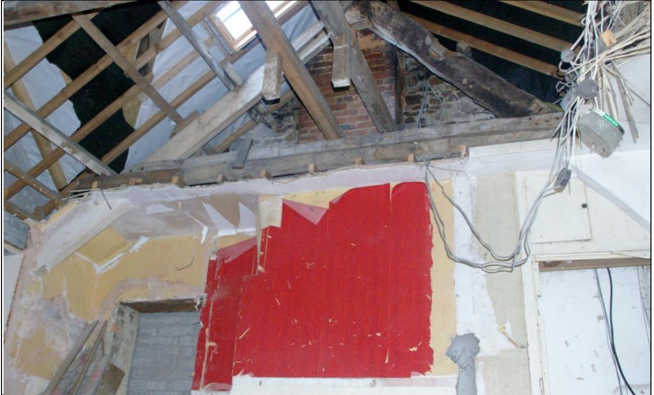
The historic trusses within the roof structure above the former open hall; from the north-west.
