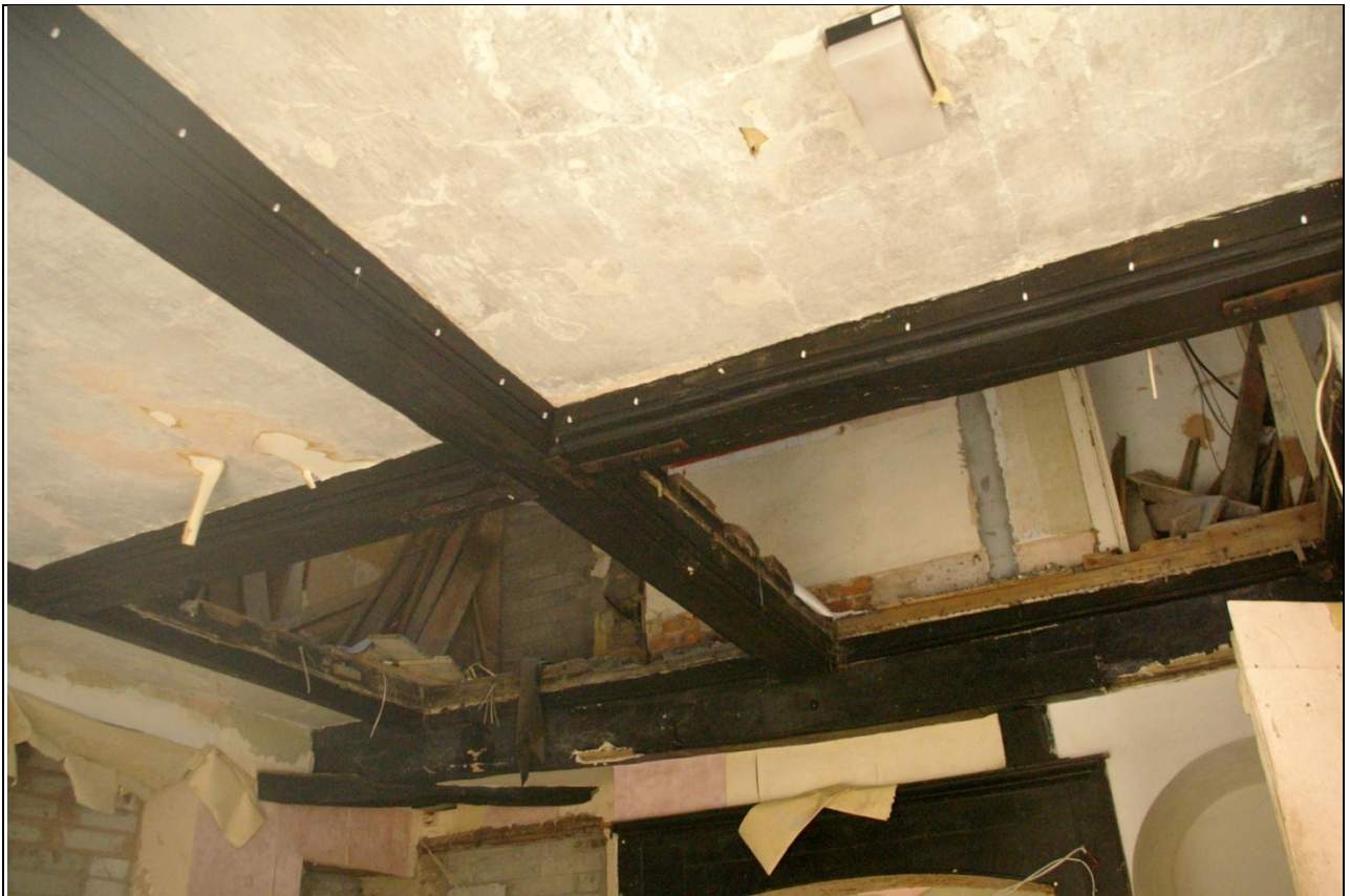
The cross beam roof, inserted into the open hall in the 17 th century; from the north-west.
