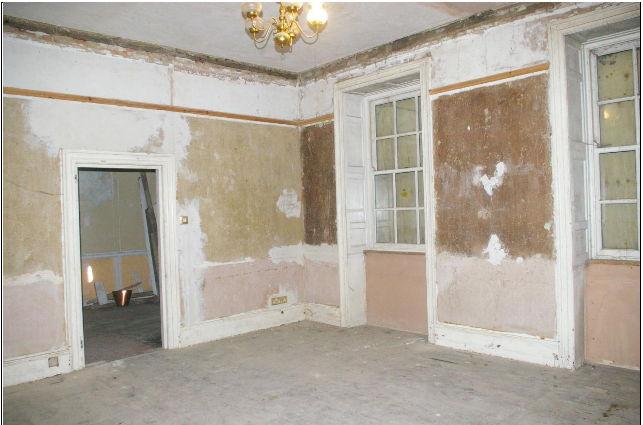
The dining room in the Manor House, showing panelled casements; from the north-west.
