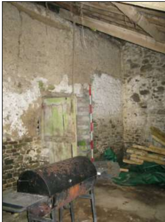
The southern end of the west wall of the barn (2m scale).
