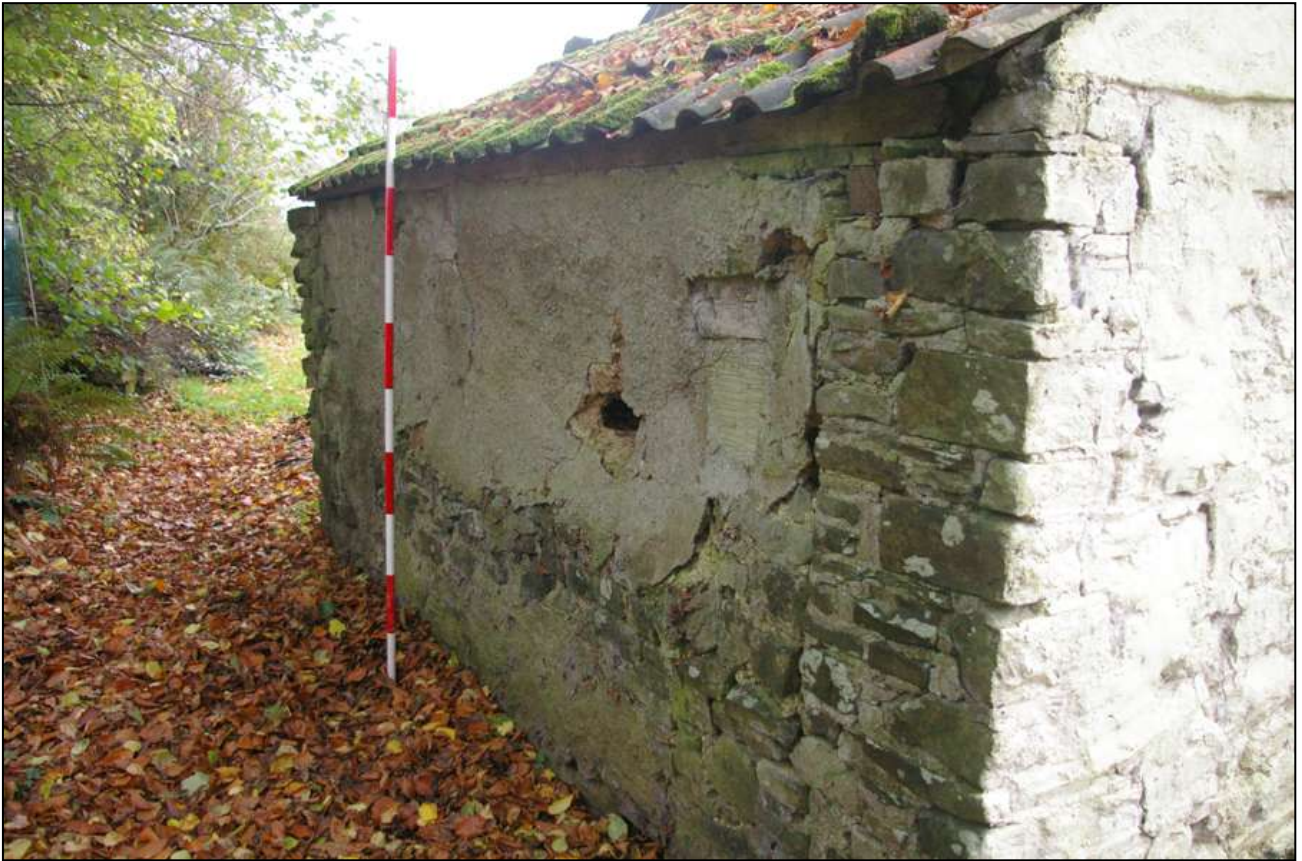
The south facing wall of the lean-to attached to the south end of the barn (2m scale).
