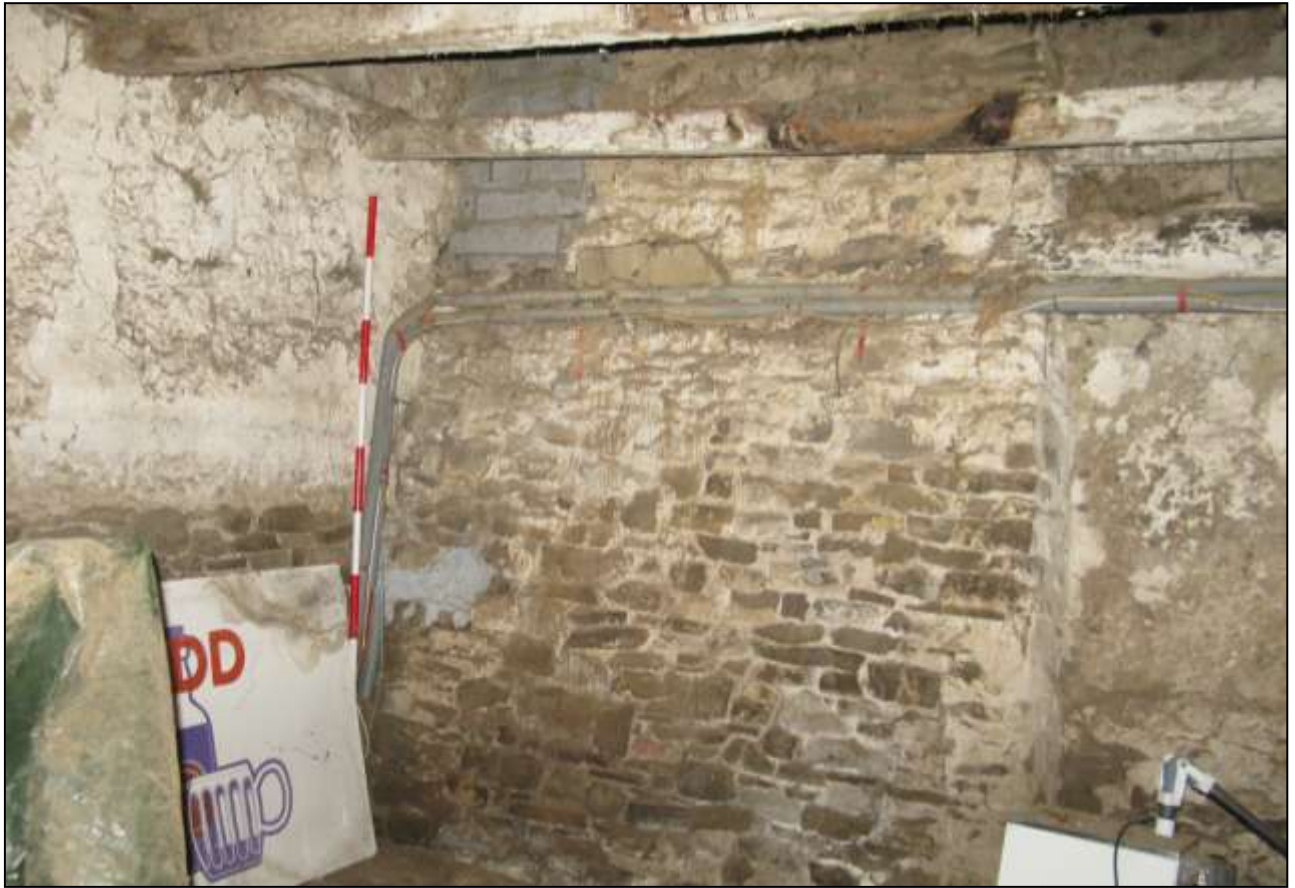
The west end of the north wall showing internal buttress (no scale).
