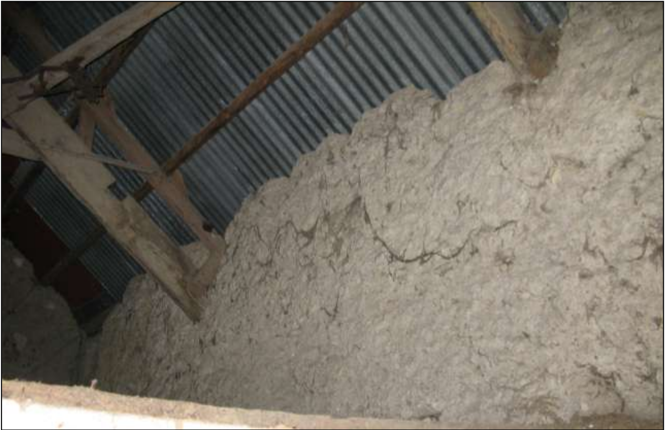
Top of east wall showing the feet of the roof trusses (no scale).
