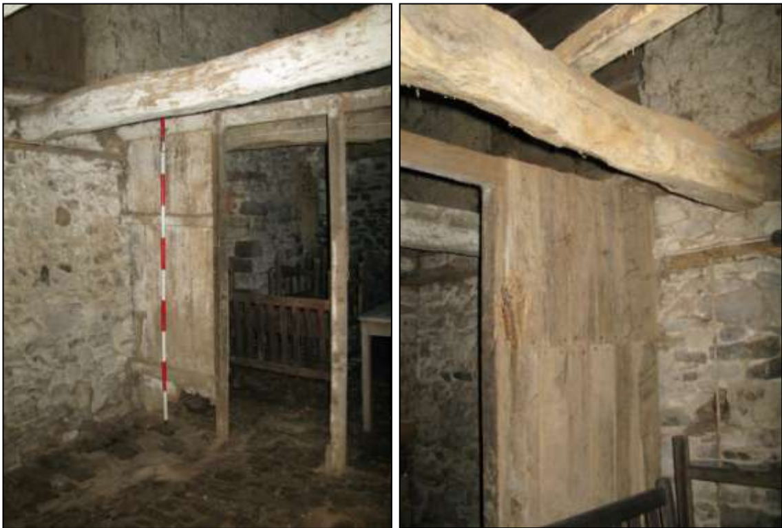
Left: The southern end of the east wall showing the doorway and remains of the partition (2m scale). Right: The rear of the partition (no scale).
