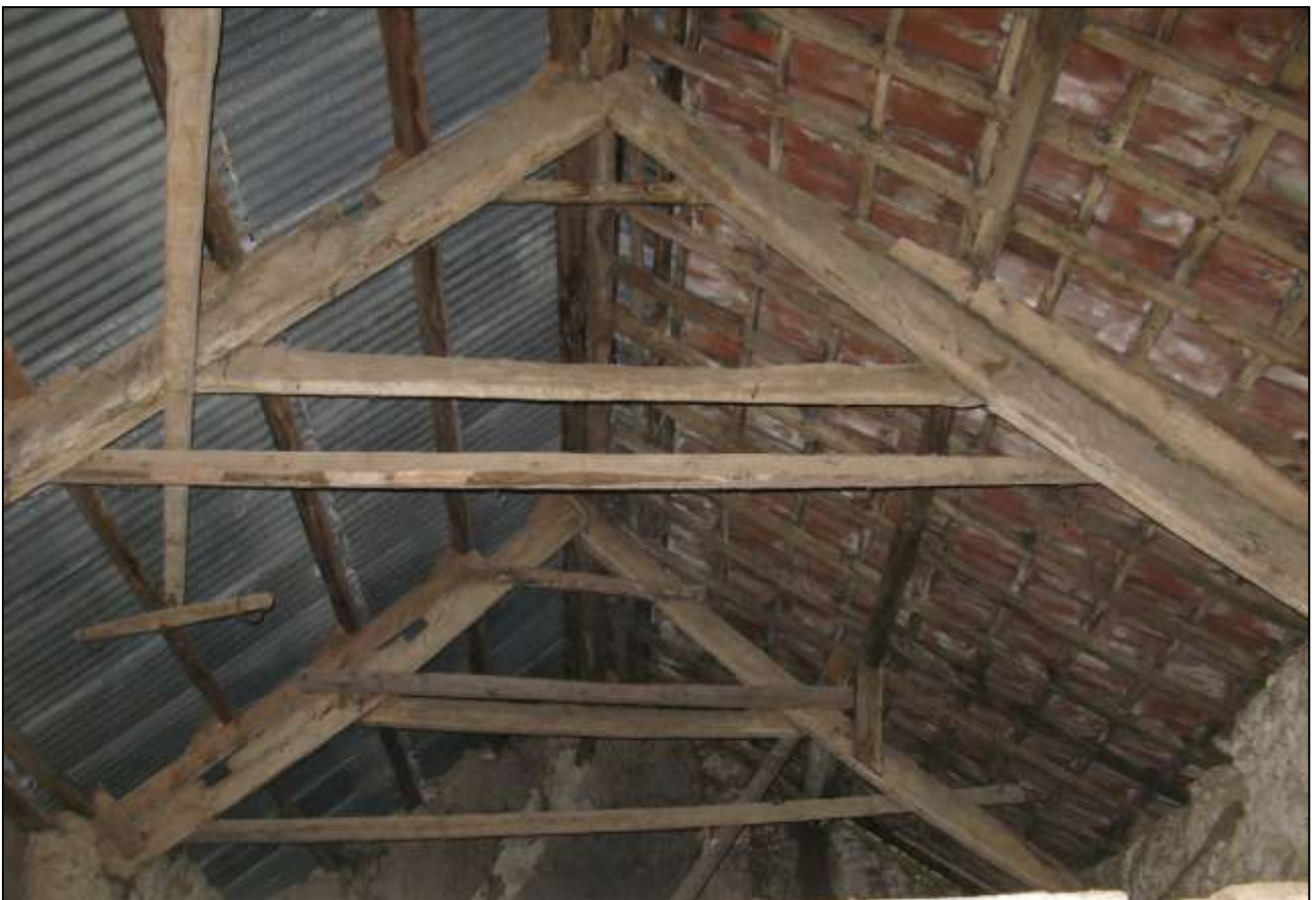
The roof trusses at the southern end of the building viewed from the north (no scale).
