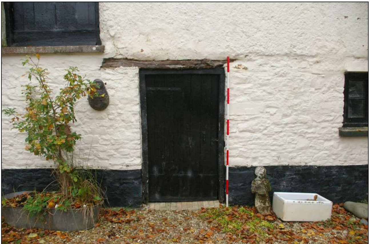
The doorway and window at the north end of the east facing elevation (2m scale).
