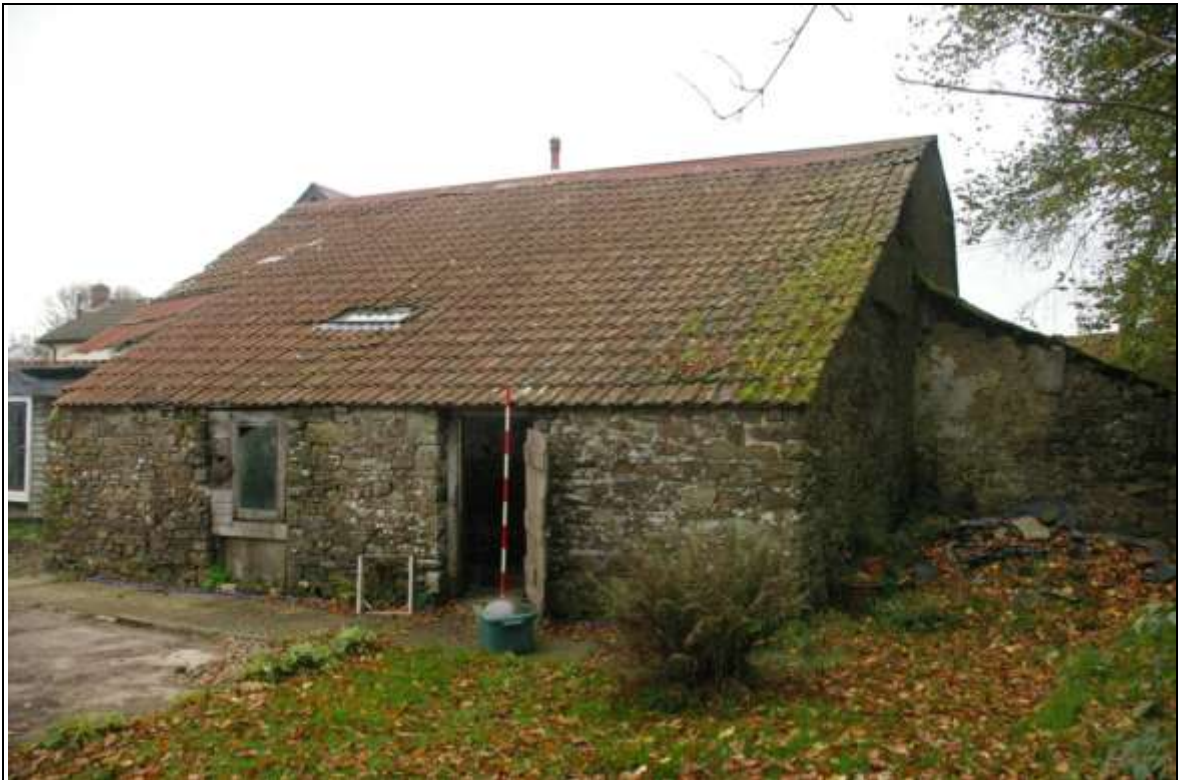
Figure 6: The west facing wall of the rear lean-to (Building 2) viewed from the south west (2m scale).
