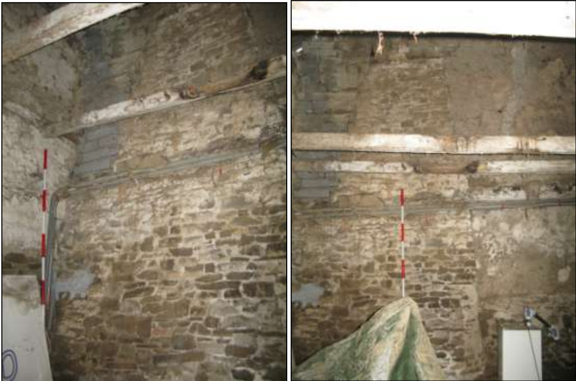
Left: the west end of the north wall showing internal buttress (2m scale). Right: Central part of the north wall (2m scale).
