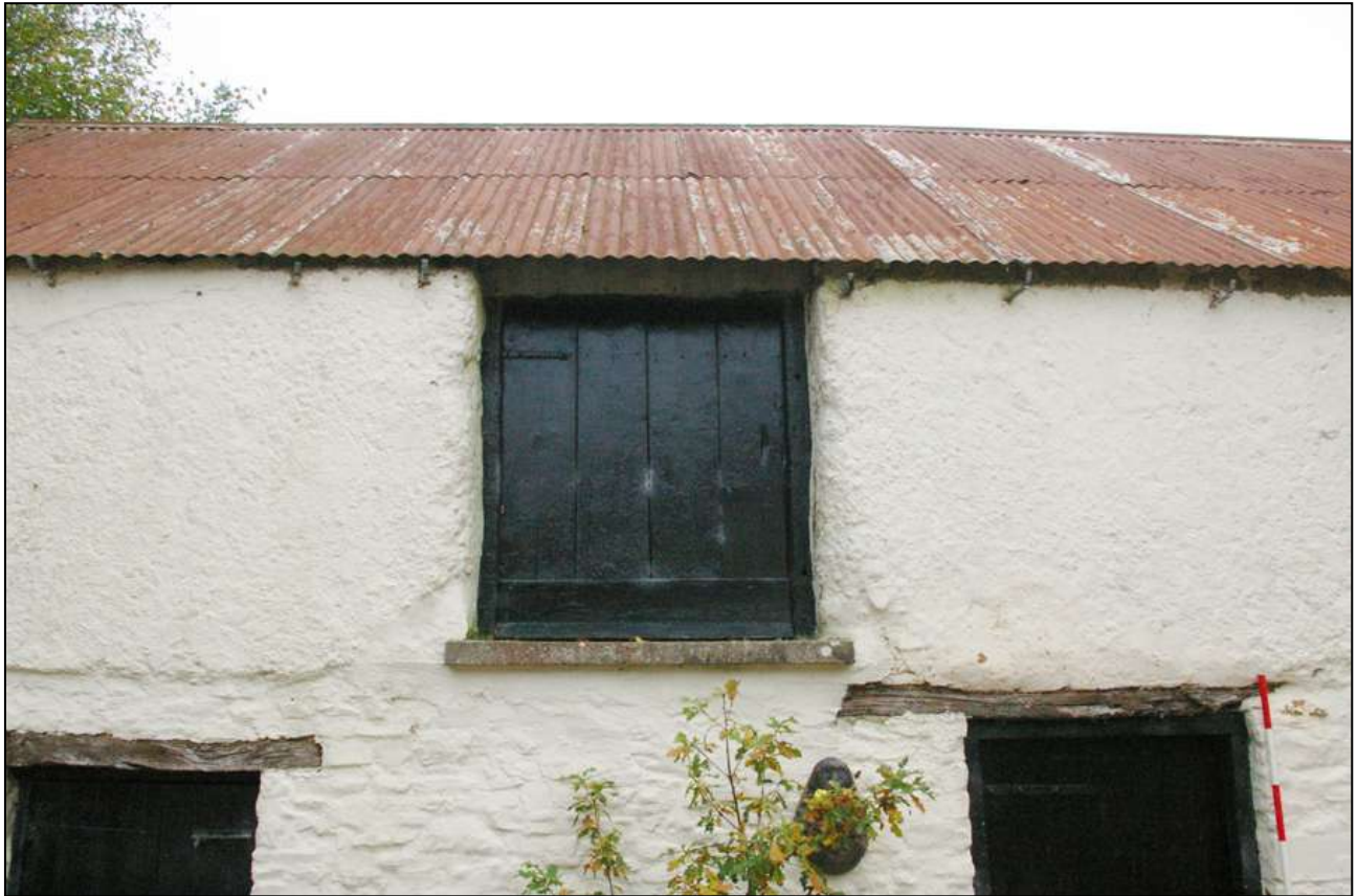
The first floor loading door in the east facing elevation (2m scale).
