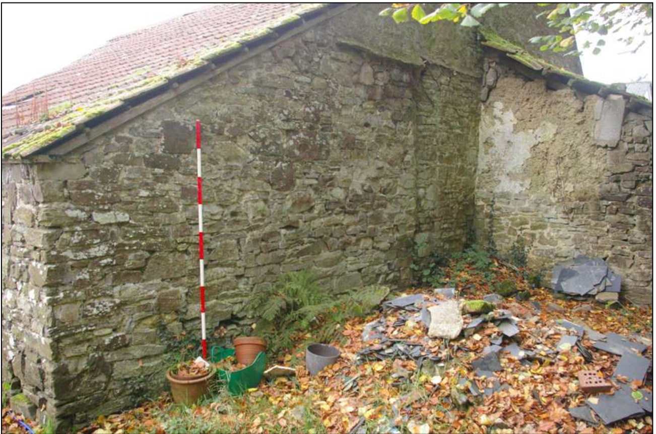
The south facing wall of the barn between the lean-tos (2m scale).
