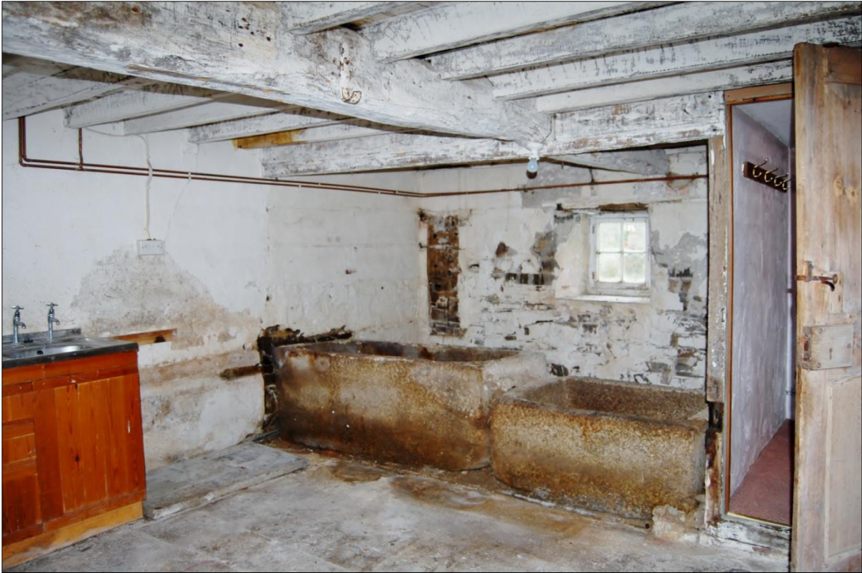
Figure 9: The dairy, including the stone salting troughs; from the north; taken during 2015 survey.
