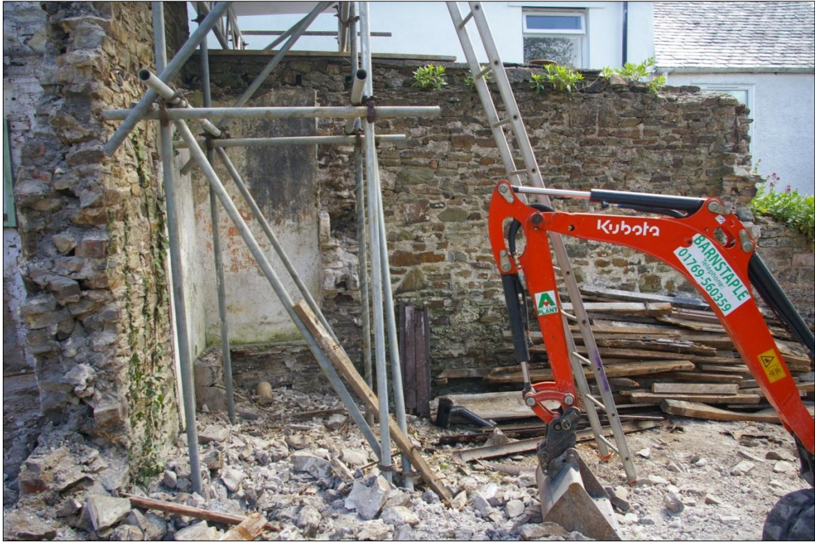
THE OUTSIDE TOILET BETWEEN THE BARN AND THE (NOW DEMOLISHED) OUTBUILDING; VIEWED FROM THE WEST (NO SCALE).
