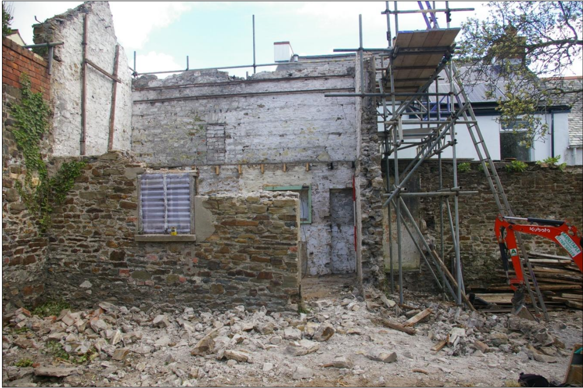
THE BARN STRUCTURE FOLLOWING PARTIAL DEMOLITION OF THE SOUTH AND WEST WALLS; VIEWED FROM THE WEST (2M SCALE).
