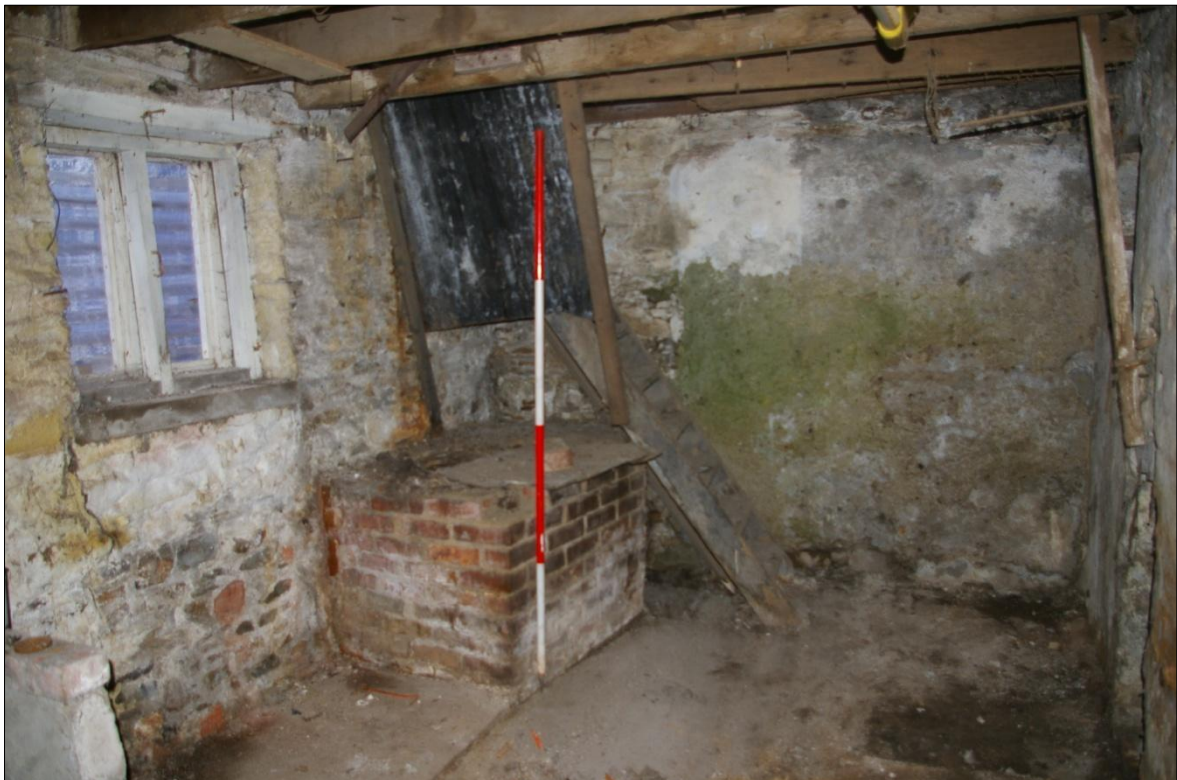
THE BRICK BUILT COPPER IN THE NORTH-WEST CORNER OF THE BARN, WITH WOODEN STAIRS RISING TO THE LOFT ABOVE; VIEWED FROM THE SOUTH-EAST (2M SCALE).
