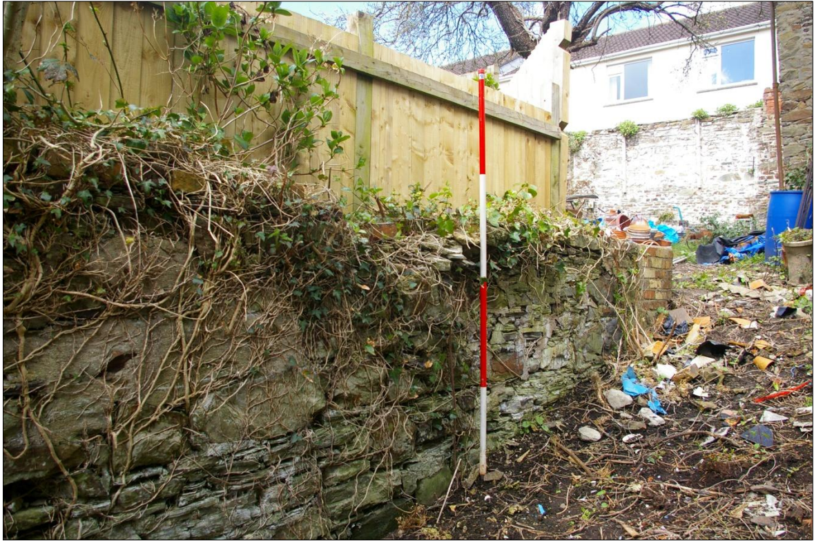
THE LARGE SLATE-STONE WALL TO THE SOUTH-WEST OF THE DEVELOPMENT SITE, FORMING A RETAINING WALL TO THE LEVEL LAWN AREA; VIEWED FROM THE SOUTH-EAST (2M SCALE).
