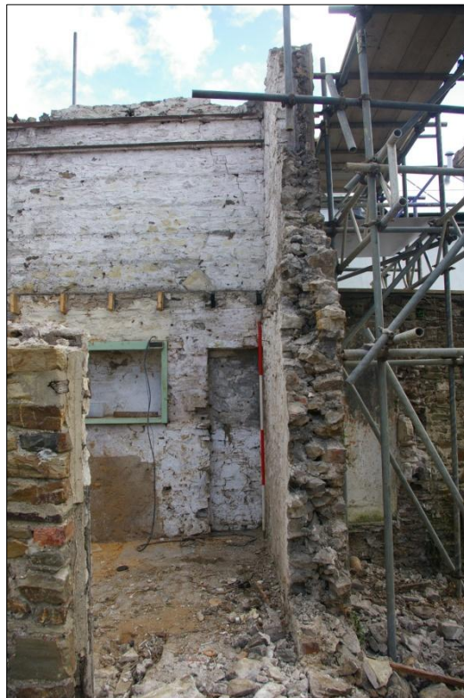
DETAIL OF THE PHASING OF THE BARN STRUCTURE, SHOWING THE SOUTH WALL OBSTRUCTING THE EARLIER BLOCKED DOORWAY IN THE EAST WALL; VIEWED FROM THE WEST (2M SCALE).
