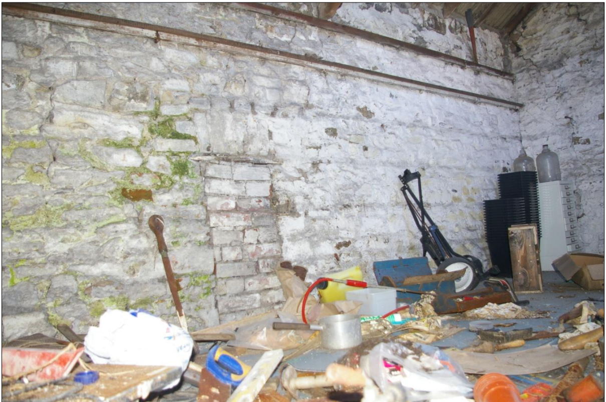
FIGURE 13: DETAIL SHOWING THE FIREPLACE IN THE EAST WALL OF THE LOFT SPACE; VIEWED FROM THE NORTH-WEST (NO SCALE).
