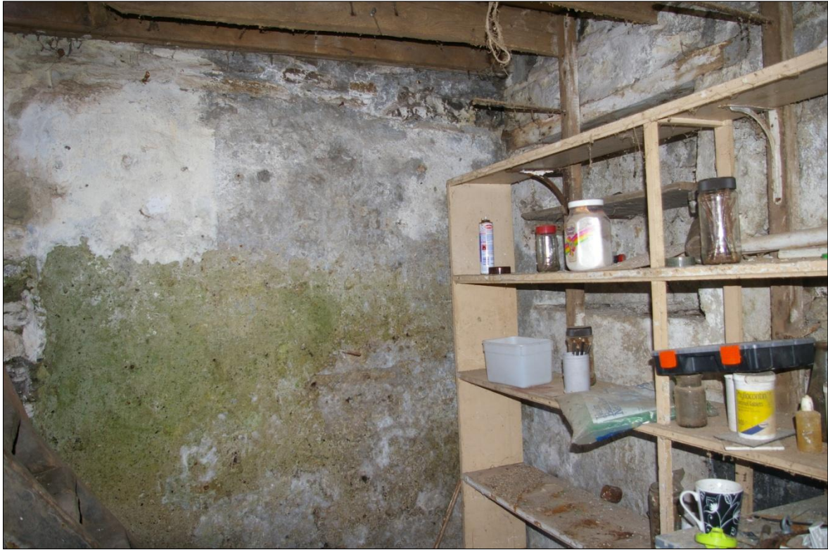
THE INTERNAL FACE OF THE NORTH WALL OF THE BARN, SHOWING THE SURVIVING LIME PLASTER WITH WHITEWASH; VIEWED FROM THE SOUTH-WEST (NO SCALE).
