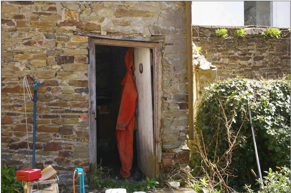
DETAIL OF THE WEST ELEVATION OF THE BARN, SHOWING THE DOORWAY IN THE SOUTH-WEST CORNER; VIEWED FROM THE WEST (NO SCALE).
