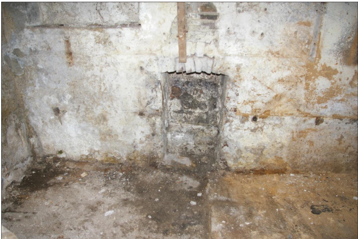
DETAIL OF THE INTERNAL FACE OF THE EAST WALL OF THE BARN, SHOWING THE SMALL FIREPLACE WITH STONE DRESSED JAMBS TO THE SIDE, AND SMALL HANDMADE BRICK SEGMENTAL ARCH, FOLLOWING REMOVAL OF BLOCKING; VIEWED FROM THE WEST (NO SCALE).
