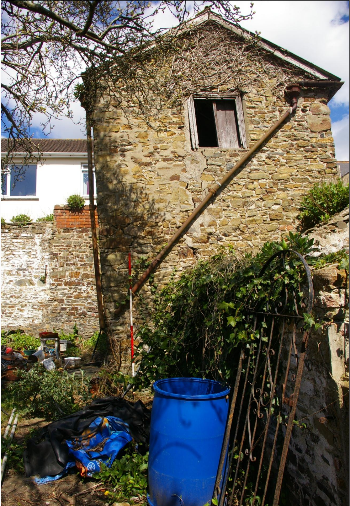
FIGURE 11: SOUTH ELEVATION OF THE MAIN OUTBUILDING, SHOWING THE WOODEN FRAMED WINDOW AND STRUCTURAL CRACK TO THE WEST; VIEWED FROM THE SOUTH (2M SCALE).
