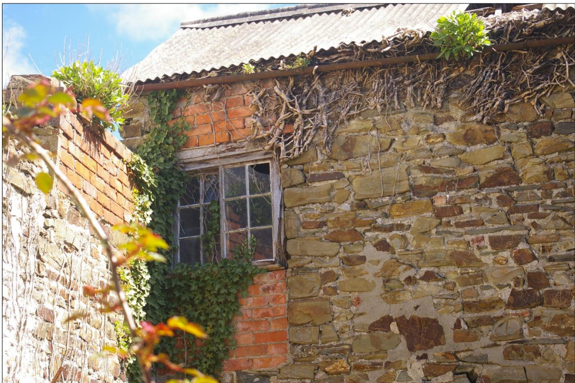
DETAIL OF THE WEST ELEVATION OF THE BARN, SHOWING THE SLIDING 'YORKSHIRE' SASH SET INTO THE BLOCKED LOADING DOOR; VIEWED FROM THE WEST-SOUTH-WEST (NO SCALE).
