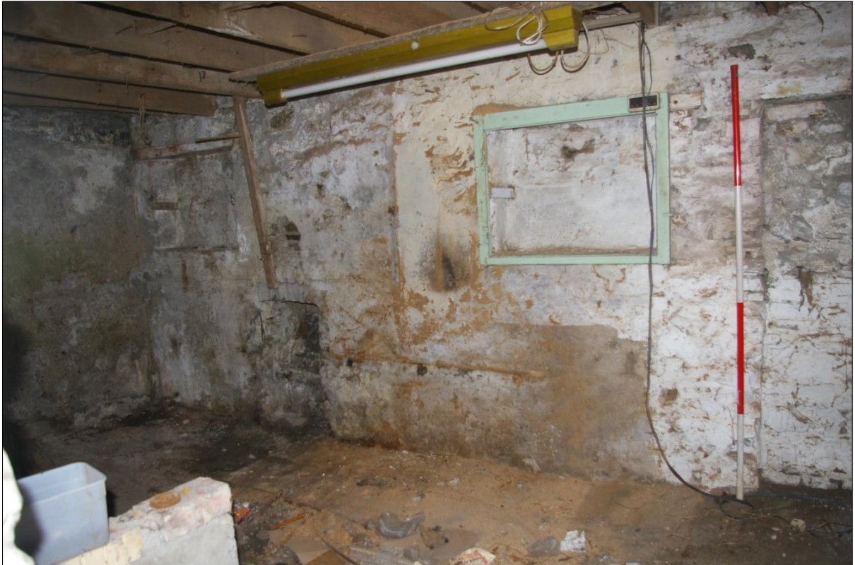
FIGURE 12: DETAIL OF THE INTERIOR ELEVATION OF THE EAST WALL, SHOWING THE BLOCKED DOORWAY, BLOCKED WINDOWS AND FIREPLACE; VIEWED FROM THE SOUTH-WEST (2M SCALE).
