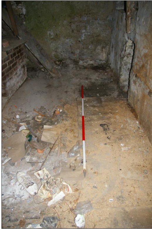
DETAIL OF THE CENTRAL REPAIRED SECTION OF CONCRETE FLOOR, WITH THE EARLIER LIME-CRETE REPAIR TO THE NORTH; VIEWED FROM THE SOUTH (2M SCALE).
