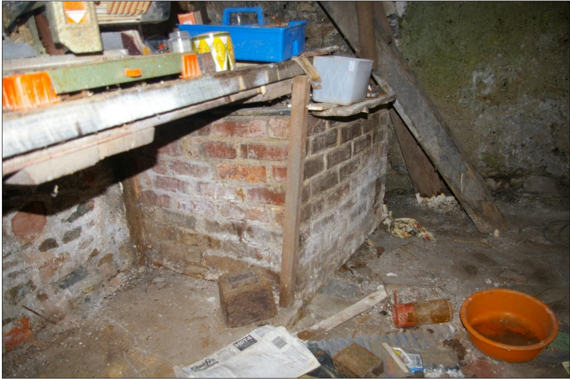
DETAIL OF THE BRICK BUILT COPPER IN THE NORTH-WEST CORNER OF THE BARN; VIEWED FROM THE SOUTH-EAST (NO SCALE).
