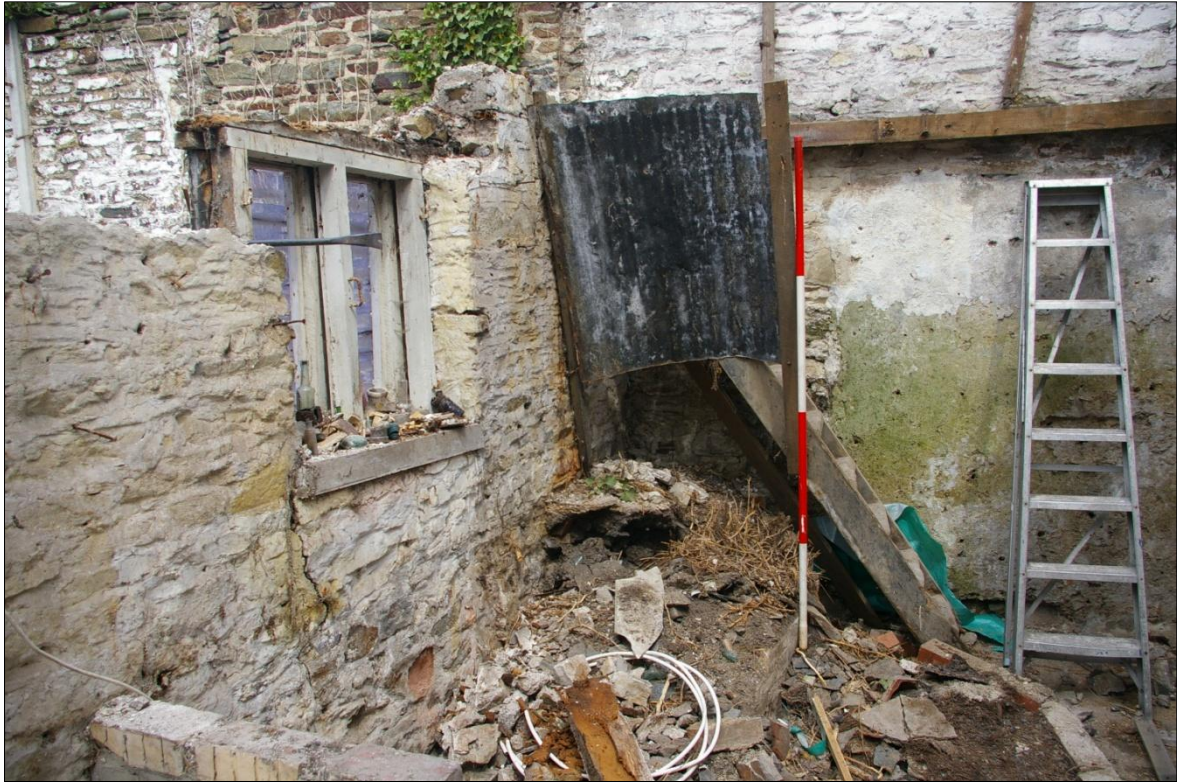
DETAIL FOLLOWING THE REMOVAL OF THE BRICK COPPER, SHOWING ITS EXTENSIVE BACK-FILLING WITH 19 TH CENTURY RUBBISH; VIEWED FROM THE SOUTH (2M SCALE).
