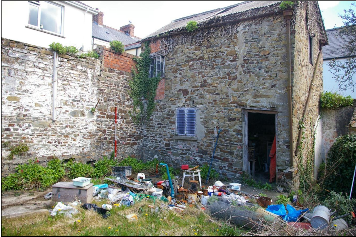
THE WEST ELEVATION OF THE BARN AND ADJACENT NORTH PLOT WALL; VIEWED FROM THE SOUTH-WEST (2M SCALE).
