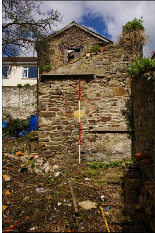
SOUTH ELEVATION OF THE OUTBUILDING, SHOWING DETAIL OF REMAINS OF A POSSIBLE TEMPORARY STRUCTURE; VIEWED FROM THE SOUTH (2M SCALE).
