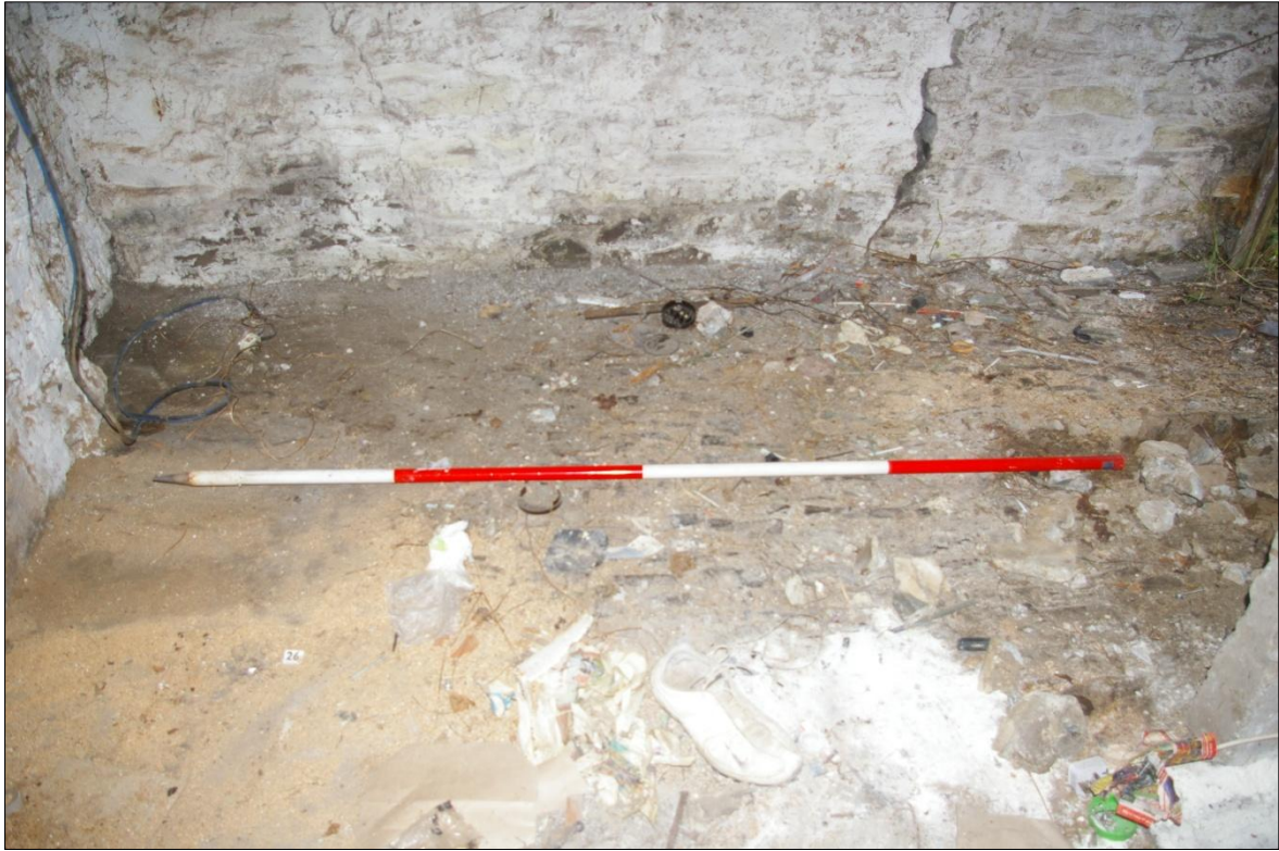
DETAIL OF THE COBBLE FLOOR WITHIN THE BARN BETWEEN THE BLOCKED AND CURRENT DOORWAYS; VIEWED FROM THE NORTH (2M SCALE).
