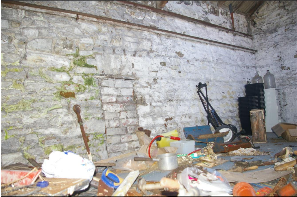
DETAIL OF THE INTERNAL FACE OF THE EAST WALL OF THE BARN, SHOWING THE BLOCKED FIREPLACE; VIEWED FROM THE NORTH-WEST (NO SCALE).
