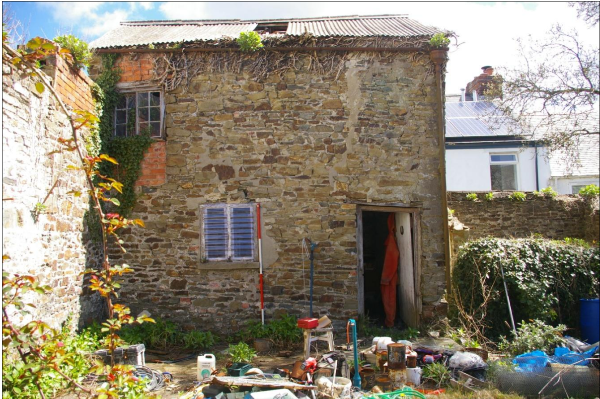
FIGURE 10: WEST ELEVATION OF THE MAIN OUTBUILDING SHOWING THE STRUCTURAL CRACK TO THE SOUTH, AND BLOCKED LOADING DOOR TO THE NORTH; VIEWED FROM THE WEST (2M SCALE).
