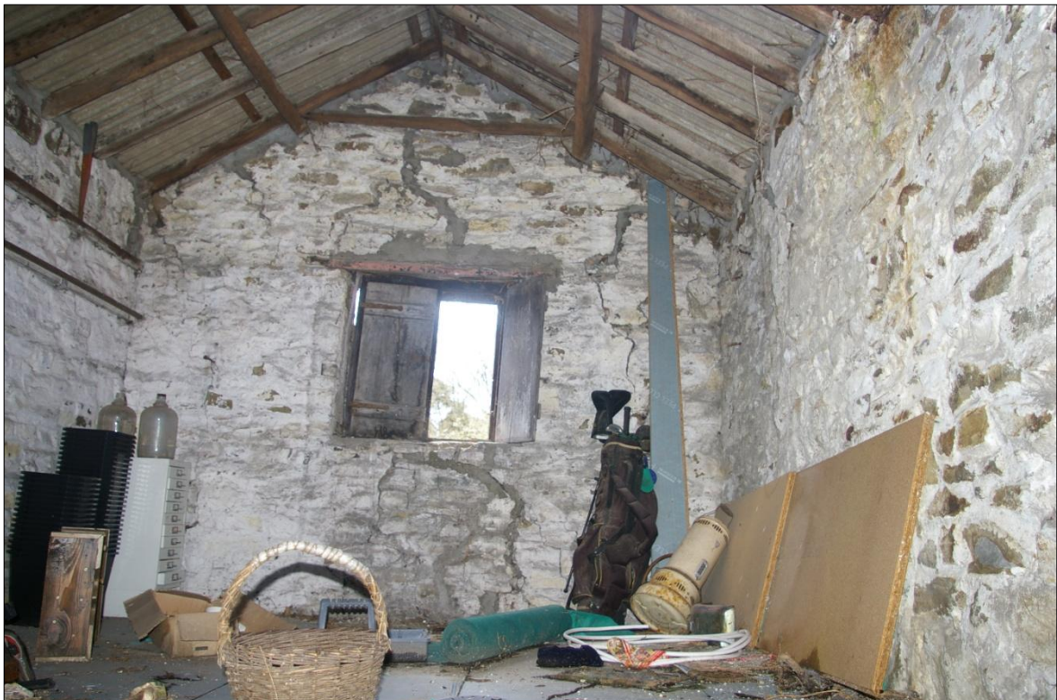
THE LOFT SPACE WITHIN THE BARN, SHOWING THE SURVIVING TIMBER WINDOW WITH PLANK SHUTTERS AND THE WHITEWASHED WALLS; VIEWED FROM THE NORTH (NO SCALE).
