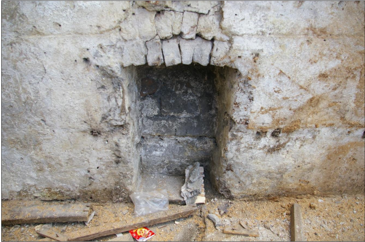
DETAIL OF THE GROUND FLOOR FIREPLACE WITHIN THE EAST WALL OF THE BARN STRUCTURE; VIEWED FROM THE WEST (NO SCALE).
