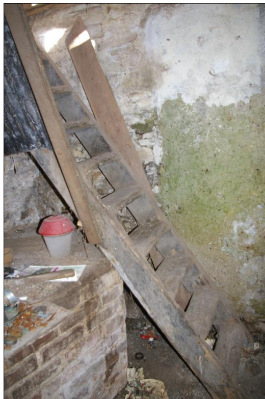
THE TIMBER STEPS IN THE NORTH-WEST CORNER OF THE BARN LEADING TO THE LOFT; VIEWED FROM THE SOUTH-EAST (NO SCALE).
