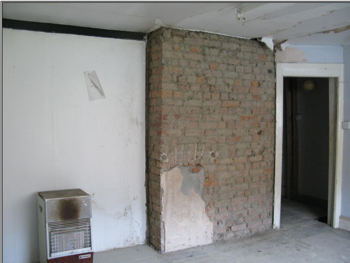
Figure 15: Chimney stack in Room 9 showing blocked opening.
