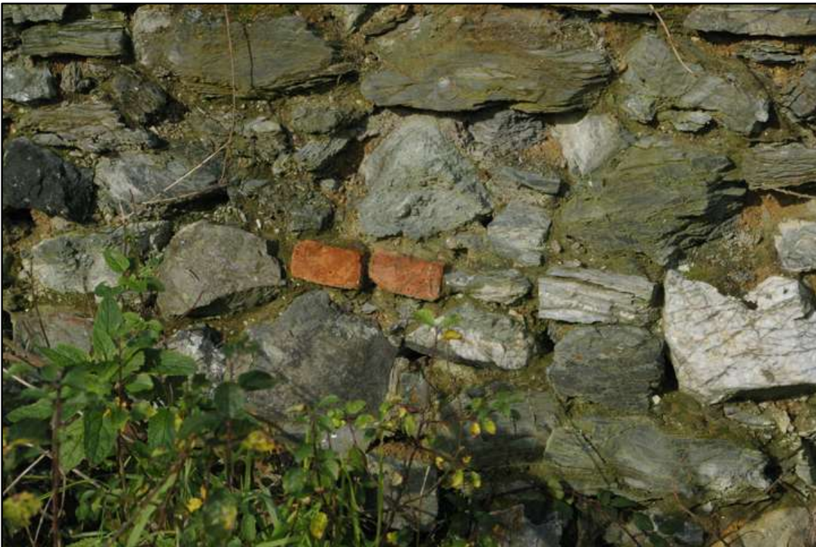
Bricks in south facing wall of ruin adjacent to tips c.5m×13m; looking north (2m scale).
