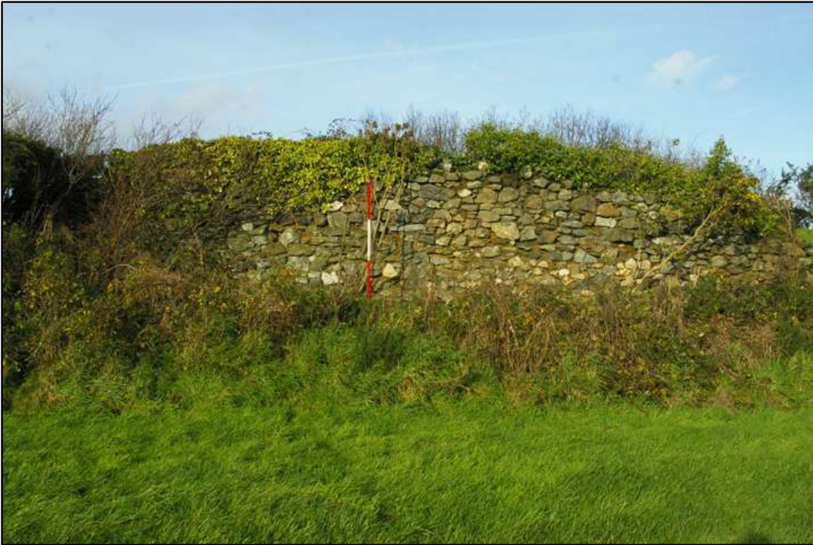
South side of ruin adjacent to tips c.5m×13m; looking north (2m scale).
