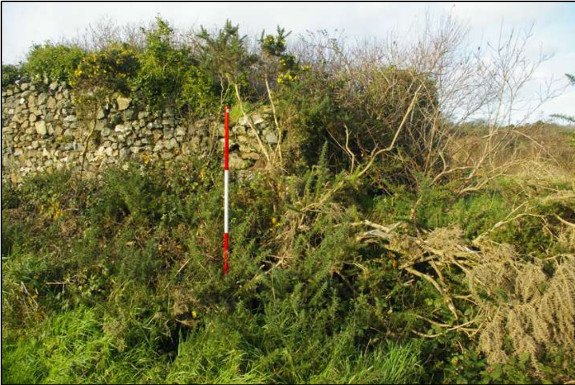
South-east corner of ruin adjacent to tips c.5m×13m; looking north-east (2m scale).
