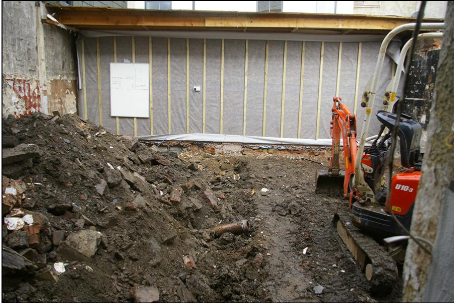
FIGURE 2: EXCAVATED PART OF THE MAIN STORE ROOM, SHOWING CENTRAL SERVICE; VIEWED FROM THE EAST (NO SCALE).
