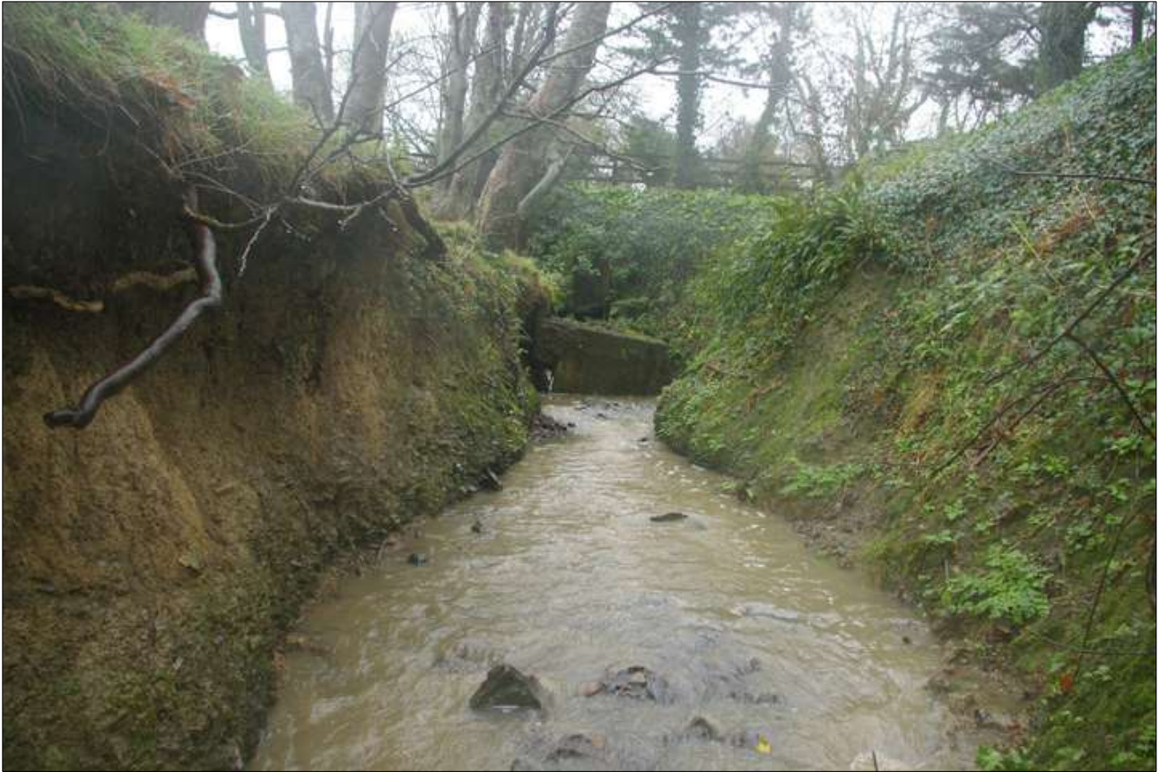
The culvert and watercourse at the northern end of the northern boundary; looking north (no scale).
