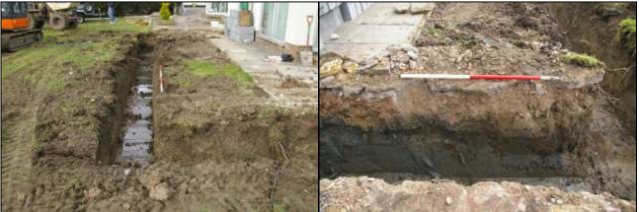
(Left) Figure 6: Western footing, aligned north-south; viewed from the south (2m scale).
