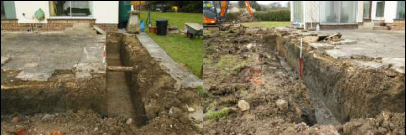
(Left) Figure 2: Eastern footing, aligned north-south; viewed from the south (2m scale).
