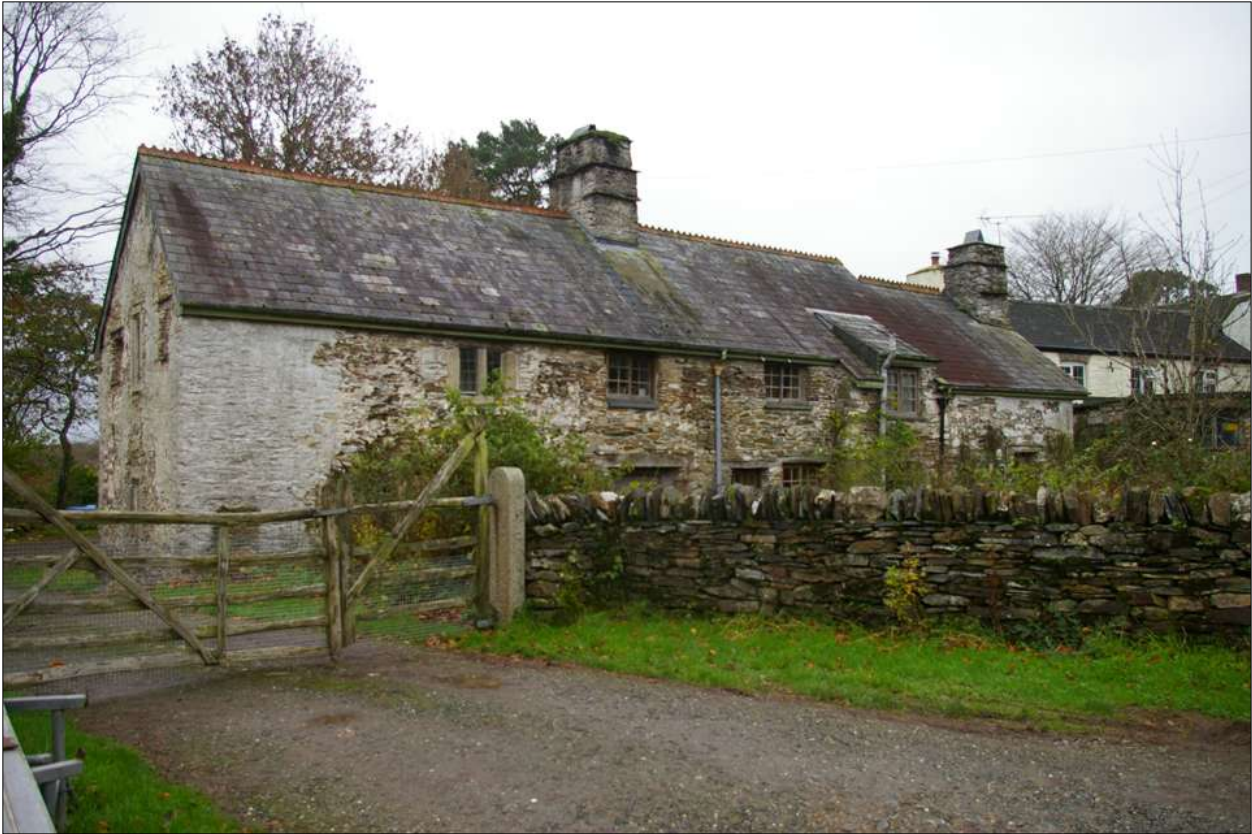
The GII Listed White Cottage in Lower Methereil, viewed from the north.
