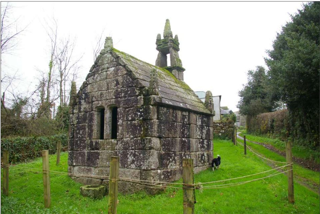
The GI Listed holy well at Dupath Farm, viewed from the north.
