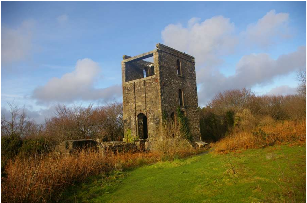
The enginehouse and part-ruined buildings, on the moorland, a Grade II Listed building; viewed from the south-south-east.
