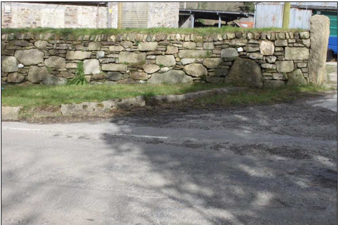
FIGURE 15: NEWLY BUILT HEDGEBANK TO TRELOWETH FARMYARD (OPPOSITE NO. 5), THE KERB IN FRONT INCLUDES NUMEROUS RE-USED GRANITE GATE POSTS AND LINTELS, FROM THE SOUTH (NO SCALE).
