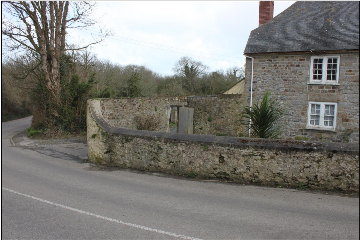
Grade II Listed boundary walls to Treloweth Farmhouse; viewed from the south.
