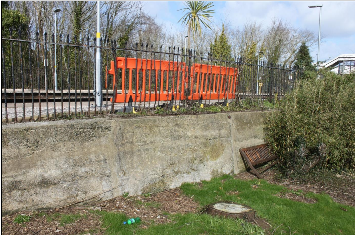
Repairs at western end in Kingdom Hall plot; viewed from the south.
