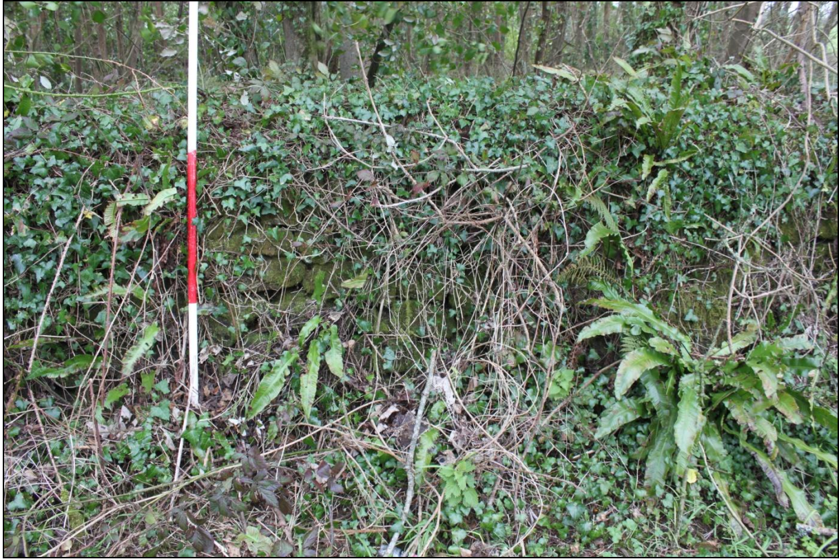
Stone wall/facing along road of woodland (detail); viewed from the north-east (2m scale).
