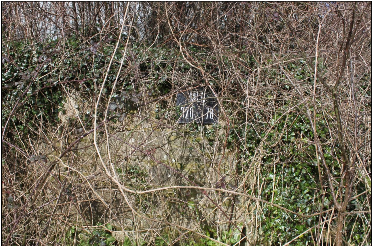
Western end of platform retaining wall, with sign (detail); viewed from the south-east.
