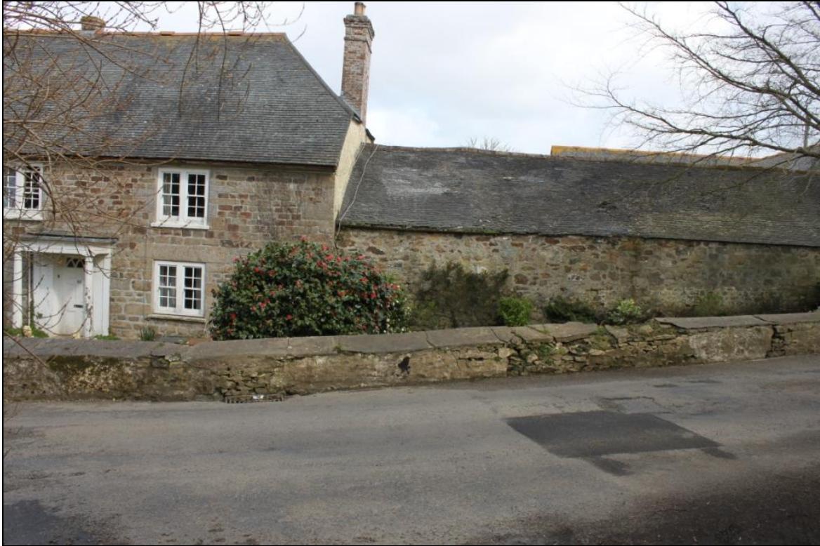
FIGURE 12: TRELOWETH FARMHOUSE (NO.10) AND PARTS OF ITS GRADE II LISTED GARDEN WALLS, NOTE THE CRACKS AND DAMAGE, VIEWED FROM THE SOUTH-WEST (NO SCALE).
