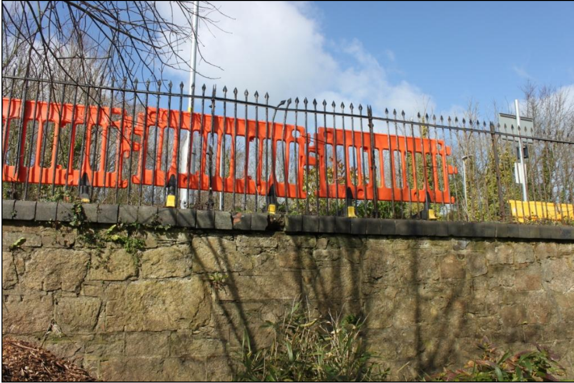
FIGURE 16: DAMAGED RAILING AND BRICK CAPPING TO THE PLATFORM, VIEWED FROM THE SOUTH IN THE KINGDOM HALL GARDEN (NO SCALE).
