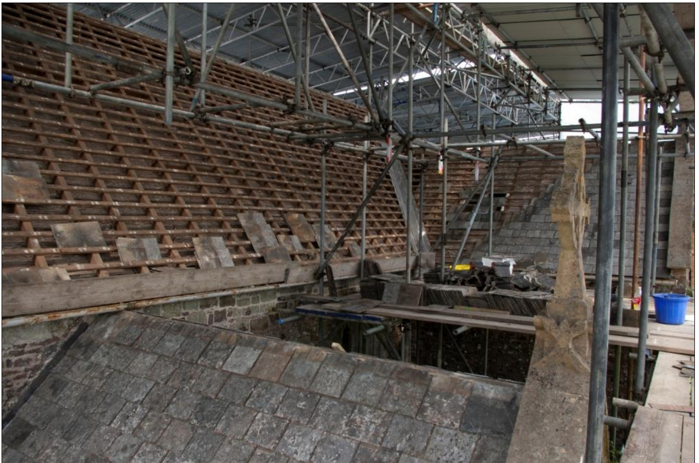
Figure 3: View of roof of the nave, from above the south porch, viewed from the south-west (no scale).
