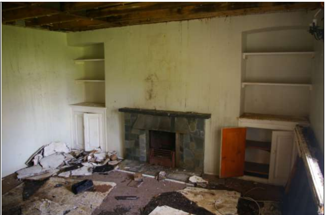
Room 1, showing modern fireplace within possibly replaced stack, ceiling is also 20 th century, with steel RSJ inserted; from the north-east
