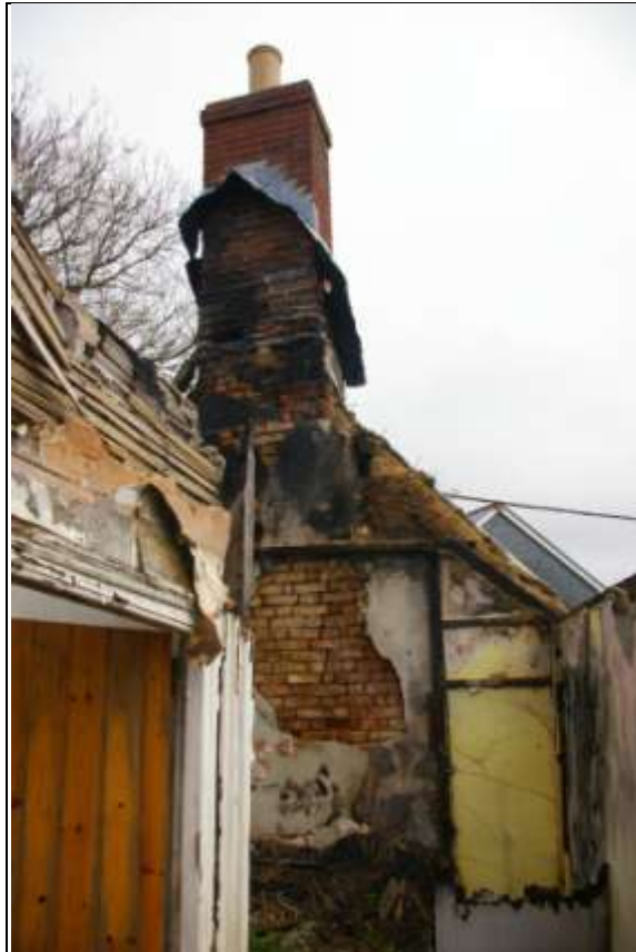
The eastern chimney stack, the upper shaft of which is in 20 th century brickwork but the rest of which (and gable) all appears original, of historic brick and cob; from the west, south-west.
