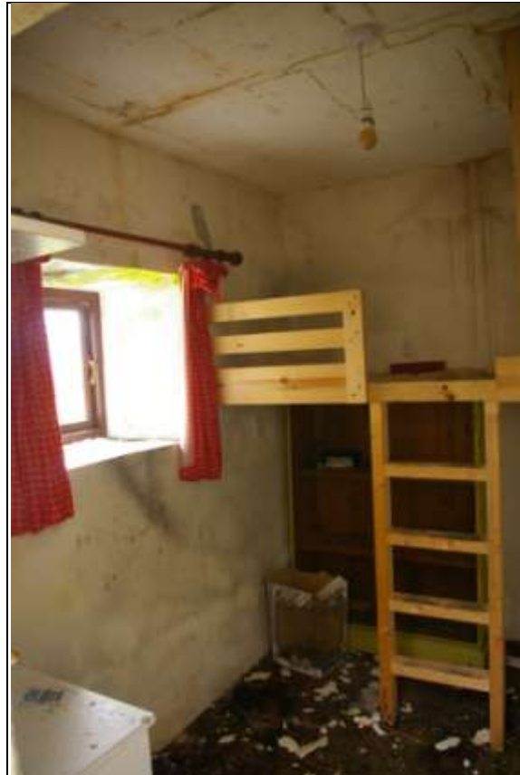
Room 7, wholly renovated and modernised, walls may have been partially replaced with concrete block in places; from the east, north-east.
