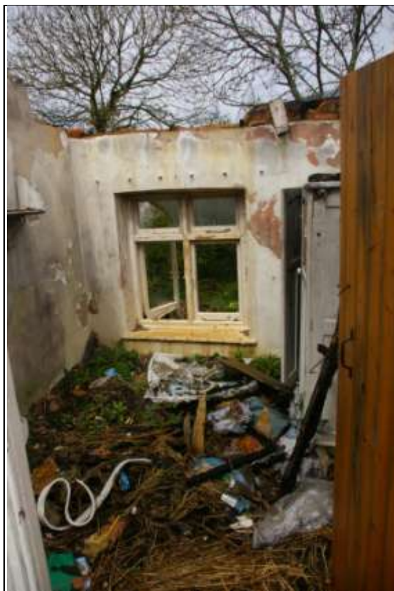
Room 13, mid 20 th century window, modern plank door in moulded original door frame; from the south, south-east.
