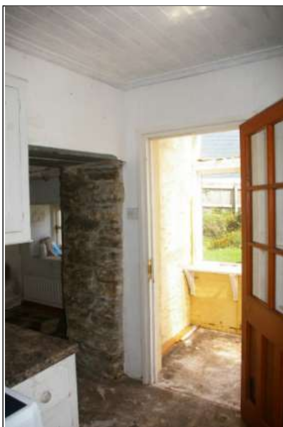
The rear wall of the 19 th century extension, from within Room 5, showing the forced opening to Room 4 and also Room 6, the part glazed lobby/conservatory; from the south-west.
