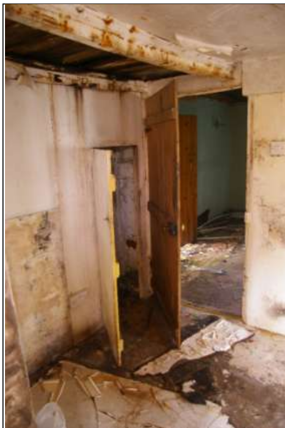
The door to Room 3 and modern cupboard under the stairs in Room 4, the wall under the stairs is of brick and timber framing and is of 19 th century date, probably the original division of the space; from the south-east.
