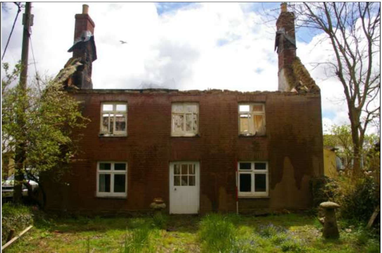
The north elevation of the farmhouse; from the north, north-west (2m scale).
