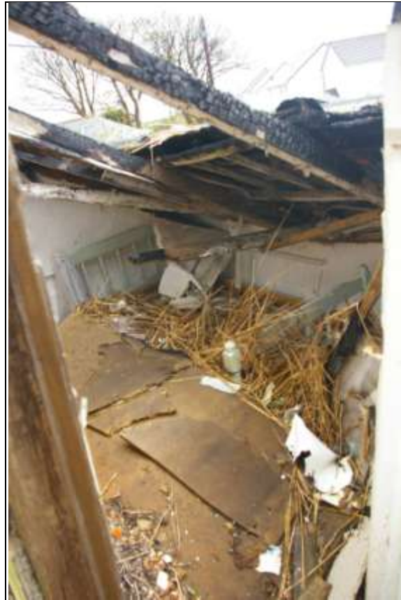
The small loft-style bedroom, Room 10, showing part of the surviving 19 th century roof structure; from the west, north-west.
