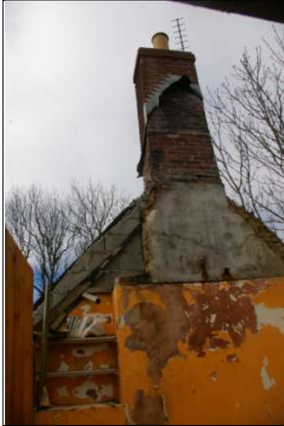
The western chimney stack, the upper shaft of which is wholly 20 th century and much of the south part of the gable appears to have been rebuilt in concrete blocks; from the east, south-east.
