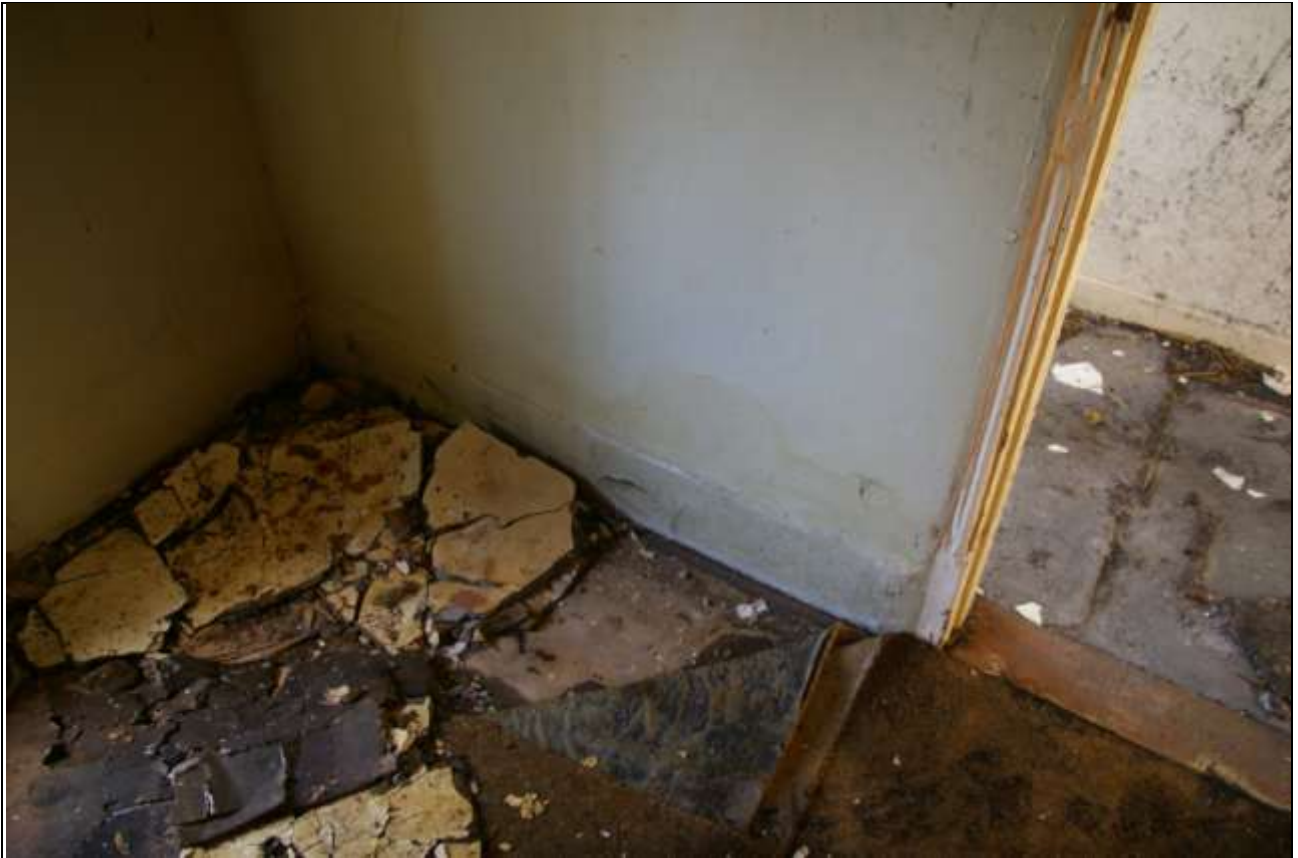
Section of surviving original deep plain plaster skirting, the only section found in the house, in the north-east corner of Room 1, along the partition wall; from the south-west.
