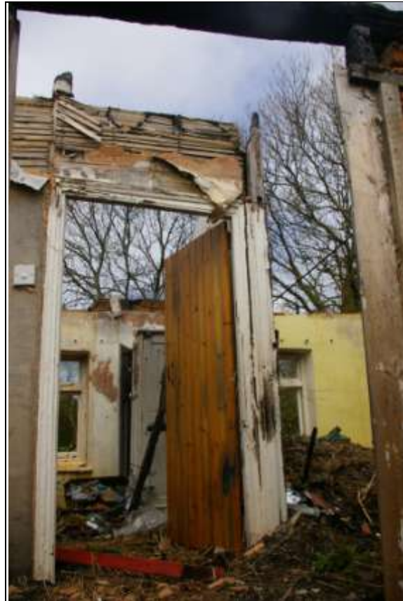
The landing, with the surviving lathe and plaster walls of Room 13 and original moulded door frame; from the south.
