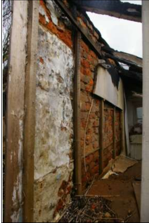
The brick rear wall of the house, with timber noggin and later surface mounted timber framing, visible within Room 10; from the west, south-west.
