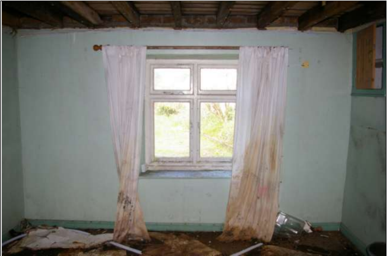
Mid 20 th century replacement window in Room 3, also showing the 20 th century ceiling with steel RSJ fitted; from the south.
