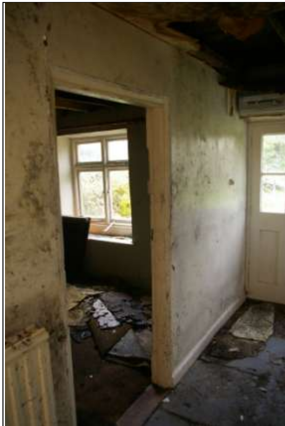
View of the original lathe and plaster partition wall to Room 1 and the moulded door frame, the door is modern, with mid 20 th century replacement window beyond; from the south-east.
