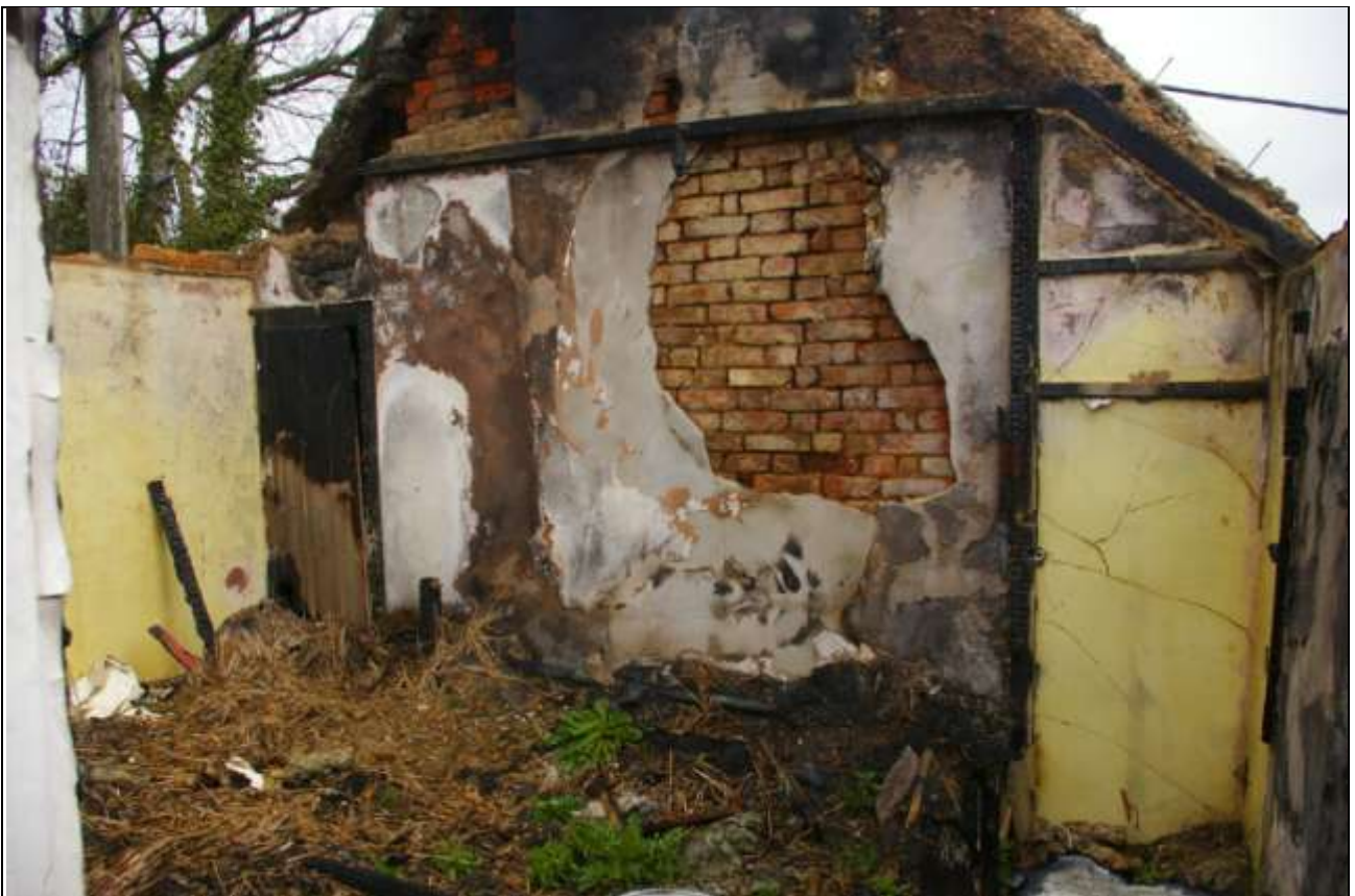
Room 12, the eastern chimney stack with small cupboard and surviving cob and lime plaster to the walls in places; from the south-west.
