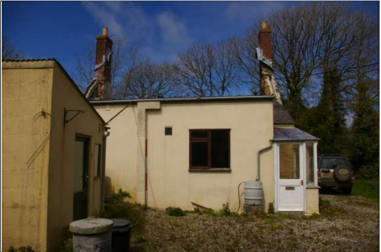
The rear of the house, with modern extension and part glazed lobby; from the south (2m scale).
