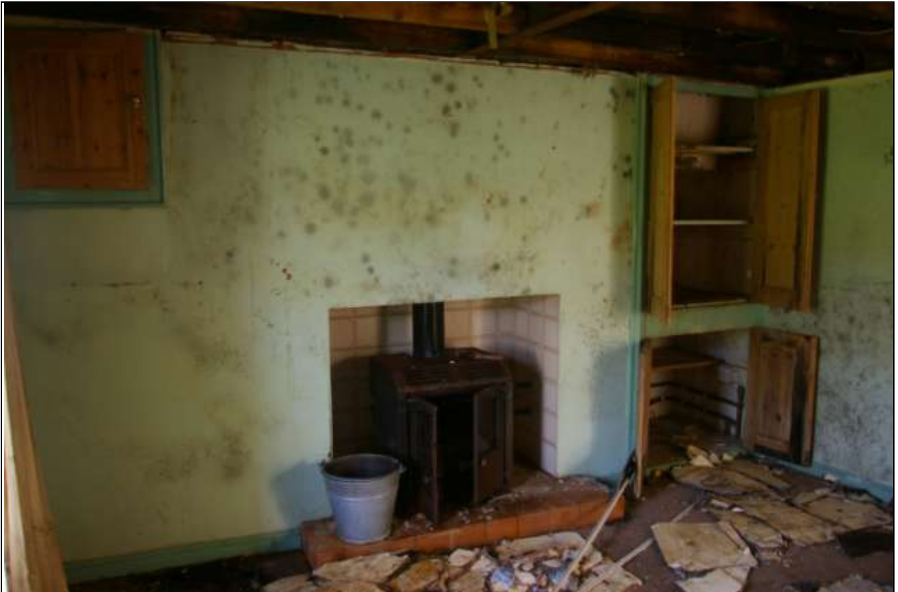
Room 3, with the altered original fireplace, now with stove, with small original beaded cupboard to the north and large 19 th century cupboard to the south, occupying position of former oven; from the north-west.
