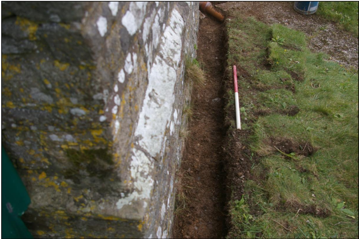
Figure 3: The trench alongside the west wall of the tower; viewed from the north (scale 1m).
