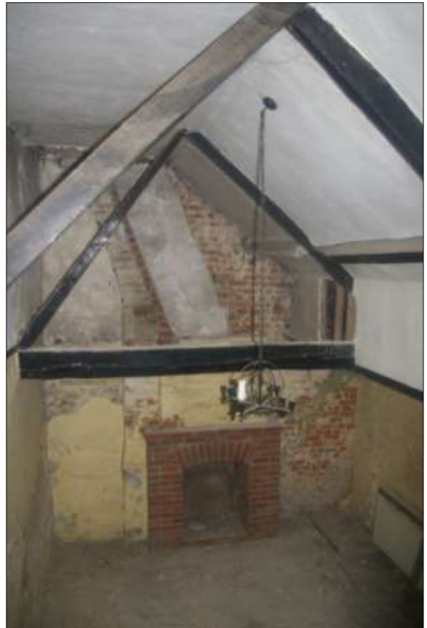
Figure 18: Room 7 viewed from the stair showing the scar of the laundry hood to the left of the fireplace
