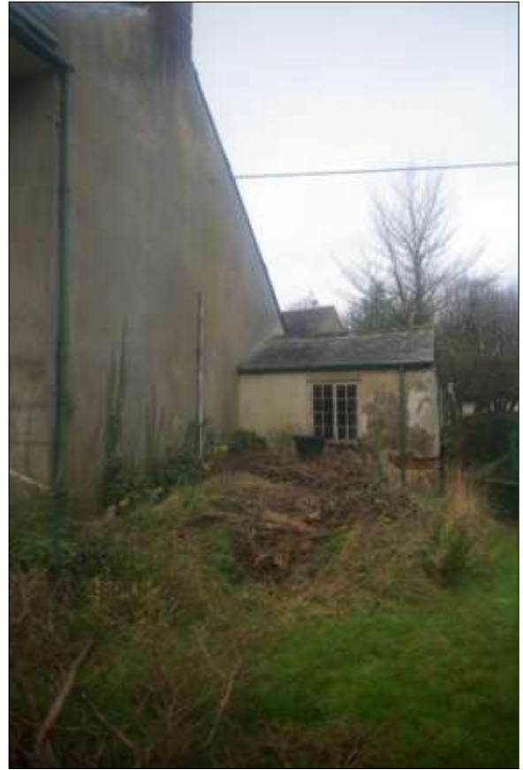
Figure 11: Raised area (probable remains of a demolished extension) to the east of the house.
