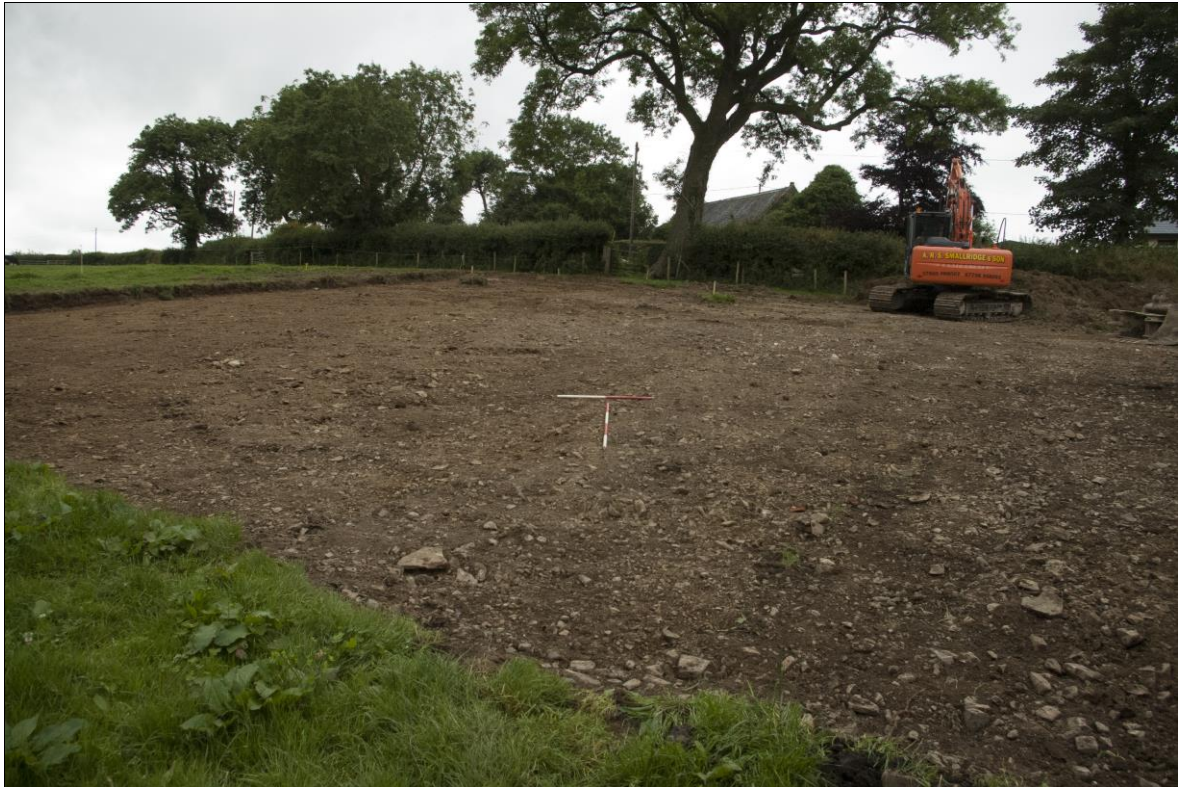
Figure 2: Post-excitation view of the site; viewed from the south-east (scale 1m and 2m).
