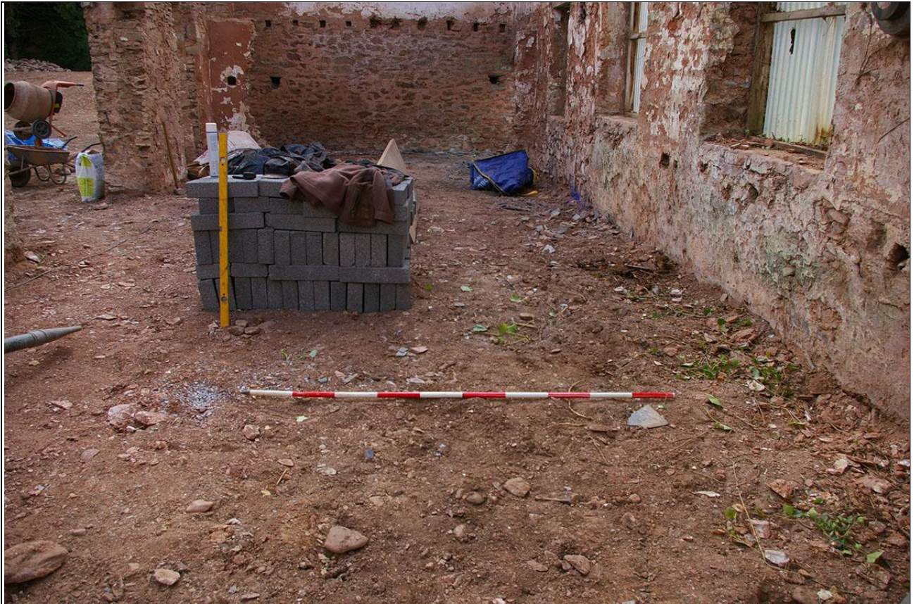
The largely stripped out and removed floors in the workshop building; from the west (2m scale).
