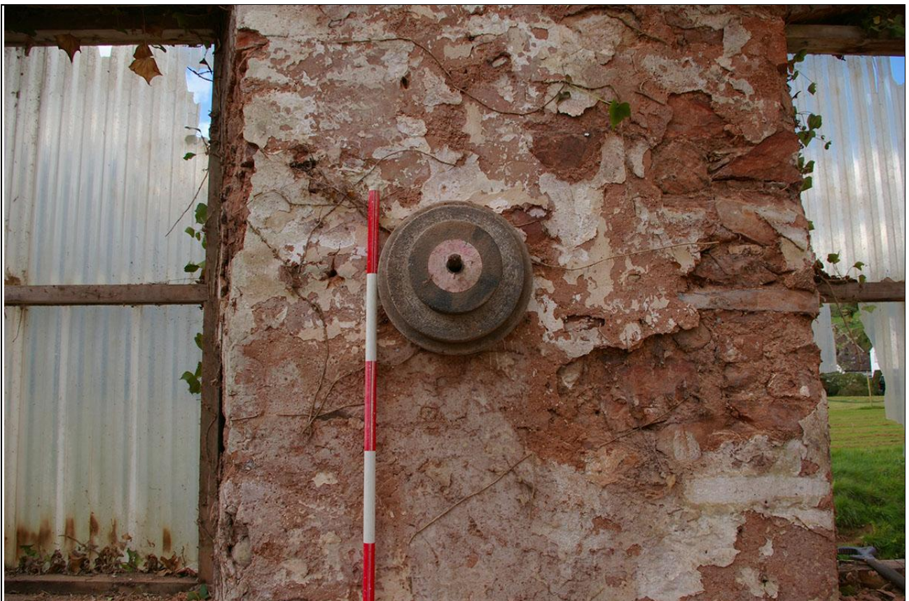
Piece of bracing machinery still attached to the south wall of the workshop; from the north (2m scale).
