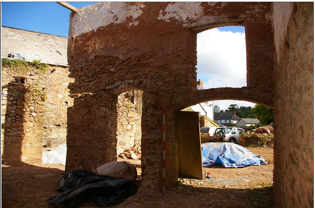
The interior face of the north wall of the workshop, east end; from the south (2m scale).
