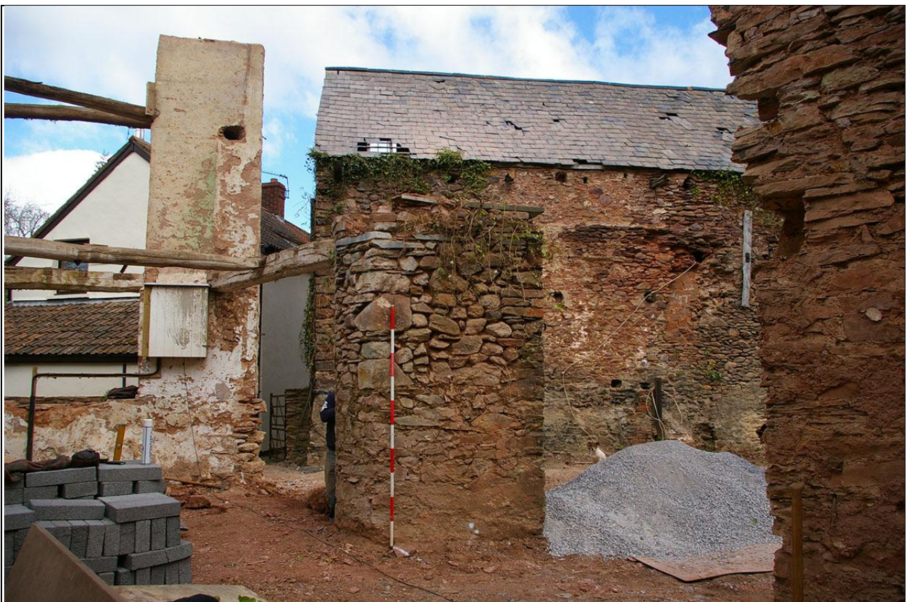
The intersect between the wheel pit bracing piers and the workshops later north-west section of walling/timber bracing; from the south-east (2m scale).
