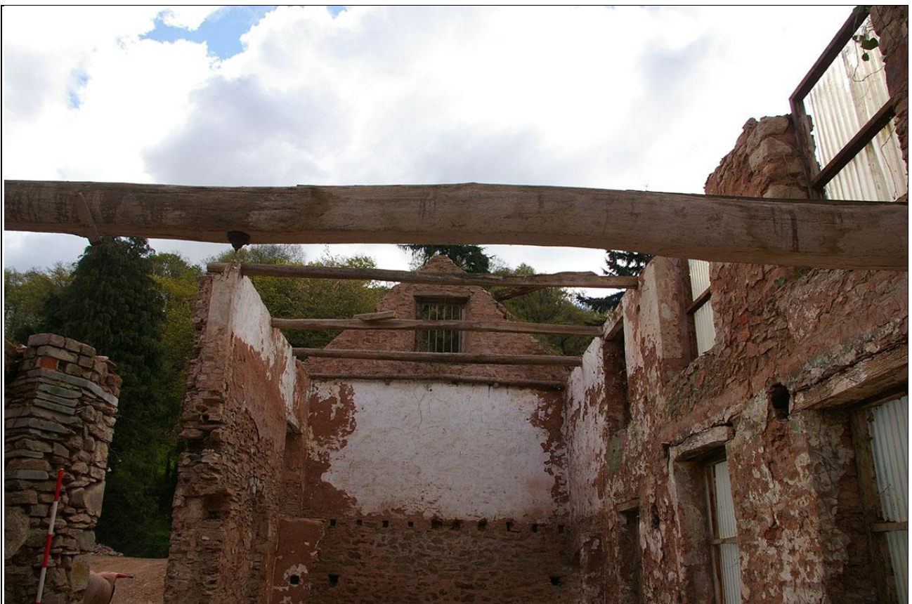
The surviving first and loft floor beams in the workshop building; from the west (2m scale).
