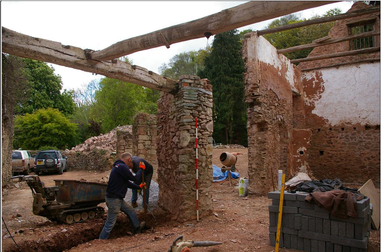
The intersect between the wheel pit bracing piers and the workshops later north-west section of walling/timber bracing; from the south-west (2m scale).
