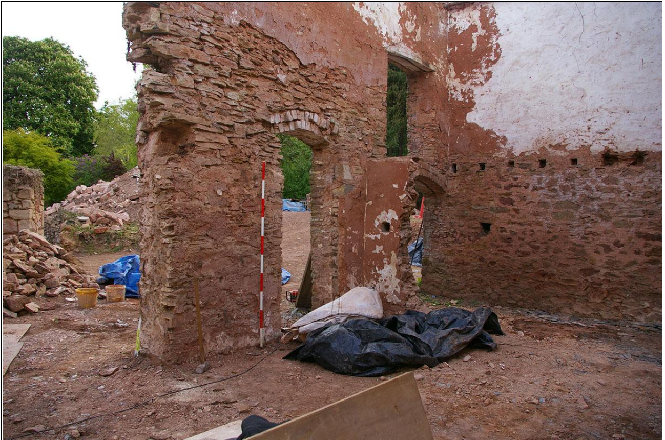
View of the east elevation, south end; from the north-west (2m scale).
