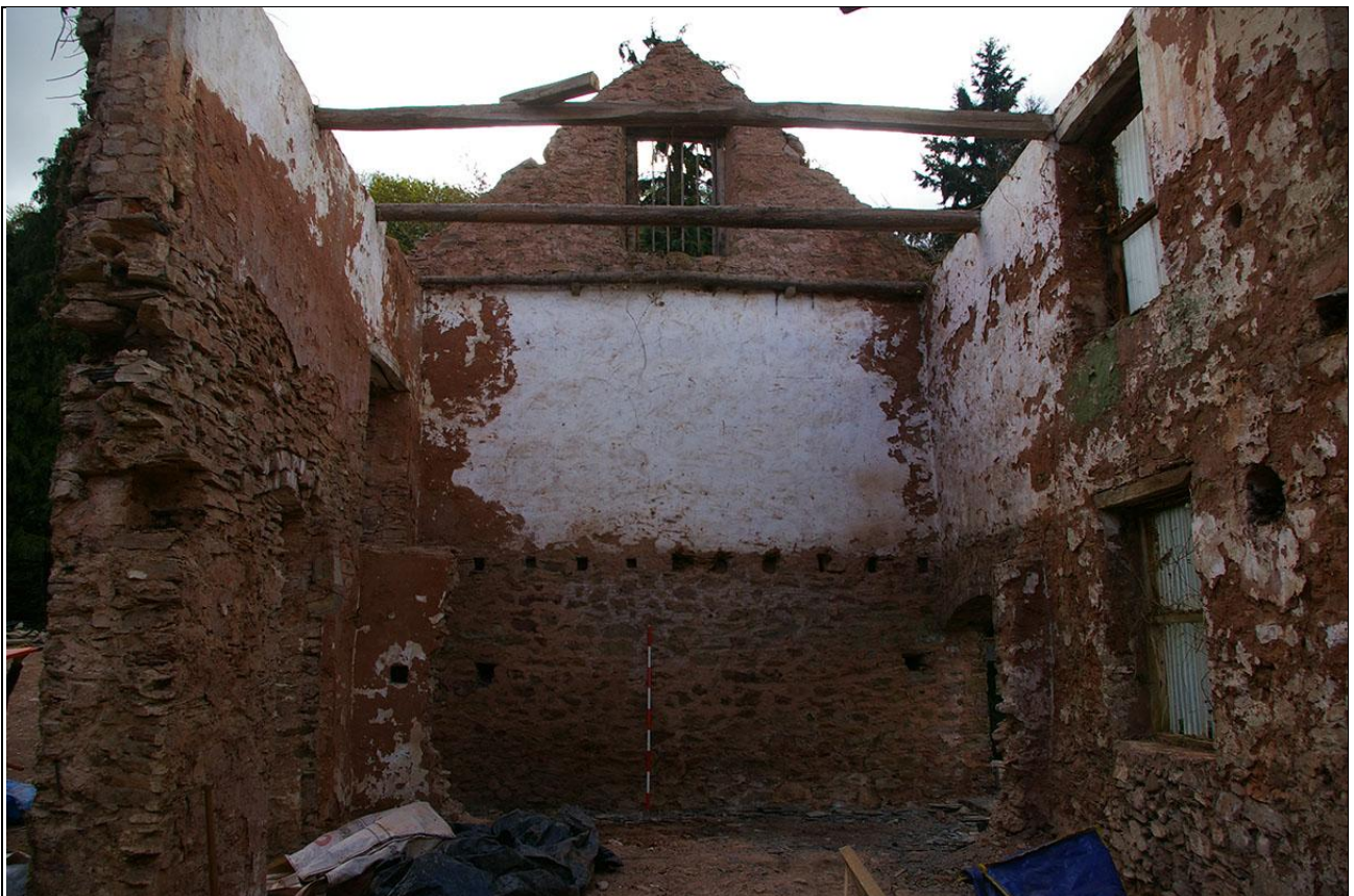
Wide view of the east end of the workshop, the earlier phase of the building; from the west (2m scale).
