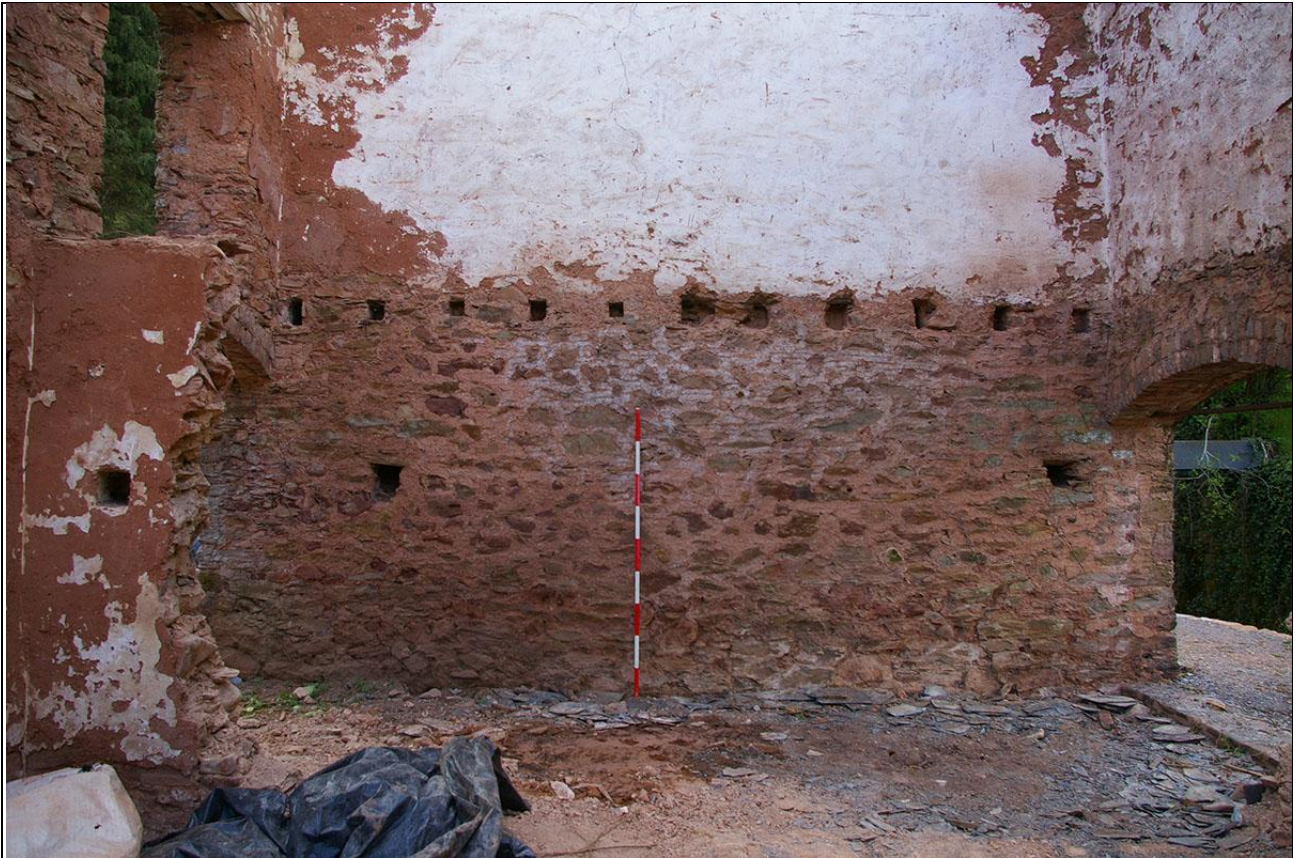
The sockets from the former first floor and ragged stub of the heavy stone partition floor, also showing sockets in it for some timber fixings within the building; from the west (2m scale).
