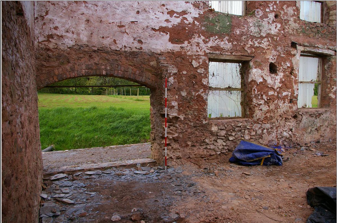
The interior face of the south wall of the workshop, east end; from the north (2m scale).
