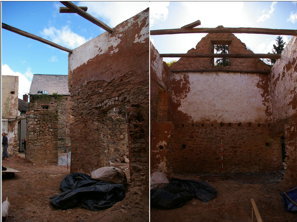
Left: The north elevation of the workshop, where it is open to the former wheelpit; from the south-east (2m scale). Right: The interior face of the east gable wall of the workshop; from the west (2m scale).
