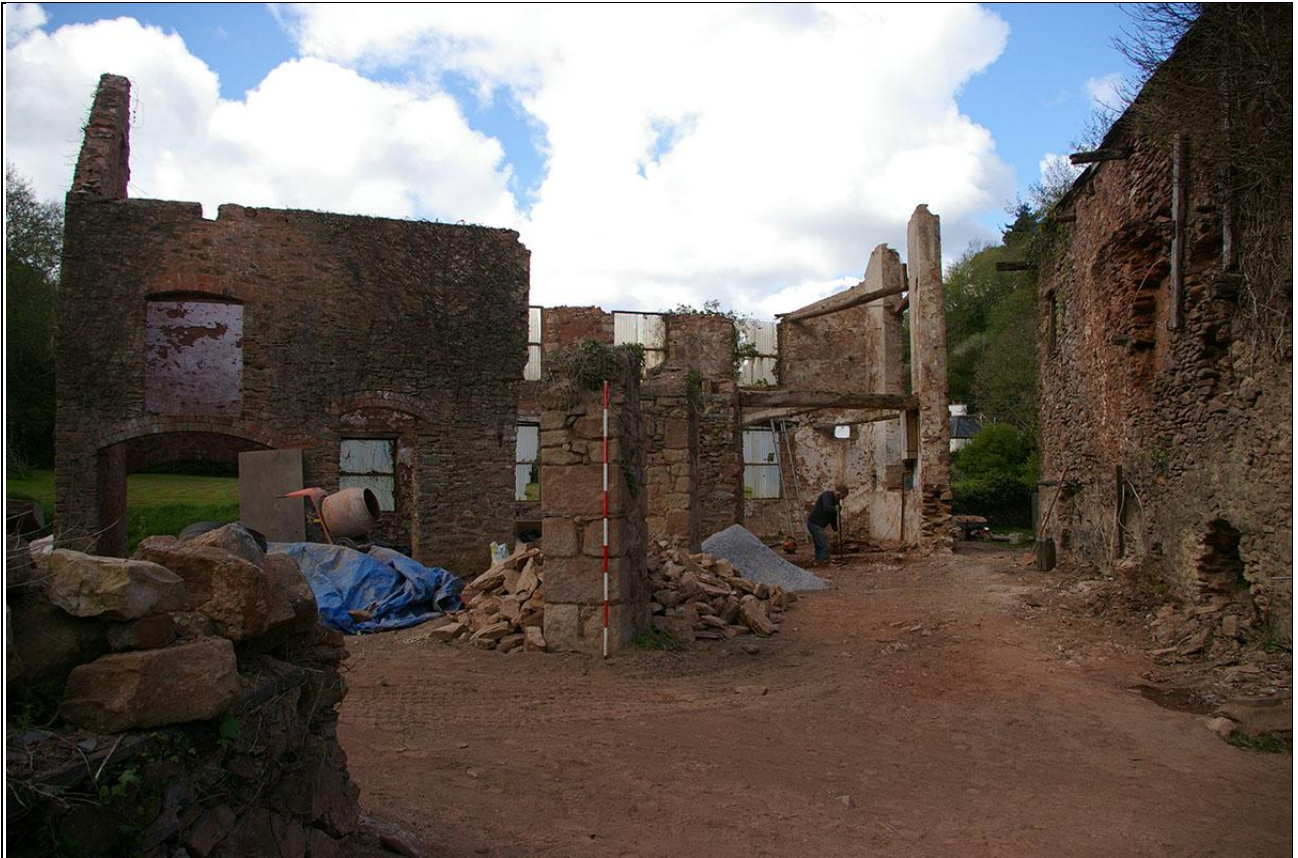
Wide view showing the workshop, infilled wheelpit and bracing piers and the older mill building; from the east (2m scale).
