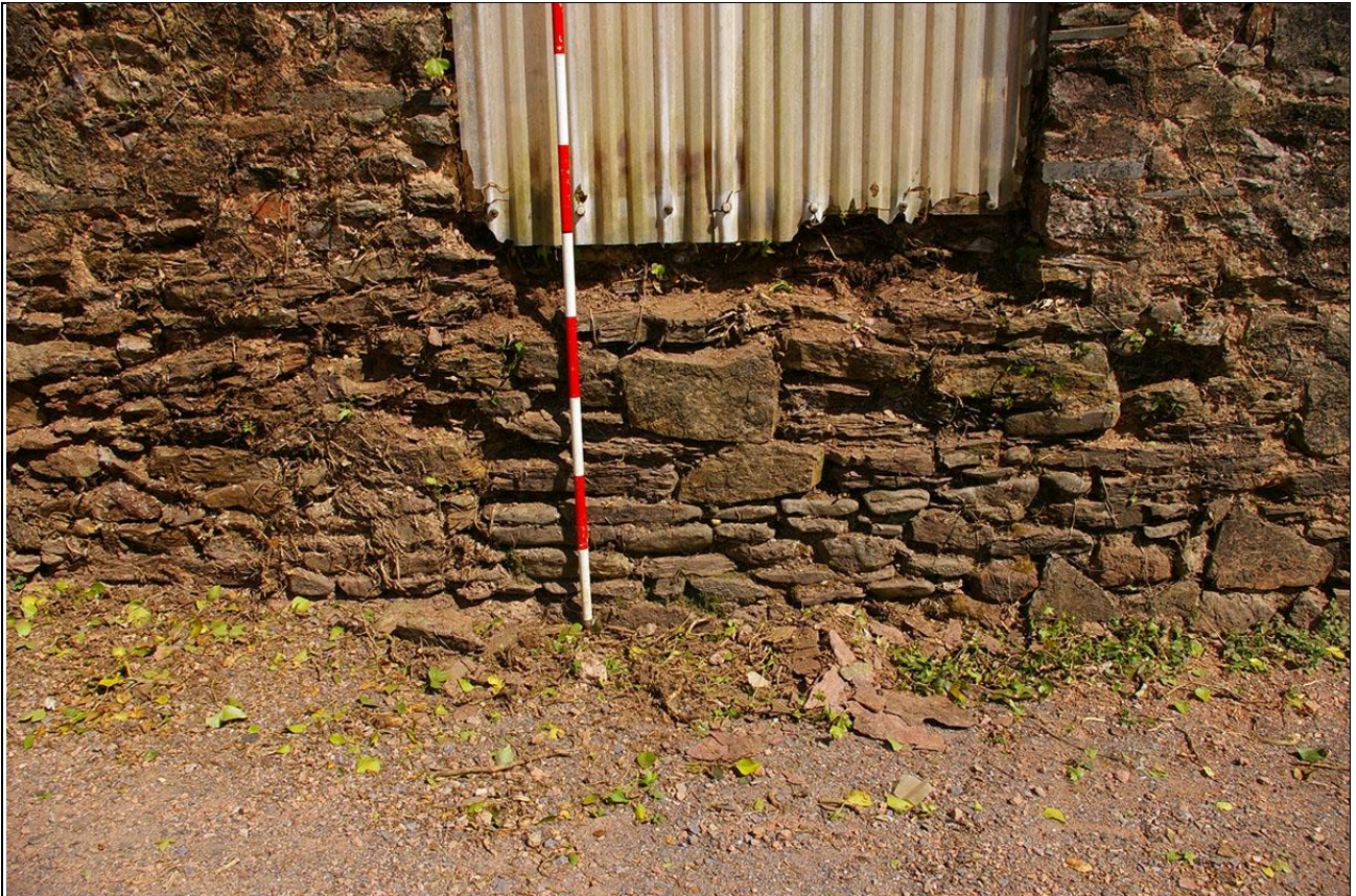
Build line visible in wall of south elevation, between extension to left and original walling to right; from the south (2m scale).
