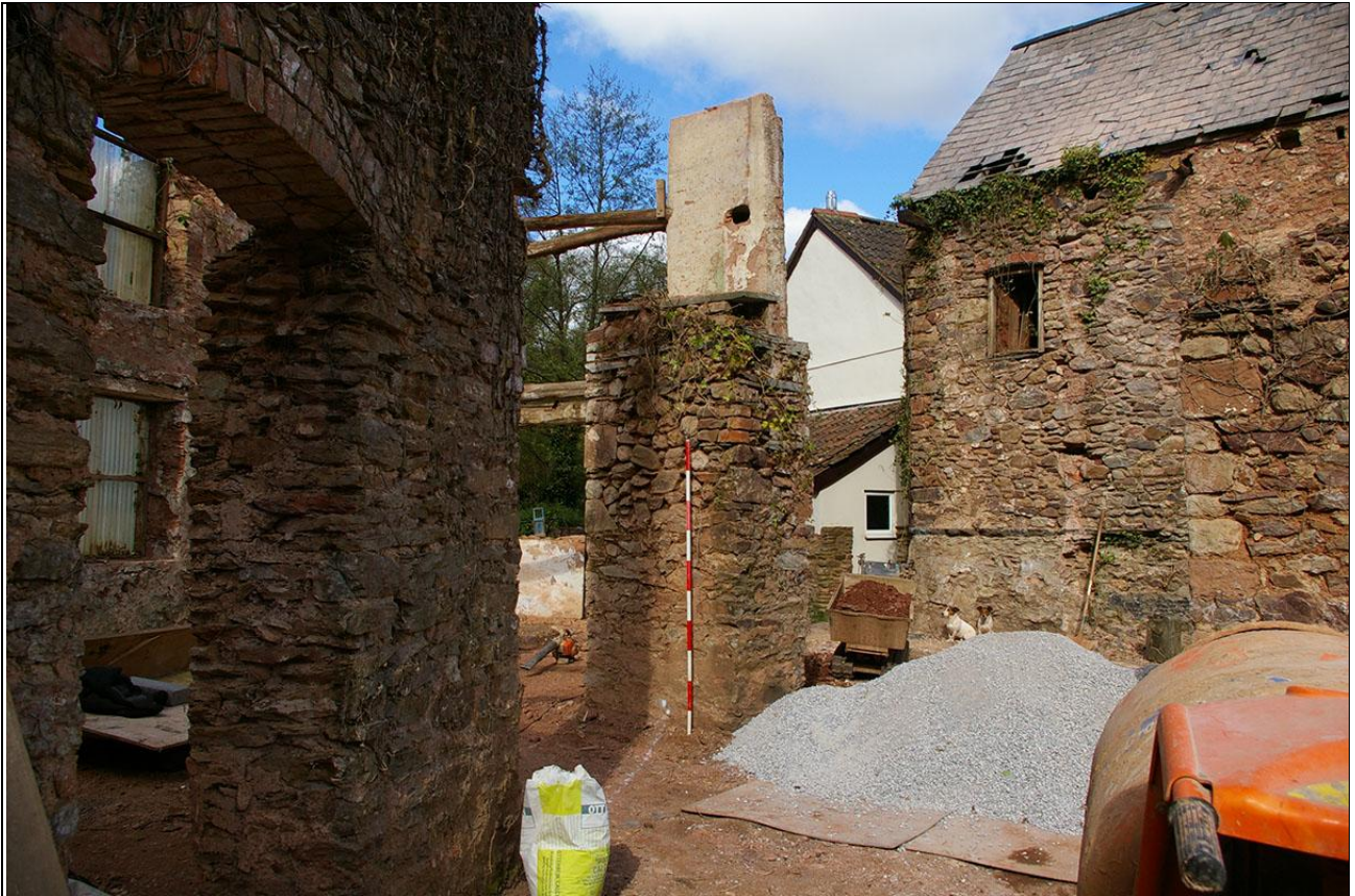
View of the oblique angle where the two structures of different phases, workshop and wheel pit walls intersect; from the east (2m scale).
