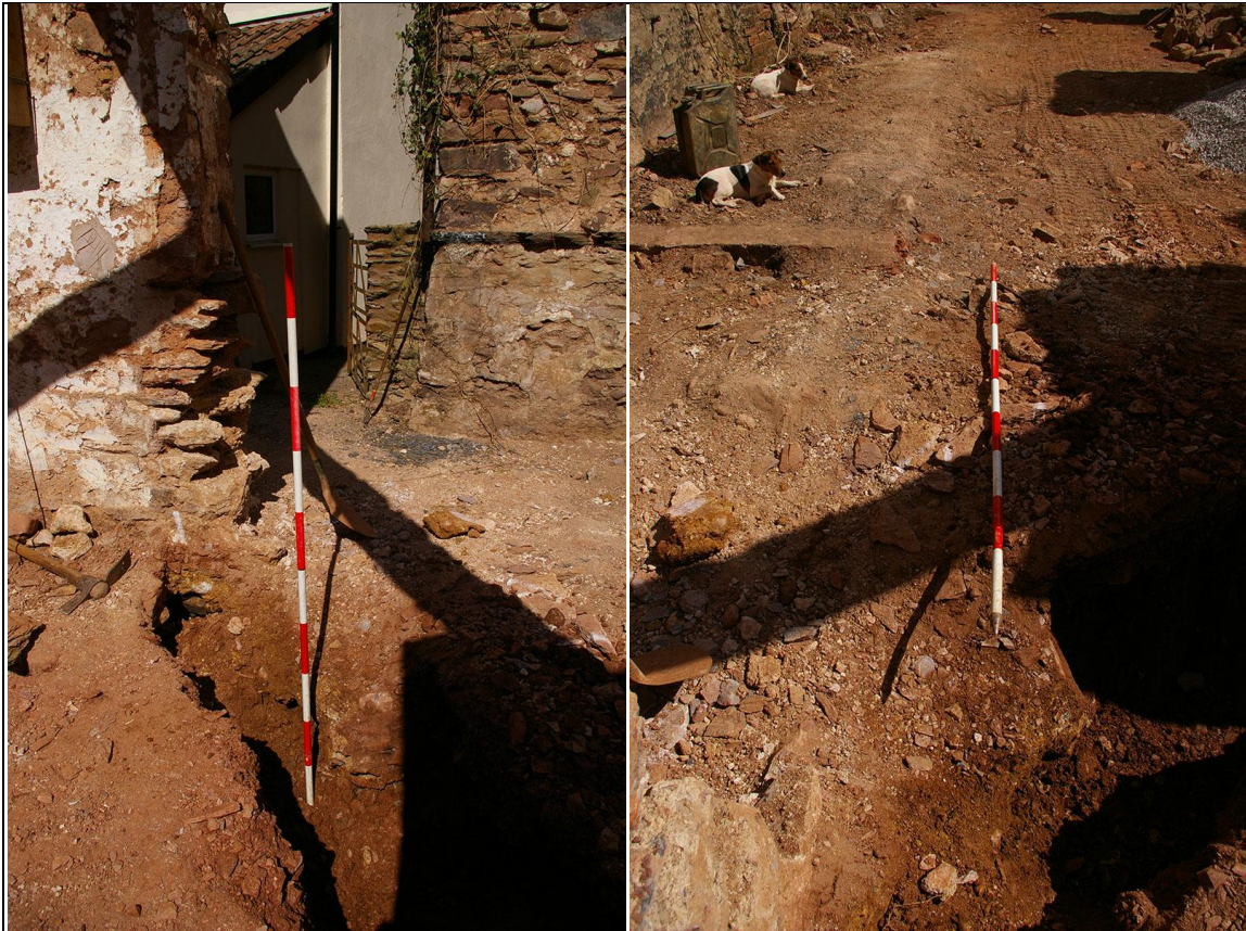
Left: The trench 1 where it abuts the north-west corner of the workshop building; from the east (2m scale). Right: The below ground surviving footings of the wheelpit retaining walls; from the south (2m scale).
