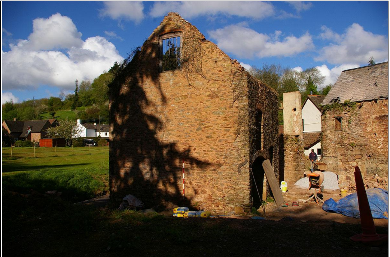
The east elevation of the workshop building; from the south-east (2m scale).
