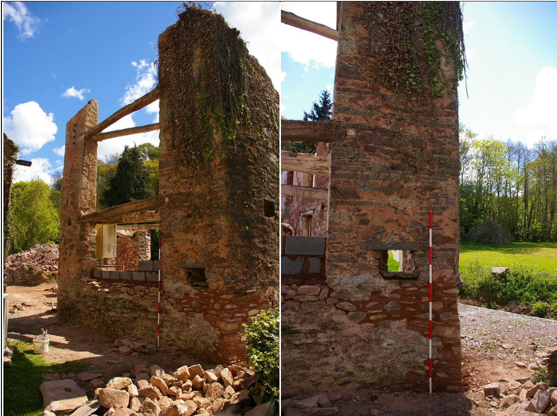
Left: The west elevation; from the south-west (2m scale). Right: The south-west corner; from the west (2m scale).
