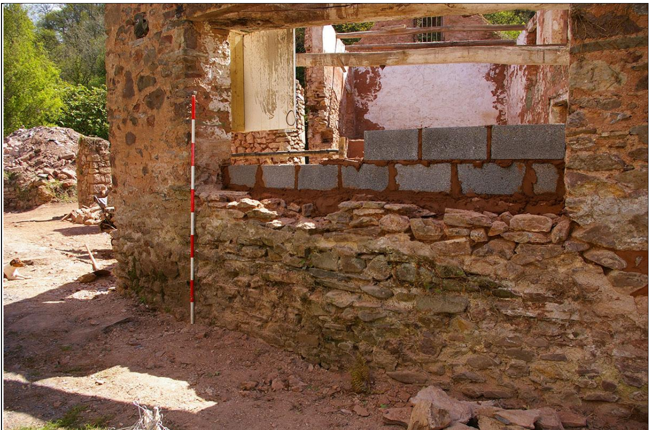
The heavier and earlier base of the west elevation of the workshop; south-west (2m scale).
