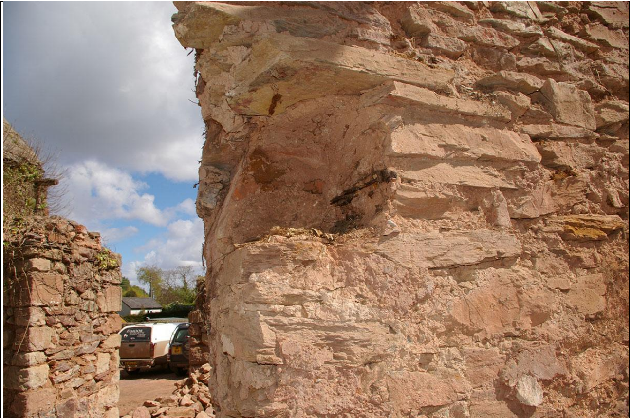
Large socket for timber, now removed, at the west ragged end of the north wall of the workshop, showing heavy iron nails in situ in the walls; from the south.
