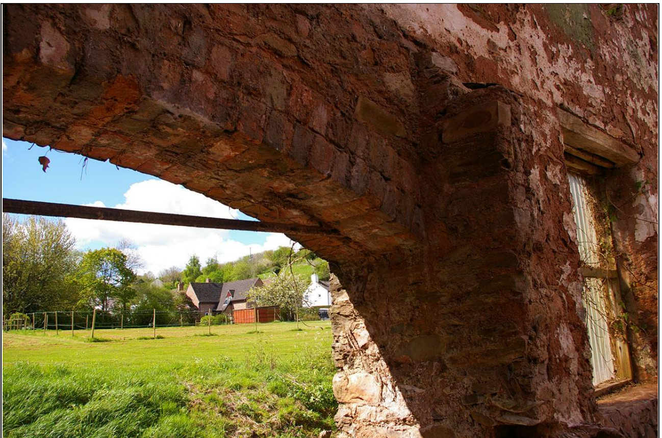
Ironwork bracing to the archway to the east of the south wall; from the north-east.
