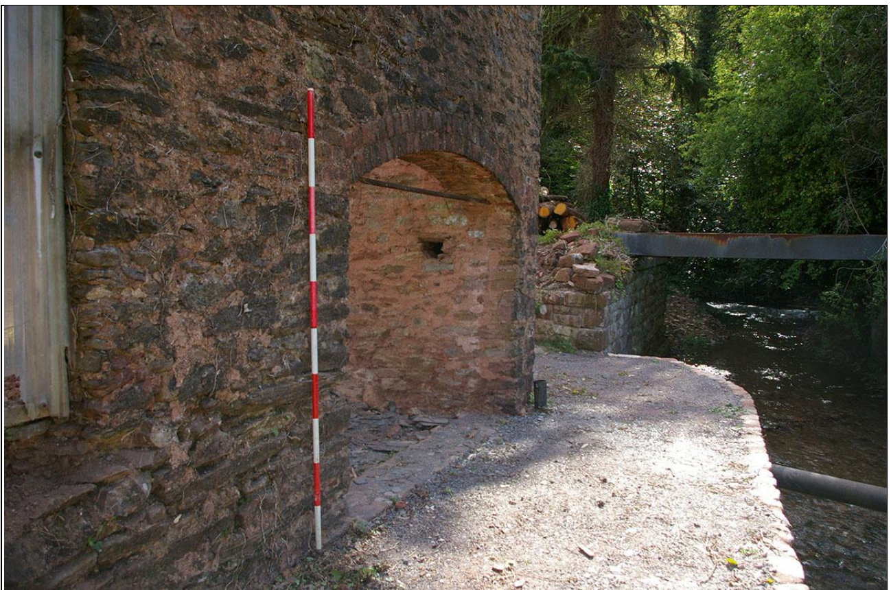
The large arched opening in the east of the south elevation; from the south-west (2m scale).
