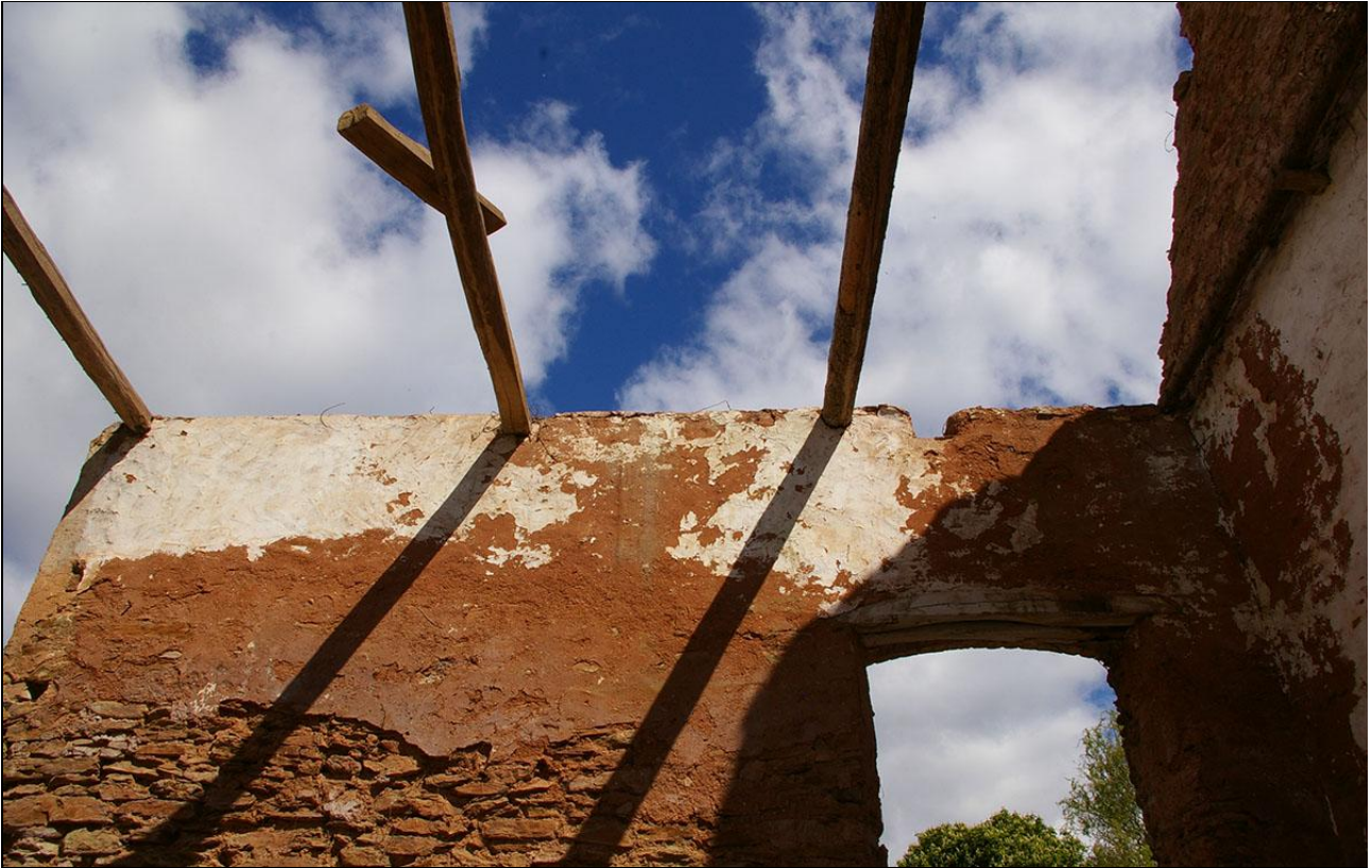
Two squared and roughly shaped/chamfered heavy beams to the left, two lighter weight, rounded and embarked poorer quality inserted beams to the right, suggesting a loft; from the south.
