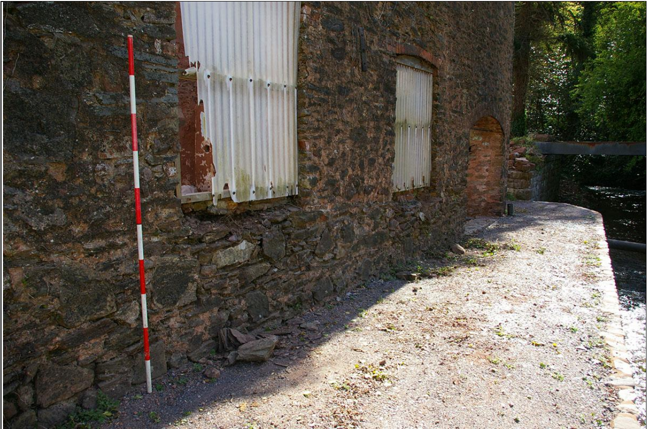
The east end of the south elevation and build line at the second window where the earlier building is abuted by early 20 th century stonework; from the south-west (2m scale).
