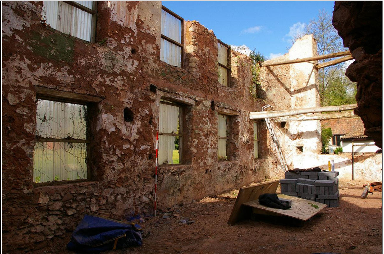
The interior face of the south wall of the workshop; from the north-east (2m scale).
