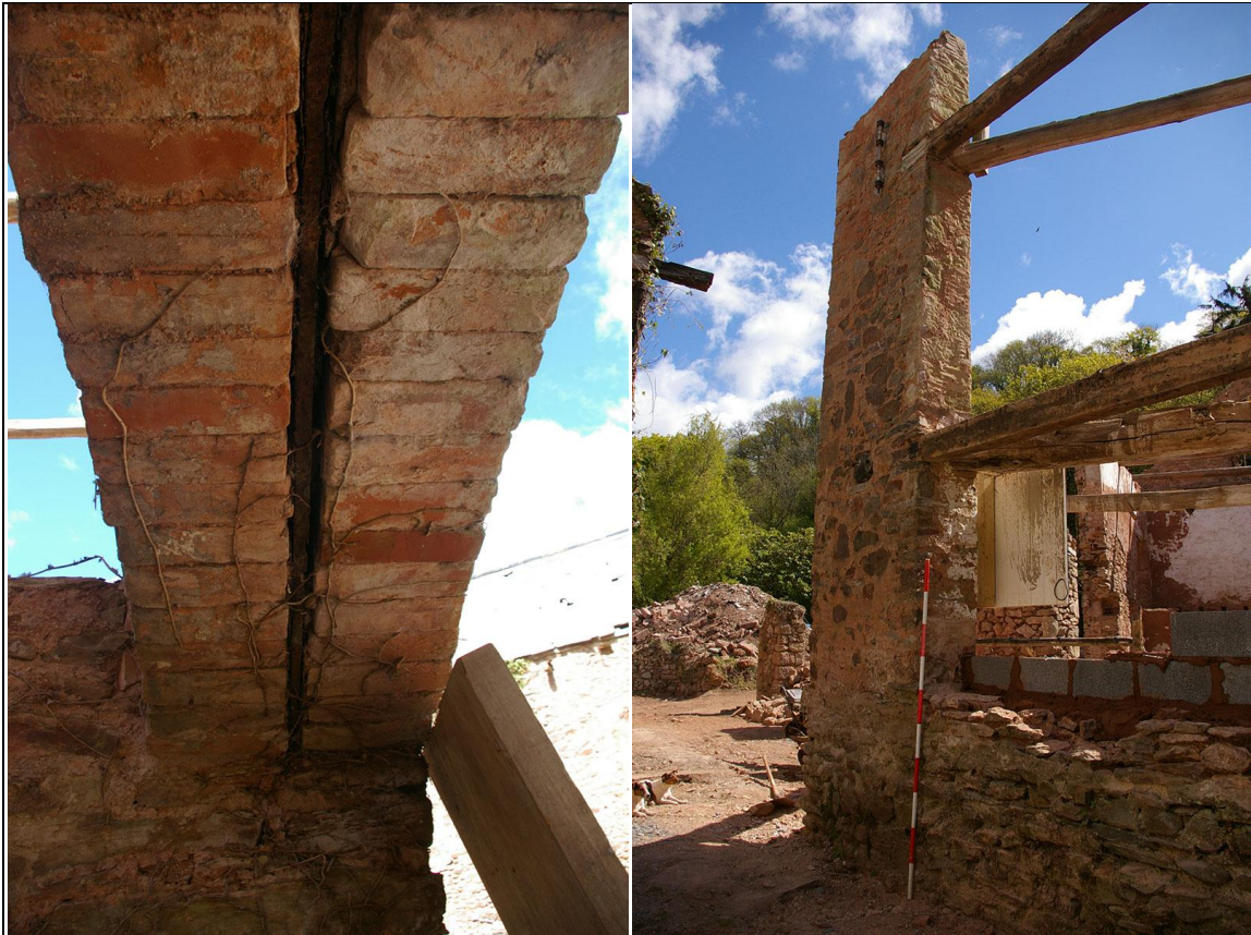
Left: The ironwork lintel bracing within the brickwork of the archway to the north wall; from the east. Right: The north-west corner of the workshop; from the south-west (2m scale).
