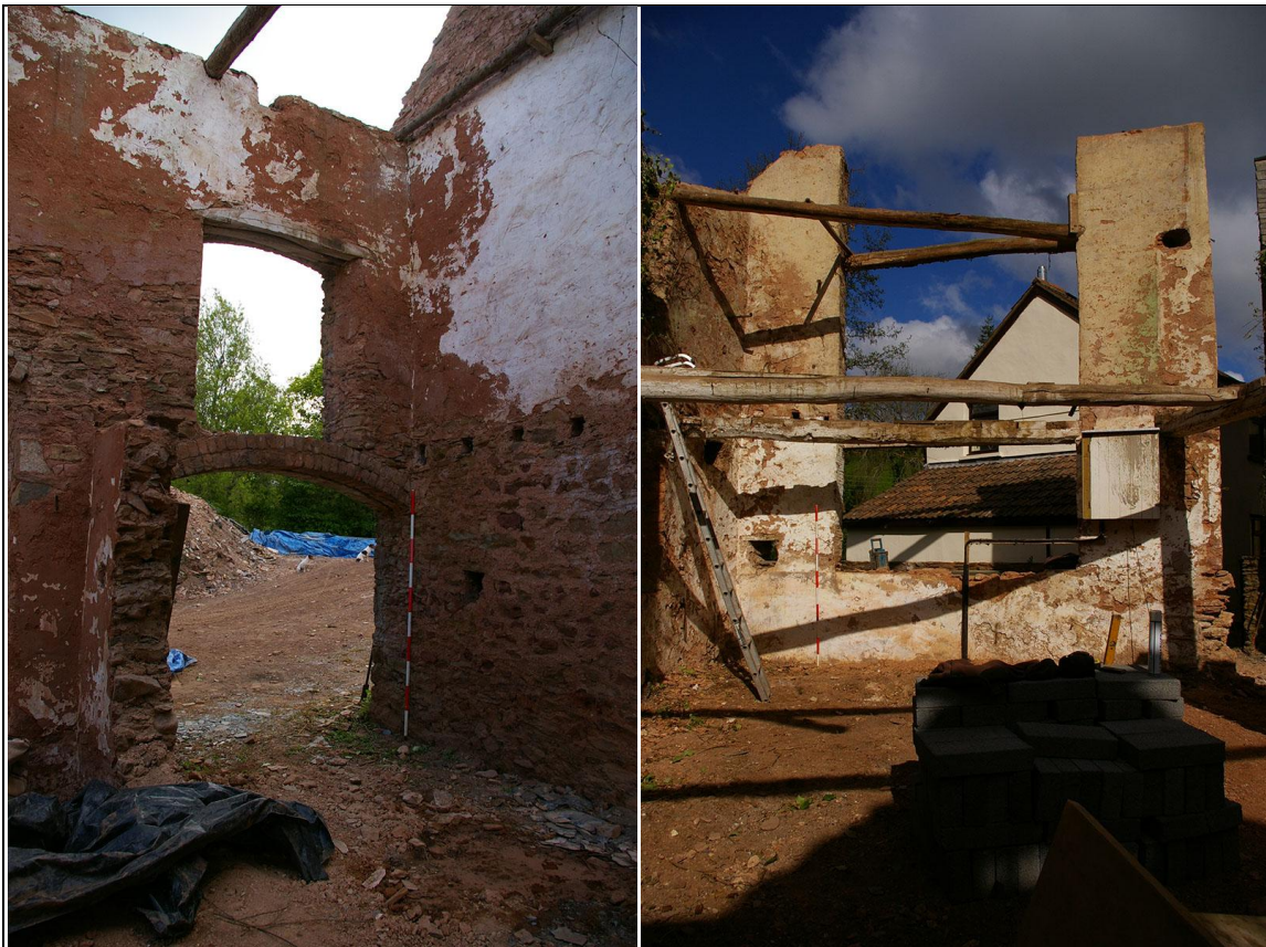
Left: The wide arched opening at ground floor in the north elevation, opposite that to the south; from the south-west (2m scale). Right: The west end of the workshop; from the east (2m scale).
