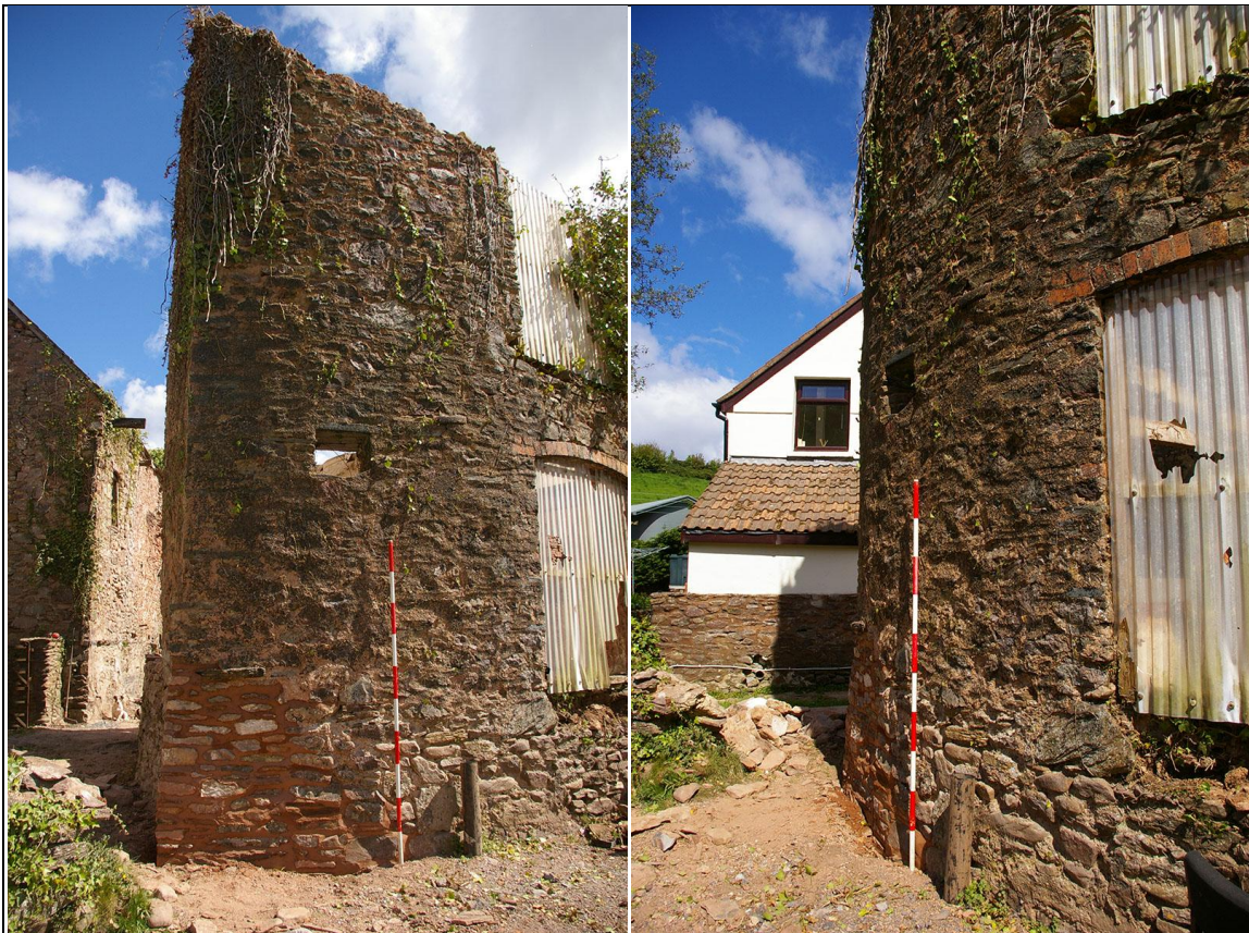
Left: Wider angle of south-west corner of the workshop building; from the south. Right: The curving south-west wall of the workshop building; from the south-east.
