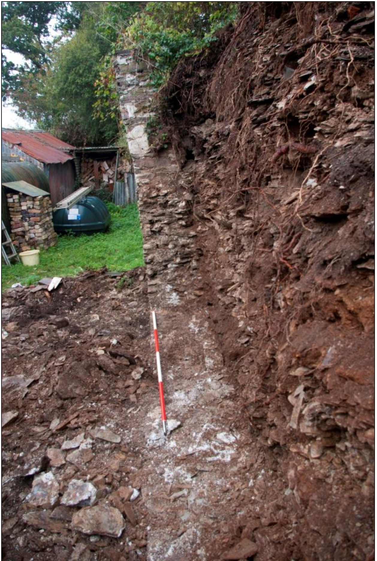
Figure 4: Shot of historic wall footing (scale 2m). Note the lean on the remaining historic wall, the upper corner was removed prior to the rebuilding.
