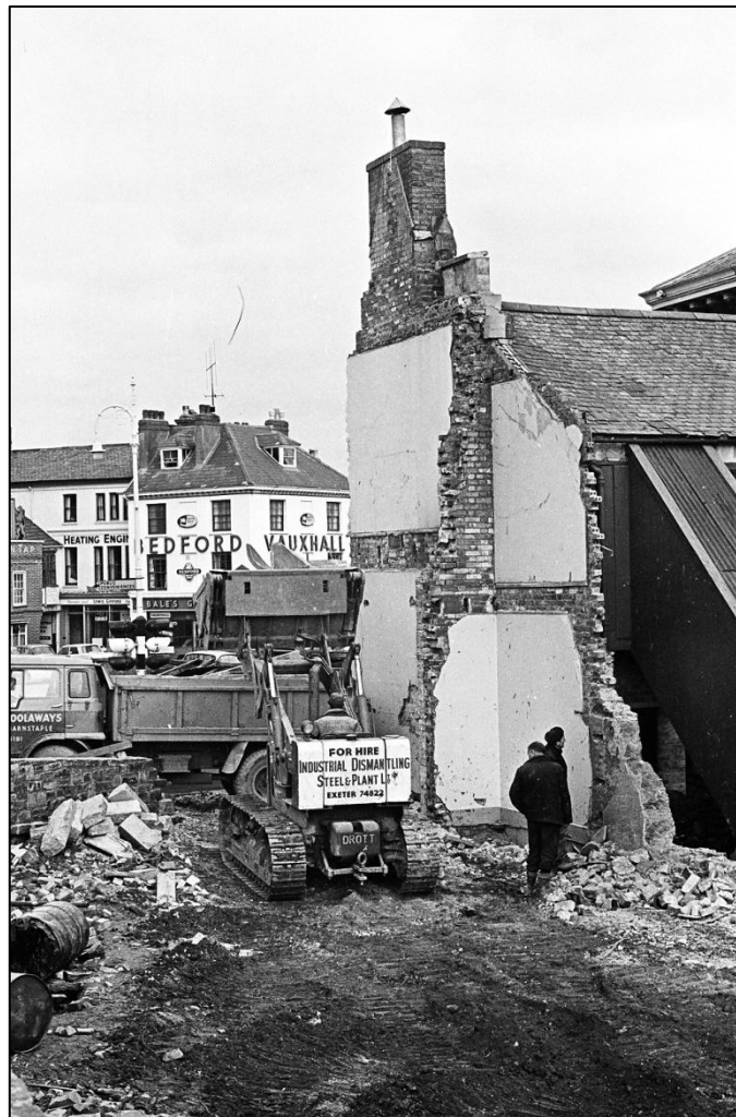
FIGURE 13: PHOTOGRAPH OF 1963 SHOWING BRIDGE END HOUSE IN THE PROCESS OF DEMOLITION (NDA).
