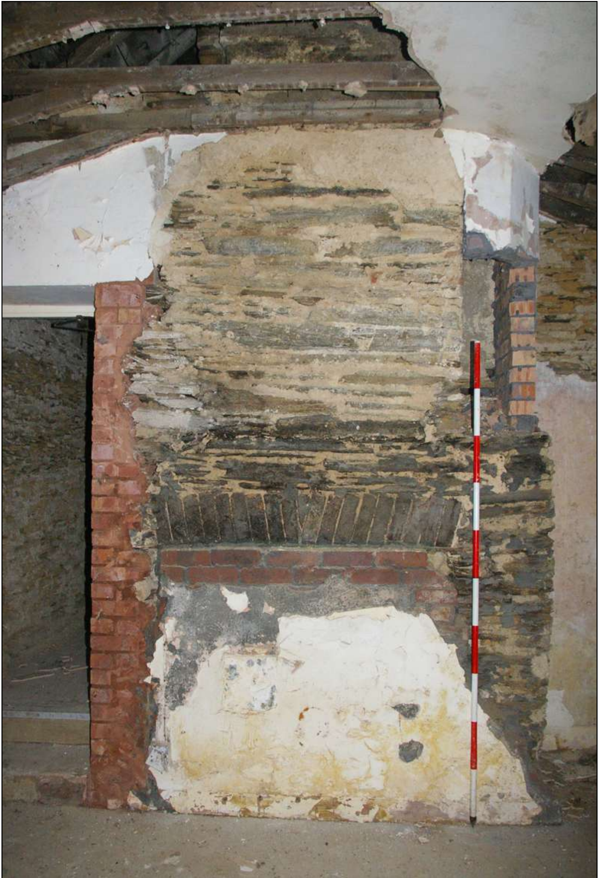
Figure 15: The stack in R3 in 2015, showing the blocked fireplace with segmental arch, the rebuilt upper stack with dressed stonework, and the forced doorway to the left; viewed from the west (scale 2m).
