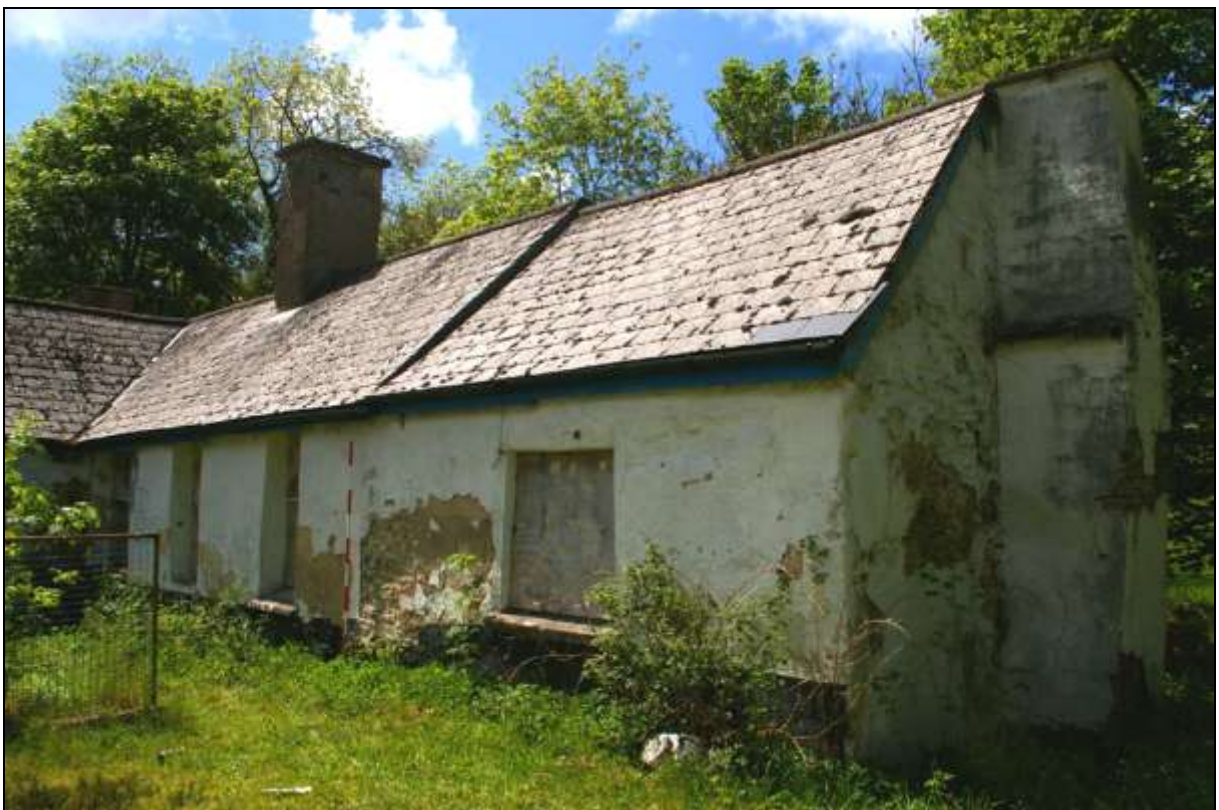
Figure 9: The eastern end of the south-facing elevation of the main range in 2012, viewed from the south-east (scale 2m).
