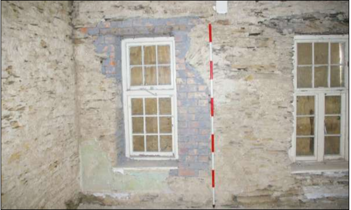
Figure 13: The south wall of R2 in 2015, showing the blocked round-headed arched doorway with forced window; viewed from the north (scale 2m).
