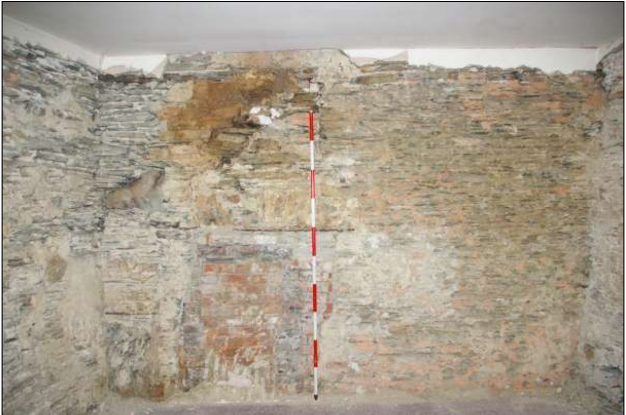
Figure 12: East wall of R1 in 2015, showing the thin timber lacing (top) and the blocked fireplaces and disturbed flue stonework; viewed from the west (scale 2m).
