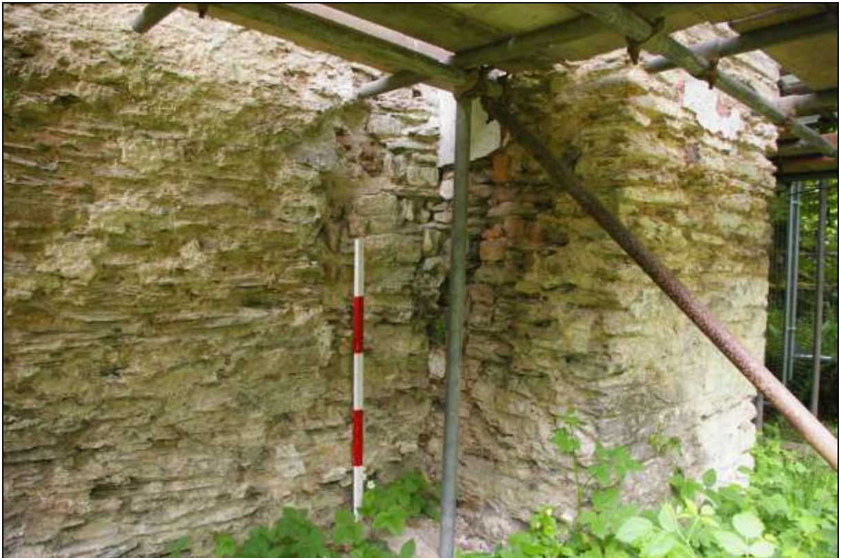
Figure 8: View of the disturbed stonework next to the eastern chimney stack (scale 1m).
