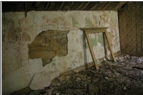
Figure 64: View of the plastered walls within Room I of Section 3 and the surviving but loose timber fireplace surround; from the north-west.
