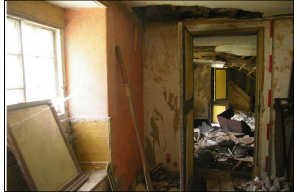
Figure 145: Door to Room G and window in Room H, Section 3; from the south, south-east.
