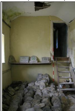
Figure 88: The south wall of Room M, the two storey solid partition wall between Sections 1-3 and 4; from the north.
