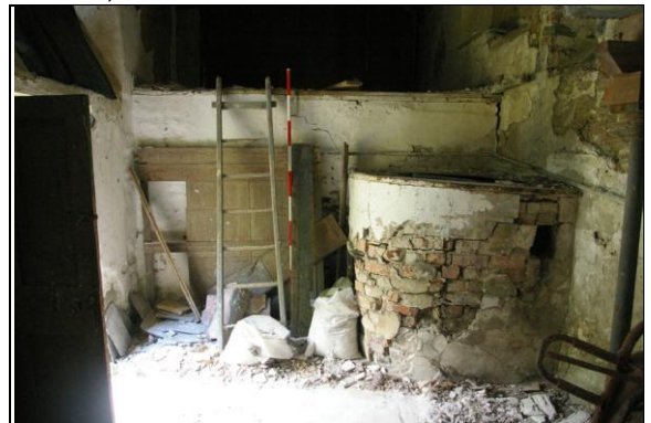
Figure 131: The stone partition wall of first floor height only, between Room E, Section 2 and Room H, Section 3, with copper built up against it; from the south.
