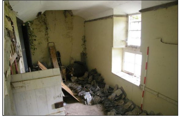
Figure 89: View along the east wall of Room M, Section 4; from the south-west.
