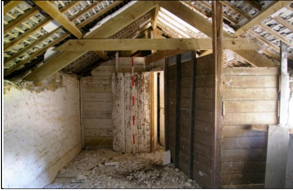
Figure 109: The early boarded partitions which form the rooms on the first floor in Section 1; from the south.
