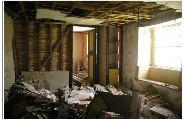
Figure 146: The lathe and plaster partition wall between Room G and H, in Section 3; from the north, north-east.
