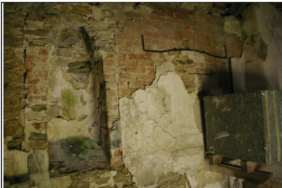
Figure 136: View of the in-wall fireplace and the forced brick fireplace, both in the east wall of Room E, Section 2; from the west, north-west.
