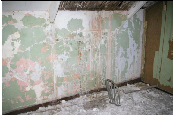
Figure 70: The plastered and painted east wall of Room J, Section 3; from the north-west.
