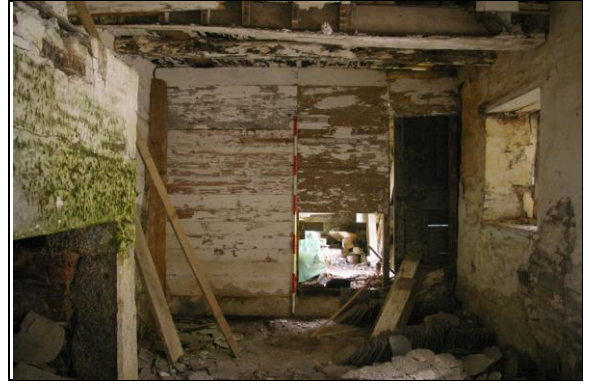
Figure 121: The boarded partition between Room D and Room E, in Section 2; from the north.
