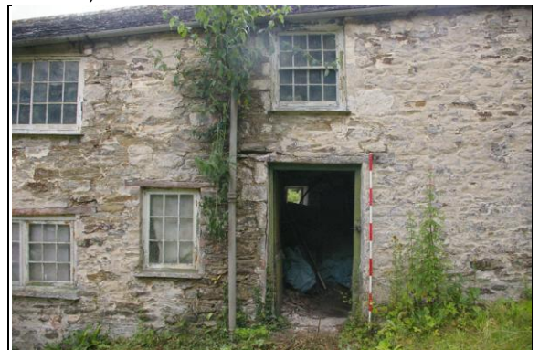
Figure 52: Some of the openings in Sections 1 and 2, showing original stone quoins and patching with brick as openings have been reduced or forced; from the west.
