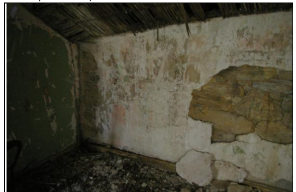
Figure 68: View to the north-east corner of Room I, Section 3; from the south-west.
