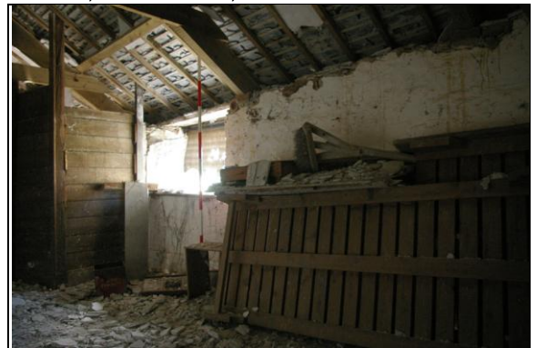
Figure 107: View along the east wall of Room B, Section 1, with window; from the south-west.
