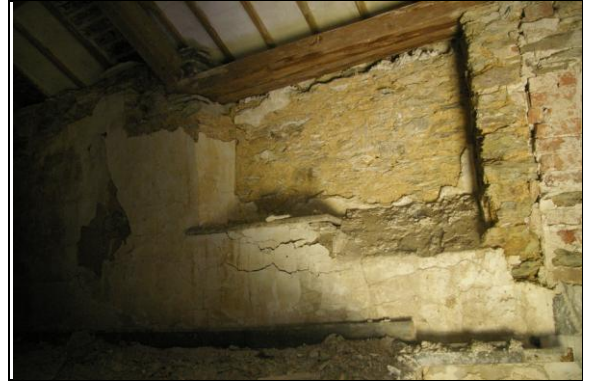
Figure 137: The blocked window, at first floor level in the east wall, Room E, Section 2; from the south-west.
