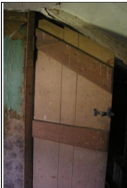
Figure 80: The door between Rooms J and K, showing it has been cut down to fit with the later inserted partition; from the north.
