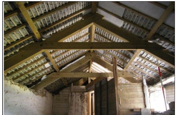
Figure 108: View of the modern timber framed A-frames in the roof, Section 1; from the south.
