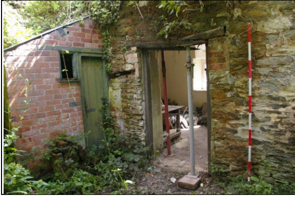
Figure 37: The various blocked and forced openings in the west elevation of Section 4; from the south-west.
