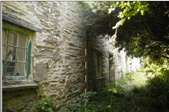
Figure 39: View of the significantly disturbed area of stonework between Section 3 and Section 4, on the west elevation; from the north-west.
