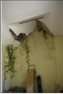
Figure 85: View of the odd space left the demolished stack in Room M, Section 4; from the south-east.
