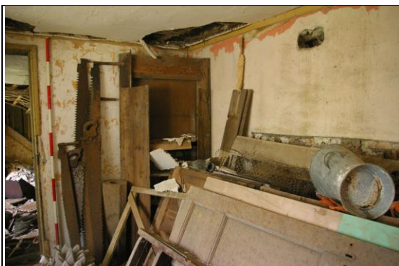
Figure 144: The east wall, with the scar of the fireplace showing behind the contents of the room; from the south-west.
