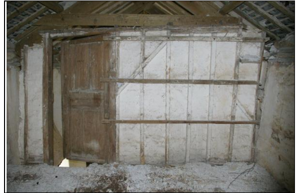
Figure 114: The north wall of Room C, Section 1, a timber and lathe and plaster partition, with panelled door from the south.
