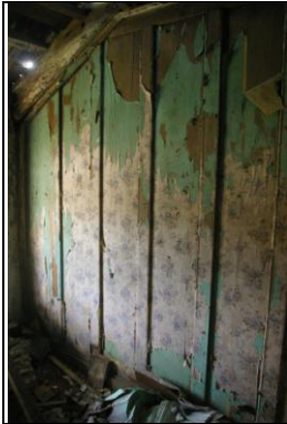
Figure 78: One of the later timber partitions which forms Rooms J and K; from the north-west.
