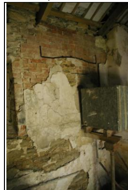
Figure 139: The fireplace forced in the east wall of Section 2, at first floor level and rebuilt in brick; from the north-west.
