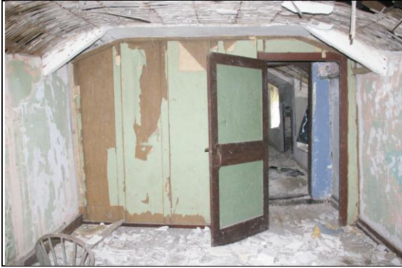
Figure 69: View of the later plank and board partition wall which forms Room J, in Section 3; from the north.
