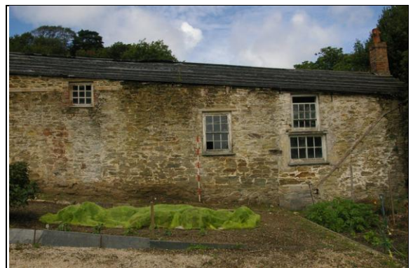
Figure 28: The east elevation of Section 4, showing infill and blocked openings; from the east.
