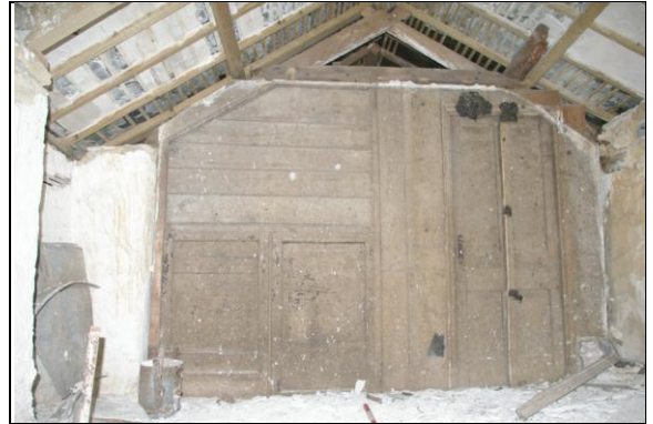
Figure 138: The boarded partition/lathe and plaster cupboard space, between Room E, Section 2 and Room I, Section 3, on the first floor; from the south.
