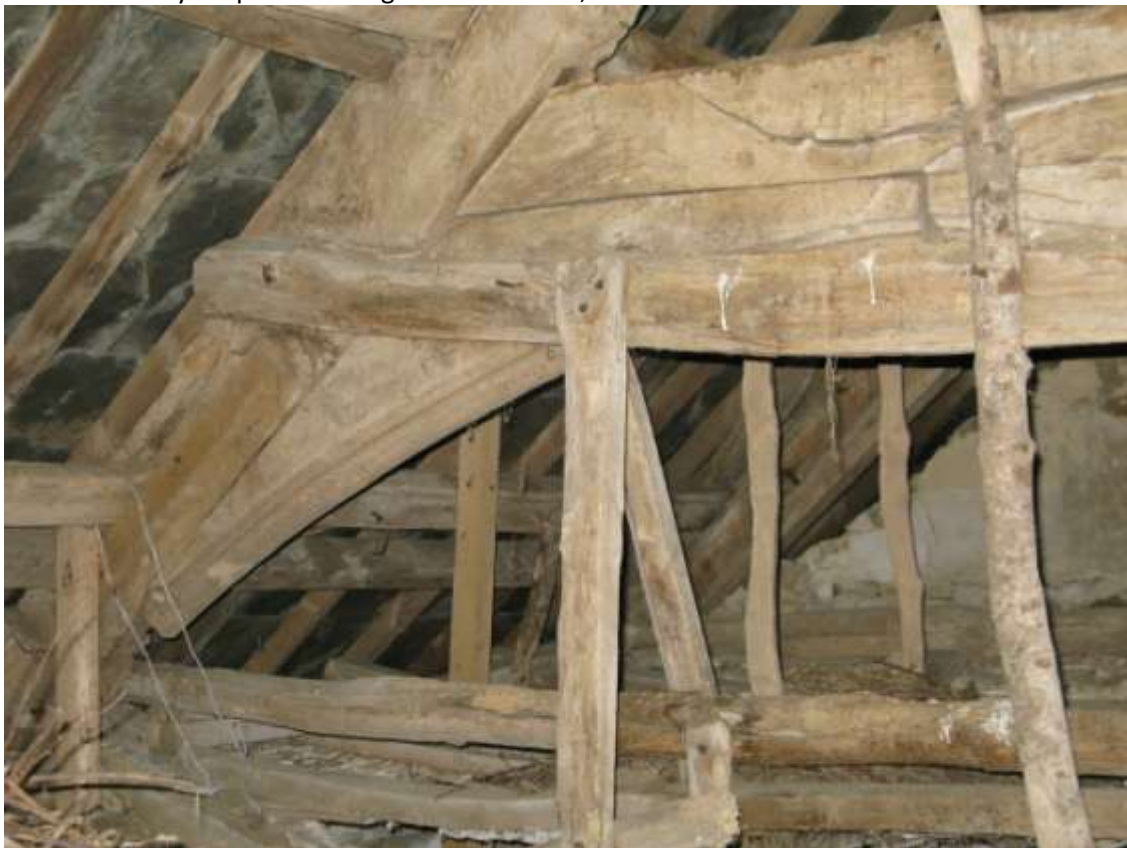
Detail of the west side of the arch-braced truss; from the south.
