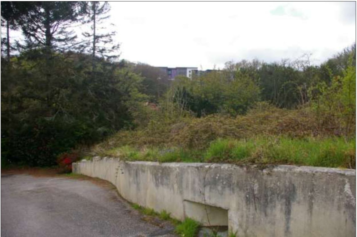
The concrete wall with drainage that has been installed to retain the made ground; from the north-east.
