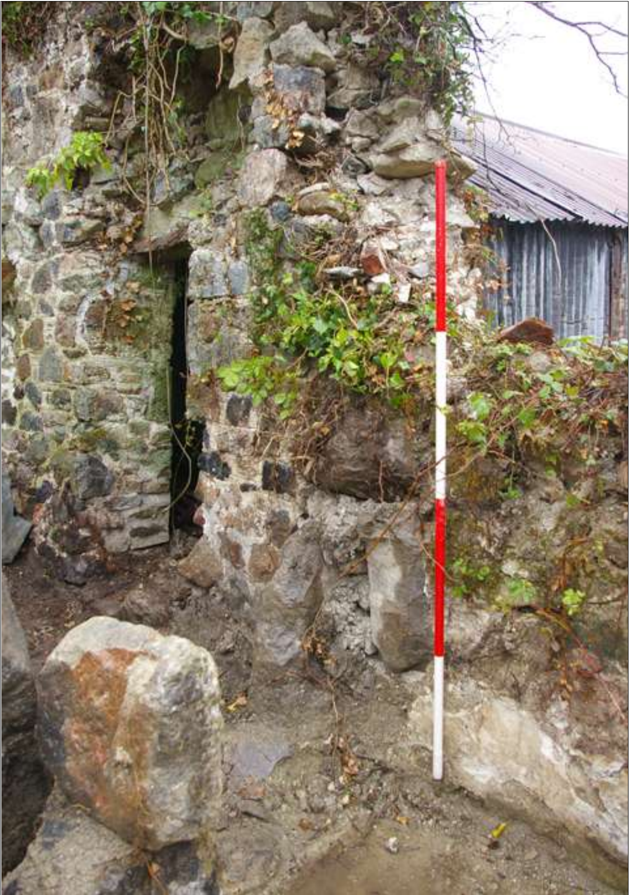
The north-eastern corner of the cottage; viewed from the south-west (scale 2m).
