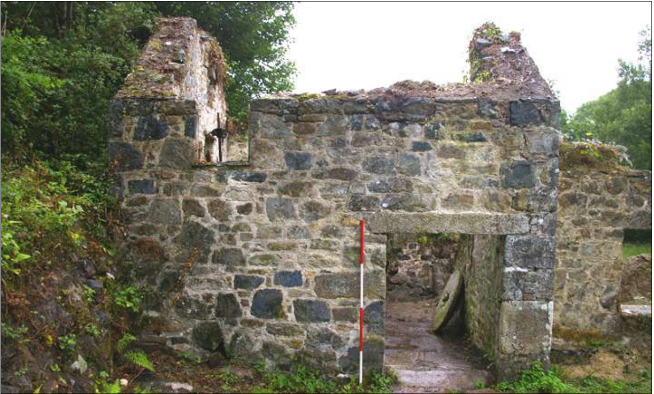
The western elevation of the mill; viewed from the west (scale 2m).
