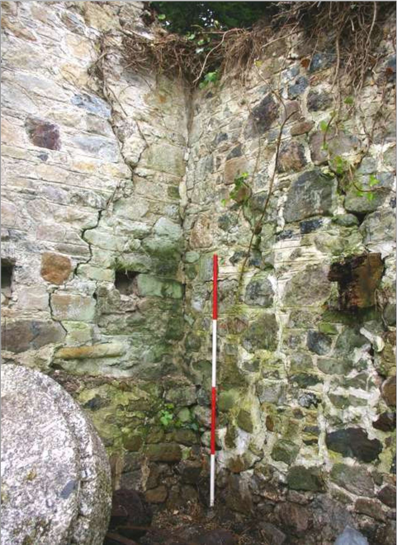
The north-east corner of the Mill, showing structural cracks; viewed from the south-west (scale 2m).
