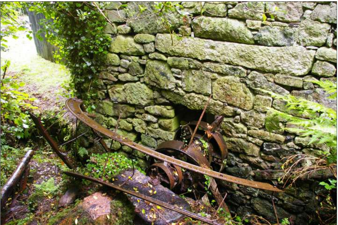
The wheelpit, showing the collapsed wheel in situ ; viewed from the north.
