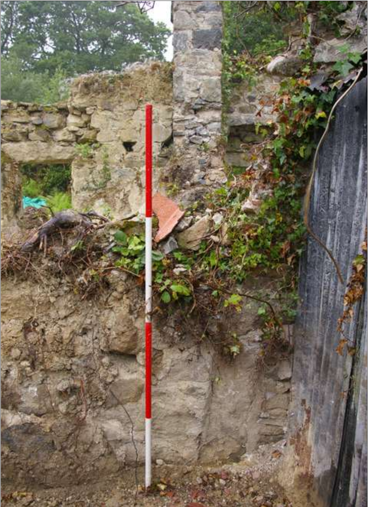
The northern end of the east wall of the cottage; viewed from the east (scale 2m).
