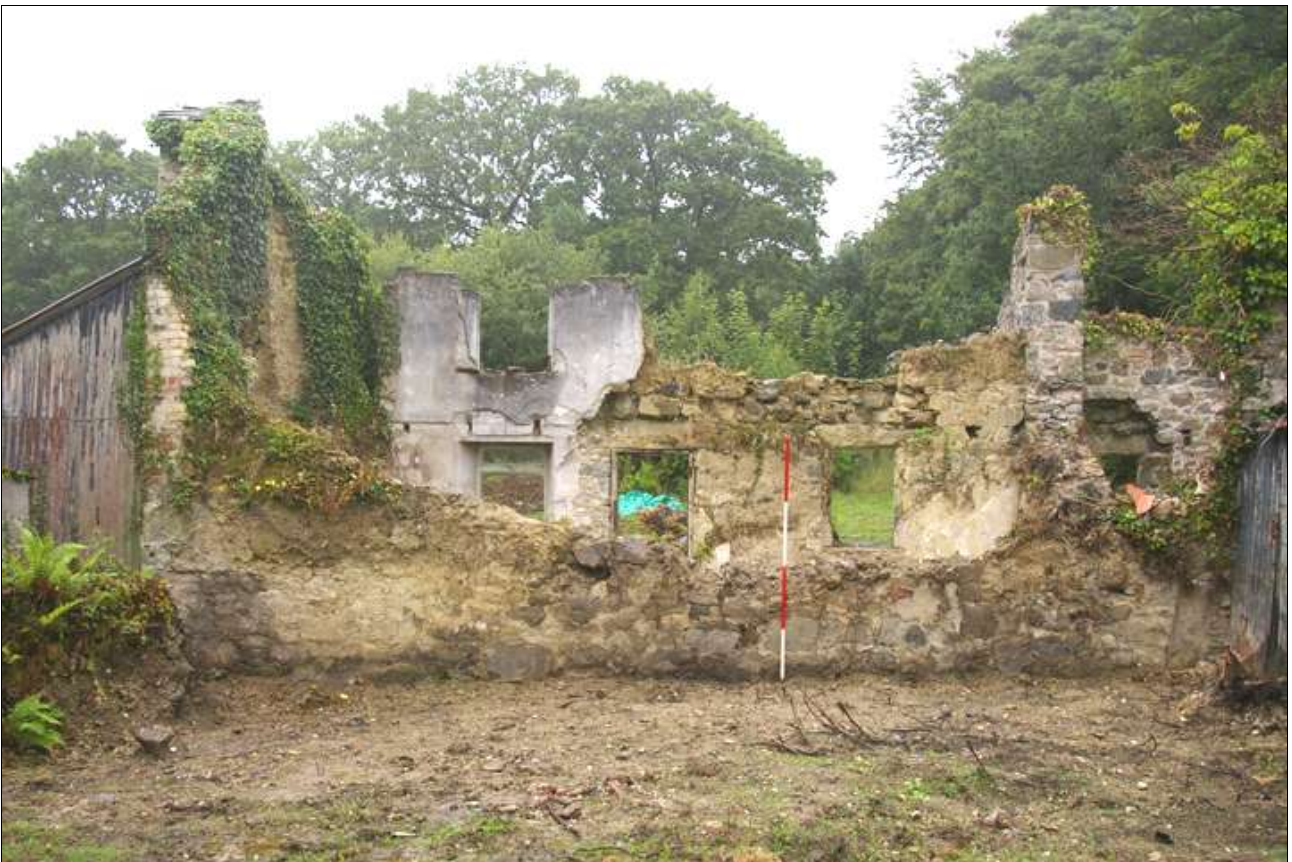
The remains of the east elevation of the cottage; viewed from the east (scale 2m).
