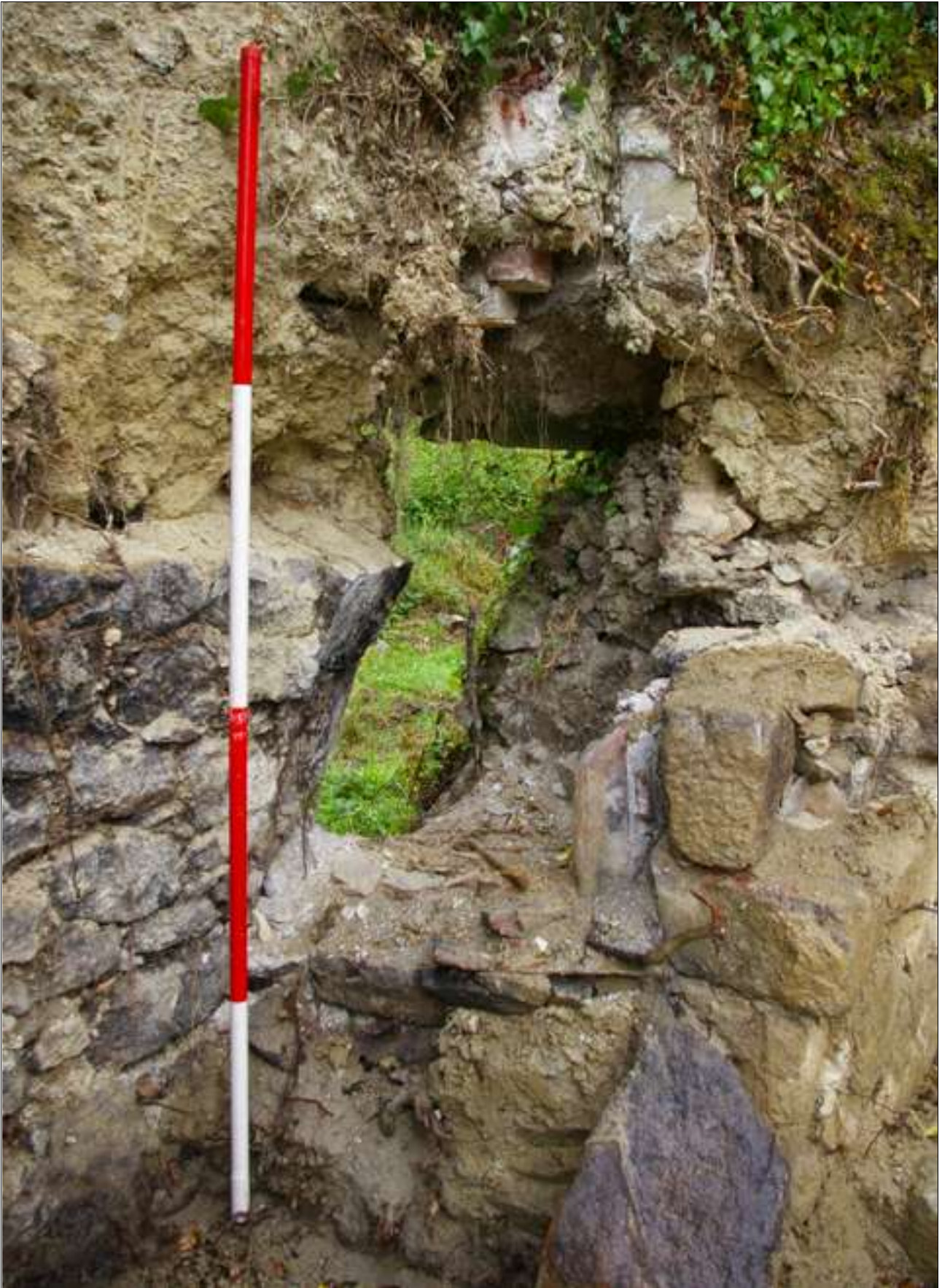
As above, showing the breach through to the bread oven, with elements of the cloam oven in situ (scale 2m).
