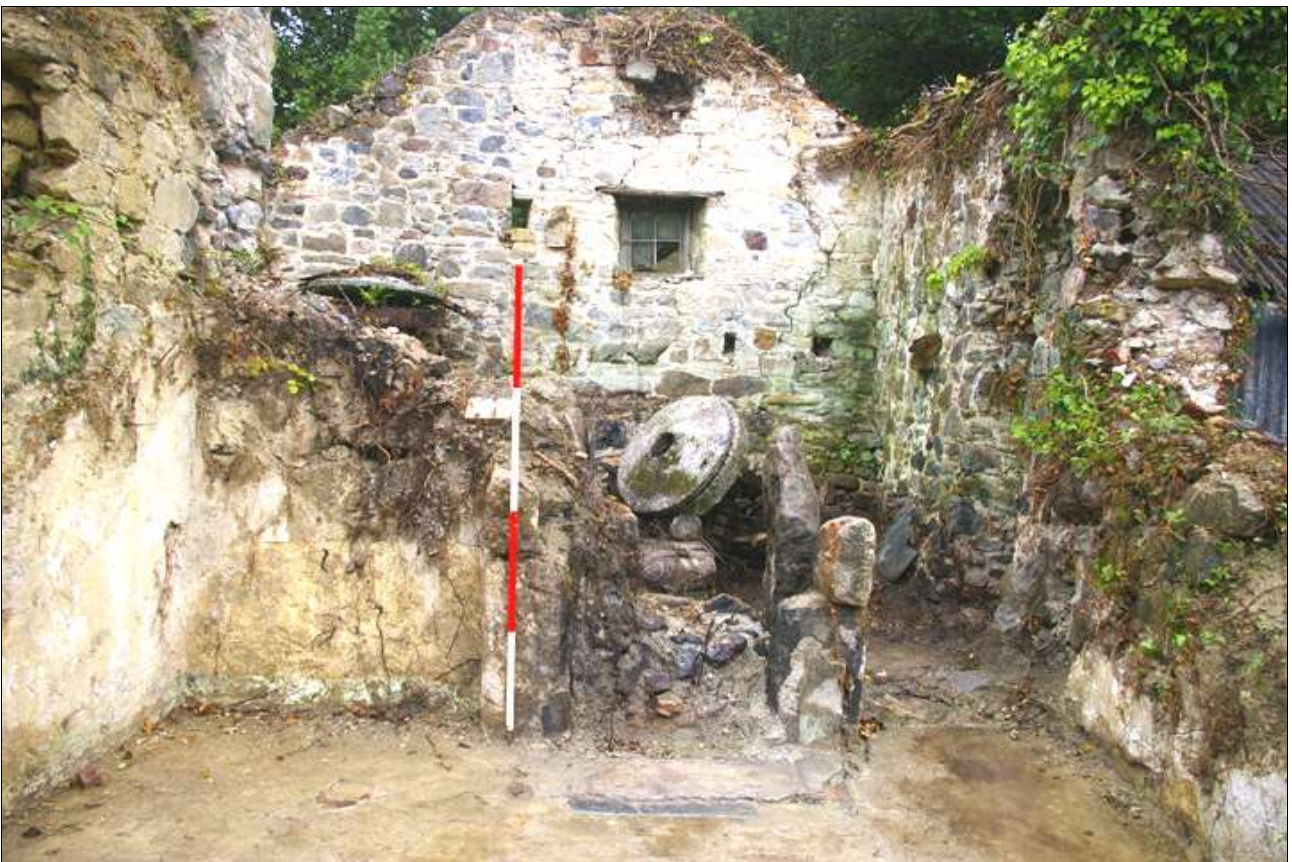
The internal elevation of the north wall of the cottage; viewed from the south (scale 2m).
