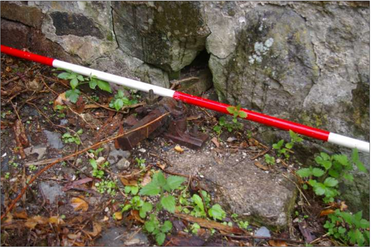
The upstream layshaft protruding from the front (west) wall of the mill; viewed from the south-west (scale 2m).
