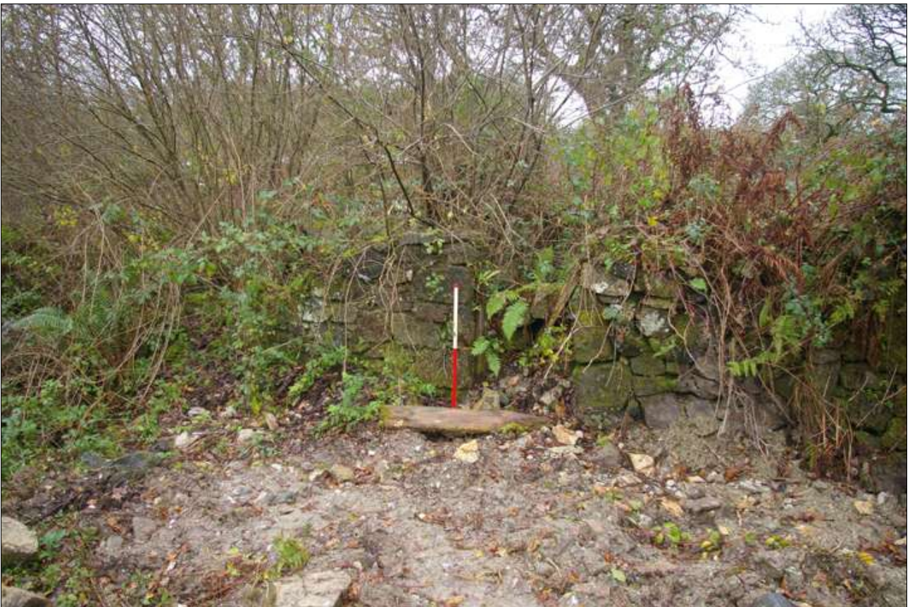
The eastern elevation of the collapsed building to the west of the mill and cottage; viewed from the north-east (scale 1m).
