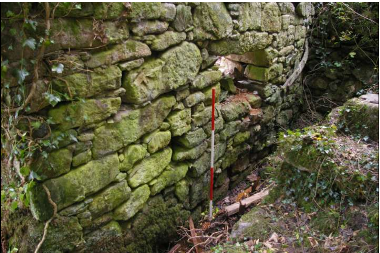
The exterior of the north wall of the mill, following the removal of the wheel; viewed from the north-east (scale 2m).
