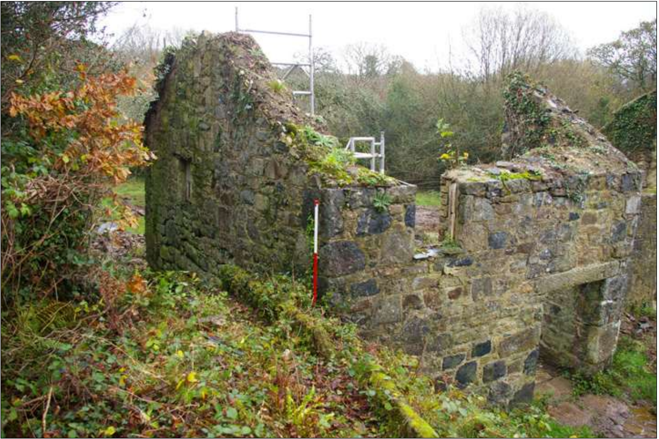
The mill building viewed from the top of the leat; viewed from the north-east (scale 1m).
