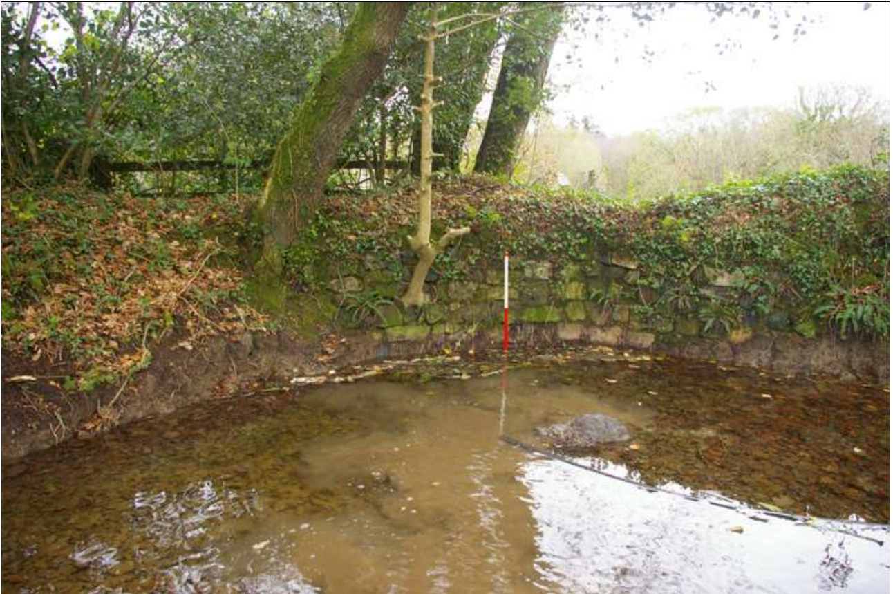
As above, showing the stone walling (rebuild?) where the culvert leading to the leat is located; viewed from the north-west (scale 1m).
