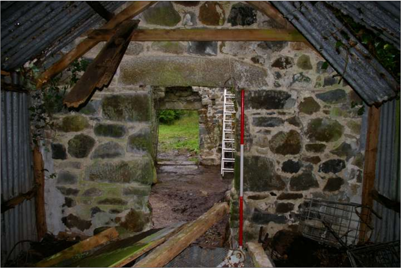
The door in the east elevation of the mill; viewed from the east (scale 2m).
