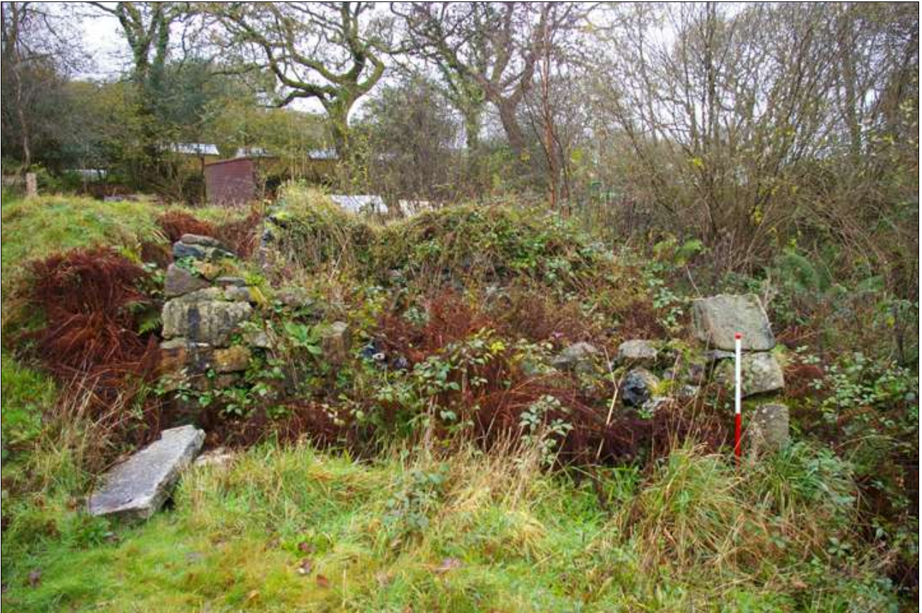
The east elevation of the collapsed building south-west of the mill and cottage; viewed from the east (scale 1m).
