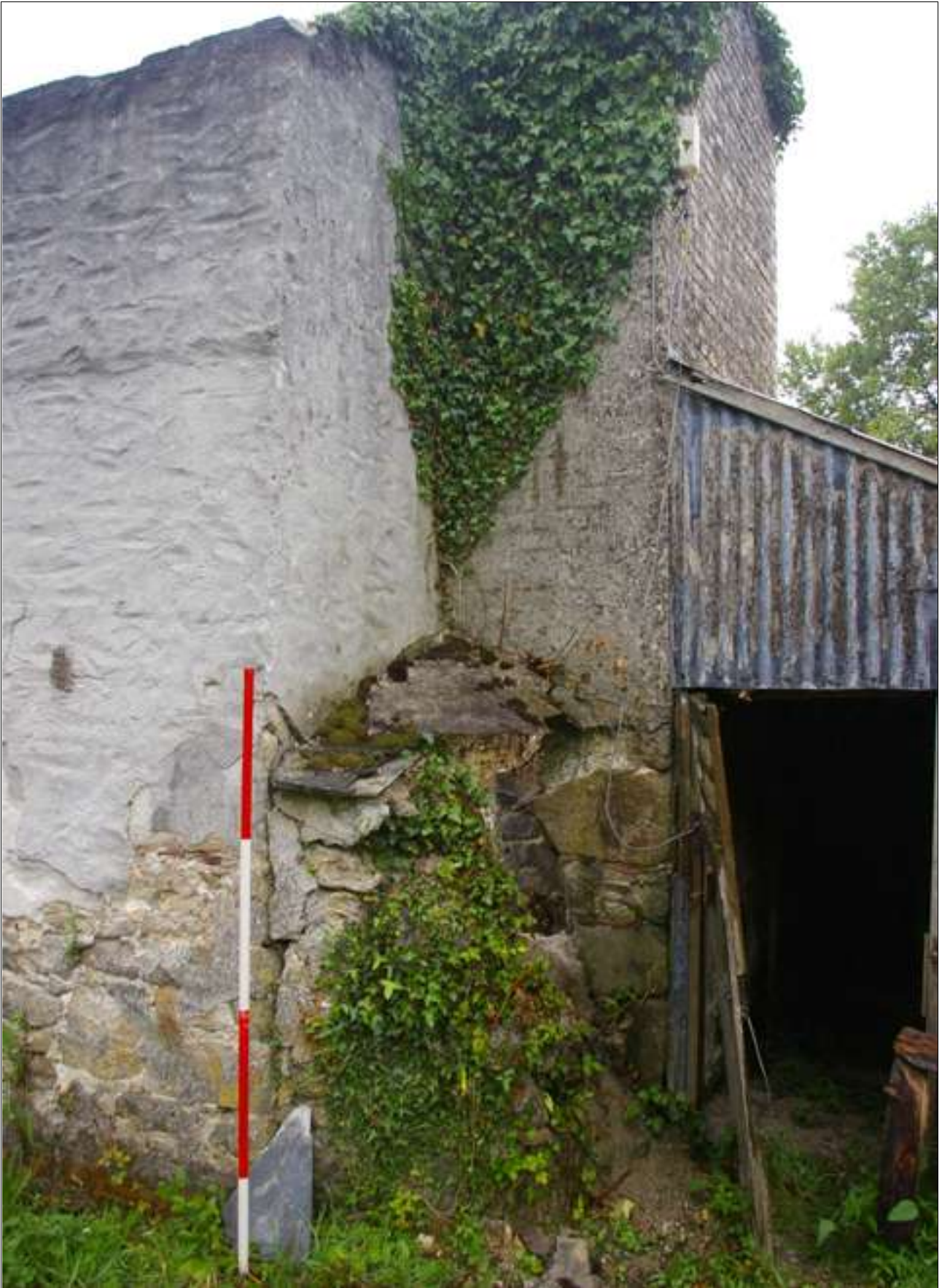
The bread oven in the angle of the southern chimney stack; viewed from the west (scale 2m).
