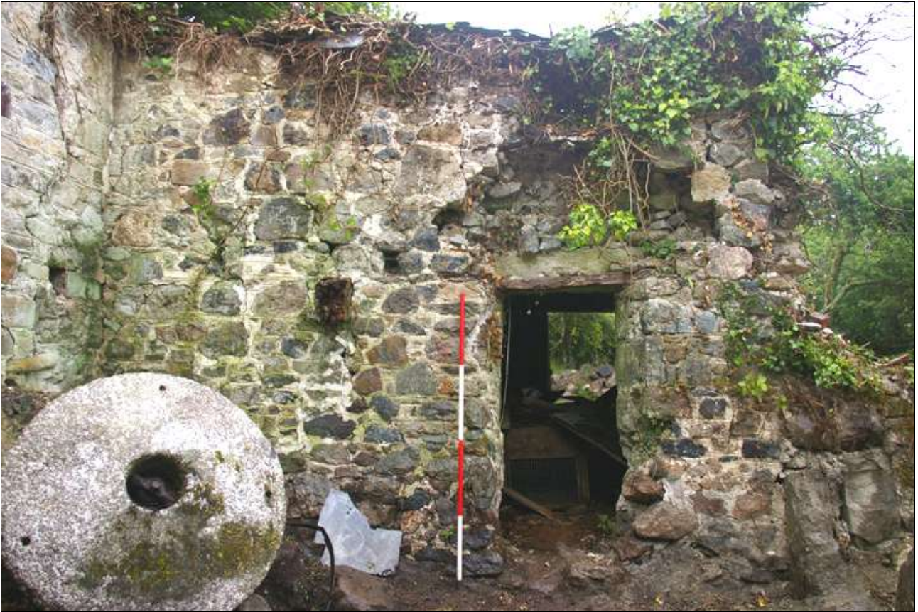
The east wall of the Mill; viewed from the west (scale 2m).
