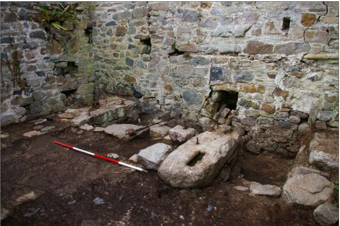
The floor of the mill following the removal of the mill machinery; viewed from the south-east (scale 2m).
