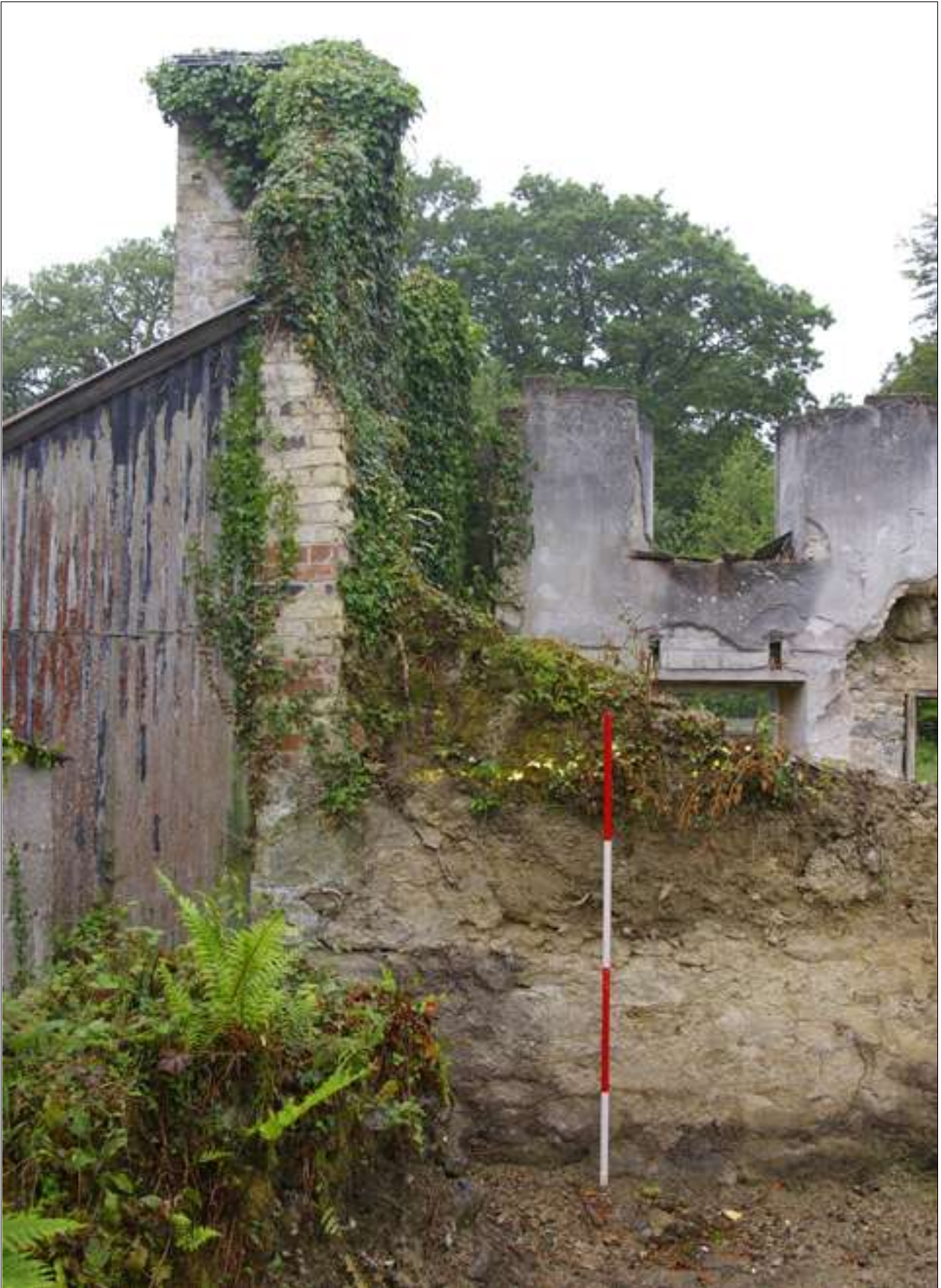
The southern end of the east wall of the cottage; viewed from the east (scale 2m).
