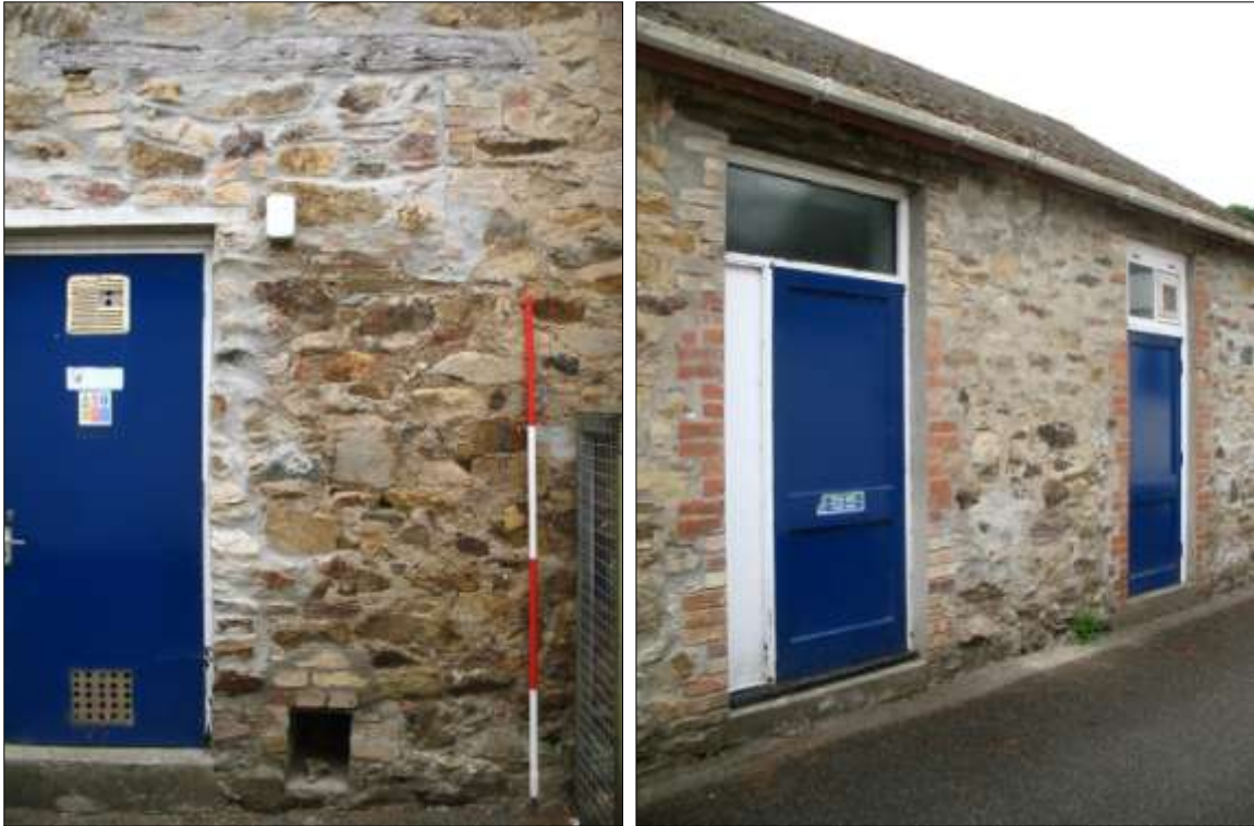
LEFT: HIGH BLOCKED OPENING AND FORCED DOORWAY (SCALE 2M).
