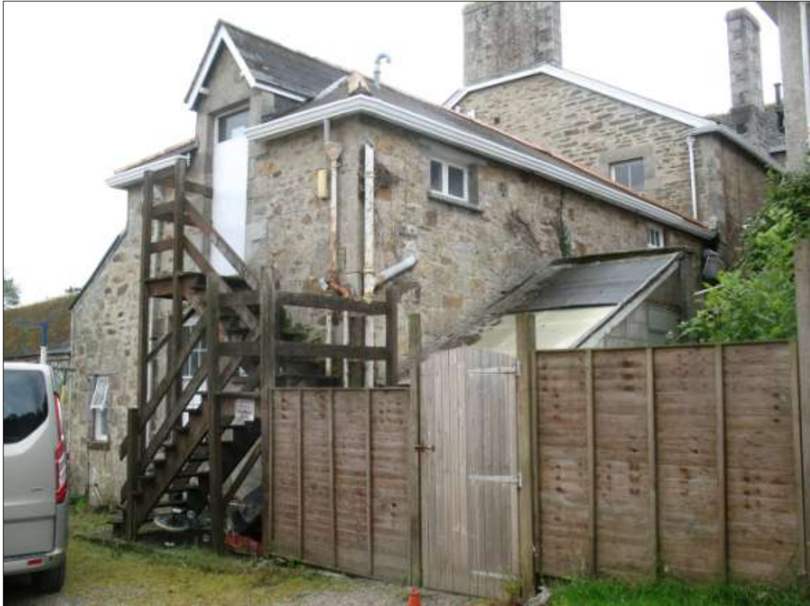
AS ABOVE, VIEWED FROM THE NORTH-WEST. NOTE THE CONTRASTING STONEMWORK OF THE BACKBLOCK.
