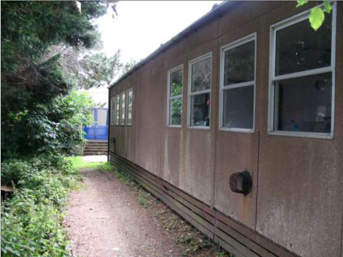
THE NORTH ELEVATION OF TC#2, WITH THE DOORS OF TC#1 TO THE LEFT; VIEWED FROM THE WEST.
