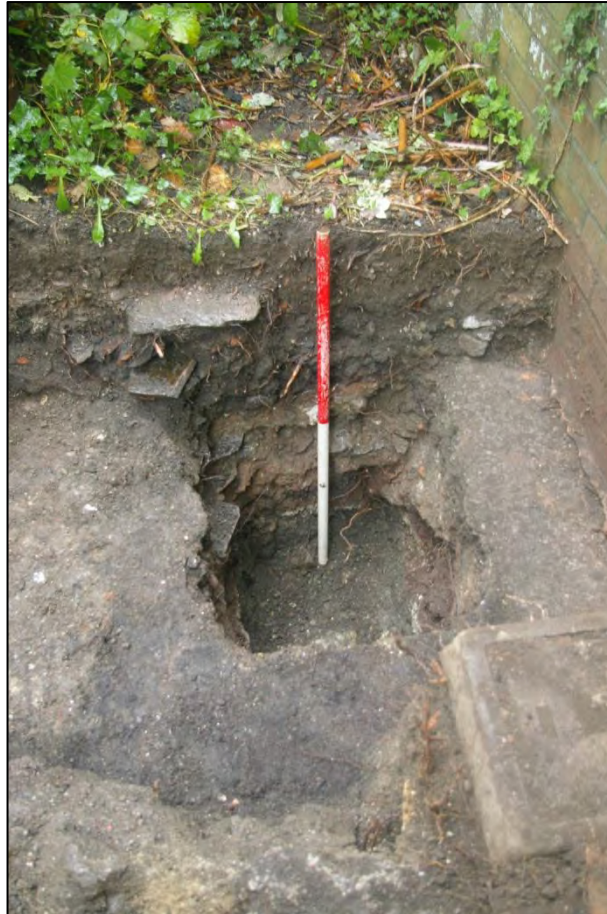
TEST PIT 2, WALL FOOTINGS {203} MID-EXCAVATION; VIEWED FROM THE SOUTH-WEST (0.30M & 1M SCALES).
