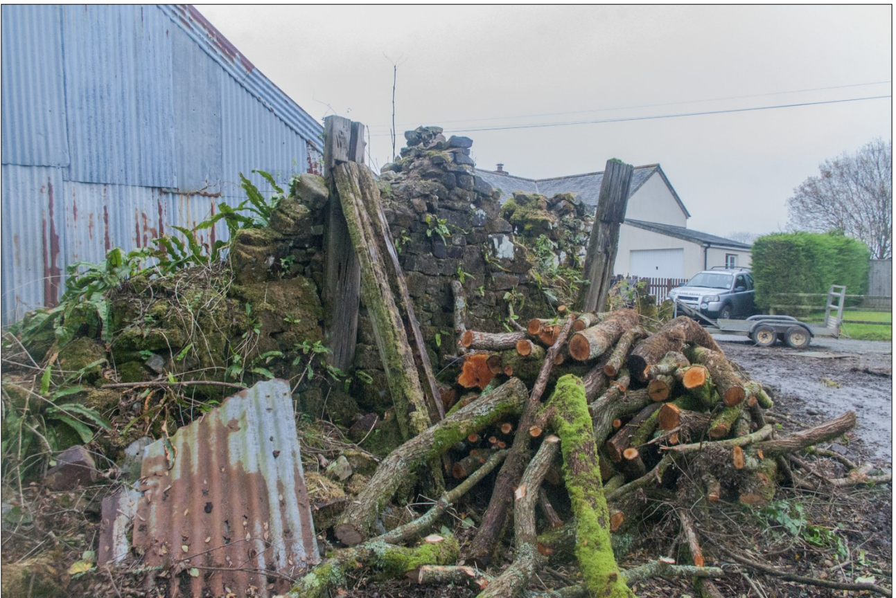
The timber posts braced against the ruined west elevation; from the west.
