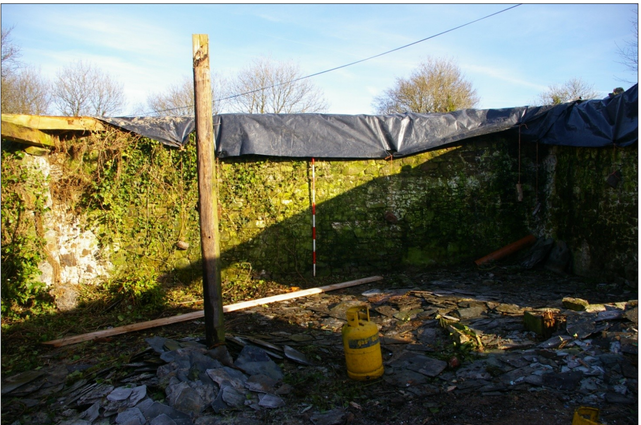
The internal face of the east wall of the warehouse; from the west (scale 2m).
