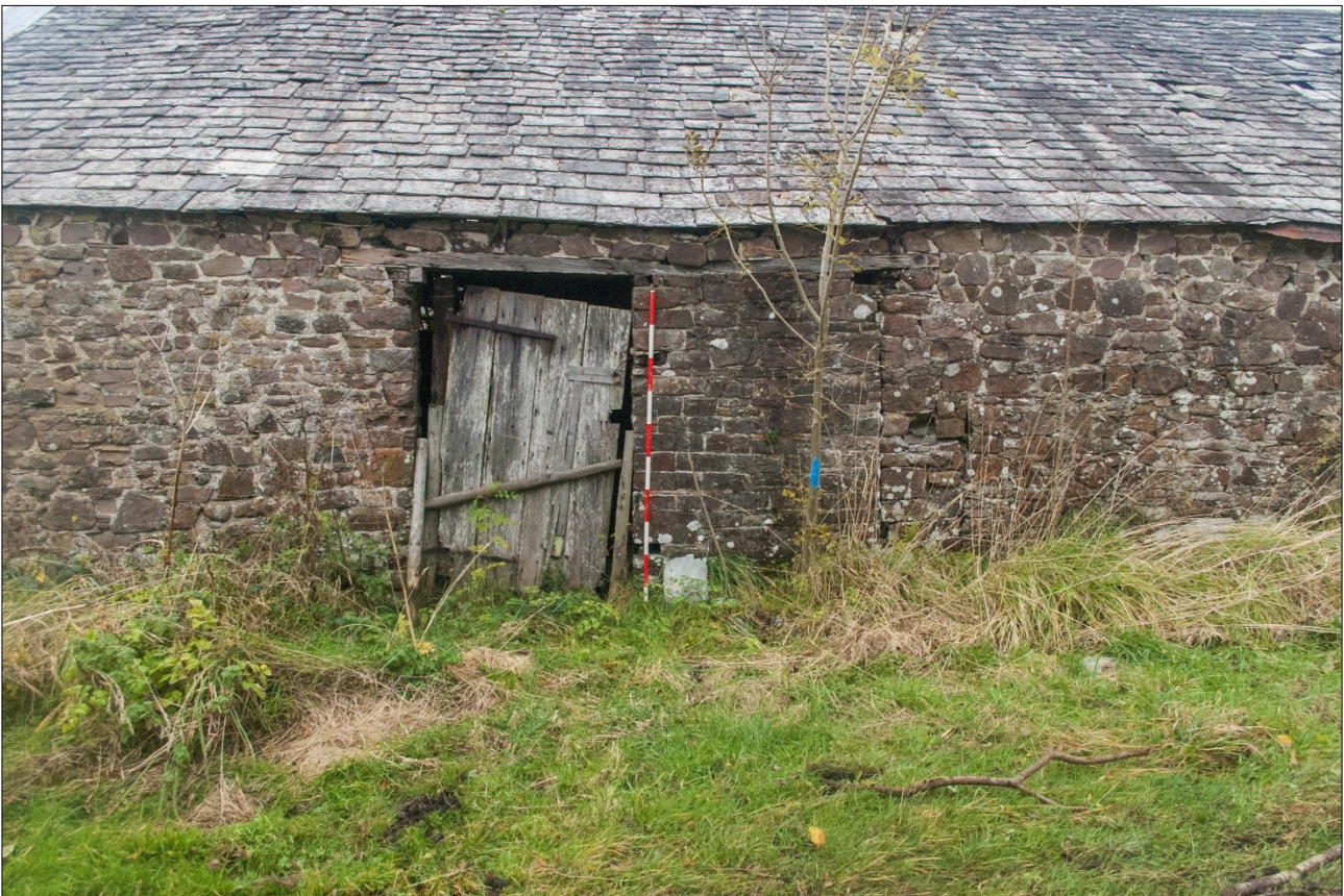
The west doorway in the south elevation showing the partly-blocked opening; from the south (scale 2m).
