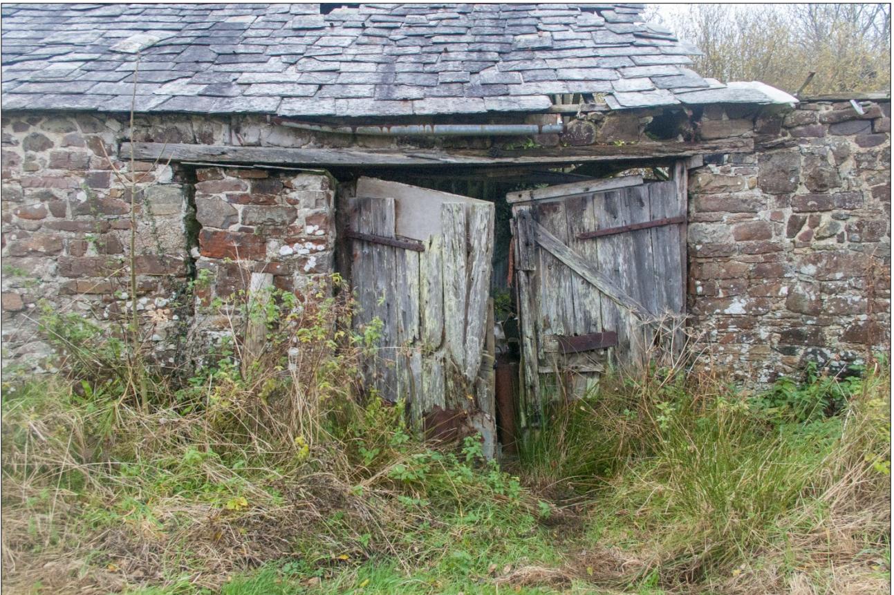
Double doors to the east end of the south elevation; from the south.
