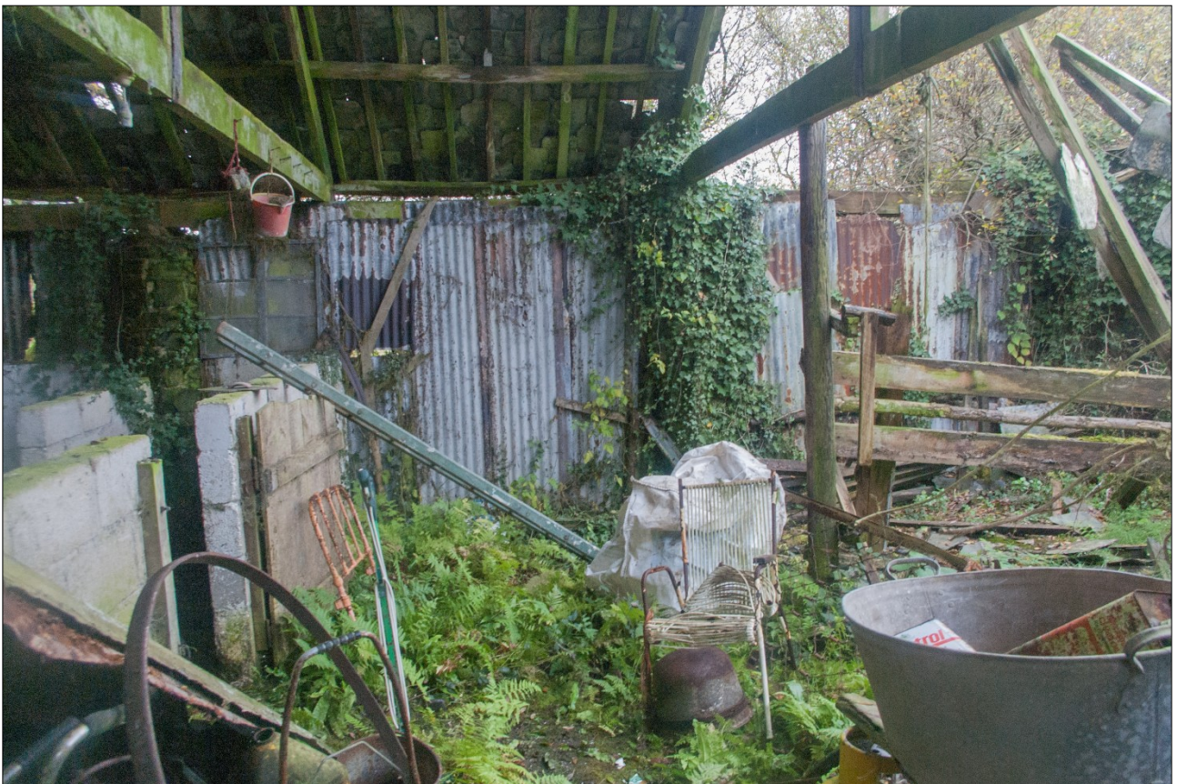
View into the interior of the warehouse, from the double doors at the east end of the south elevation; from the south.
