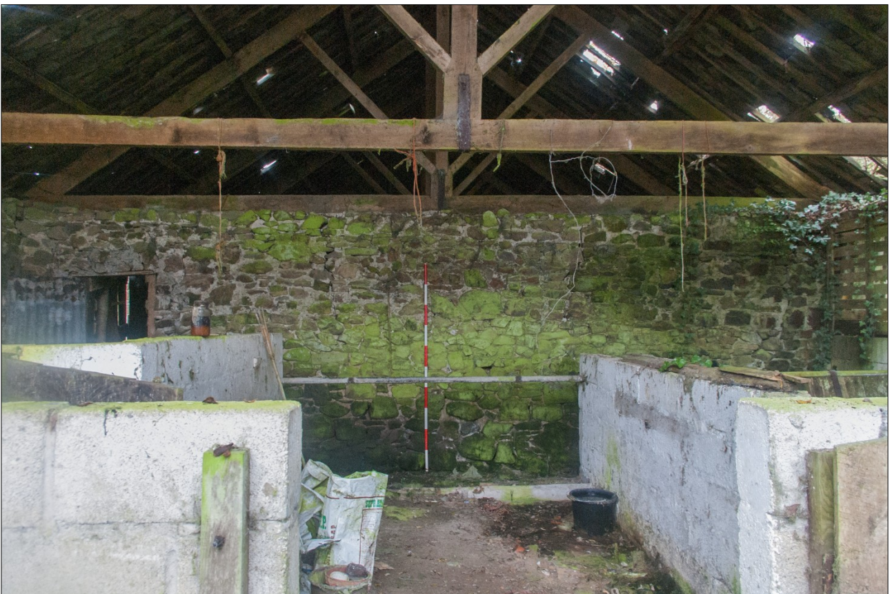
View of the central partition wall and the surviving central portion of the roof; from the east (scale 2m).
