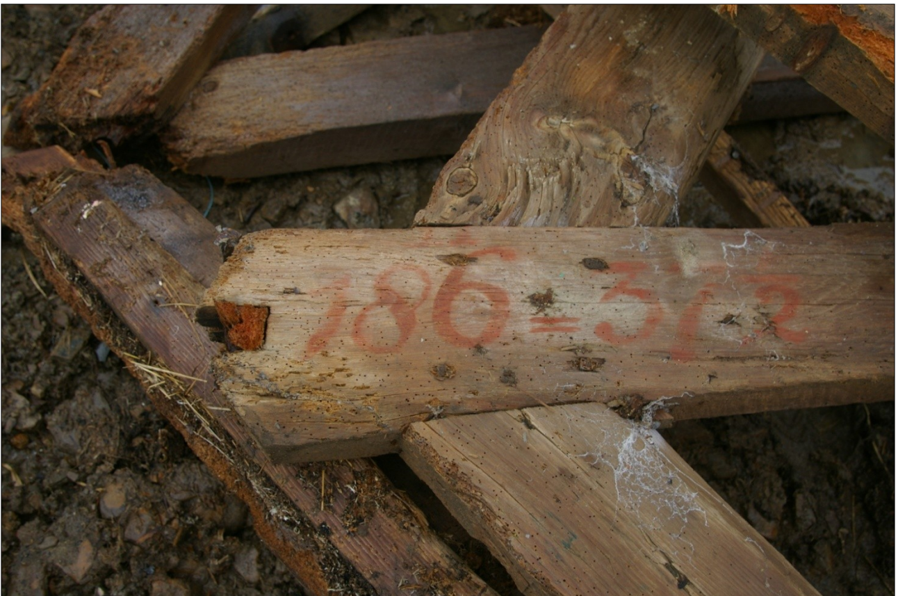
Detailed view of kingpost at apex, showing pegs, bolts, and graffiti; from the south.
