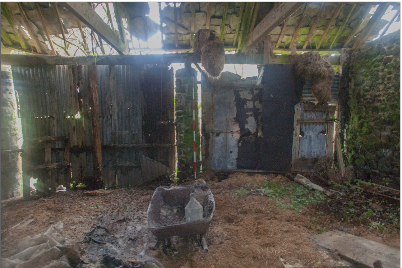
The north wall of the warehouse at the western end, showing corrugated iron sheeting infill; from the south (scale 2m).
