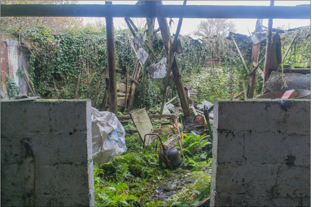
View of the east end of the warehouse where the hipped roof has failed; from the west.
