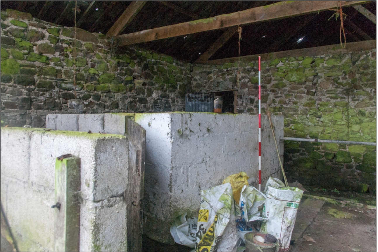
View of the concrete animal pens built in the middle of the warehouse, up against the east side of the partition wall; from the north-east (scale 2m).
