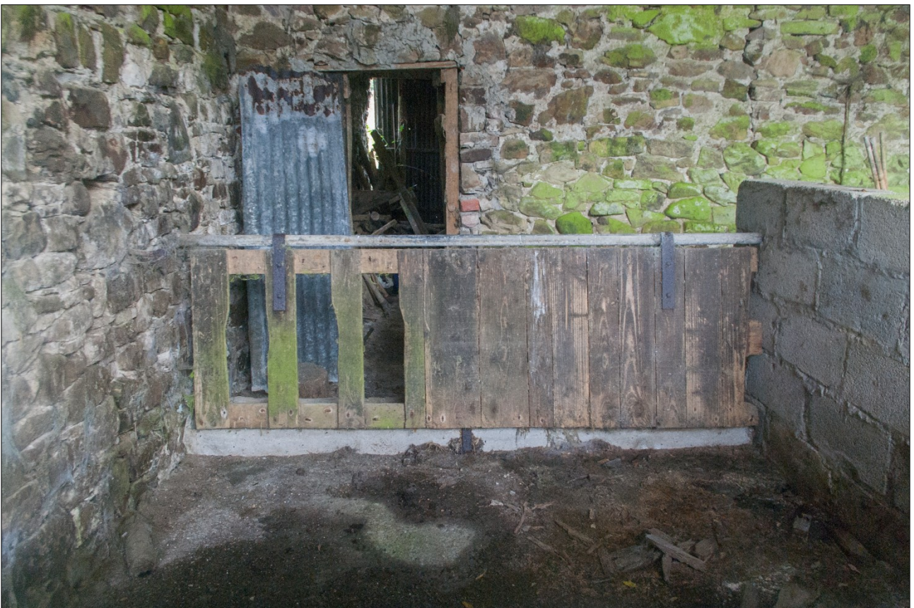
View of the forced doorway in the partition wall, leading to the western half of the warehouse; from the east.
