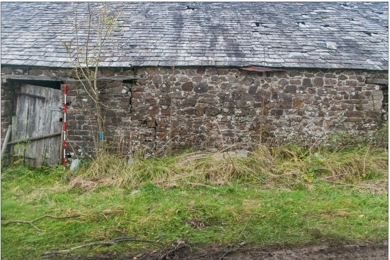
The central section of the south elevation, showing the different phases of stonework; from the south (scale 2m).
