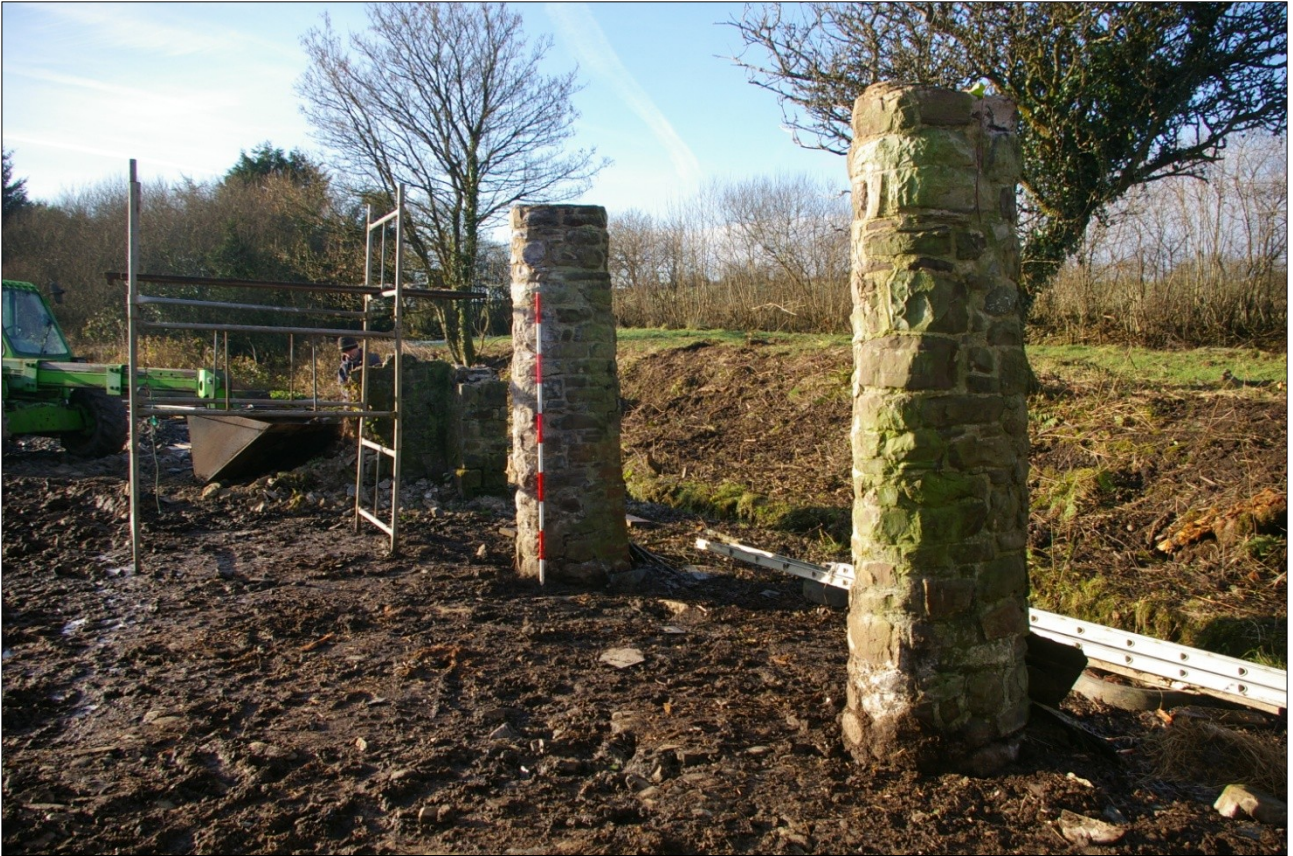
The stone pillars on the northern side of the warehouse; from the south-east (scale 2m).
