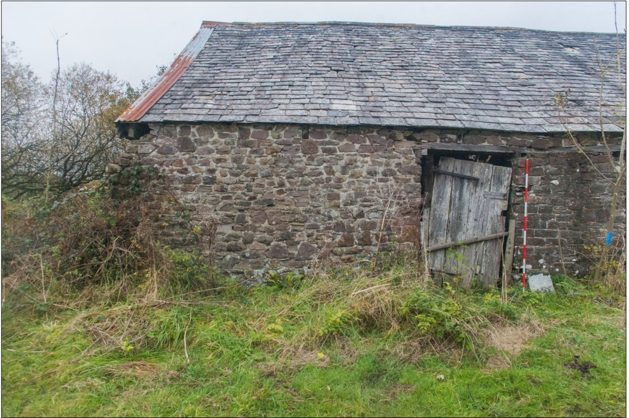
The west end of the south elevation showing the different phases of stonework; from the south (scale 2m).
