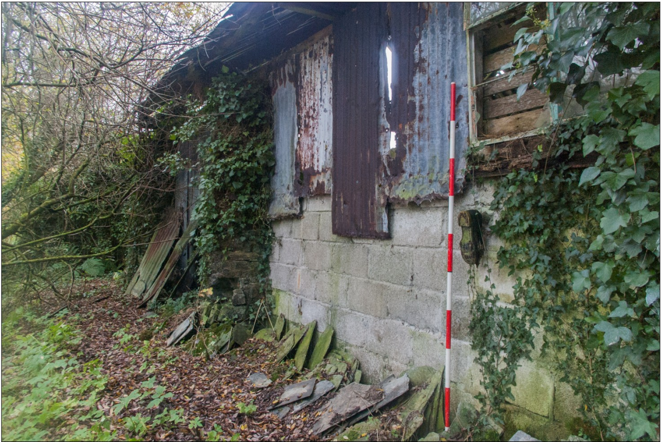
The east end of the north elevation, showing the infill concrete sections; from the north-west (scale 2m).
