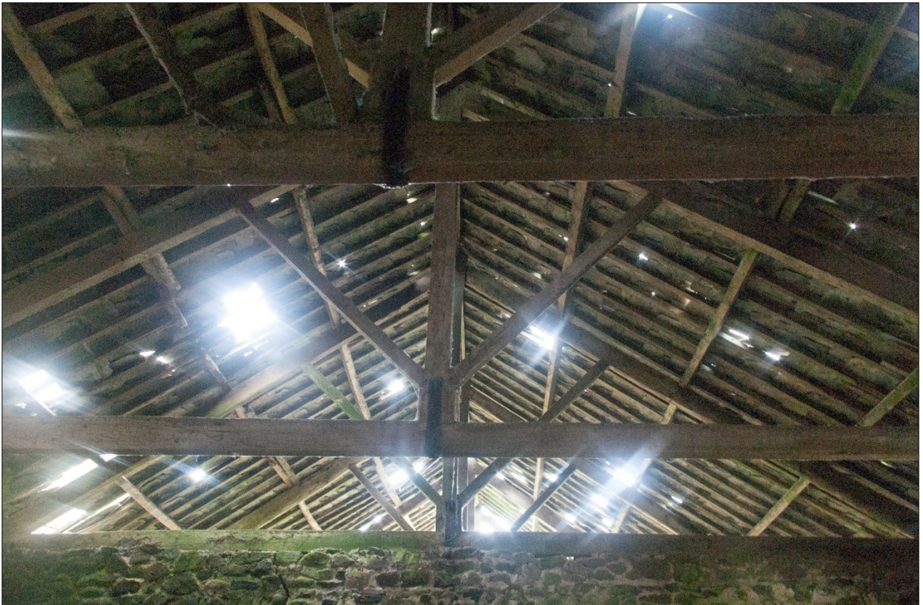
Detail of the roof trusses, showing three purlins to each pitch and the simple A-frame and king post trusses, with struts, bolted by straps, a mid or later 19 th century roof; from the west.
