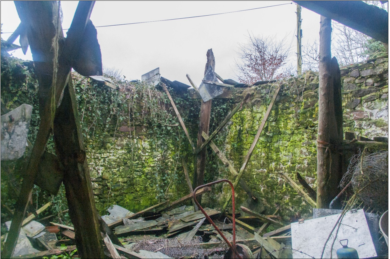
Detail of one of the hipped corners of the collapsed east end of the roof over the warehouse; from the north-west.
