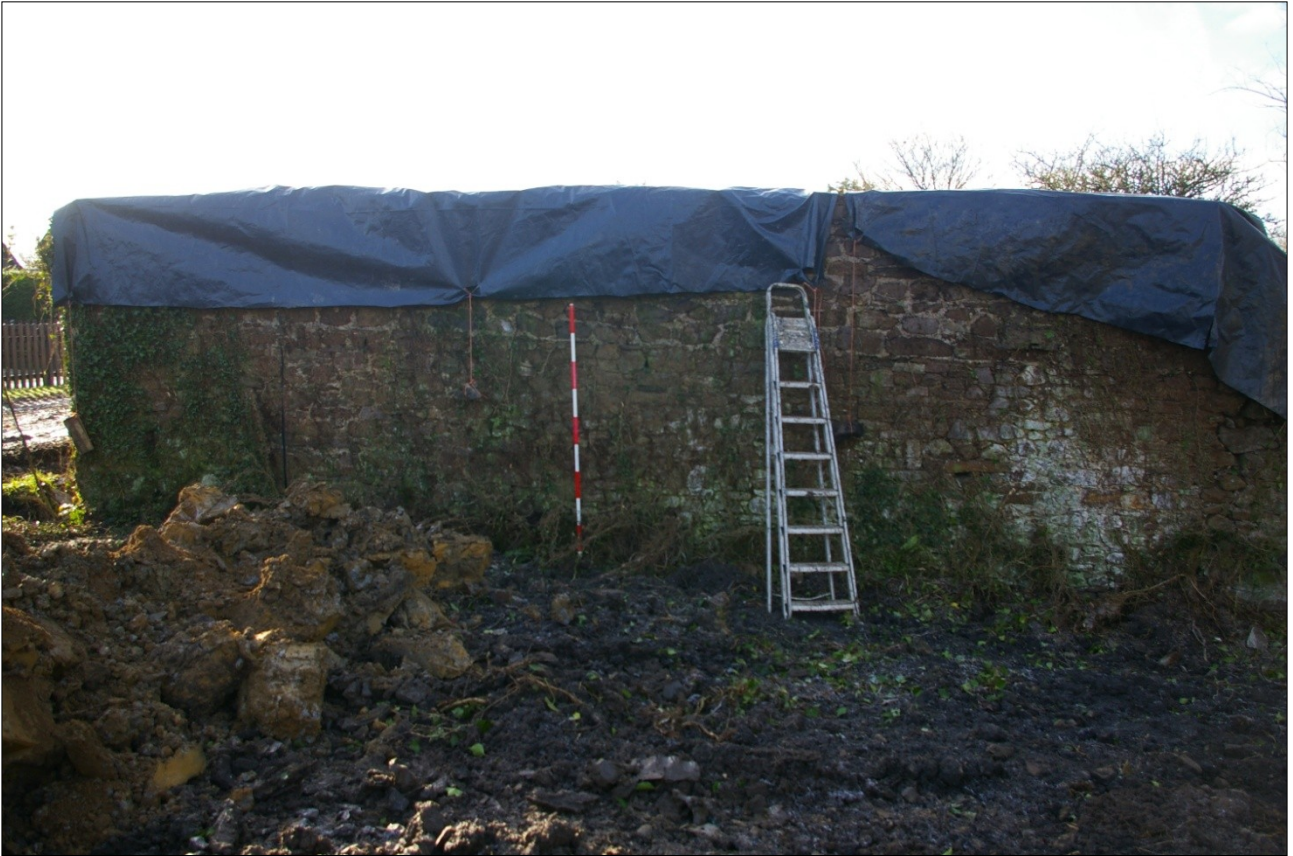
The external face of the east wall of the warehouse; from the east (scale 2m).
