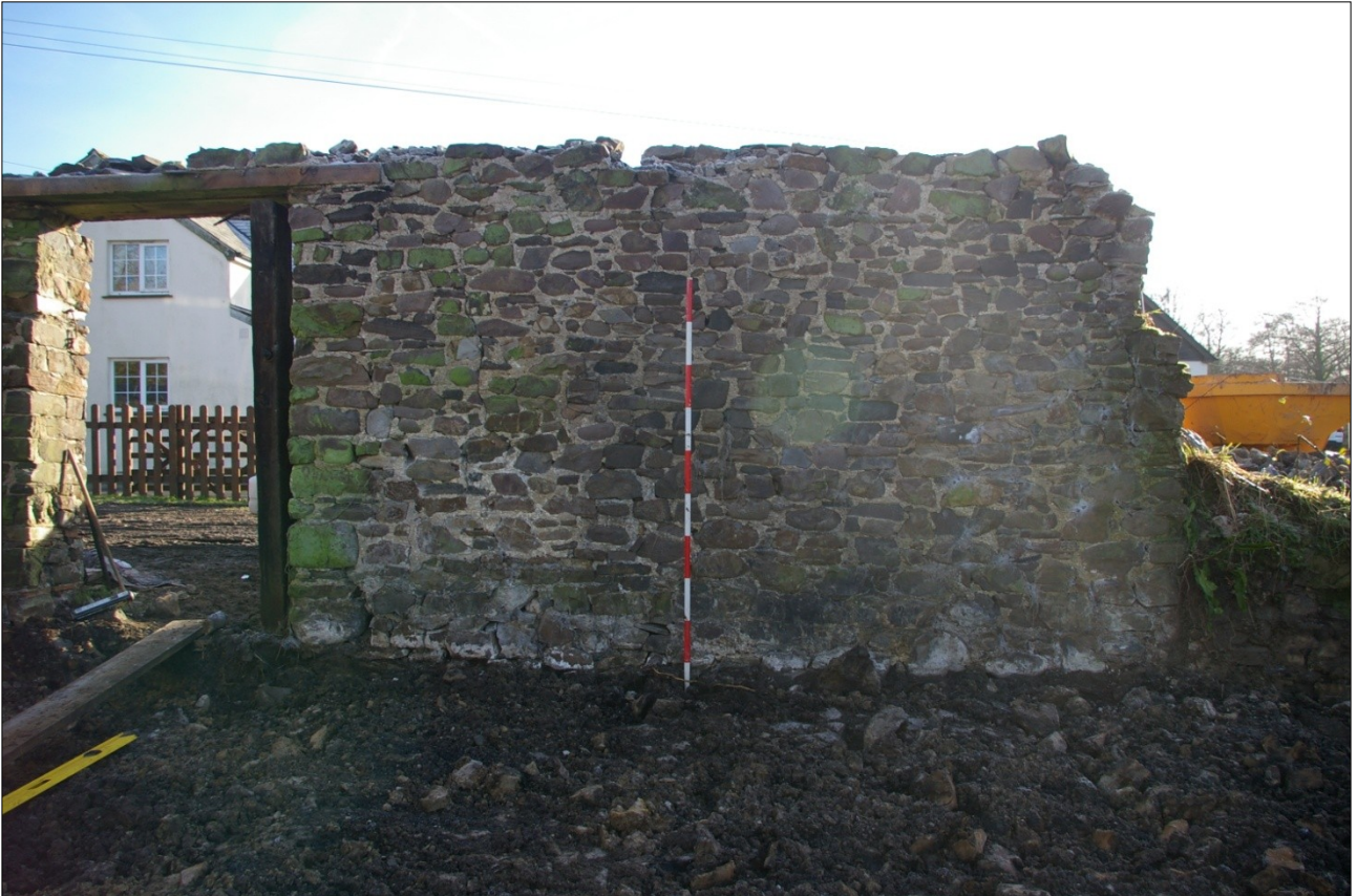
The south wall at the west end; from the north (scale 2m).
