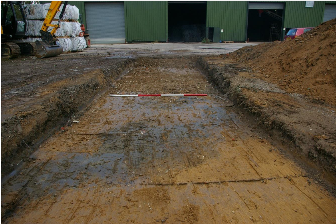
FIGURE 3: ROAD ACCESS TRENCH 01 SHOWING MADE-GROUND RUBBLE DEPOSITS; VIEWED FROM THE SOUTH (2M SCALE).
